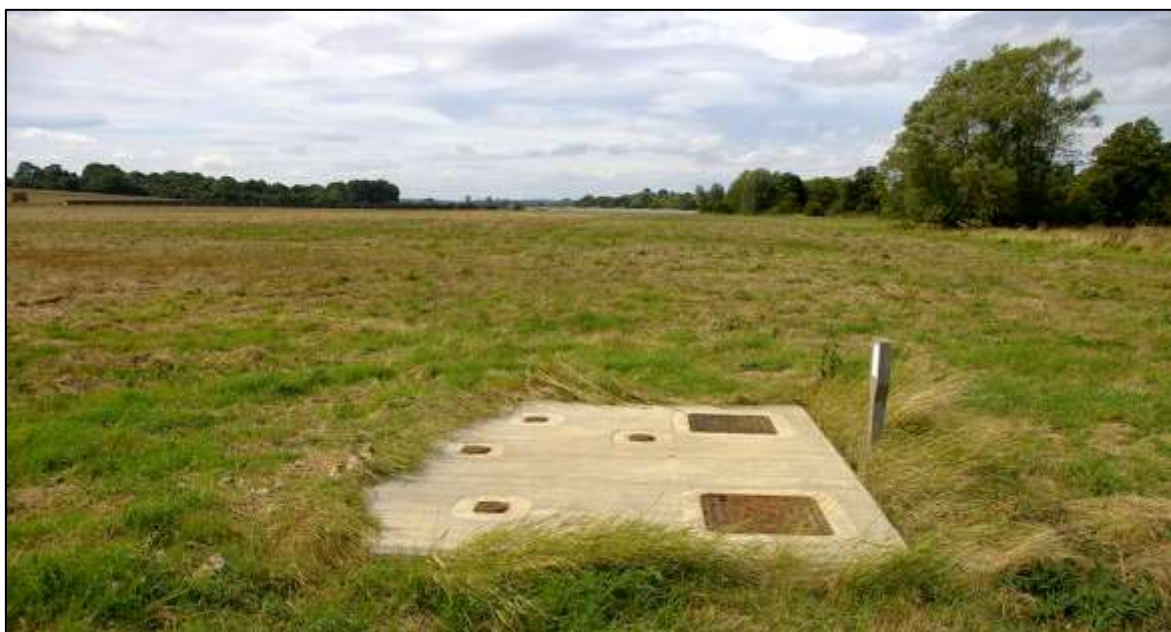
FIGURE 21: THE ACCESS TO THE PUMPING MAIN THAT RUNS ACROSS THE SITE (NORTH-EAST CORNER OF FIELD A); VIEWED FROM THE EAST.
