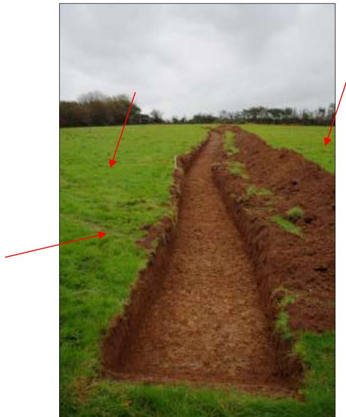
FIGURE 7: TRENCH 3, POST-EXCAVATION; VIEWED FROM THE NORTH WEST (1M SCALE). THE ARROWS MARK PATHS USED BY WALKERS.
