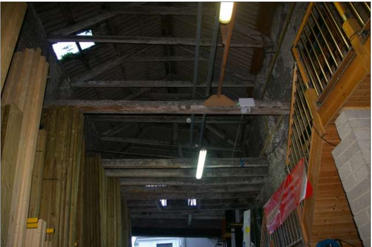
102. B2 INTERIOR, SHOWING THE SF JOISTS AND ROOF STRUCTURE; VIEWED FROM THE NORTH.
