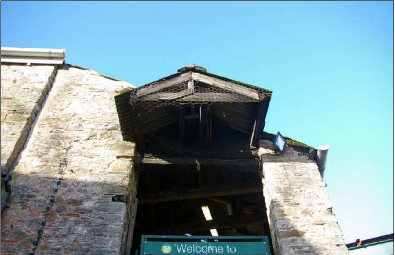
141. THE SOUTH ELEVATION OF B3, WITH FF LOADING DOOR D19 WITH PENTICE AND FLYWHEEL (S23) ABOVE; VIEWED FROM THE SOUTH.
