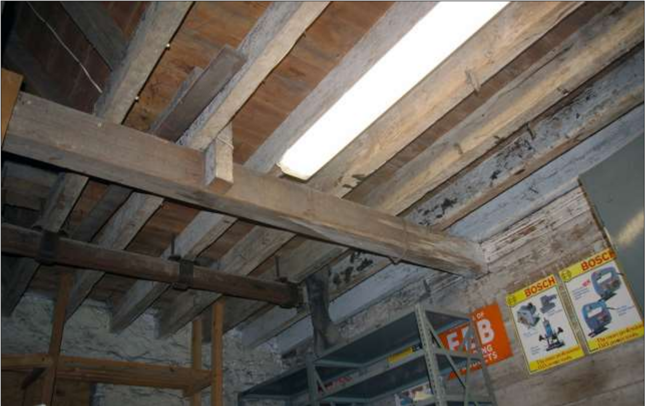
63. B1 FF R1, DETAIL OF THE JOISTS SUPPORTING THE HOPPER ABOVE; VIEWED FROM THE NORTH-EAST.
