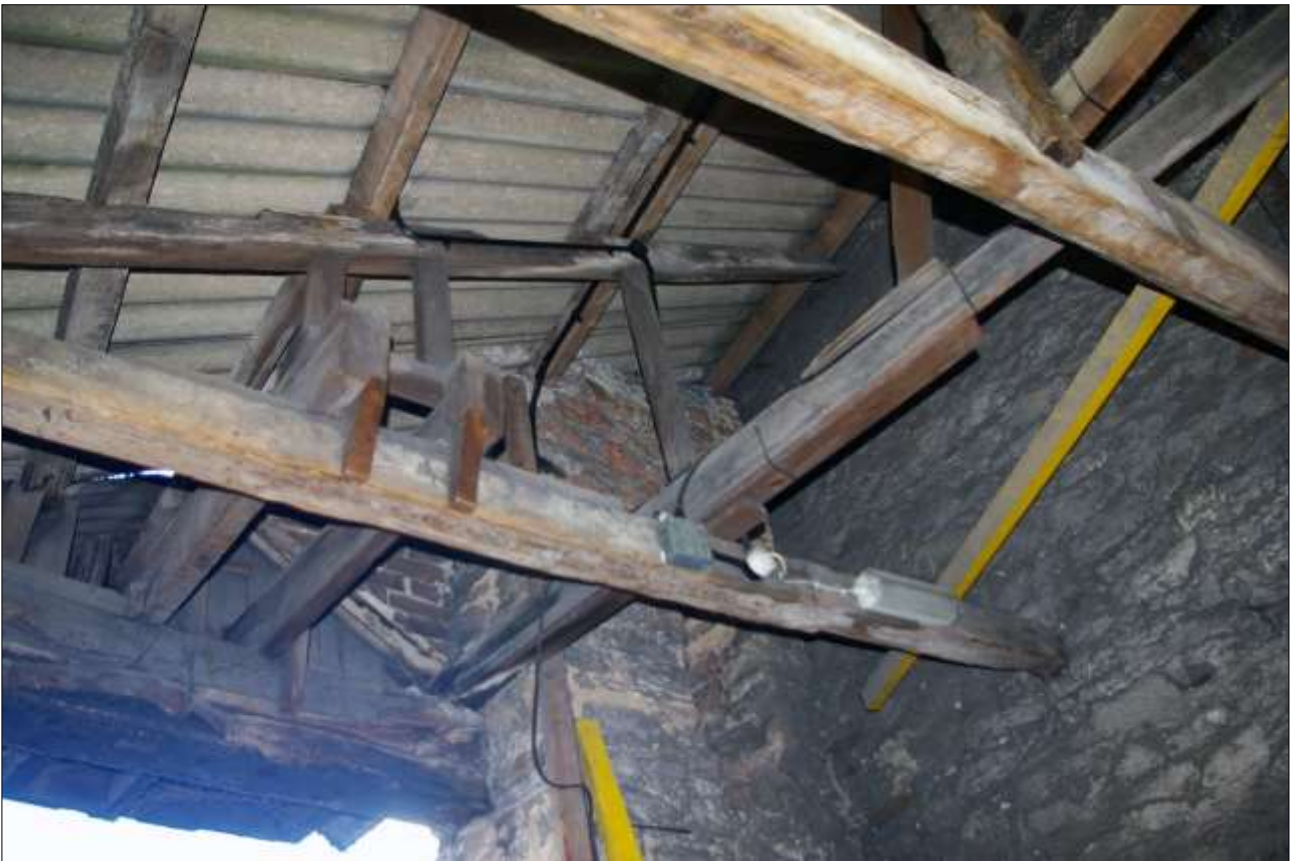
173. B3 FF INTERIOR, THE ROOF STRUCTURE OVER THE SOUTHERN END AND BEAMS FOR HOIST (S23); VIEWED FROM THE NNE.
