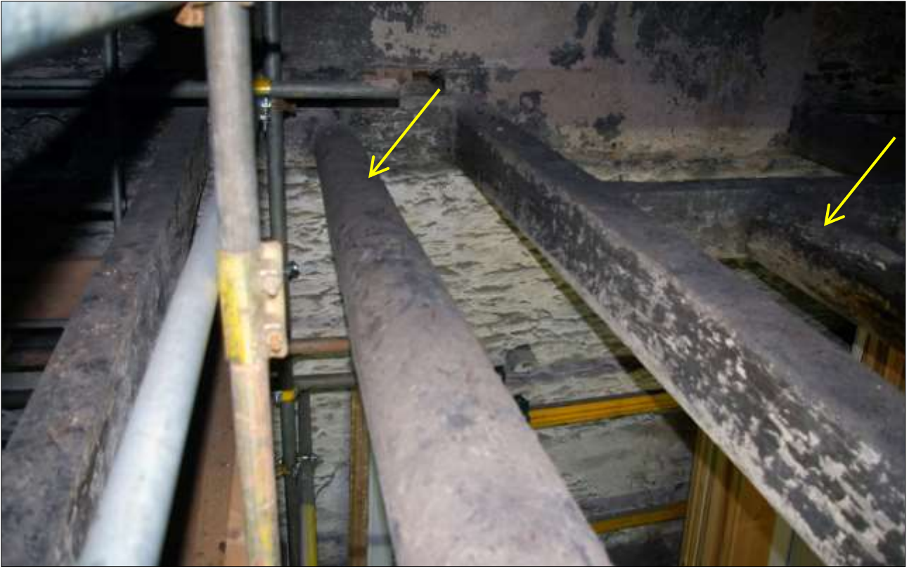
127. B2 SF INTERIOR, SHOWING THE BEAMS AND RE-USED SHIPS TIMBERS S22 (INDICATED); VIEWED FROM THE WEST.
