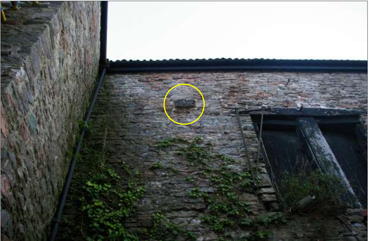
5. THE NORTH WALL OF B1, SHOWING THE SHEERLEGS AND THE PROJECTING STUB OF THE DRAGON TIE S11 (INDICATED); VIEWED FROM THE NORTH.
