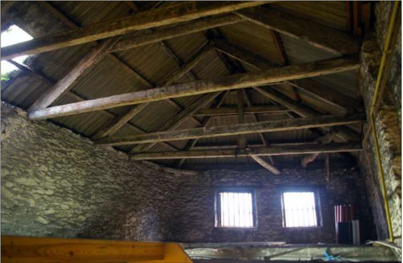
121. B2 SF INTERIOR; THE ROOF STRUCTURE OVER THE SOUTHERN END OF B2, W18 AND W19; VIEWED FROM THE NNW.
