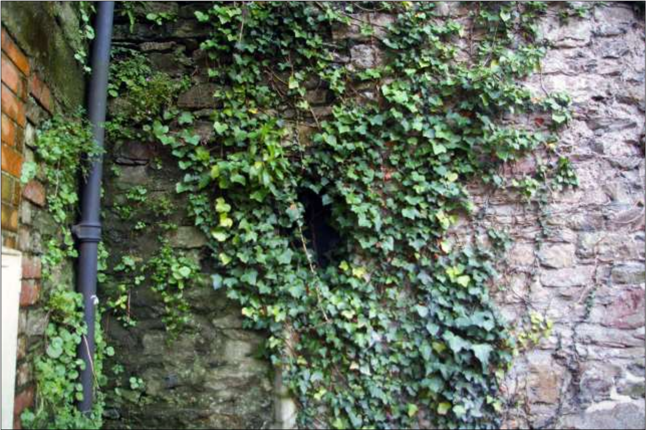
9. THE NORTH WALL OF B1, SHOWING GF WINDOW W8; VIEWED FROM THE NORTH.
