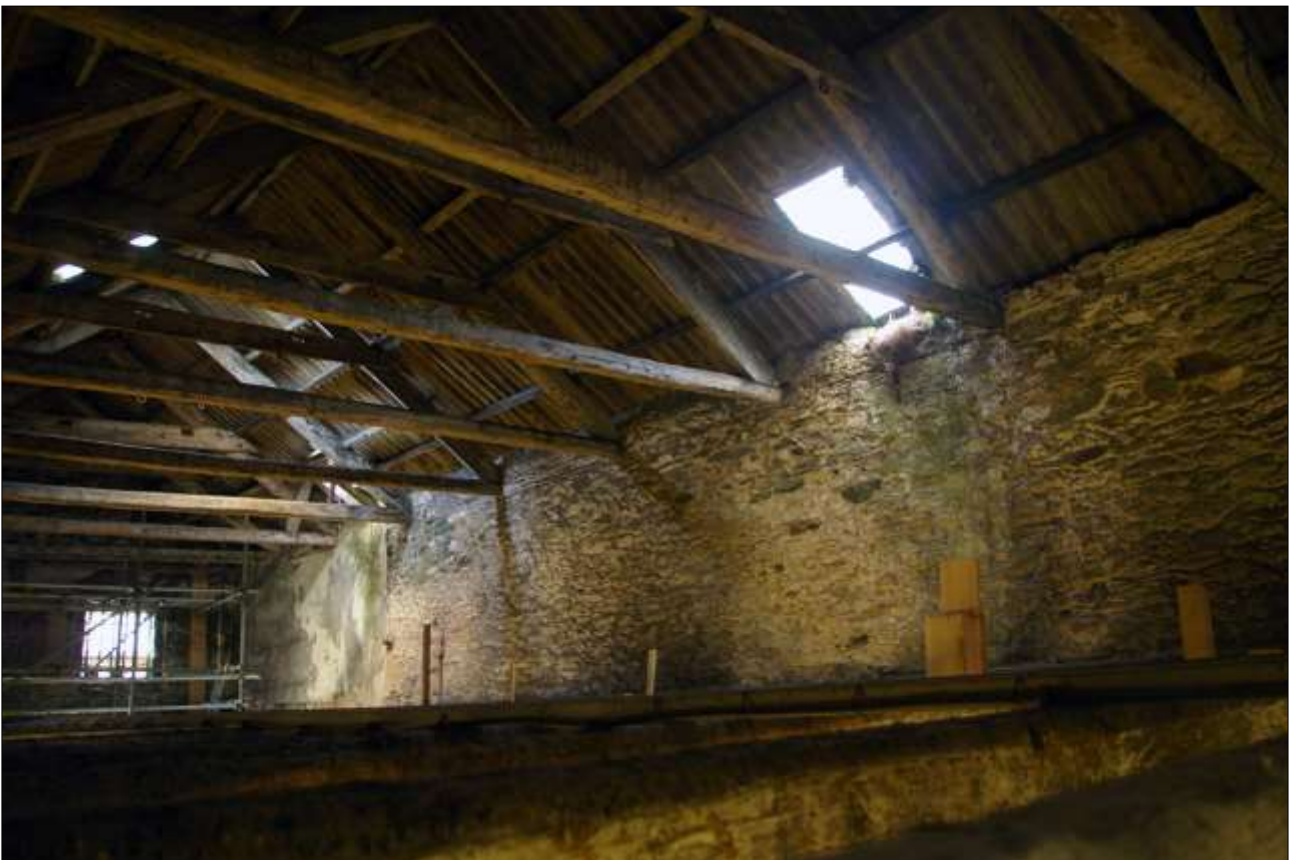
124. AS ABOVE, WITH DETAIL OF THE EAST WALL OF B2; VIEWED FROM THE SOUTH-WEST.
