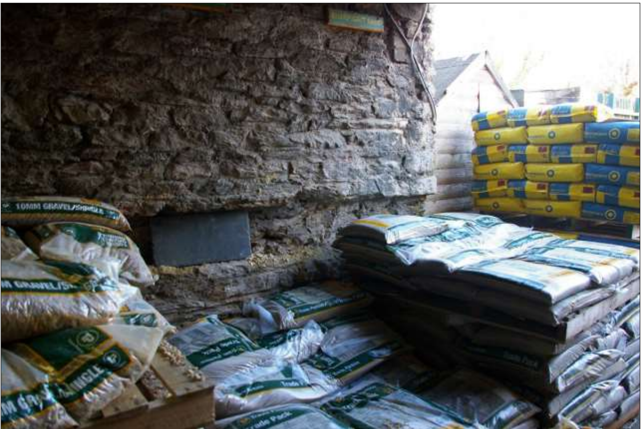
148. B3 GF INTERIOR, DETAIL OF A GROOVE IN THE STONWORK IN THE EAST WALL TO D13; VIEWED FROM THE WNW.
