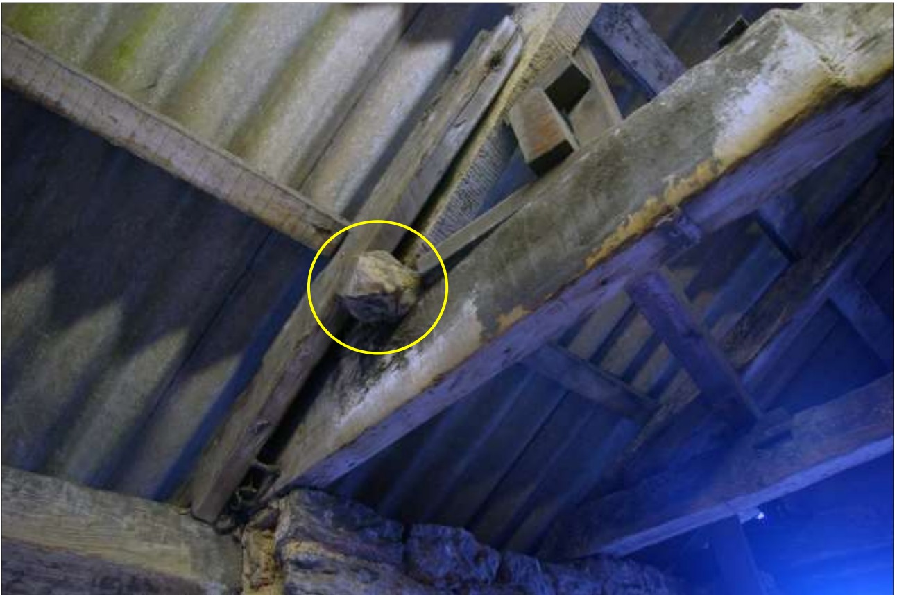
175. B3 ROOF STRUCTURE, SHOWING THE RE-USED SHAPED TIMBER (INDICATED) (S12); VIEWED FROM THE NNW.
