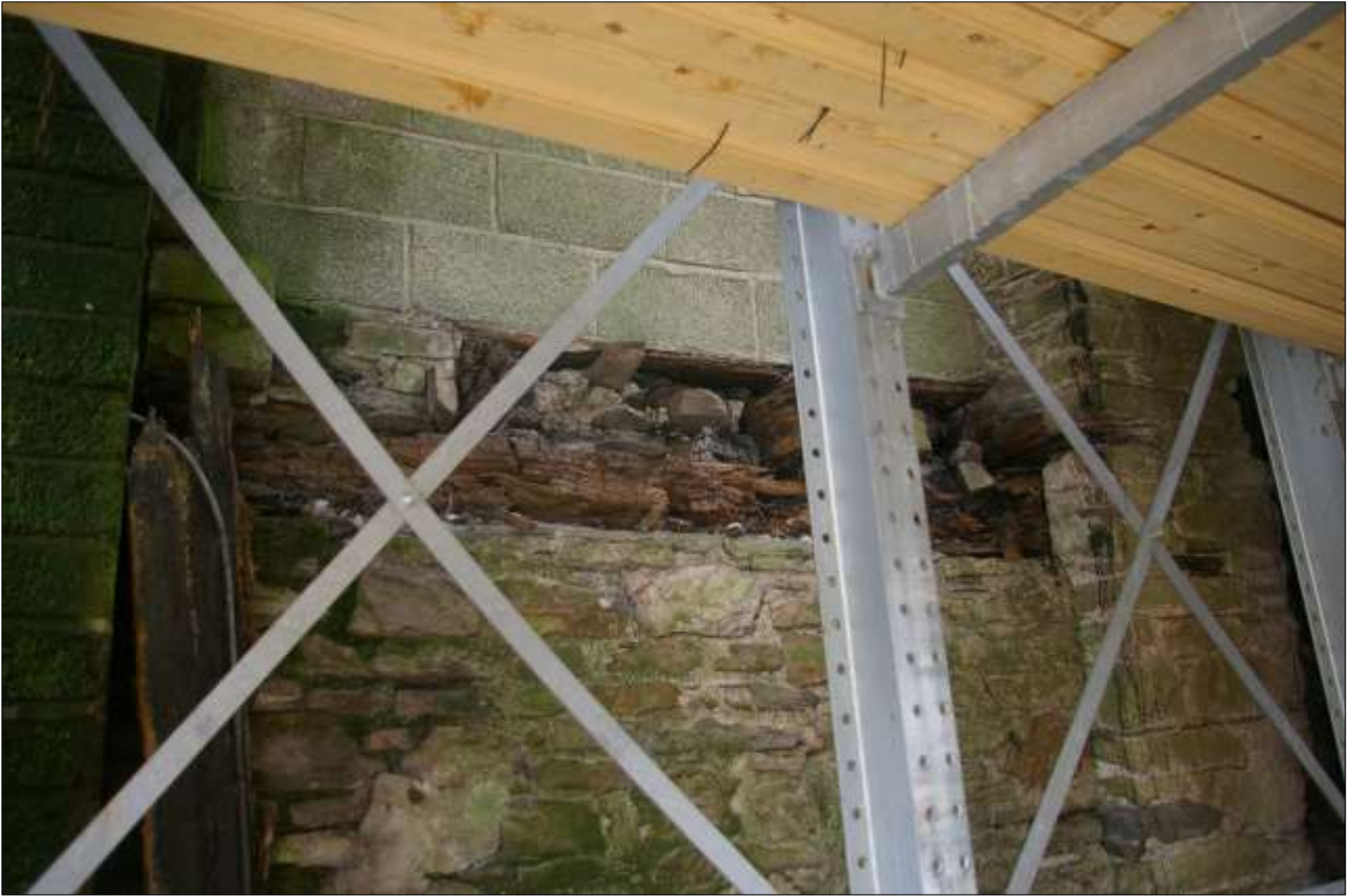
145. THE EAST ELEVATION OF B3, DETAIL OF THE DECAYED TIMBERWORK; VIEWED FROM THE SOUTH-EAST.
