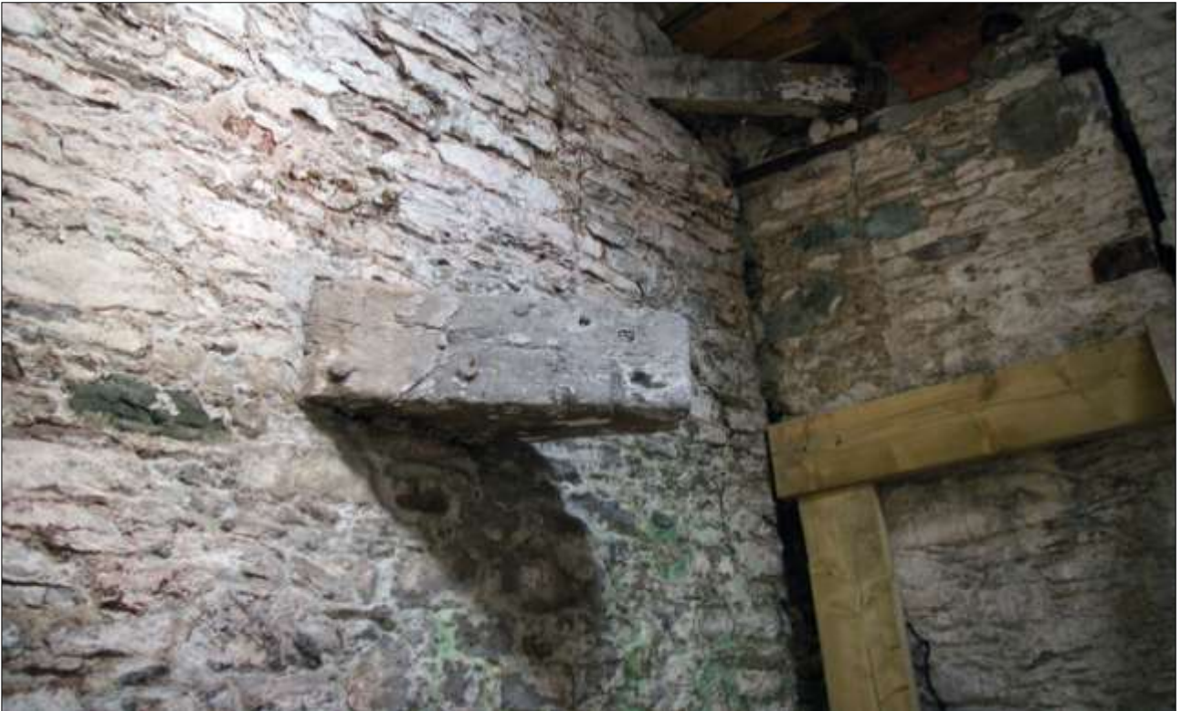
78. B1 FF R2, DETAIL OF THE DRAGON TIE (S11); VIEWED FROM THE WEST.
