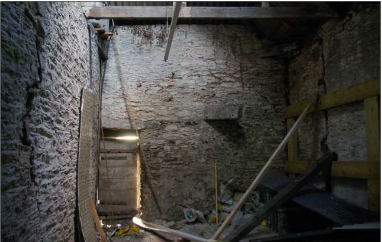
75. B1 FF R2, SHOWING D22 AND TRUNCATED DRAGON TIE (S11); VIEWED FROM THE SOUTH.
