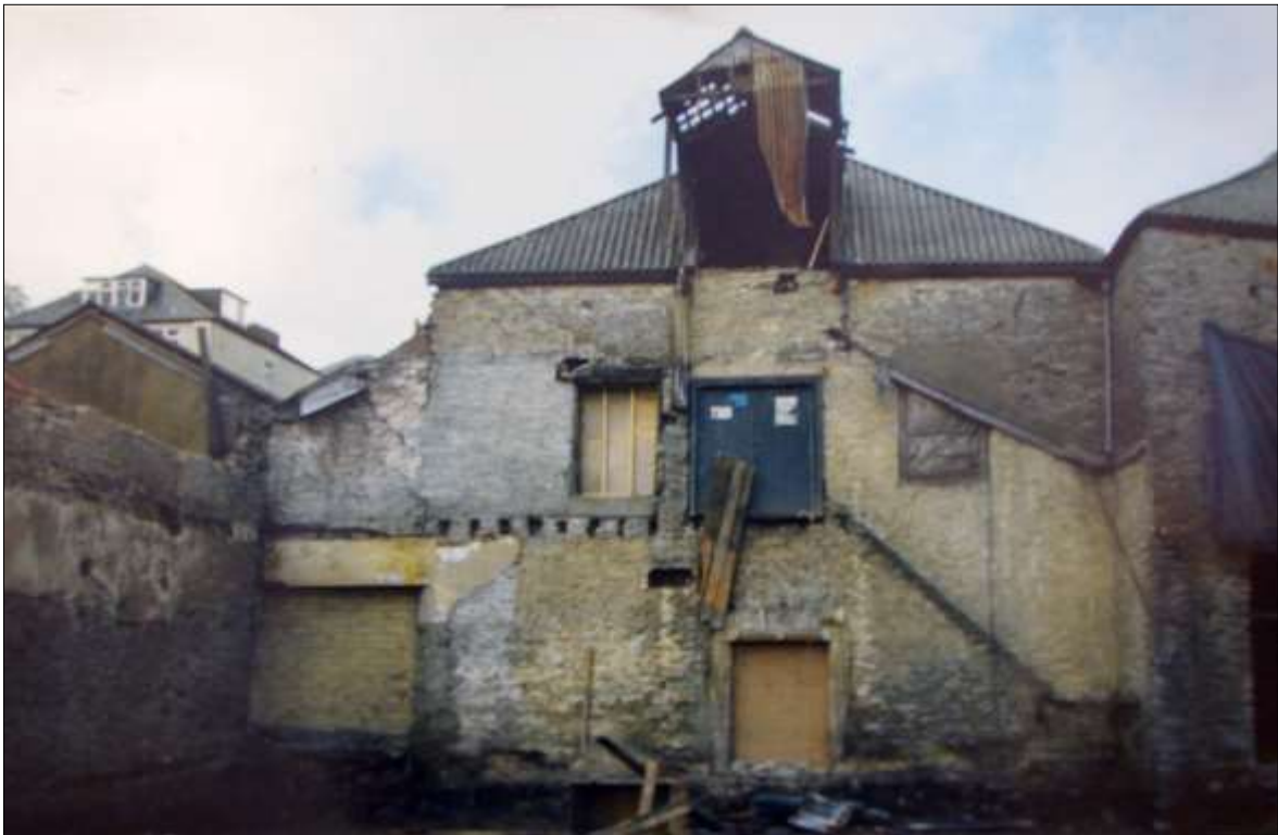
FIGURE 12: THE SOUTH ELEVATION OF BUILDING 1 FOLLOWING THE DEMOLITION OF THE 19 TH CENTURY STRUCTURE IN FIGURE 9; VIEWED FROM THE SOUTH (PRIVATE COLLECTION).
