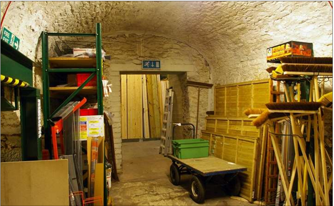
40. B1 GF, THE NORTHERN HALF OF V3 SHOWING FORCED DOORWAY D5; VIEWED FROM THE WEST.
