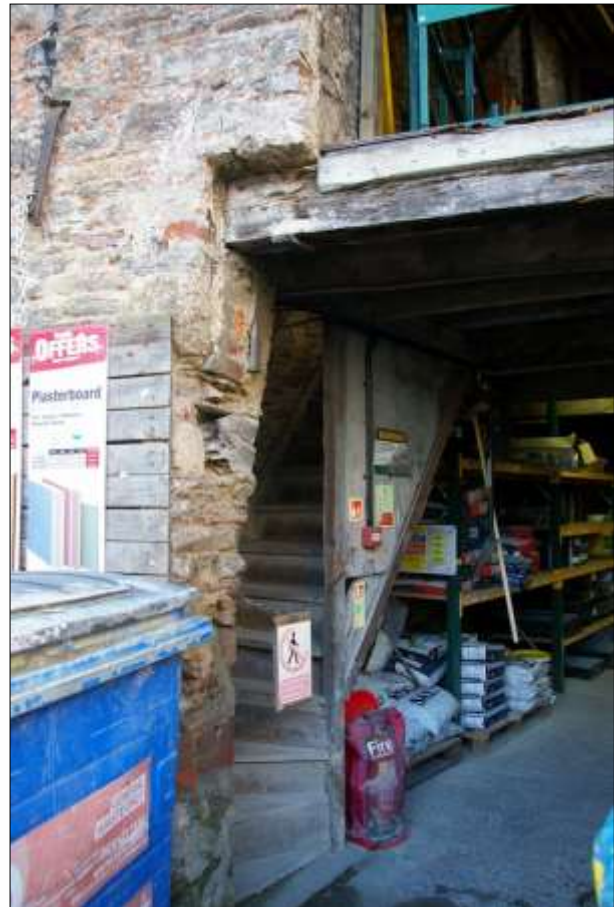
140. RIGHT: THE SOUTH ELEVATION OF B3 SHOWING THE WIDENED DOORWAY D13 WITH STAIRS (S3) BEHIND; VIEWED FROM THE SSE.
