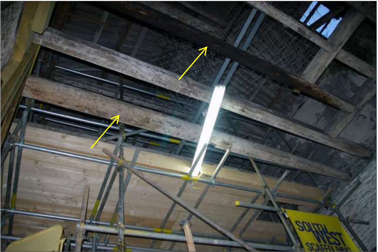
115. B2 FF INTERIOR, SHOWING THE SF BEAMS AND RE-USED SHIPS TIMBERS S22 (INDICATED); VIEWED FROM THE SSW.
