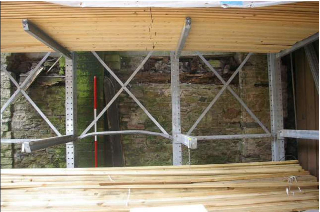
144. THE EAST ELEVATION OF B3, DETAIL OF THE BLOCKED OPENING AND DECAYED TIMBERWORK; VIEWED FROM THE EAST (SCALE 2M).
