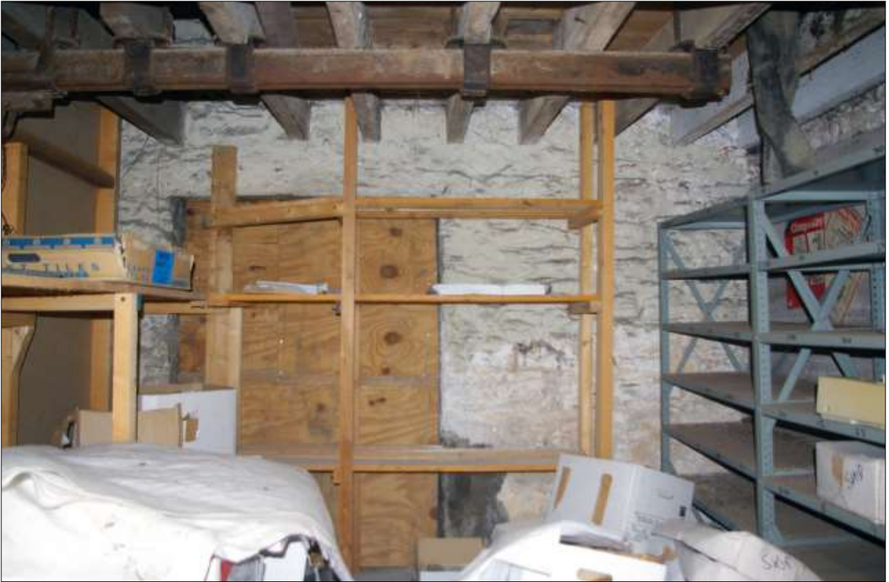
61. B1 FF R1A, VIEW OF BOARDED WINDOW W10, WITH RAIL FOR BAG HOIST AND LEATHER SLEEVE (RIGHT) ABOVE; VIEWED FROM THE NORTH.
