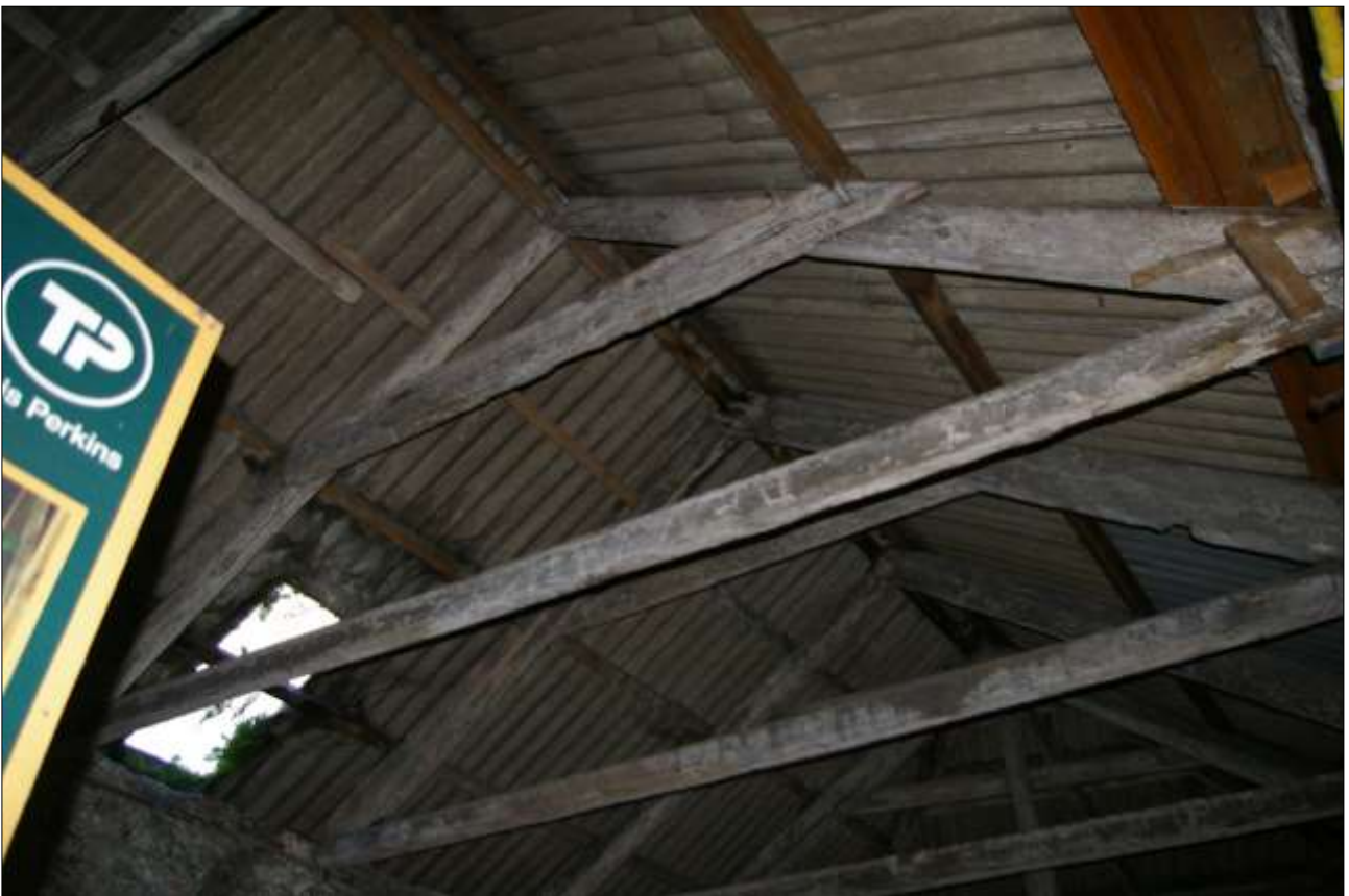
133. AS ABOVE, THE SOUTHERN HALF OF THE ROOF; VIEWED FROM THE NNW.
