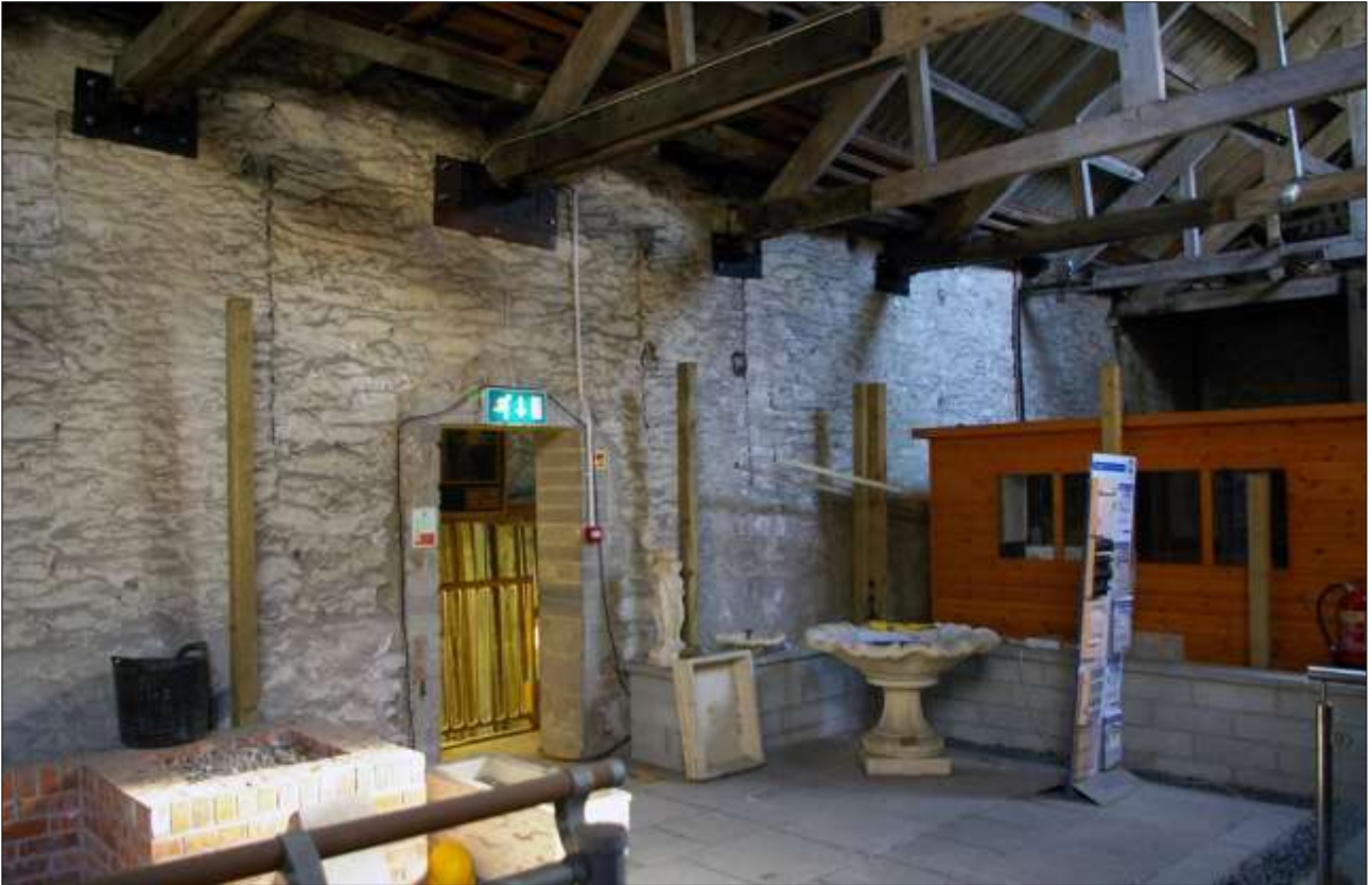
45. AS ABOVE, SHOWING THE STEEL REINFORCED TIE BEAMS ABOVE; VIEWED FROM THE NORTH-WEST.
