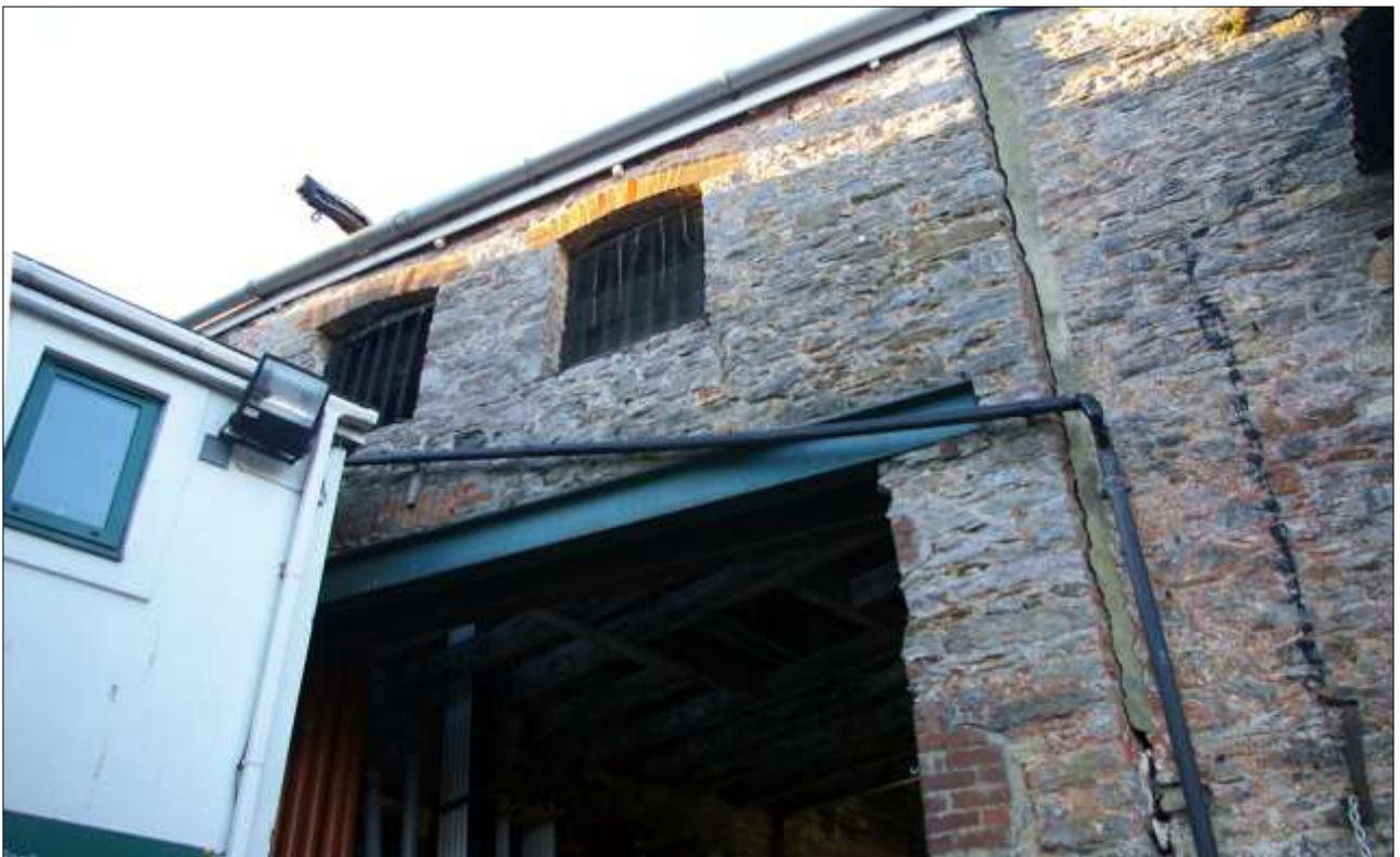
94. THE SOUTH ELEVATION OF B2, WITH LARGE FORCED GF OPENING D12 WITH W18 AND W19 ABOVE; VIEWED FROM THE SSE.
