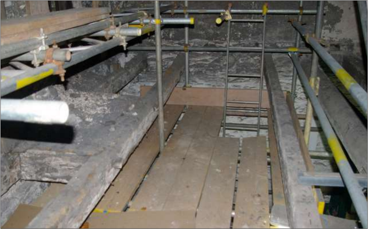
125. B2 SF INTERIOR, DETAIL OF THE BEAMS AT THE SOUTHERN END OF B2; VIEWED FROM THE WEST.
