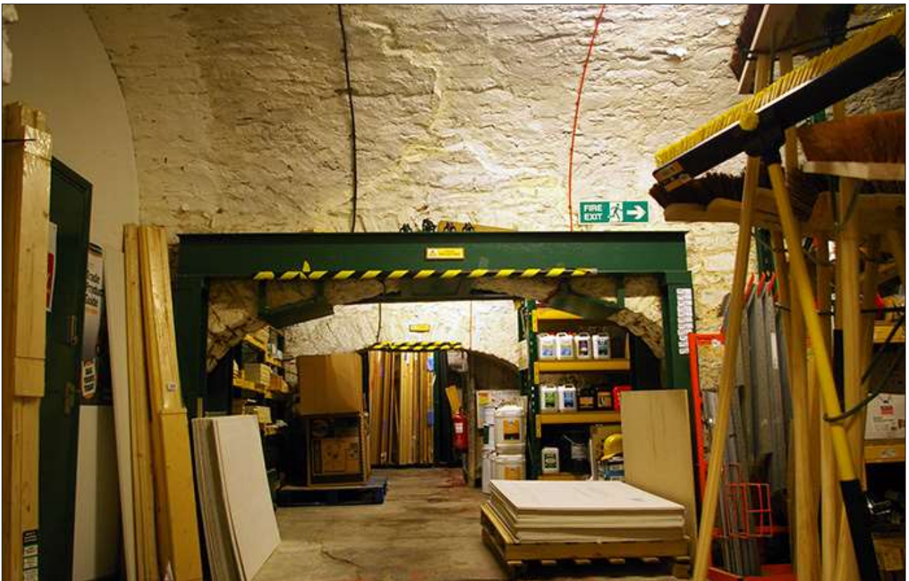
39. B1 GF, LOOKING THROUGH STEEL REINFORCED D4 FROM V3 INTO V4; VIEWED FROM THE SOUTH.
