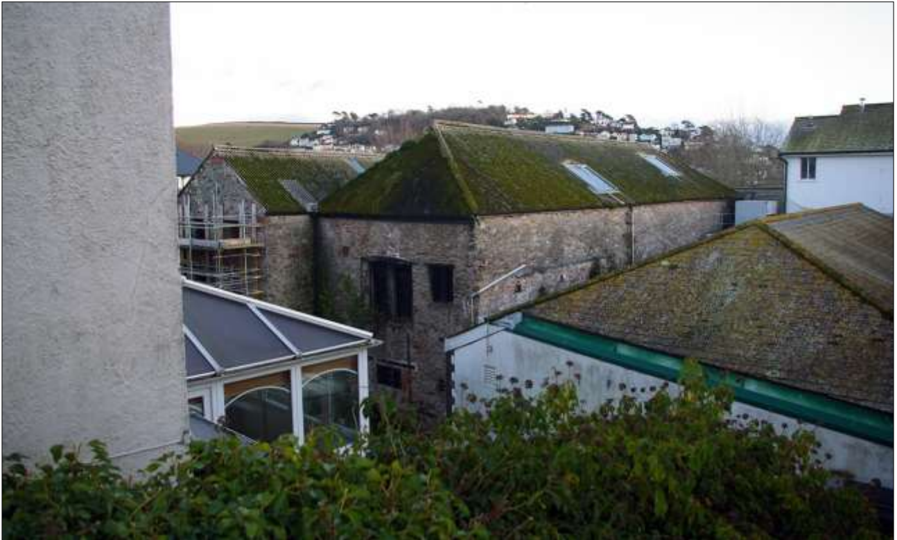
1. THE NORTH AND WEST WALLS OF BUILDING 1 (B1), VIEWED FROM THE NORTH-WEST.
