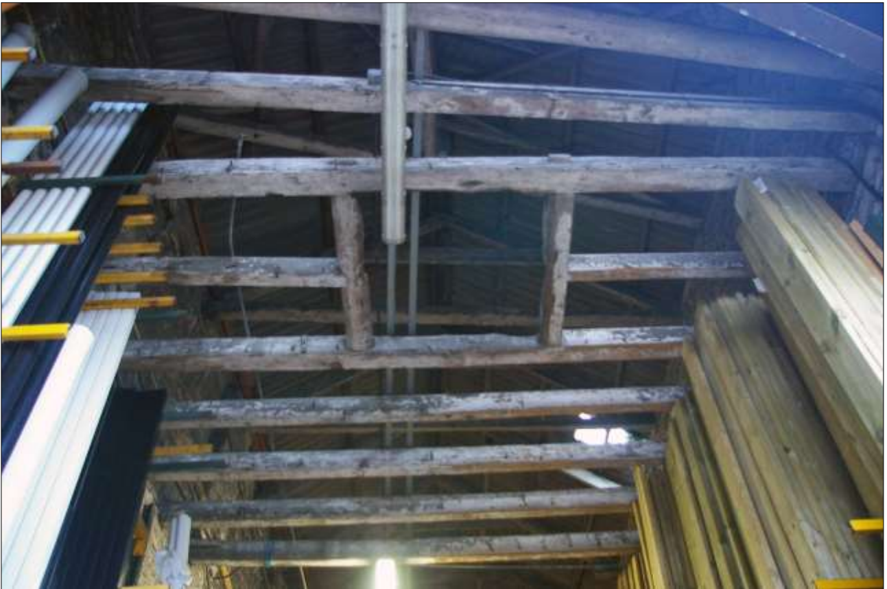
B2 INTERIOR, DETAIL OF THE SF BEAMS WITH HATCH OPENING (S20); VIEWED FROM THE SOUTH.
