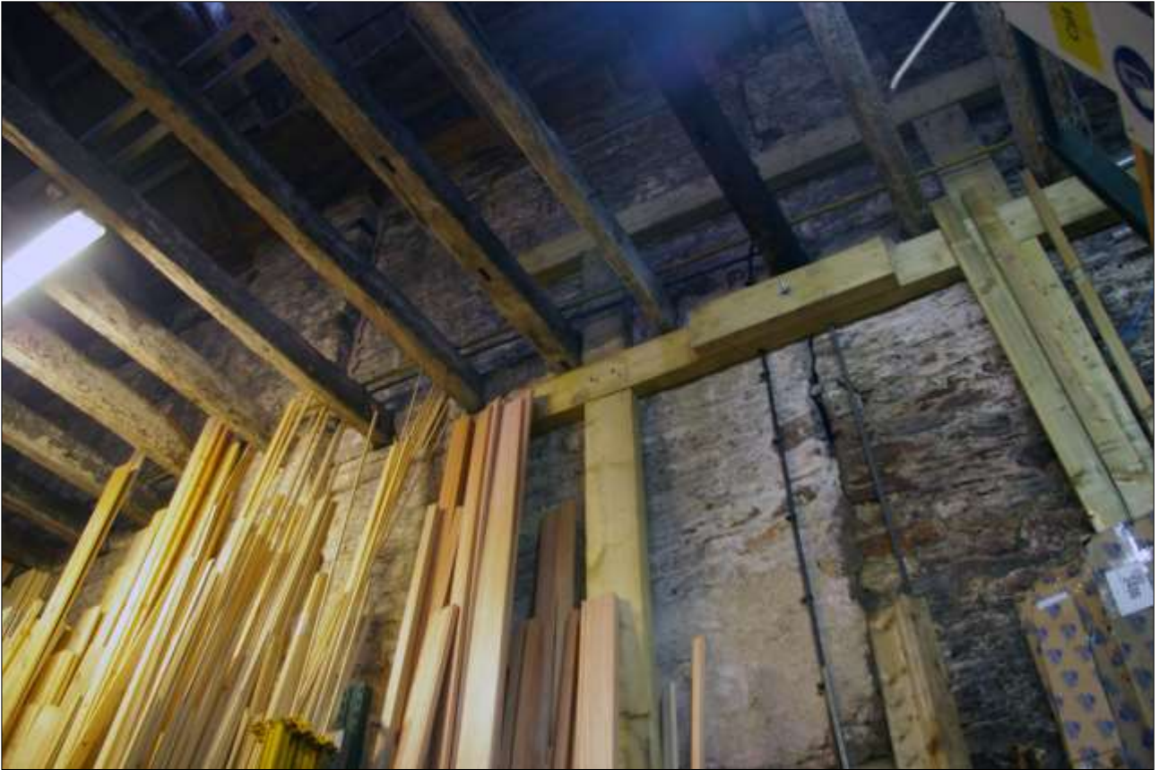
13. THE NORTHERN PART OF THE EAST WALL OF B1; VIEWED FROM THE ENE.
