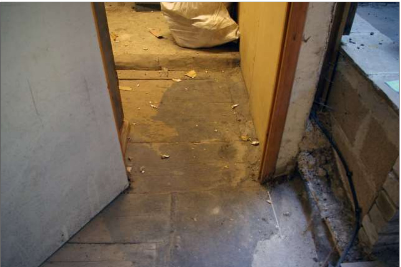
60. B1 FF R1A, VIEW THROUGH D17 INTO R1A SHOWING THE HISTORIC FLOORBOARDS (S5); VIEWED FROM THE EAST.
