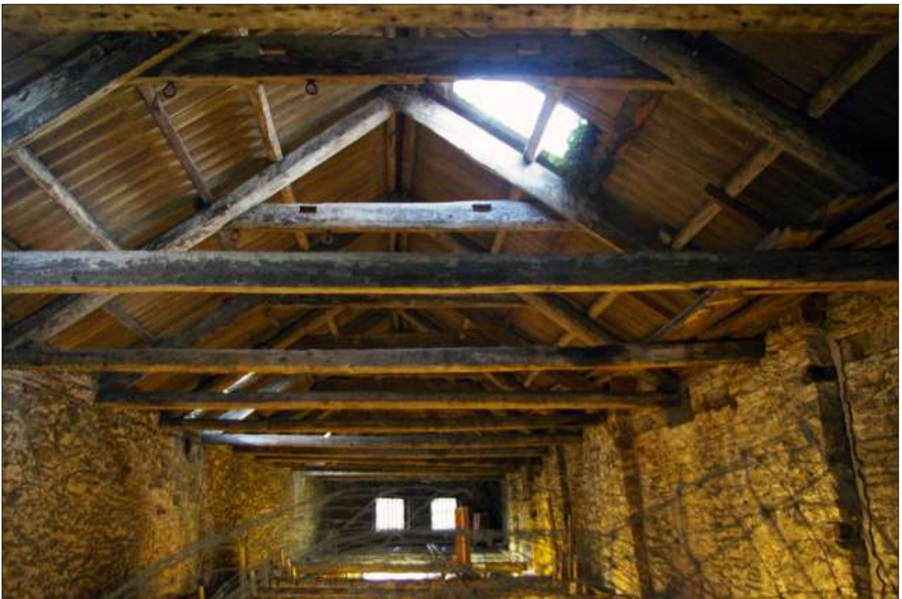
131. B2 SF INTERIOR, DETAIL OF THE ROOF STRUCTURE; VIEWED FROM THE NORTH.
