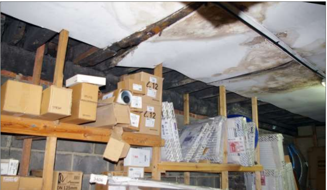
162. B3 GF INTERIOR, THE NORTHERN END, SHOWING MODERN BLOCKING TO THE EAST; VIEWED FROM THE WNW.
