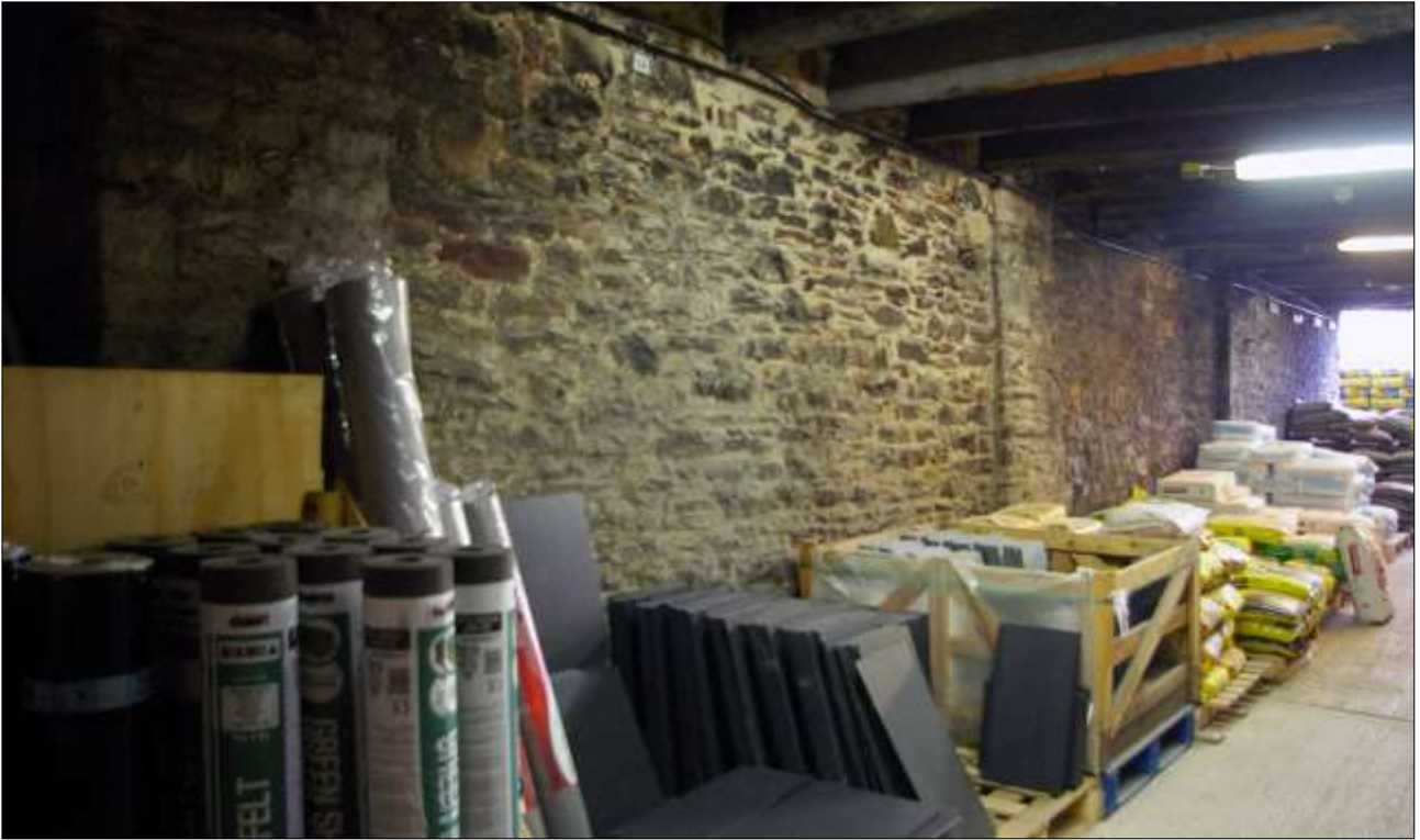
151. B3 GF INTERIOR, THE EAST WALL OF B3; VIEWED FROM THE NNW.
