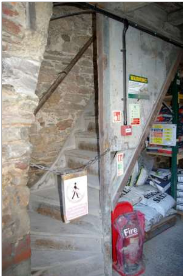
150. B3 GF INTERIOR, THE STAIRS (S3) TO THE FIRST FLOOR; VIEWED FROM THE SOUTH-EAST.
