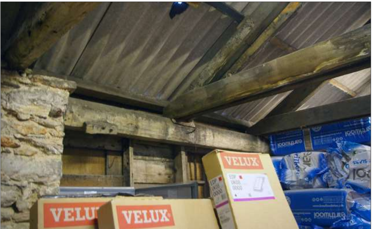
186. B3 FF INTERIOR, SHOWING ORIGINAL WOODEN FRAMEWORK TO BO17; VIEWED FROM THE WNW.
