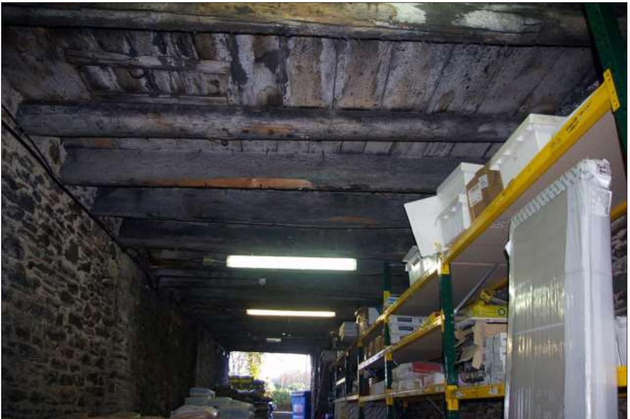
154. B3 GF INTERIOR, DETAIL OF THE MANY RE-USED BEAMS, INCLUDING SHIPS TIMBERS; VIEWED FROM THE NORTH.
