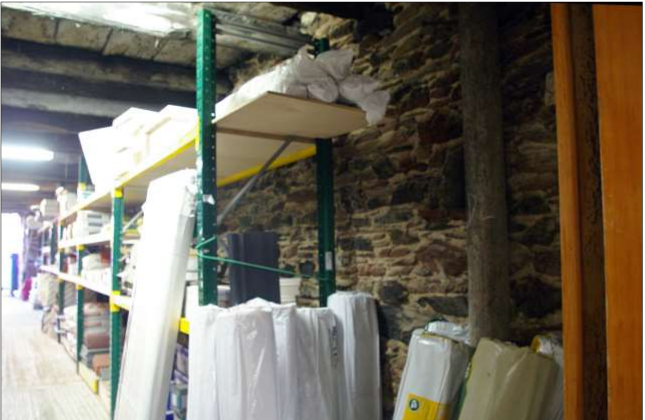
152. B3 GF INTERIOR, THE WEST WALL OF B3 (EAST WALL OF B2); VIEWED FROM THE NNE.
