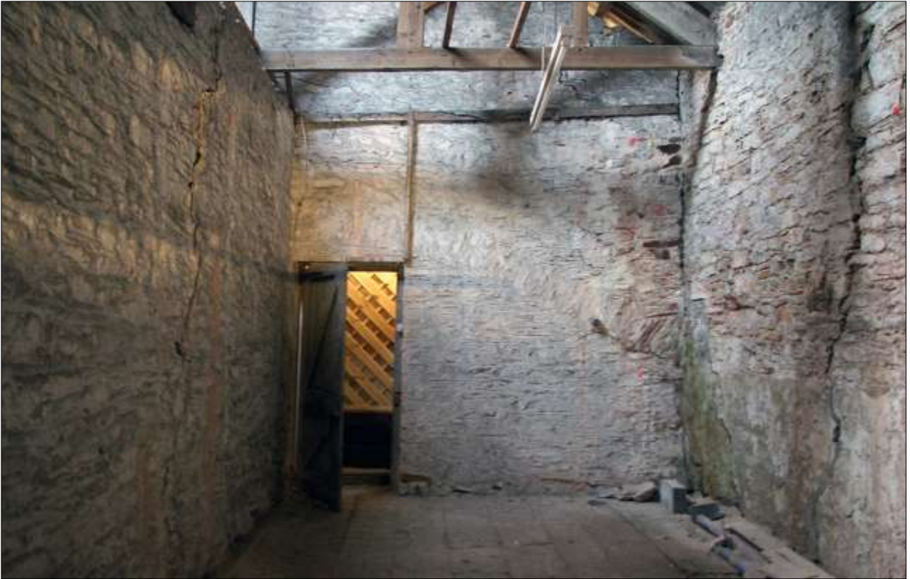
82. B1 FF R3, THE SOUTH END OF THE ROOM SHOWING D20; VIEWED FROM THE NORTH.
