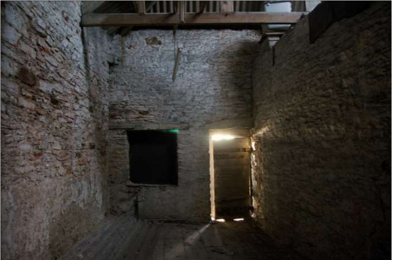
84. B1 FF R3, THE NORTH END OF R3 WITH W11 AND D21; VIEWED FROM THE SOUTH.
