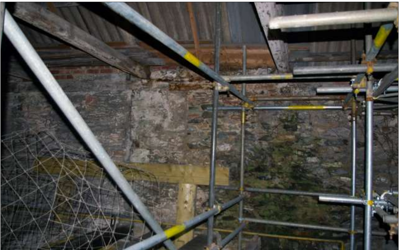
16. THE EAST WALL OF B1 AT ITS NORTHERN END AT SF LEVEL; VIEWED FROM THE WEST.
