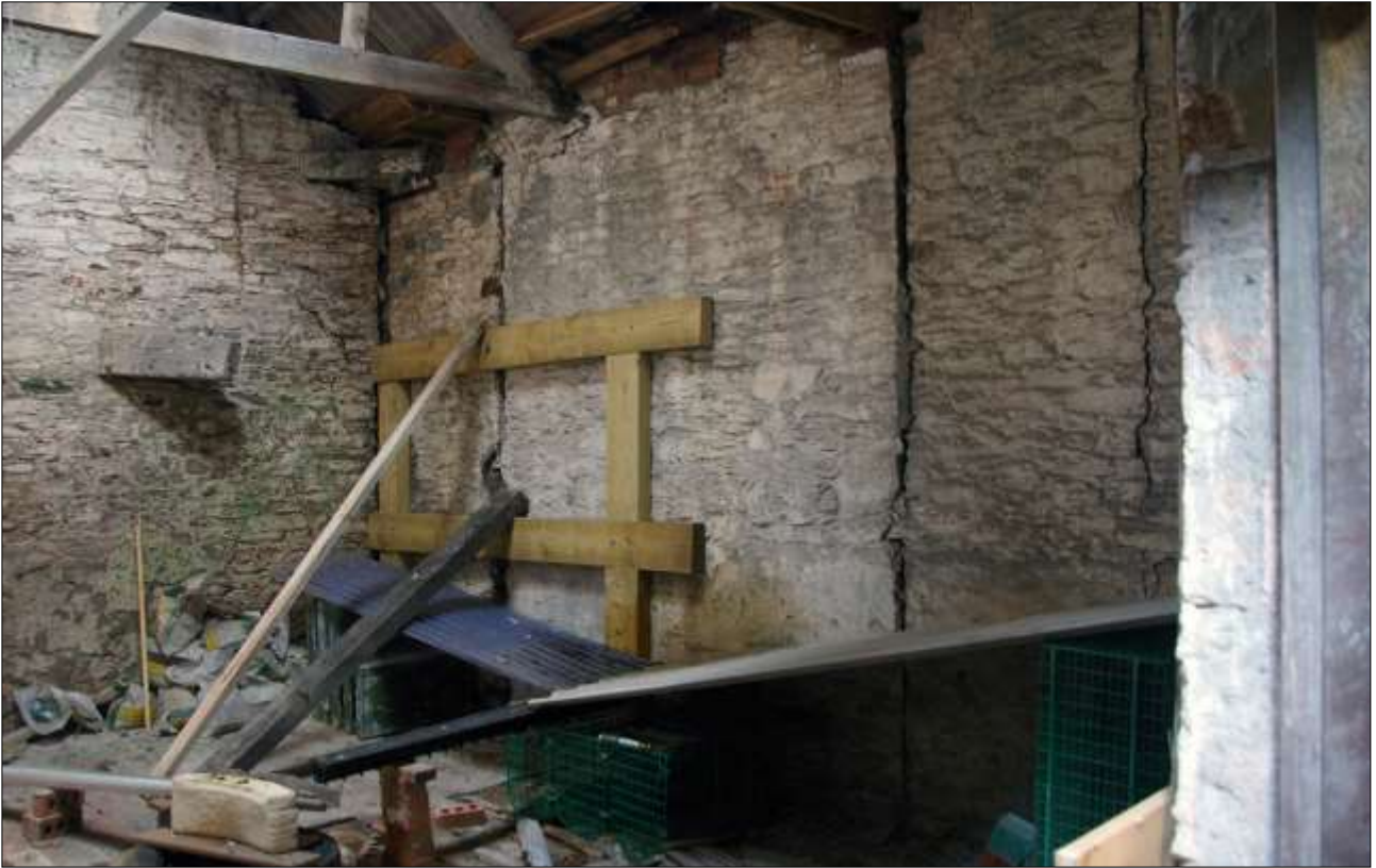
79. B1 FF R2, THE EAST WALL AND ITS BUILD LINES; VIEWED FROM THE SOUTH-EAST.
