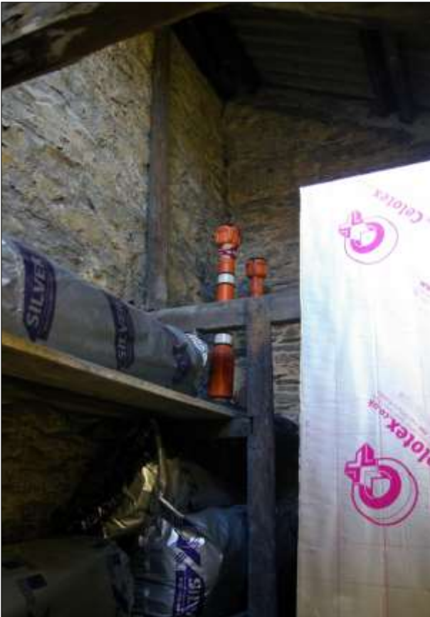
190. LEFT: B3 FF INTERIOR, THE NORTH WALL ABUTTING B2; VIEWED FROM THE SSE.
