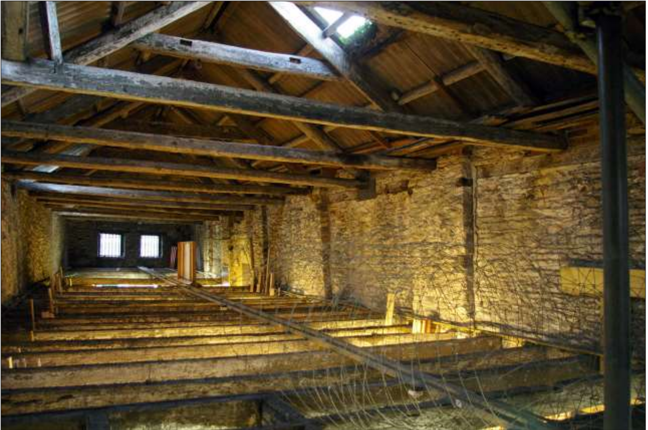
15. THE EAST WALL OF B1 AT SF LEVEL; VIEWED FROM THE NNE.
