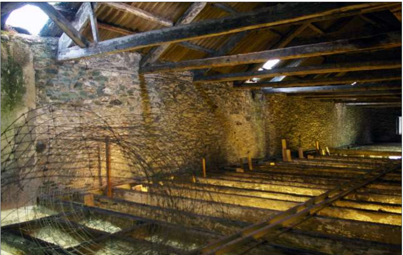
120. B2 SF INTERIOR, THE EAST WALL OF B2; VIEWED FROM THE NNW.
