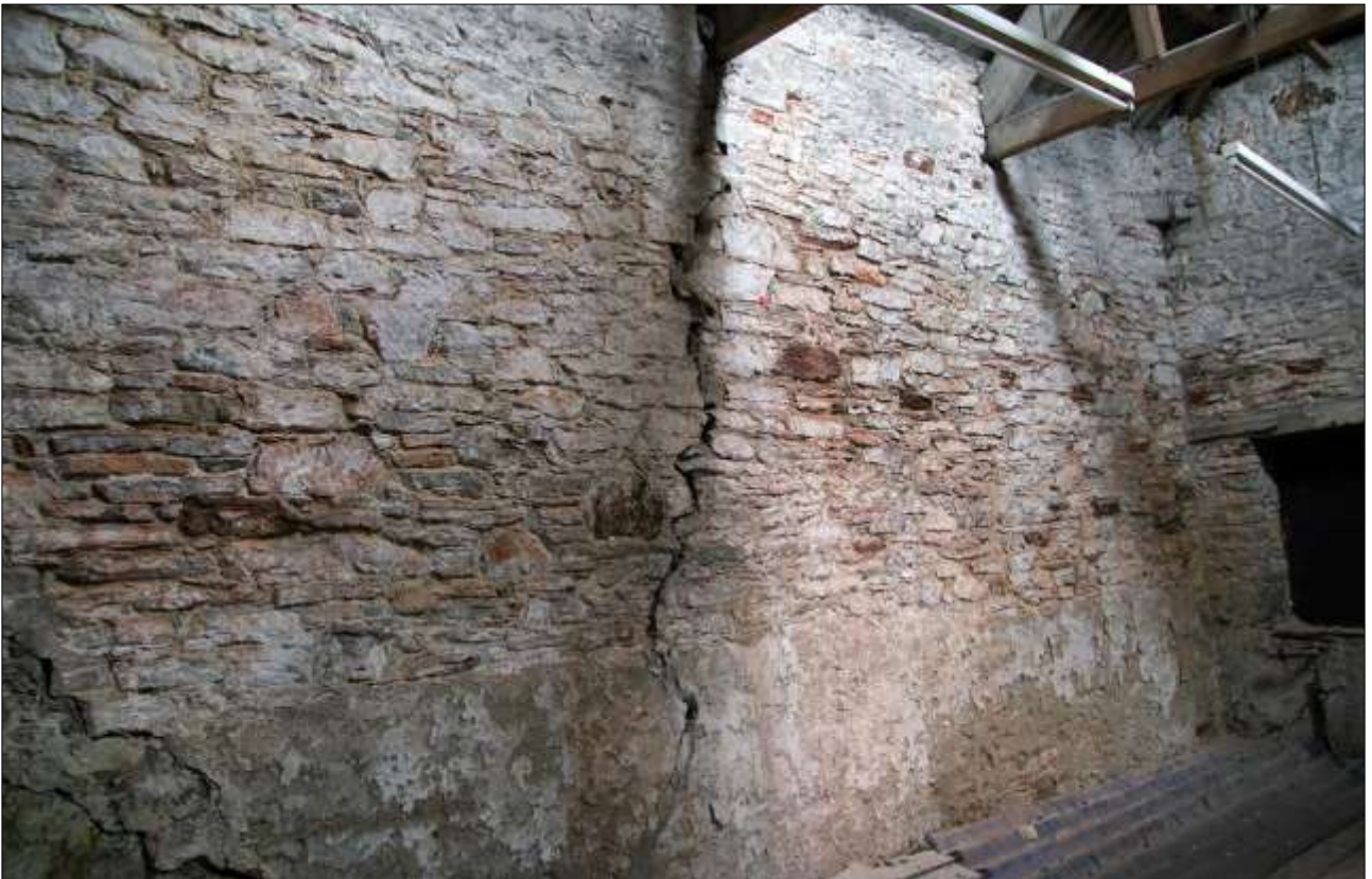
83. B1 FF R3, THE WEST WALL OF R3 SHOWING ITS STRUCTURAL CRACKS; VIEWED FROM THE SOUTH-EAST.
