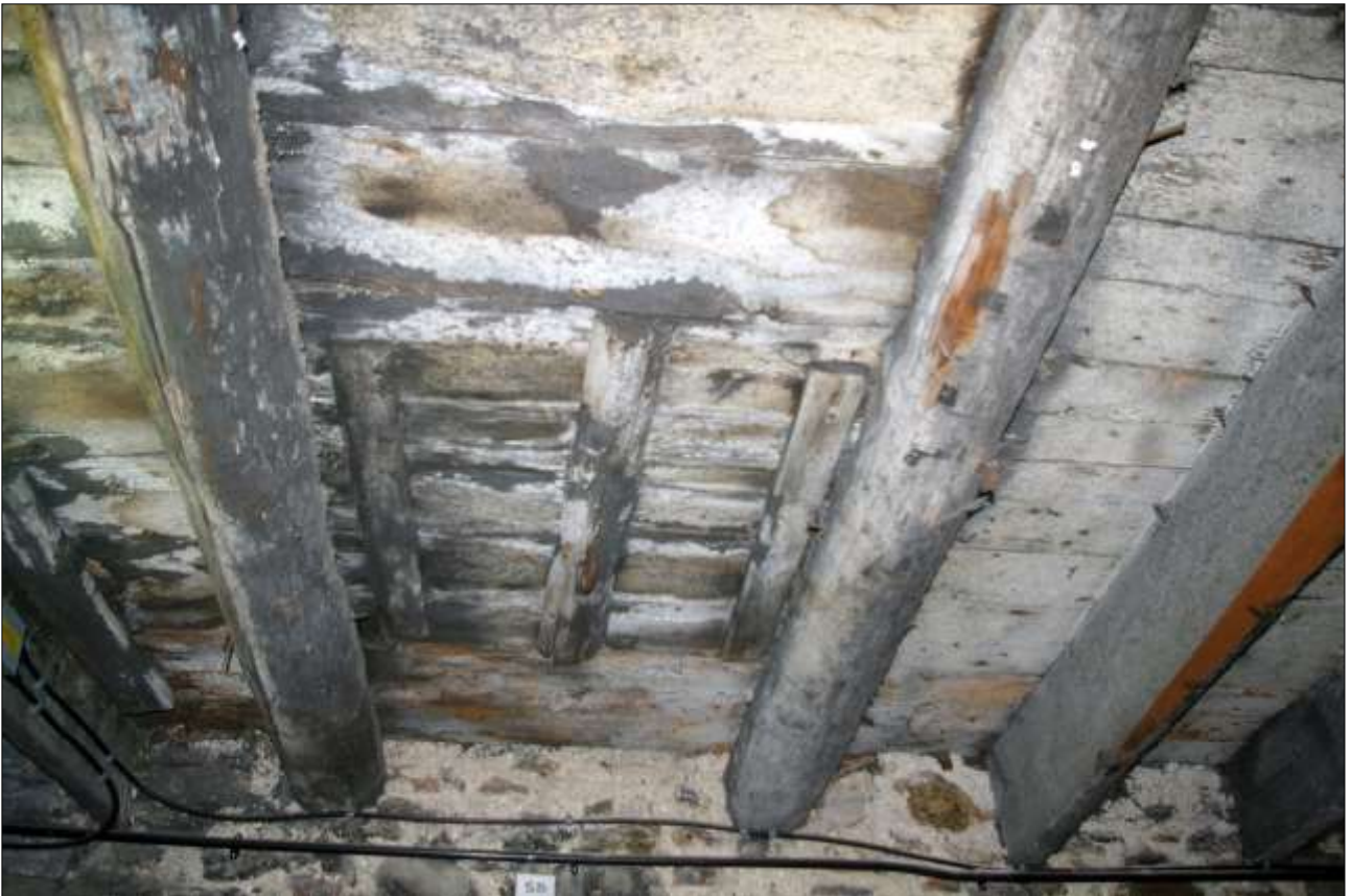
159. AS ABOVE, SHOWING A HATCH IN THE CEILING; VIEWED FROM THE WEST.
