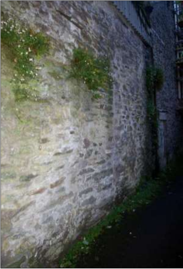
192. THE NORTH WALL OF B4, SHOWING A BLOCKED OPENING; VIEWED FROM THE ENE.
