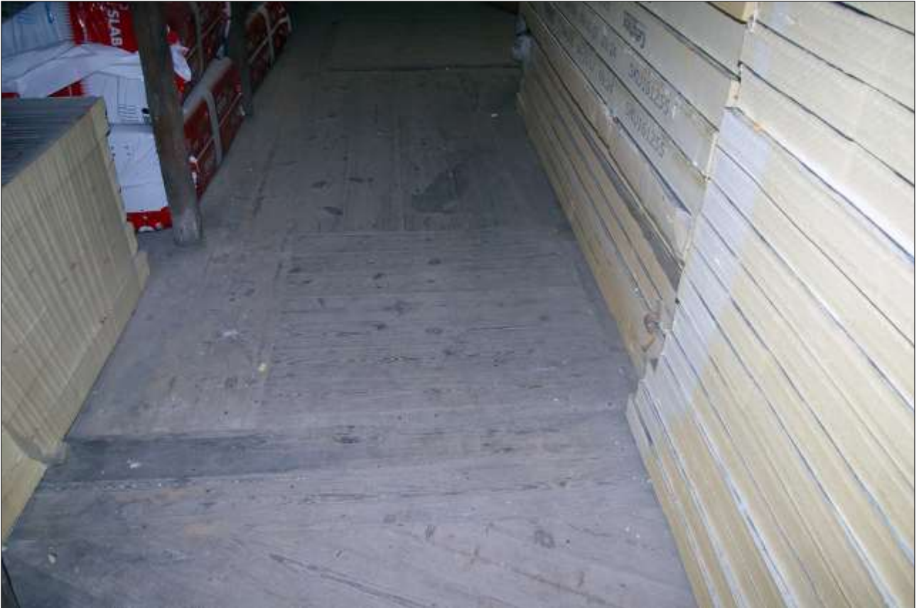
183. B3 FF INTERIOR, HISTORIC FLOORBOARDS (S13) AND HATCH (S14); VIEWED FROM THE NORTH.
