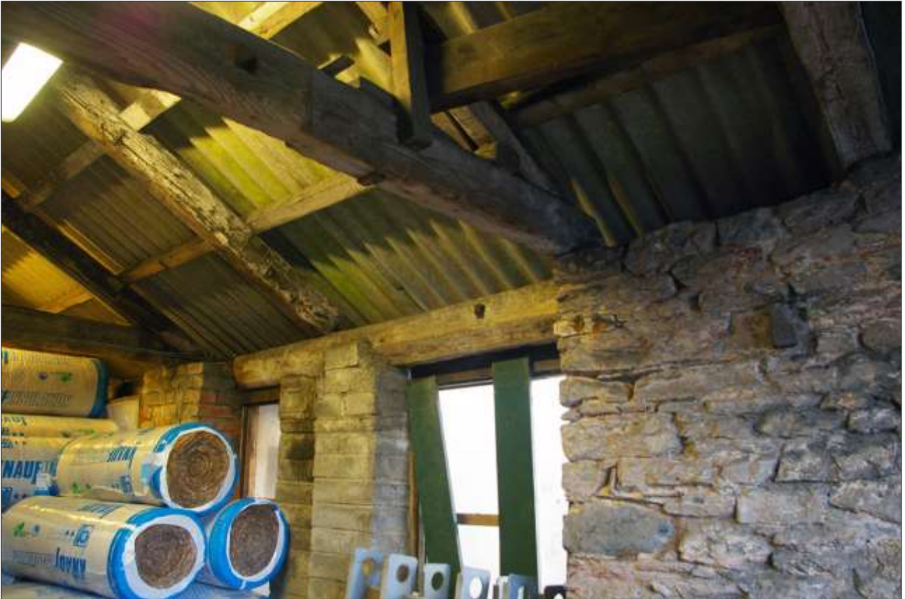
176. B3 FF INTERIOR, THE EAST WALL AND W14 AND W15 IN BO42; VIEWED FROM THE SOUTH-WEST.
