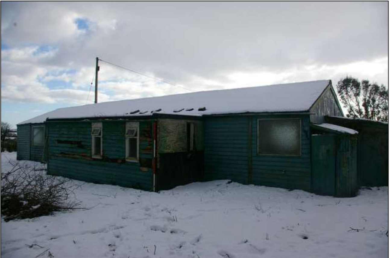
THE PORCH AND TOILET BLOCK EXTENSION ON THE NORTH SIDE OF THE MAIN BUILDING, WITH 2M SCALE; FROM THE NORTH-WEST.
