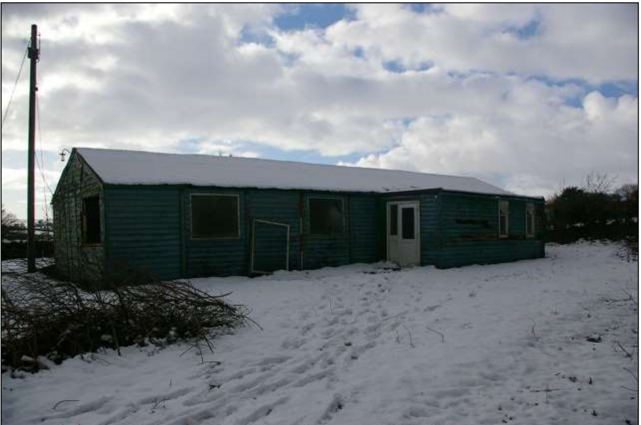
THE NORTH ELEVATION OF THE BUILDING, WITH 2M SCALE; FROM THE NORTH-EAST.
