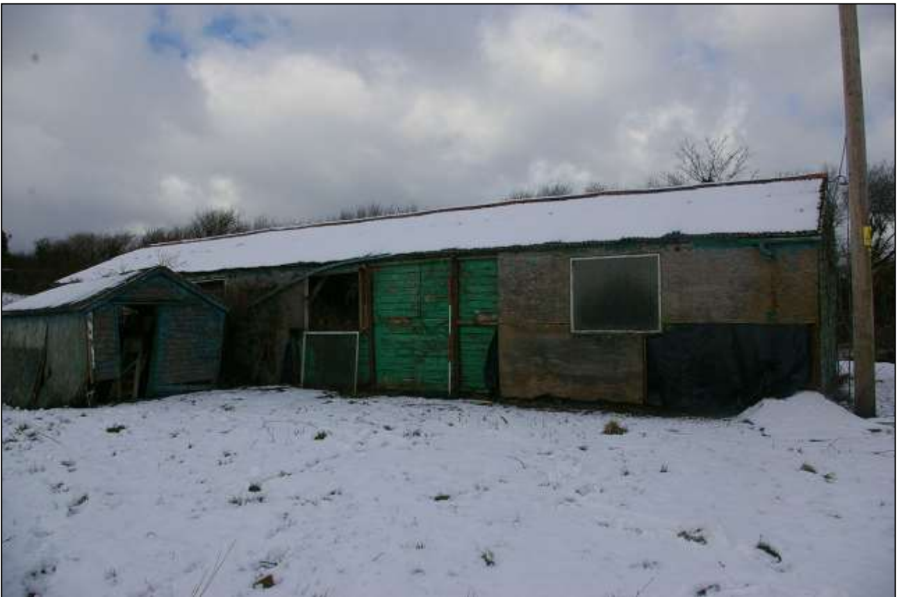
THE SOUTH ELEVATION OF THE BUILDING, WITH 2M SCALE; FROM THE EAST-SOUTH-EAST.
