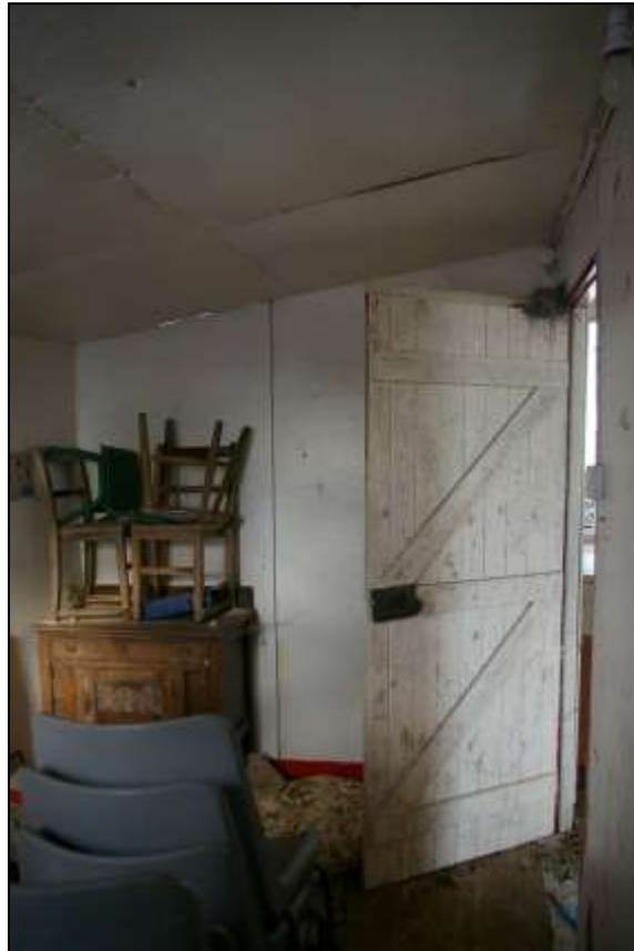
THE PLANK BOARDED DOOR, WHICH SERVES THE SMALL LEAN-TO STORE ON THE WEST END OF THE BUILDING; FROM THE SOUTH.
