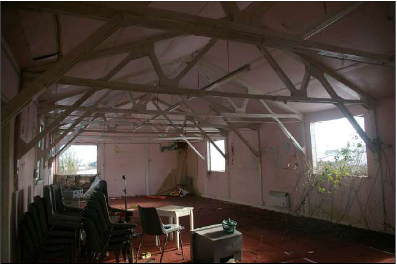
THE MAIN ROOM IN THE BUILDING, WITH OPEN TIMBER FRAMEWORK TRUSSES, BOARDED WALLS AND FLOOR; FROM THE WEST-NORTH-WEST.
