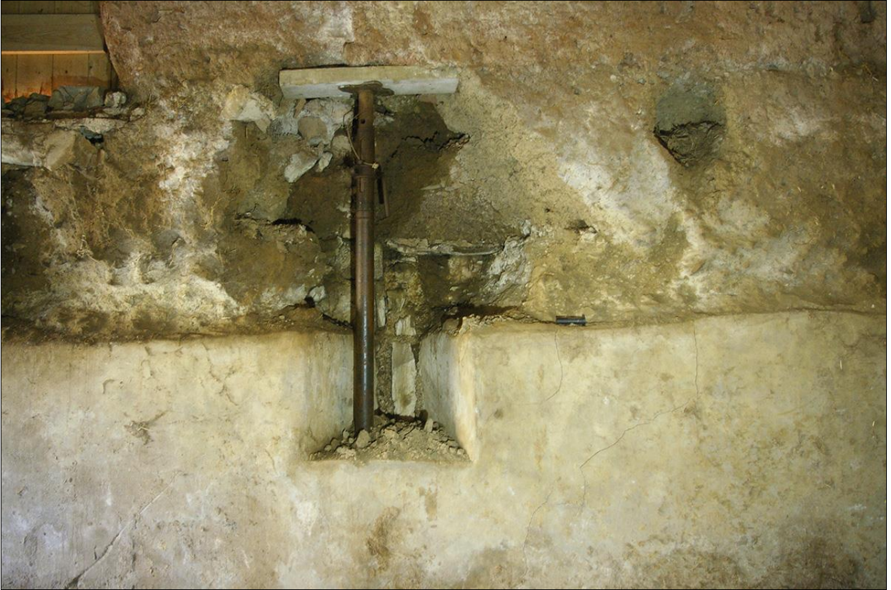
17. DETAIL OF THE CENTRAL SLIT VENT IN THE SOUTH WALL; VIEWED FROM THE NORTH.
