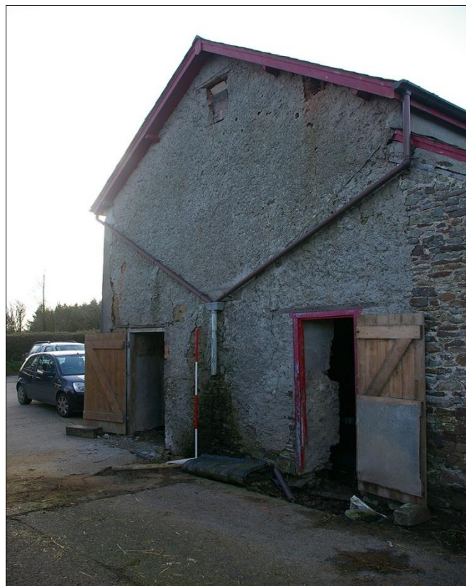
5. THE EAST GABLE WALL, SHOWING THE TWO DOORS AND OWL HOLE; VIEWED FROM THE NORTH-EAST (2M SCALE).
