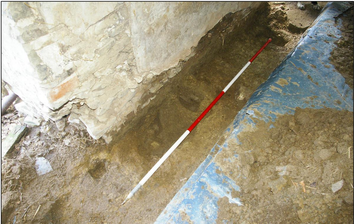
FIGURE 8: THE TRENCH VIEWED FROM A RAISED OBLIQUE ANGLE; FROM THE NORTH-WEST (2M SCALE).
