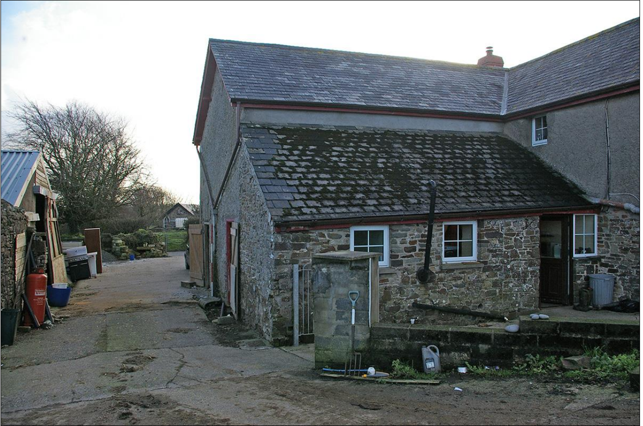
6. THE NORTH ELEVATION OF THE 'SHIPPON', WITH ABUTTING LEAN-TO; VIEWED FROM THE NORTH-EAST.
