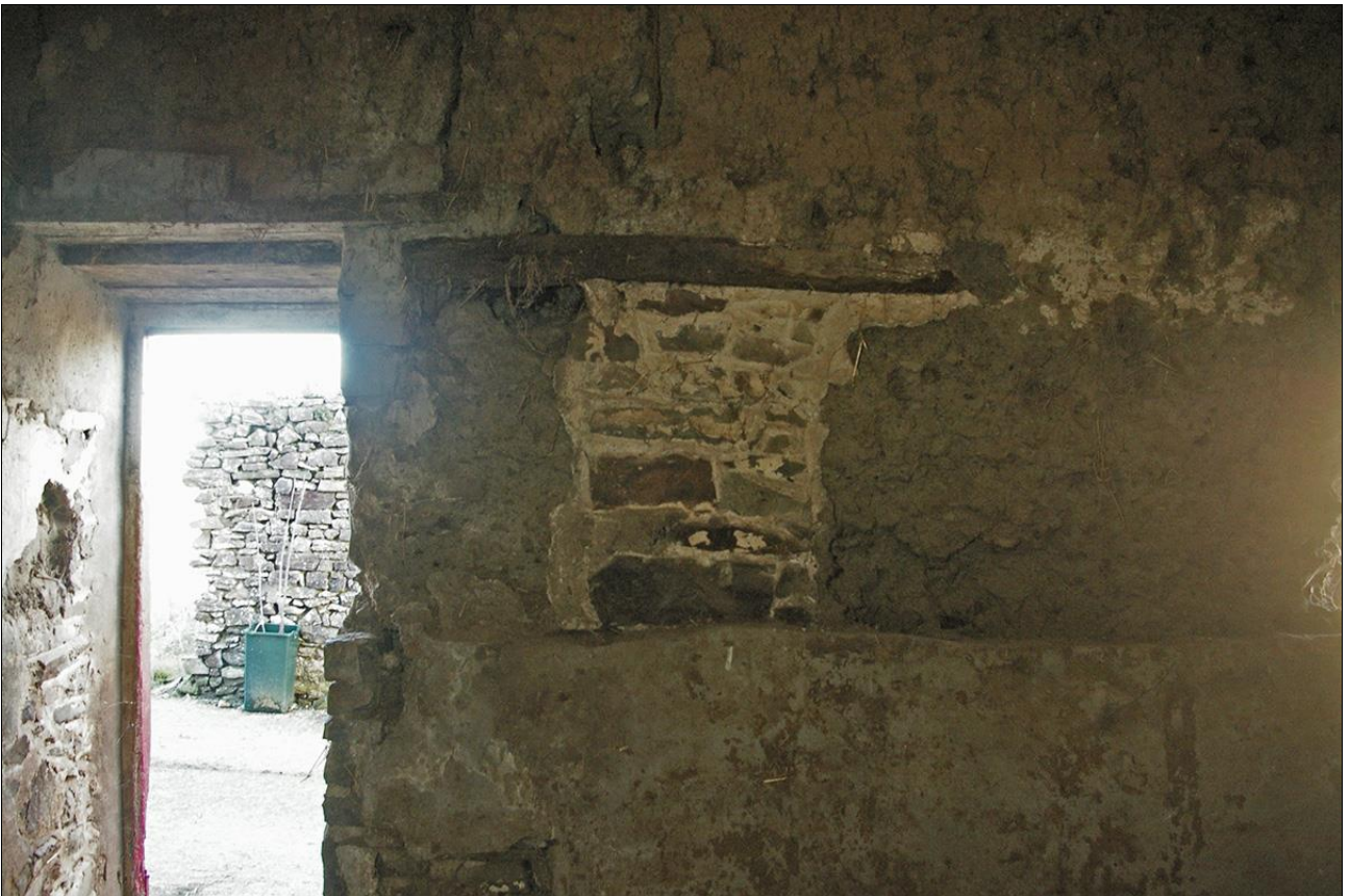
20. THE BLOCKED SLIT VENT IN THE EAST GABLE; VIEWED FROM THE WEST.
