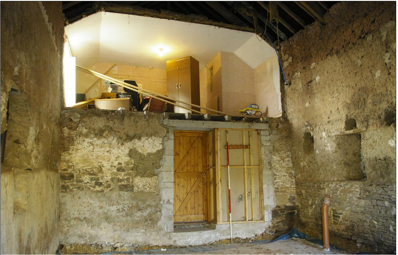
12. THE WEST WALL, PARTITION TO THE CROSS PASSAGE; VIEWED FROM THE SOUTH-EAST (SCALE 2M).
