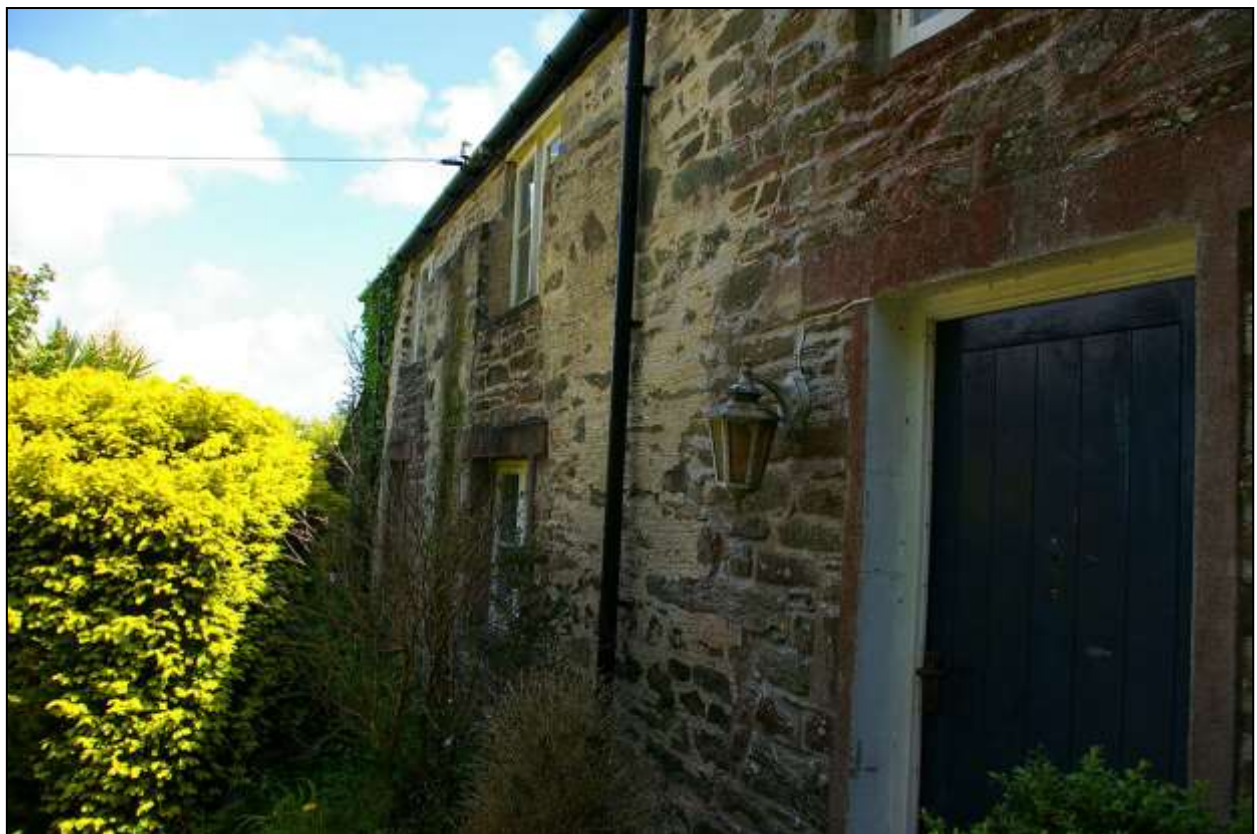
WIDER ANGLED VIEW SHOWING THE INCORPORATED RUINS AND FORCED FRONT DOOR, LEADING INTO THE INTERIOR; FROM THE WEST, NORTH-WEST.
