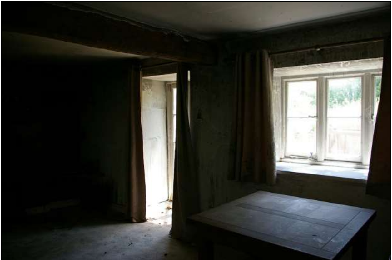
THE SOUTH WALL OF CR3, WITH FORCED PATIO DOORS AND 19 TH CENTURY WINDOW; FROM THE NORTH-EAST.
