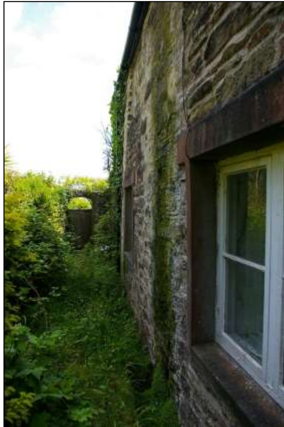
VIEW BACK ALONG THE INCORPORATED RUINED EARLIER BUILDING SHOWING THE SLIGHT BATTER TO THE WALL AND HOW THE WINDOWS AND RAISED EAVES ARE INSET BEHIND THE EARLIER WALLING, FORMING A LEDGE; FROM THE WEST.
