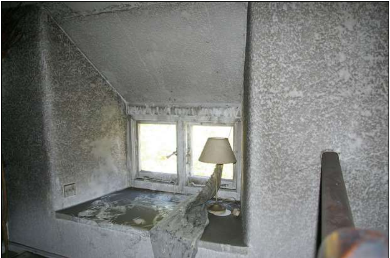
THE TWO LIGHT WINDOW SET INTO A BLOCKED LOADING DOOR IN THE FRONT WALL, CW4; FROM THE SOUTH-EAST.
