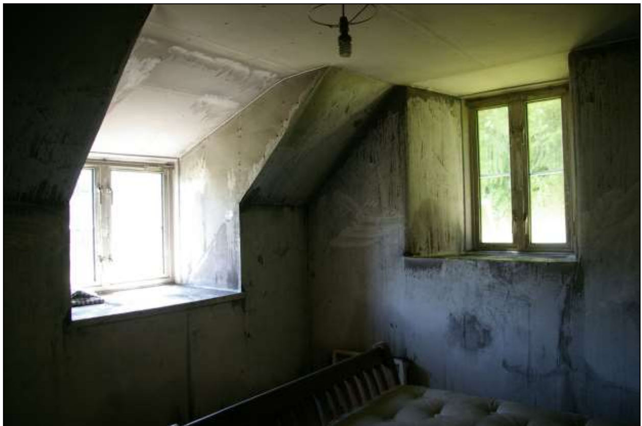
BEDROOM 1 WITH FORCED WINDOW OPENINGS AND PVC UNITS; FROM THE NORTH-EAST.
