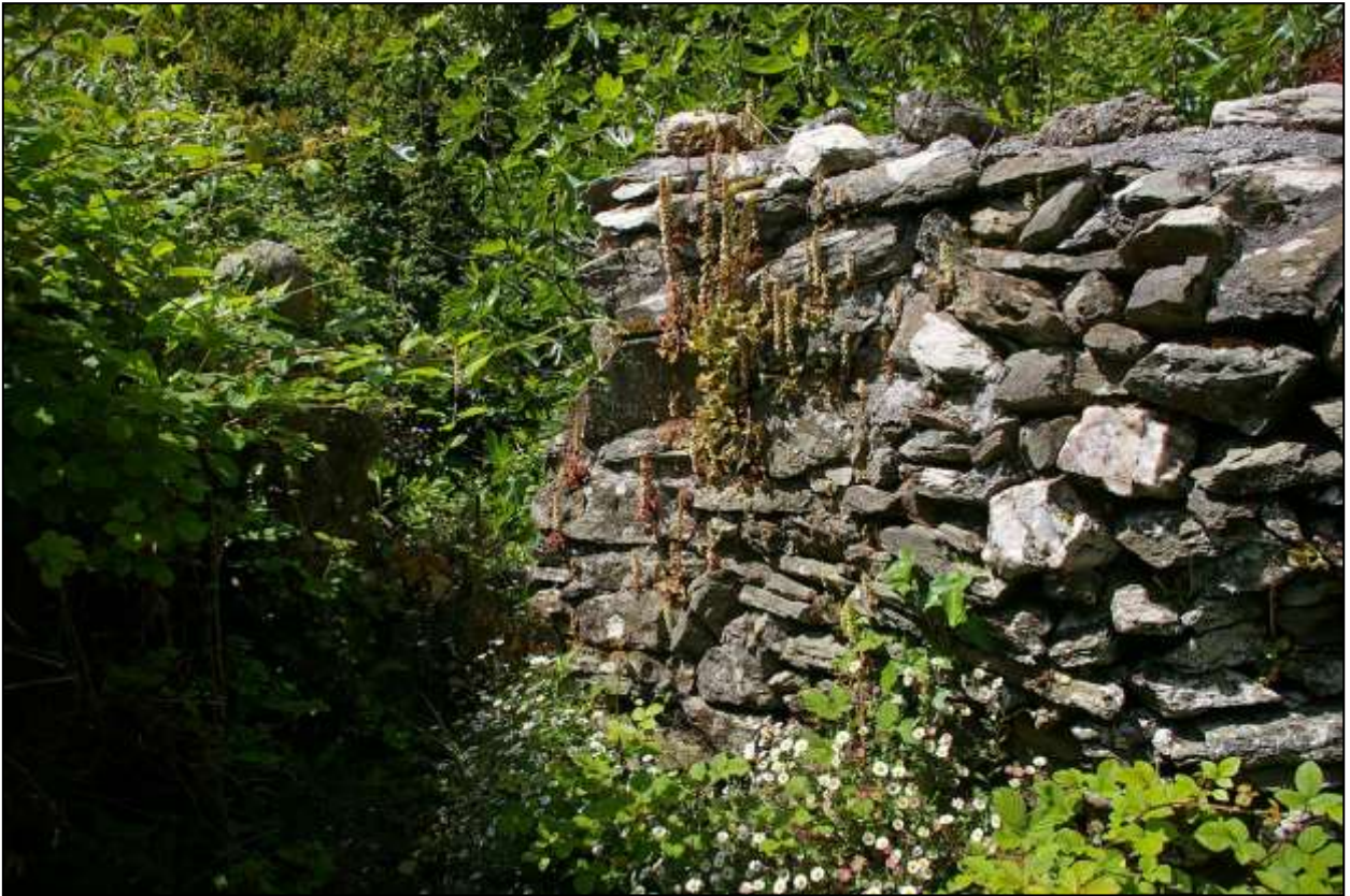
VIEW OF THE TWO DECORATIVE 19 TH CENTURY GARDEN WALLS WHICH FRAME THE REAR TERRACE TO THE FARMHOUSE, WITH A BALL FINIAL AND BLOCK OF QUARTZ, DECORATIVE QUARTZ USED THROUGHOUT THE BUILD AS A FEATURE TYPICAL OF THE PERIOD; FROM THE EAST.
