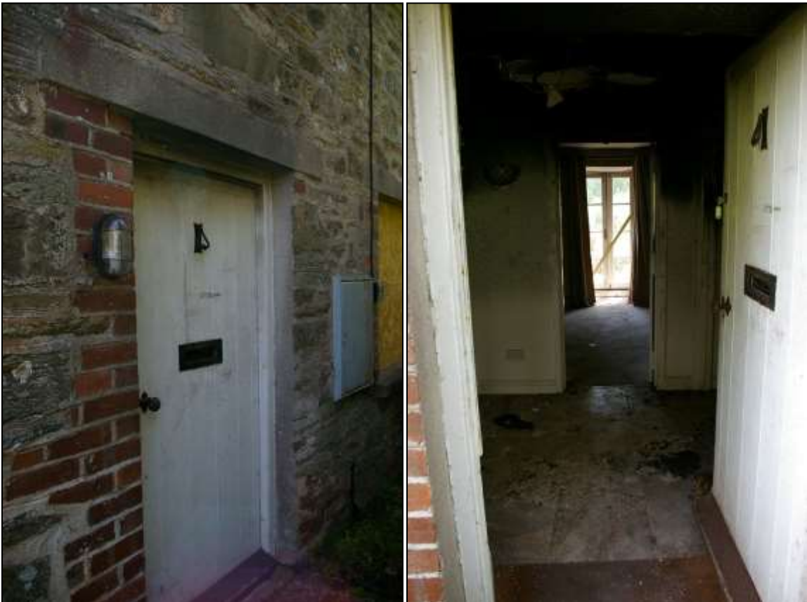
LEFT: THE FRONT DOOR TO THE COTTAGE, BRICK PATCHED REVEALS TO THE EAST, CONCRETE RENDER PATCHING TO THE WEST AND RENDERED LINTEL; FROM THE NORTH-EAST.
