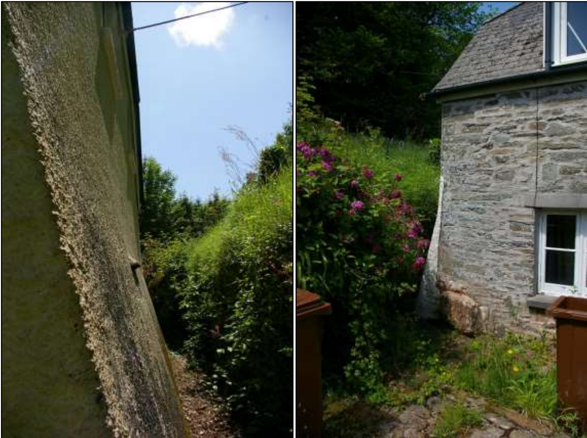
LEFT: THE WEST GABLE END OF THE COTTAGE, SHOWING HEAVY BUTTRESS AND FORCED WINDOWS SET HIGH IN APEX; FROM THE NORTH. RIGHT: VIEW OF THE SOUTH-WEST CORNER OF THE COTTAGE, SHOWING BRICK RENDERED BUTTRESS SUPPORTING THE WEST GABLE; FROM THE SOUTH-EAST.
