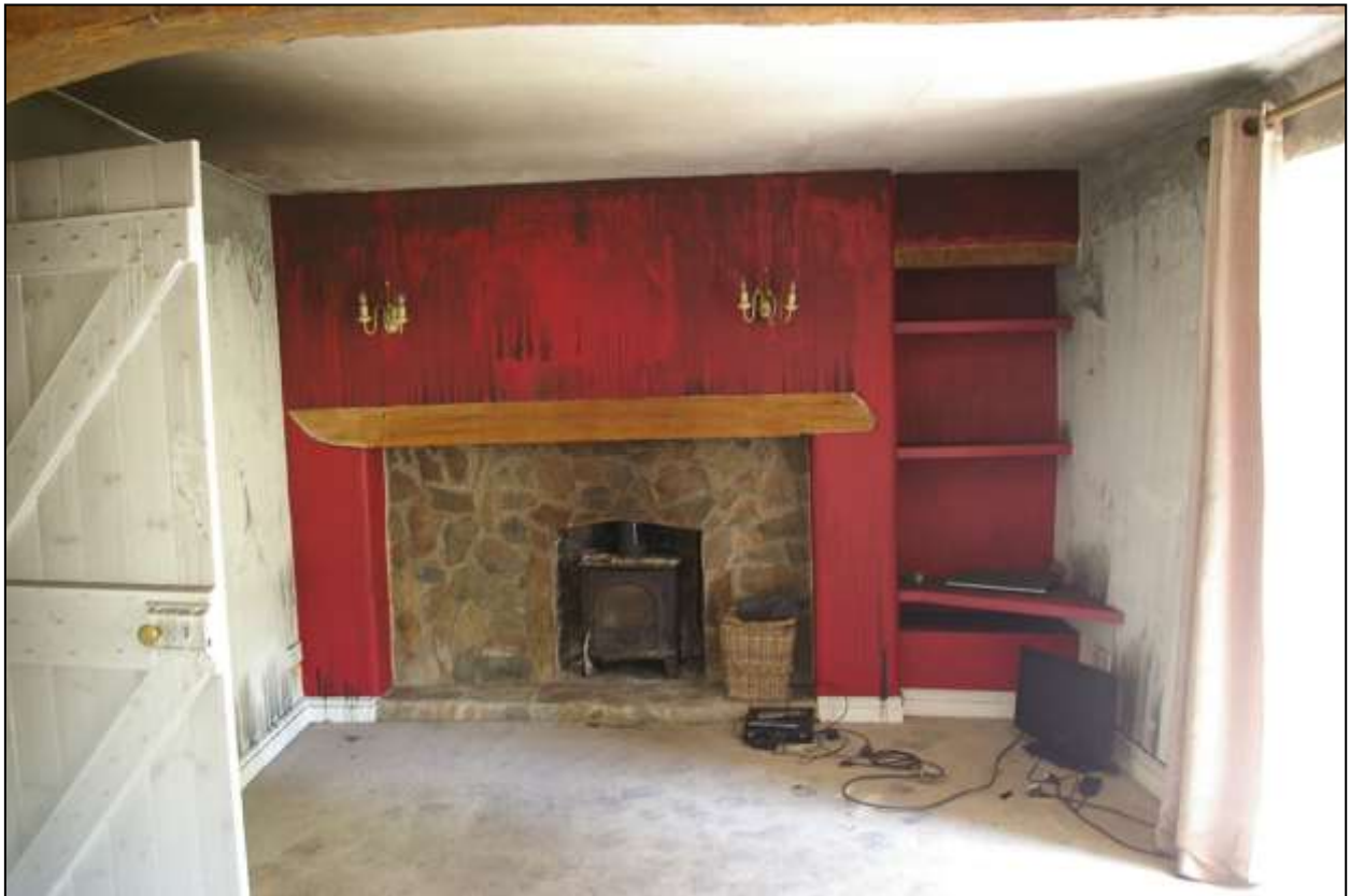
THE SHALLOW STACK AND BLOCKED FIREPLACE, WITH ALCOVE TO THE SOUTH, WITH TIMBER LINTEL; FROM THE WEST.
