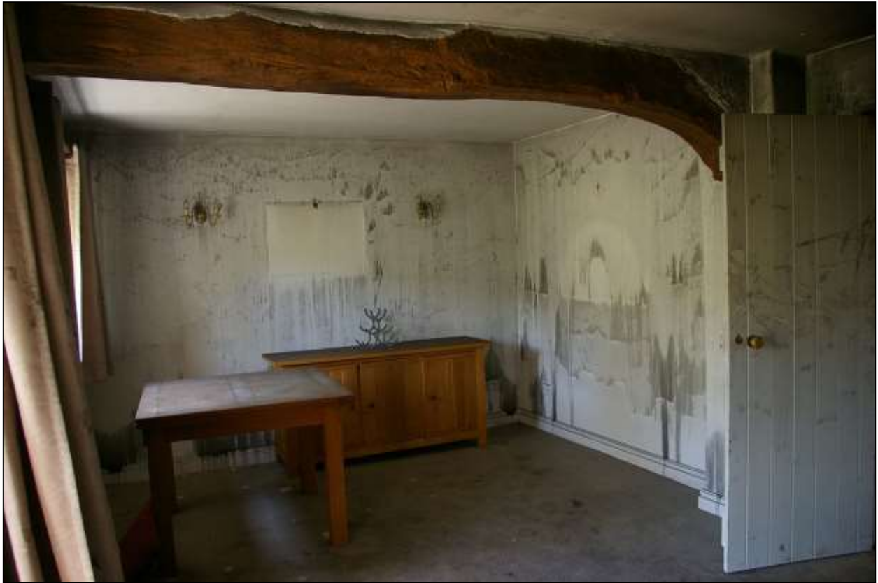
THE BEAM IN MORE DETAIL, BRACING A FORMER PARTITION LINE/WALL LINE; FROM THE SOUTH-EAST.
