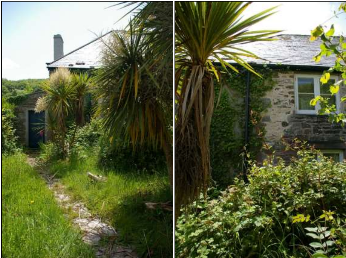
LEFT: THE LEAN-TO WITH AN OLD SECTION OF WALLING WHICH THE CONSERVATORY ABUTS FROM THE SOUTH SIDE; FROM THE NORTH, NORTH-WEST.
