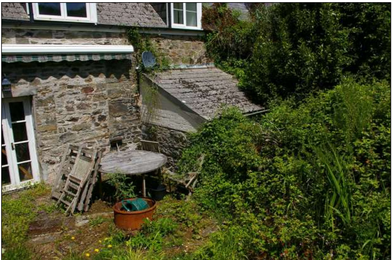
THE PROJECTING BLOCK, OF AN OLDER FORM OF PLATEY STONEWORK, OFF THE BACK OF THE SOUTH ELEVATION ACROSS THE JOIN BETWEEN COTTAGE AND FARMHOUSE; FROM THE SOUTH-WEST.
