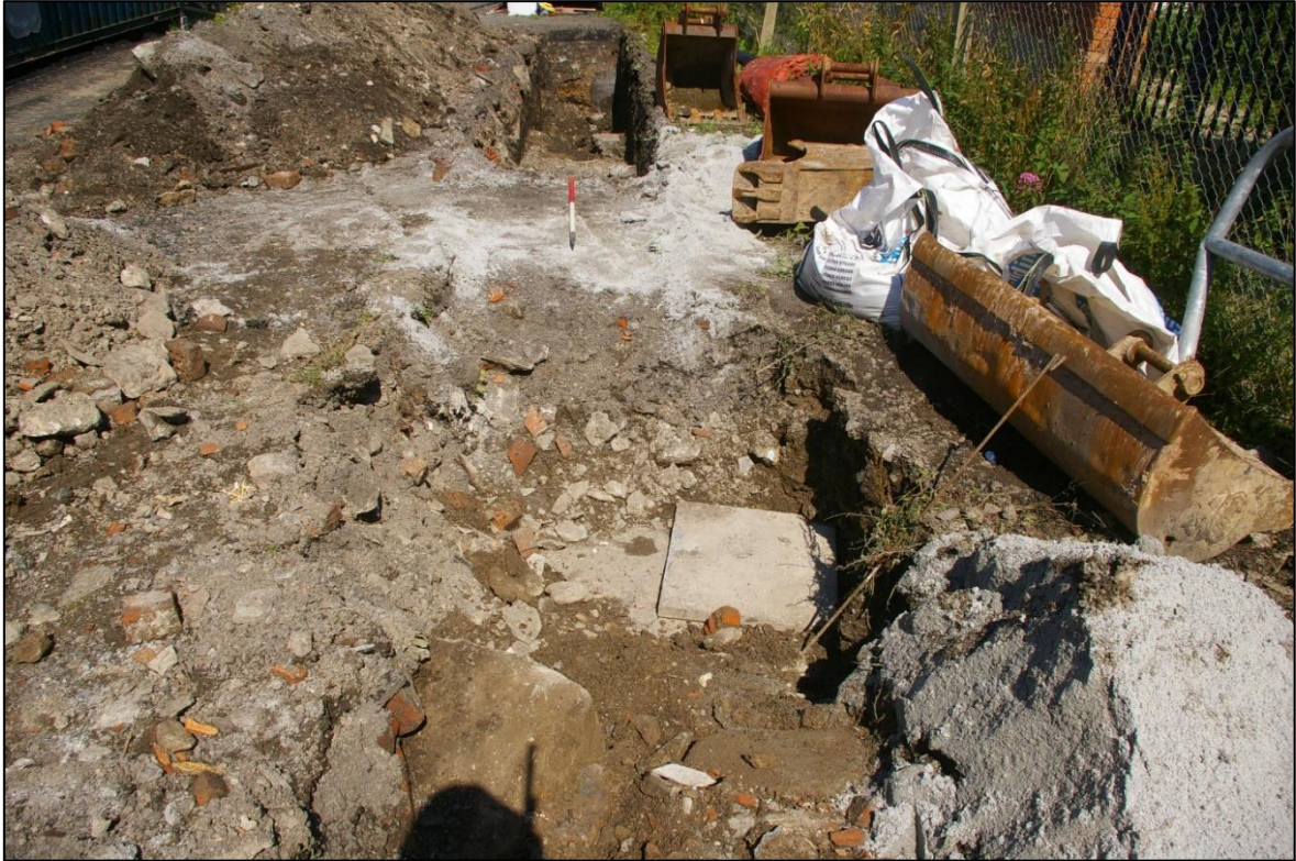
11. TRENCH 03, POST-EXCAVATION, SHOWING MODERN BRICK INSPECTION CHAMBER (COVERED BY CONCRETE SLAB); VIEWED FROM THE SOUTH-WEST (1M SCALE).
