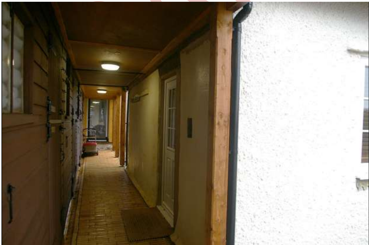
21. THE STABLES, BUILT ACROSS AND ABUTTING THE STABLES COTTAGE; FROM THE WEST.
