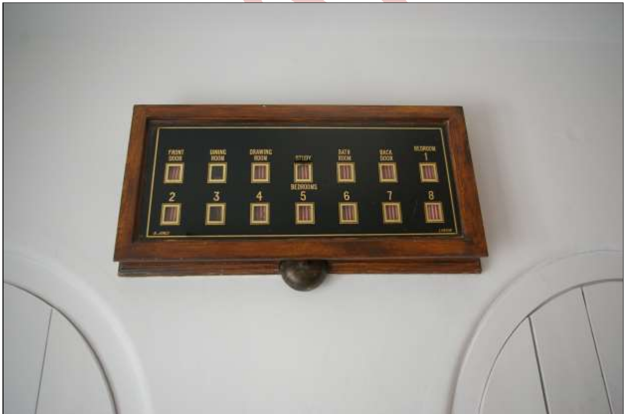
47. THE SERVANTS ELECTRIC BELL SYSTEM IN THE BOOT ROOM, ROOM 8; FROM THE WEST.
