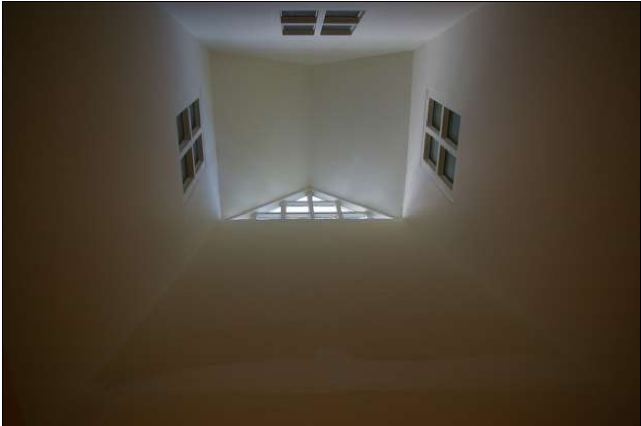
79. THE SKYLIGHT WHICH LIGHTS THE EAST CORRIDOR TO THE BEDROOMS AND THE ATTIC; FROM BELOW; THE SOUTH.
