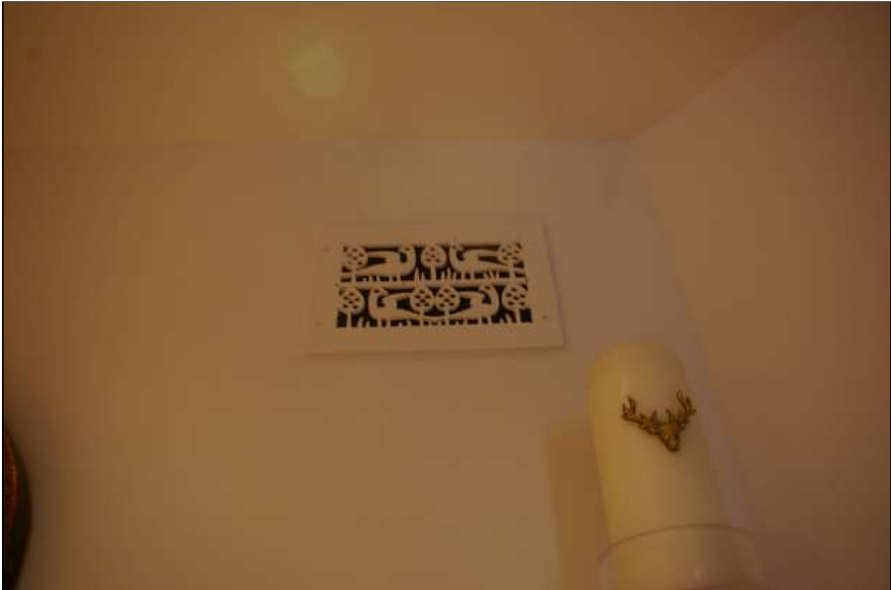
36. THE STYLISED AND VERY FINE 'ARTS & CRAFTS' AIR VENT IN THE STACK SERVING THE FIREPLACE IN AREA 5A, POTENTIALLY SHOWING 'PARTRIDGE IN A PEAR TREE' OR OTHER GAME BIRDS; FROM THE SOUTH-EAST.
