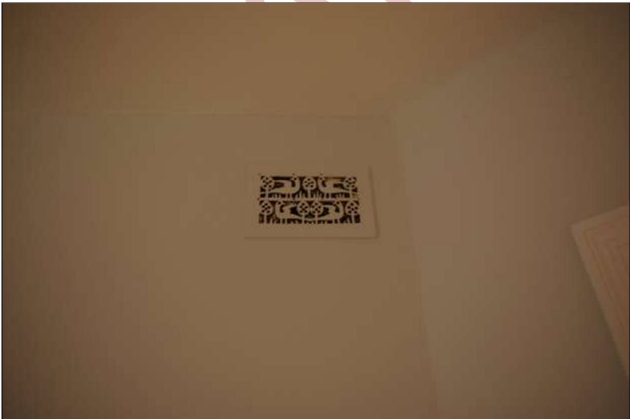
75. DETAIL OF ANOTHER OF THE GOOD MATCHED SET OF AIR VENTS TO THE STACK IN LILLYCOMBE HOUSE, IN ROOM 22; FROM THE EAST.
