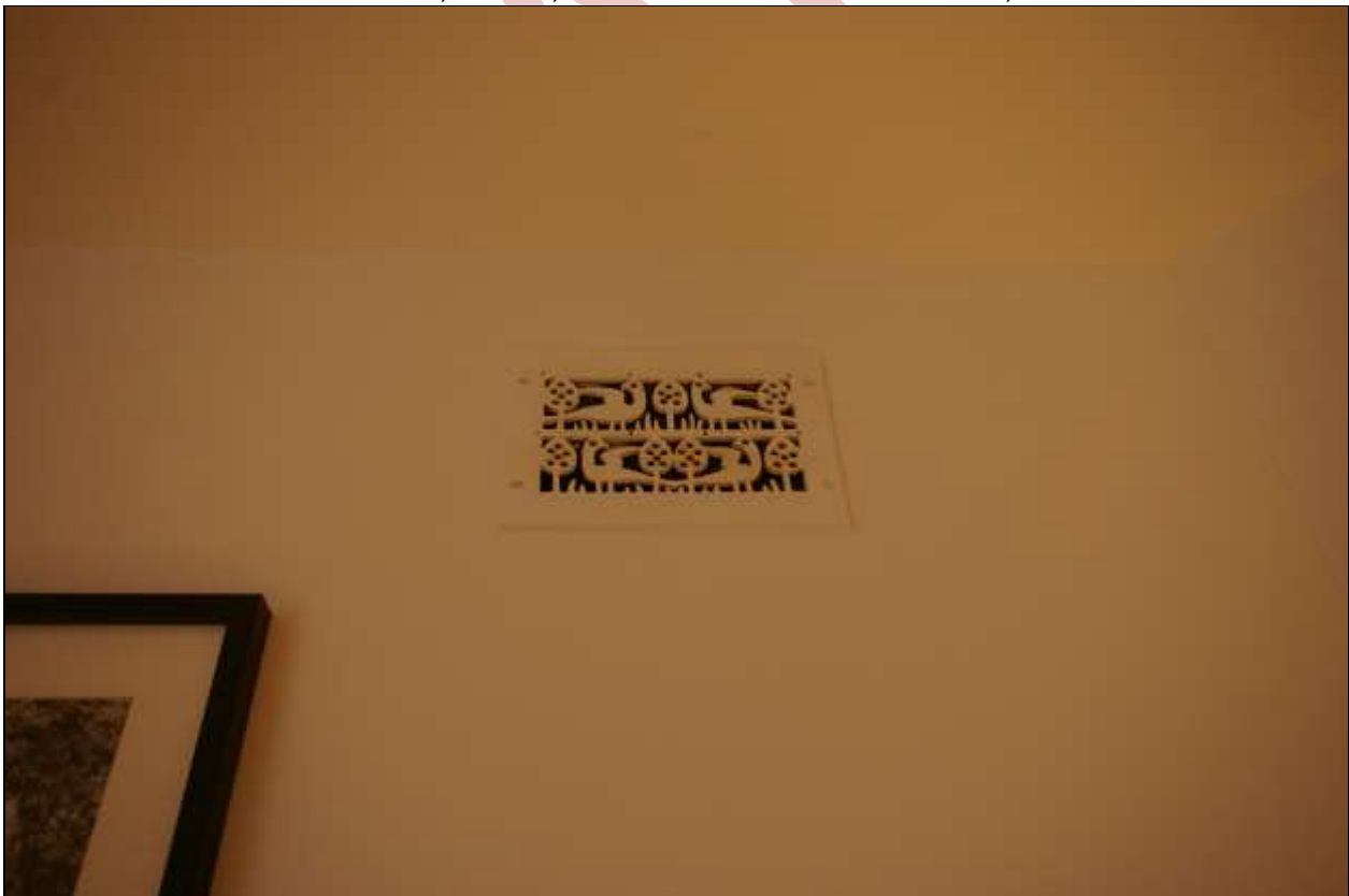
64. THE STYLISED AND VERY FINE 'ARTS & CRAFTS' AIR VENT IN THE STACK SERVING THE FIREPLACE IN ROOM 16, POTENTIALLY SHOWING 'PARTRIDGE IN A PEAR TREE' OR OTHER GAME BIRDS; FROM THE NORTH-EAST.
