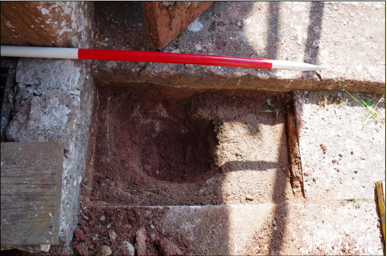
FIGURE 2: CONDUCTOR PIT 7, SHOWING THE THRESHOLD STONE AND RUBBLE FOOTINGS TO THE DEMOLISHED ENTRANCE; VIEWED FROM WEST (1M SCALE).
