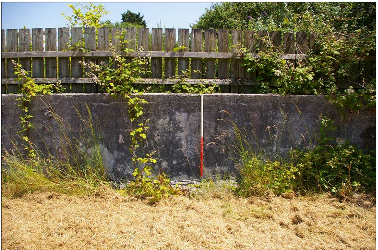
36. DETAIL OF THE MODERN CONCRETE BLOCK WALL AND WOODEN FENCE EASTERN BOUNDARY OF FIELD 2; FROM THE WEST (1M SCALE).
