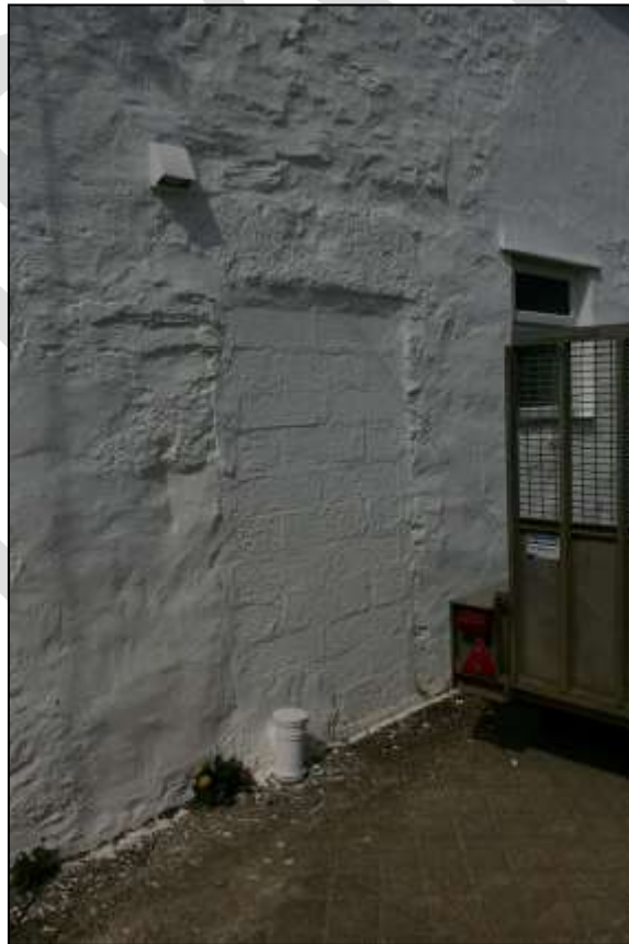
BLOCKED DOOR IN THE EAST WALL OF BUILDING D; FROM THE SOUTH, SOUTH-EAST.
