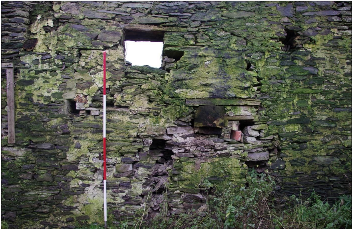
42. THE WESTERN INTERIOR WALL OF B2A & B, SHOWING SEVERAL SMALLER FORCED OPENINGS FOR MACHINE AND TRUSS SUPPORTS FOR B3. (WITH 2M SCALES). TAKEN FROM THE EAST.
