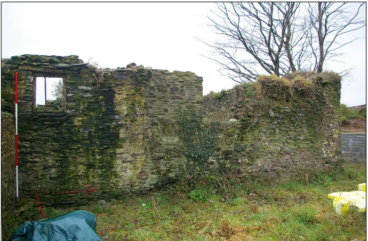
52. THE OLDER EASTERN BARN WALLS OF B2A; SHOWING THE EXTERIOR STONE PLINTH AND FORCED WINDOW OPENINGS. (WITH 2M SCALES). TAKEN FROM THE EAST.
