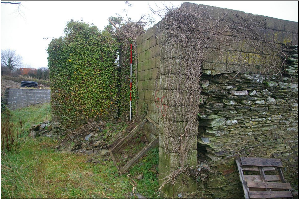
10. BUILDING 2A LOOKING AT THE REBUILT CONCRETE WALL IN THE WESTERN CORNER (WITH 2M SCALES). TAKEN FROM WEST.
