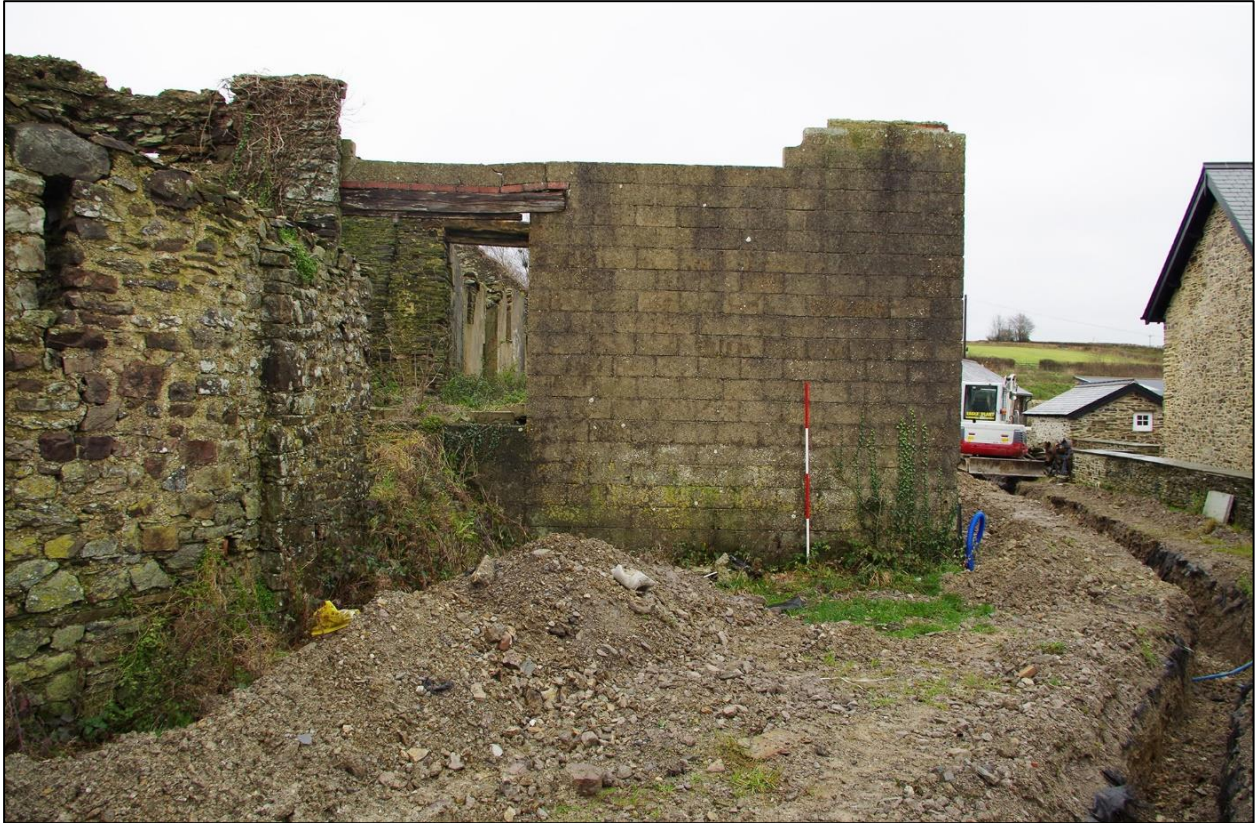
47. THE LATER ADJUSTED WESTERN CONCRETE BLOCK EXTERIOR OF B2B AND OPENED SERVICE TRENCH (TRENCH 1). (WITH 2M SCALES). TAKEN FROM THE WEST.
