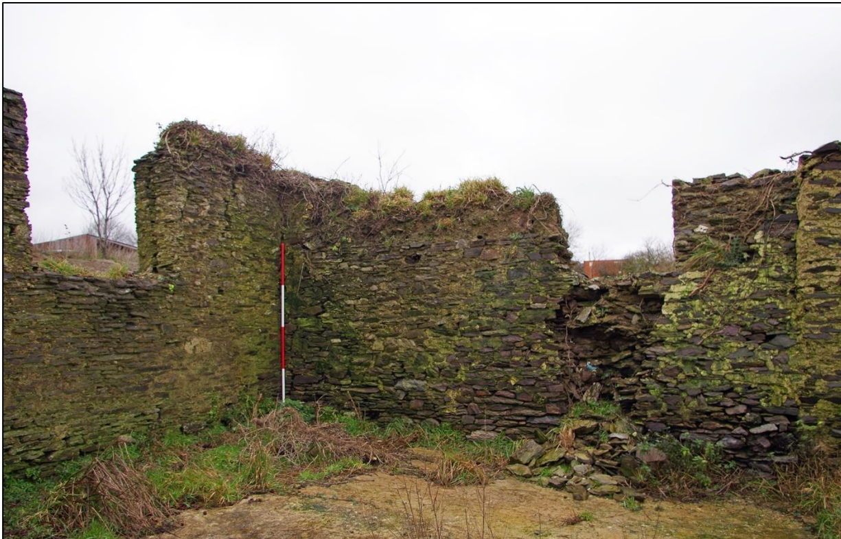
26. B2A WESTERN WALL SHOWING THE COB TOP AND FORCED WINDOW OPENINGS. (WITH 2M SCALES). TAKEN FROM THE WEST.
