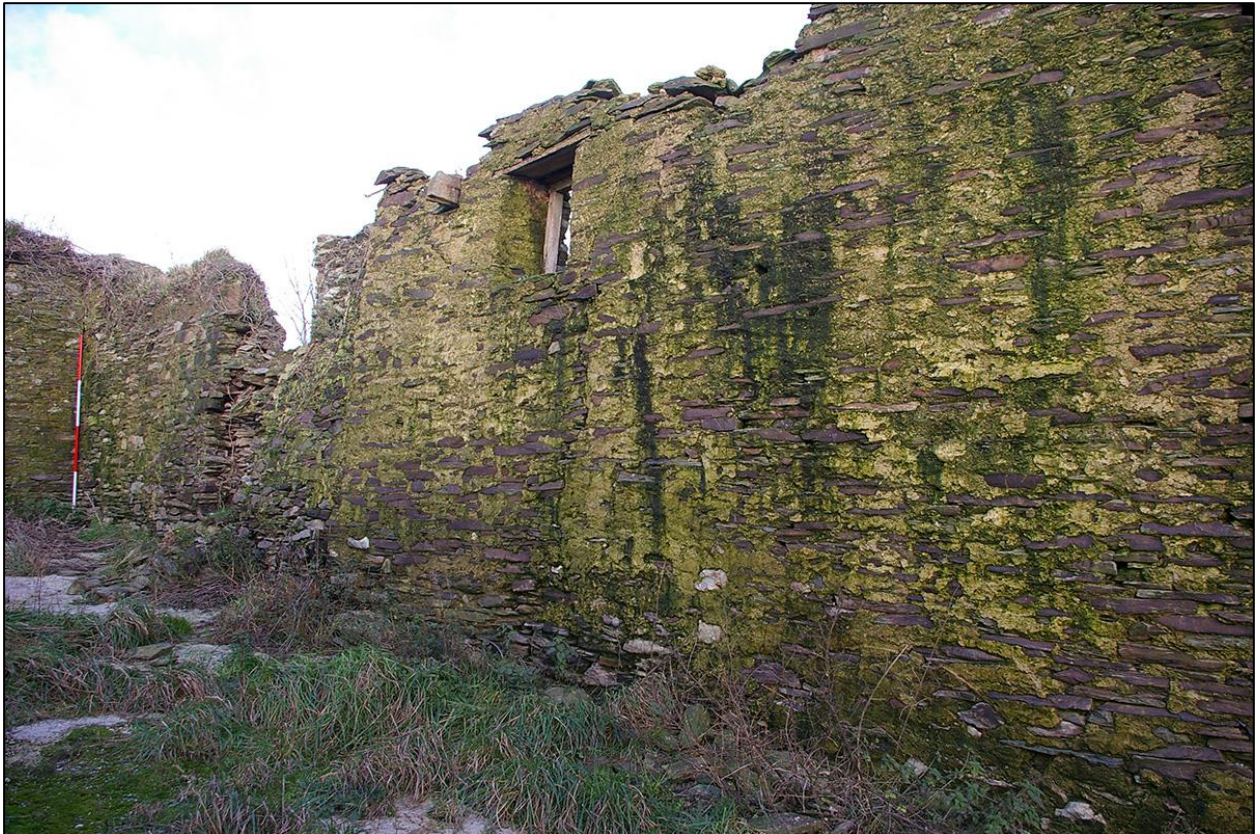
29. WESTERN WALL OF B2A AND B2B; SHOWING THE BUILD LINES AND TRUSS SCARS. (WITH 2M SCALES). TAKEN FROM THE SOUTH WEST.
