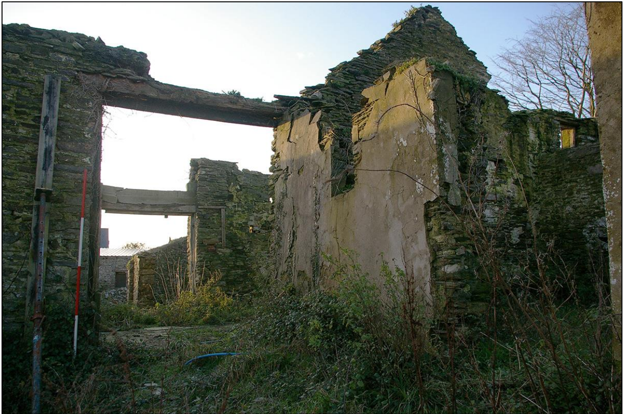
50. THE MAIN ENTRANCE FROM THE STABLES, LOOKING IN TO B2B AND B3. (WITH 2M SCALES). TAKEN FROM THE SOUTH EAST.
