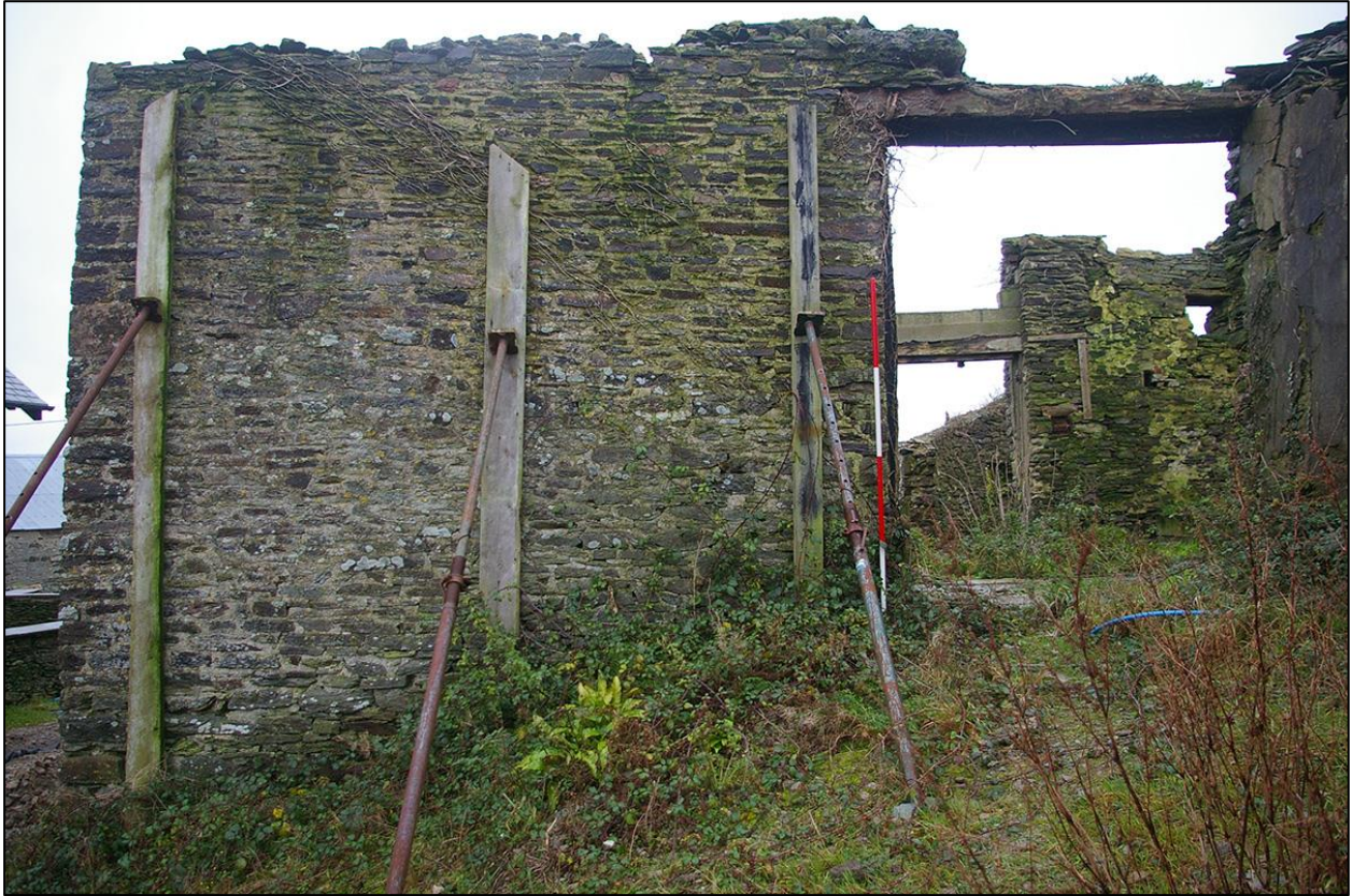
49. THE EASTERN EXTERIOR WALL OF B2B SHOWING THE EARLY DOUBLE DOORED ENTRANCE (WITH 2M SCALES). TAKEN FROM THE EAST.
