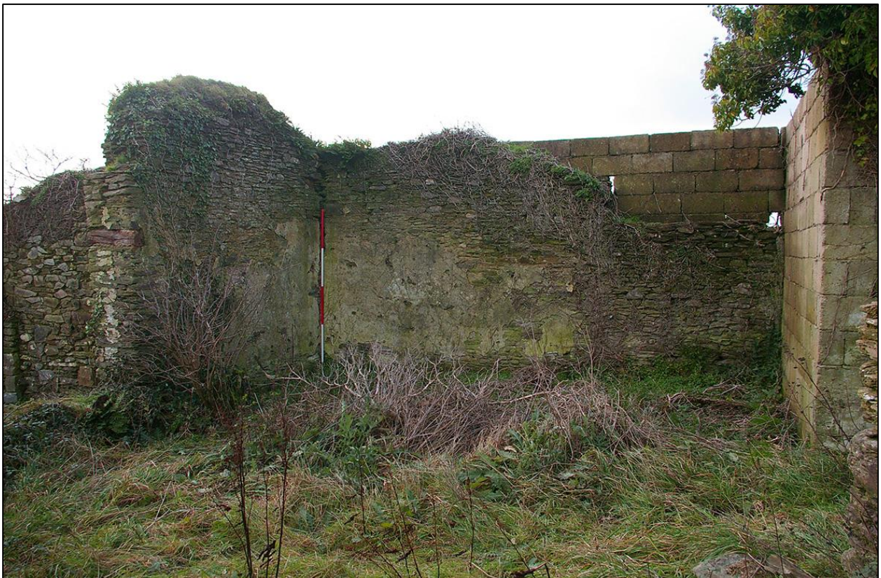
22. BUILDING 2A SOUTH WESTERN CORNER, LOOKING INTO B3 TO THE LEFT. PLASTER IS STILL VISIBLE ON SOME OF THE WALLS (WITH 2M SCALES). TAKEN FROM THE EAST.
