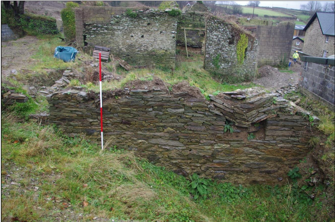
FIGURE 12: B1, WEST WALL, SHOWING WINDOW OPENINGS AND HEAVY SLATESTONE BUILD; FROM THE WEST (2M SCALE).
