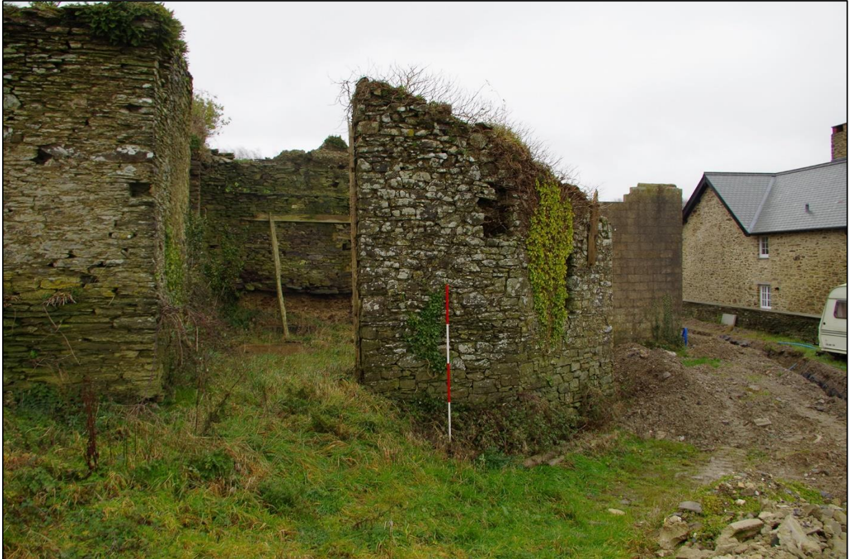
53. EXTERNAL WALLS OF B3 LOOKING DOWN TOWARDS THE FARMHOUSE. (WITH 2M SCALES). TAKEN FROM THE WEST.
