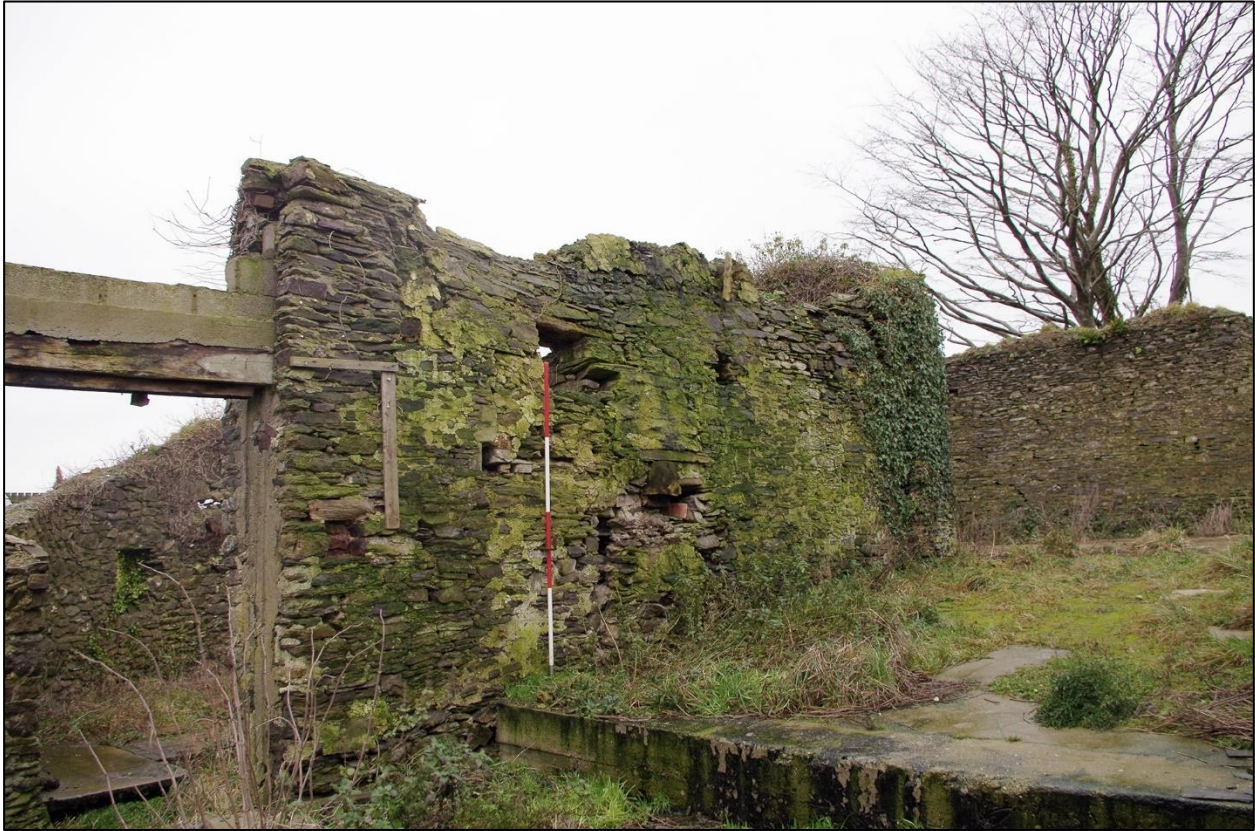
44. LOOKING UP TOWARDS B2A AND LOOKING INTO B3. (WITH 2M SCALES). TAKEN FROM THE SOUTH EAST.
