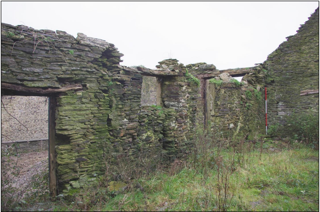
62. SOUTHERN WALL OF B4 SHOWING BOTH DOORWAYS AND WINDOWS. (WITH 2M SCALES). TAKEN FROM THE NORTH EAST.
