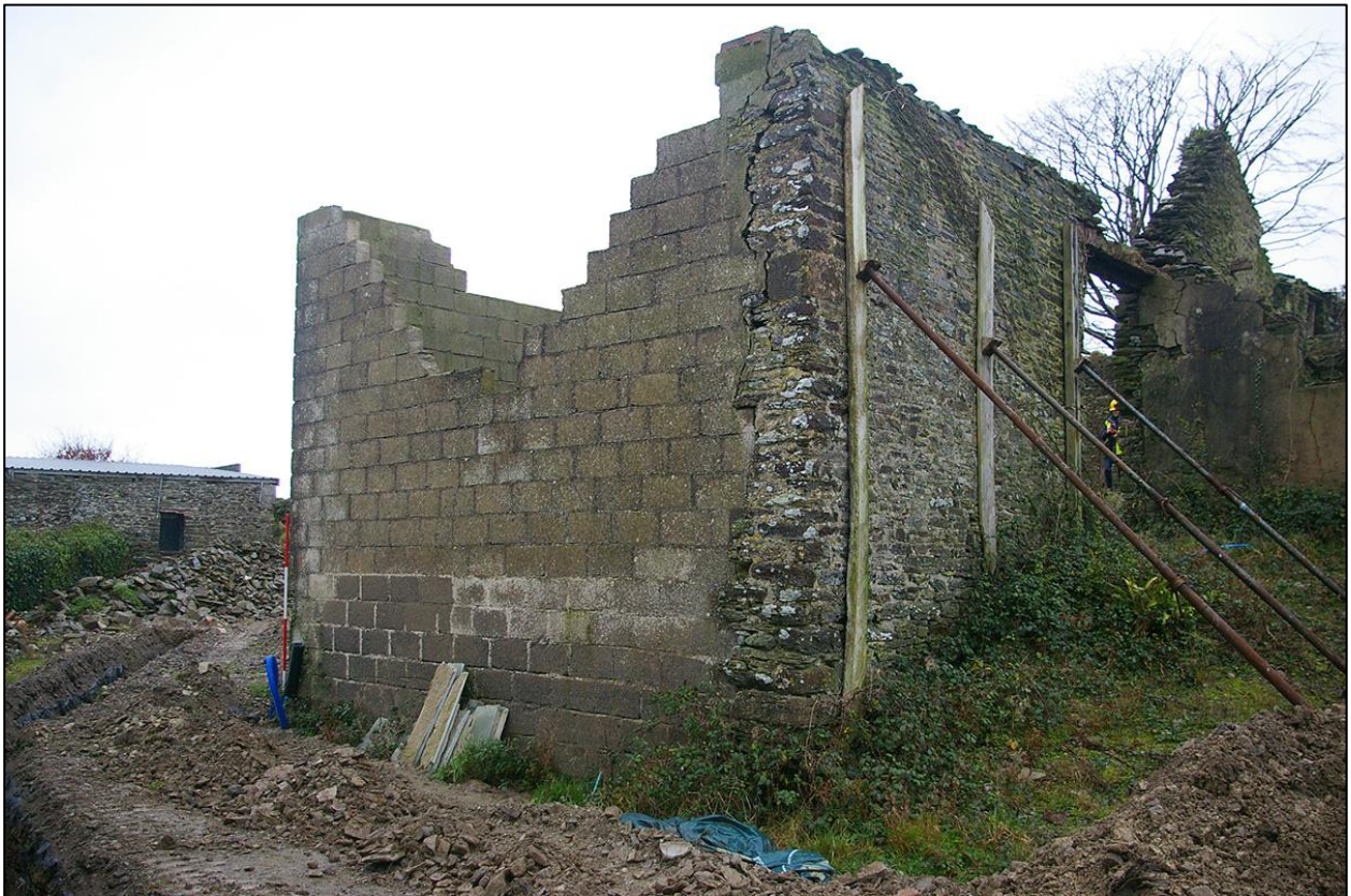
48. THE SOUTHERN WALL OF B2B. TAKEN FROM THE SOUTH EAST. (WITH 2M SCALES).
