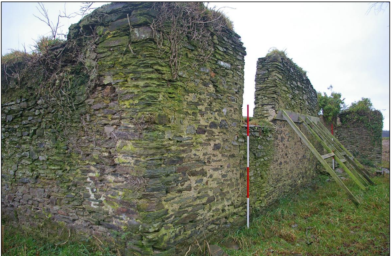
15. BUILDING 2A AND FORCED NORTHERN WINDOW. (WITH 2M SCALES). TAKEN FROM THE NORTH EAST.
