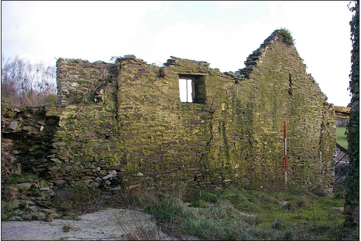
31. B2B THE STABLE GABLED WALL AND SURVIVING WINDOW OPENINGS. (WITH 2M SCALES). TAKEN FROM THE WEST.
