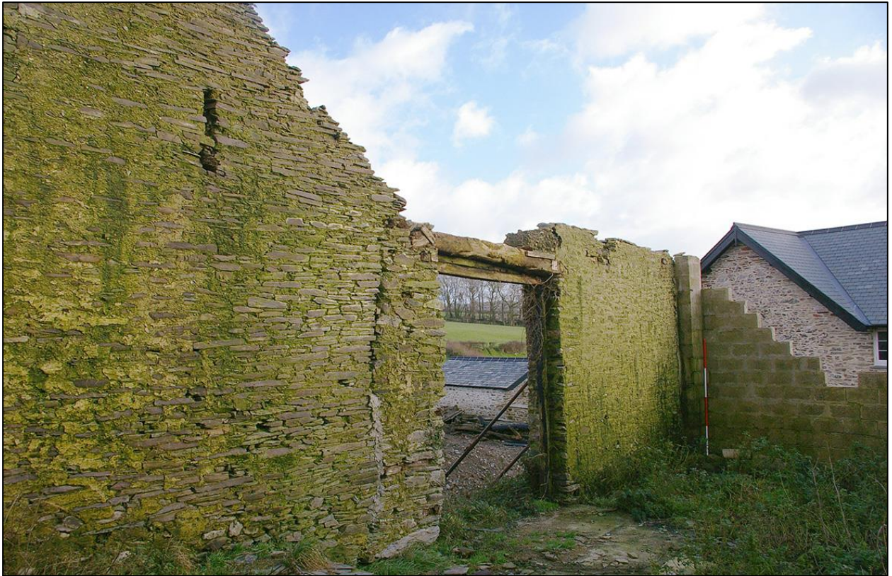
35. B2B LOOKING INTO THE FORMER DOUBLE DOORED ENTRANCE WITH TIMBER LINTEL SURVIVING. (WITH 2M SCALES). FROM THE NORTH WEST.
