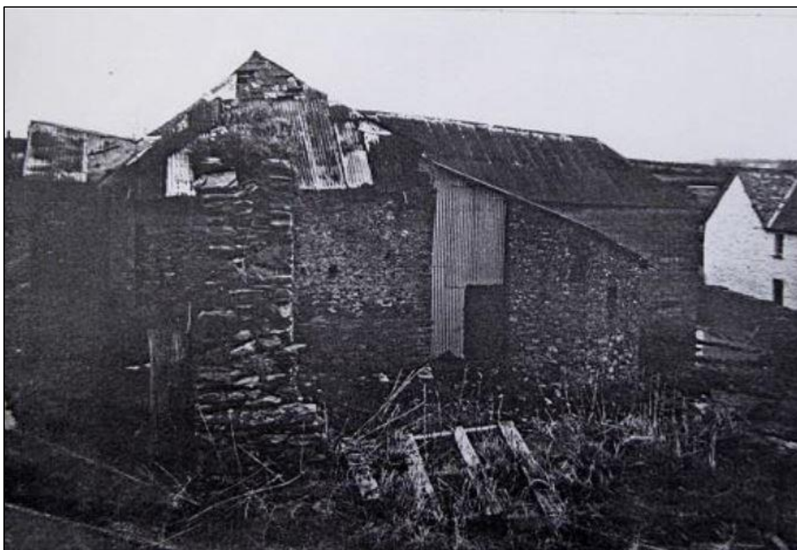
FIGURE 11: 1989 PHOTOGRAPH TAKEN FROM THE WESTERN EDGES OF THE SITE. B2A VISIBLE ON THE LEFT, WITH B3 VISIBLE TO THE RIGHT AND THE WHITE RENDERED FARMHOUSE IN THE BACKGROUND (FROM: NIMROD RESEARCH, 2017).
