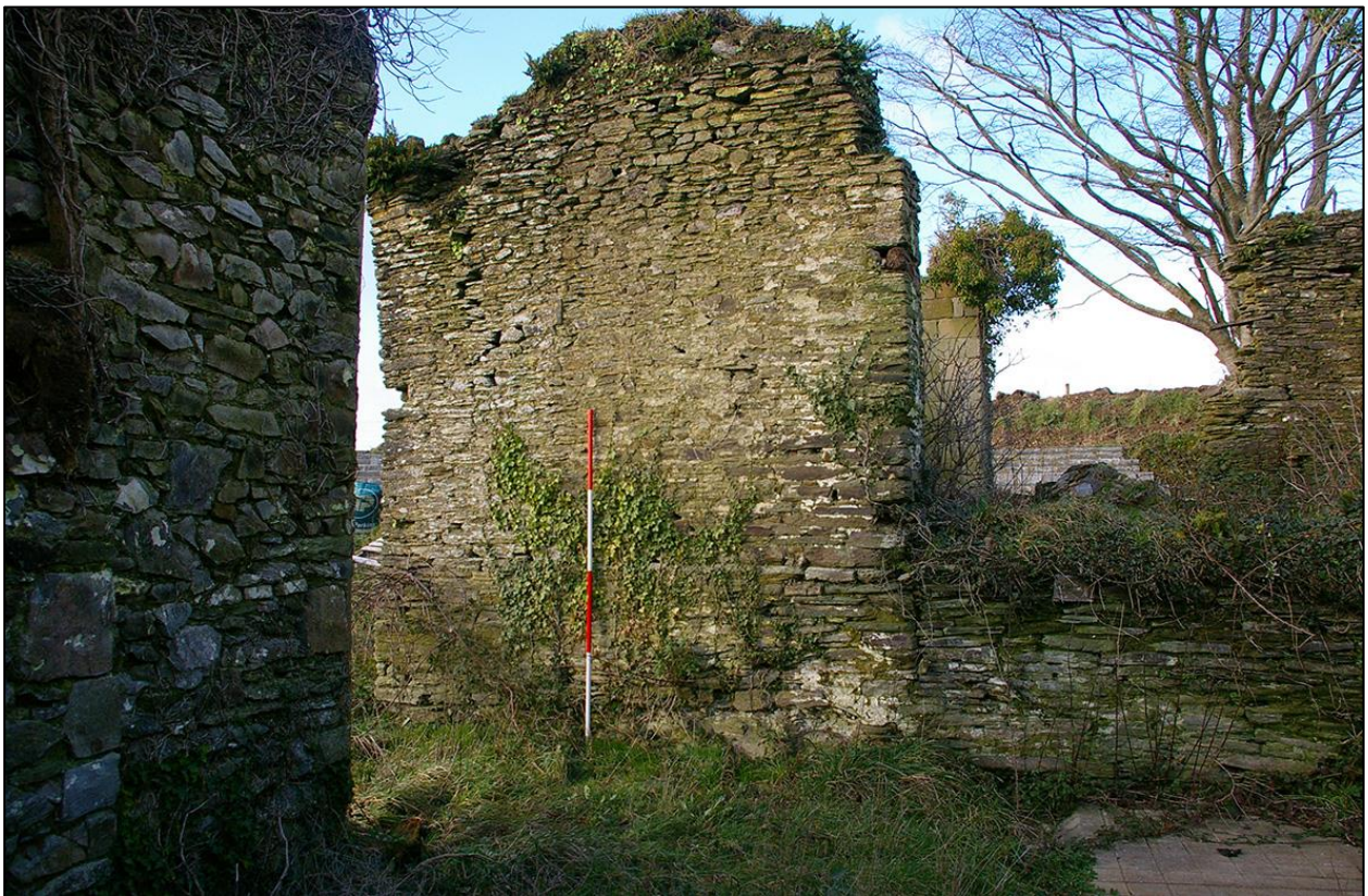
18. LOOKING INTO BUILDING 2A FROM B3; SHOWING THE WESTERN OPENING AND PARALLEL FORCED OPENINGS IN B2A. (WITH 2M SCALES). TAKEN FROM THE WEST.
