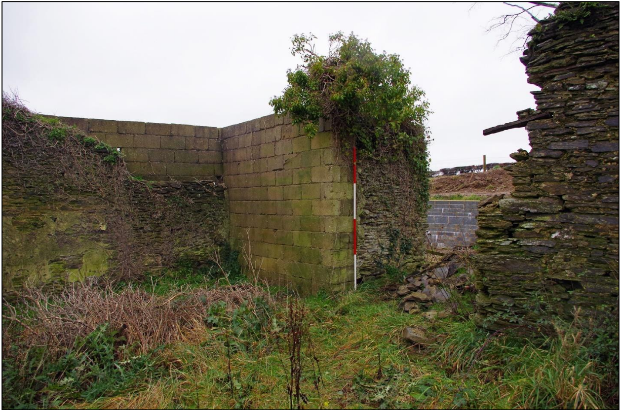
23. BUILDING 2A; SHOWING THE LATER FORCED NORTHERN OPENING TO AID THE DEVELOPMENT OF THE MACHINE HOUSE IN B3. (WITH 2M SCALES). TAKEN FROM THE SOUTH EAST.
