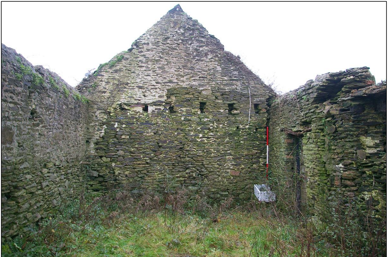
64. EASTERN GABLED END OF B4 SHOWING TRUSS HOLES FOR UPPER STORAGE AREA. (WITH 2M SCALES). TAKEN FROM THE WEST.
