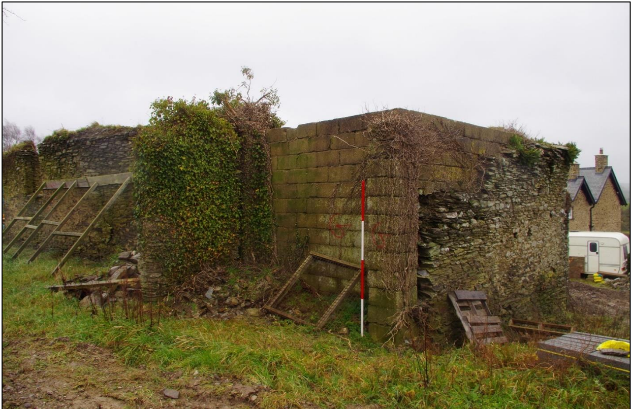
9. BUILDING 2A; WESTERN CORNER CONCRETE REBUILD (WITH 2M SCALES). TAKEN FROM THE NORTH WEST.
