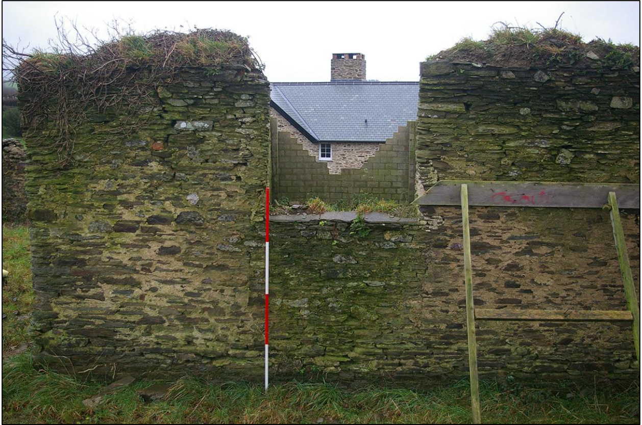
14. BUILDING 2A AND FORCED OPENING. TAKEN FROM THE NORTH.
