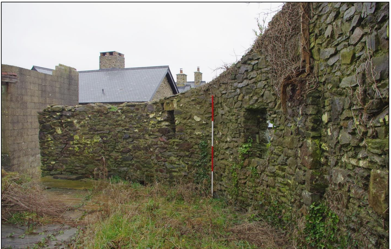
58. INSIDE B3 SHOWING THE CURVED BARN WALLS. (WITH 2M SCALES). TAKEN FROM THE SOUTH.
