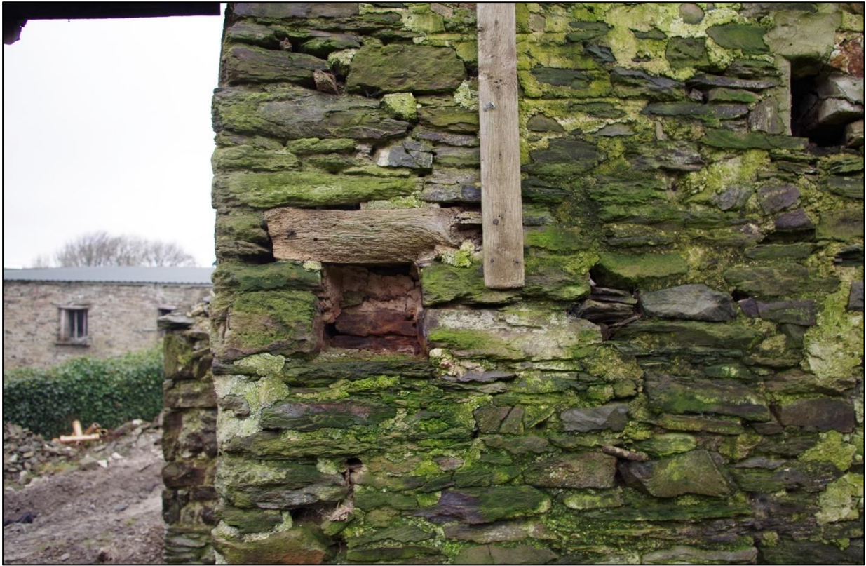
43. THE WESTERN INTERIOR WALL OF B2B SHOWING THE SMALL FORCED OPENING FOR CANDLES. TAKEN FROM THE EAST.
