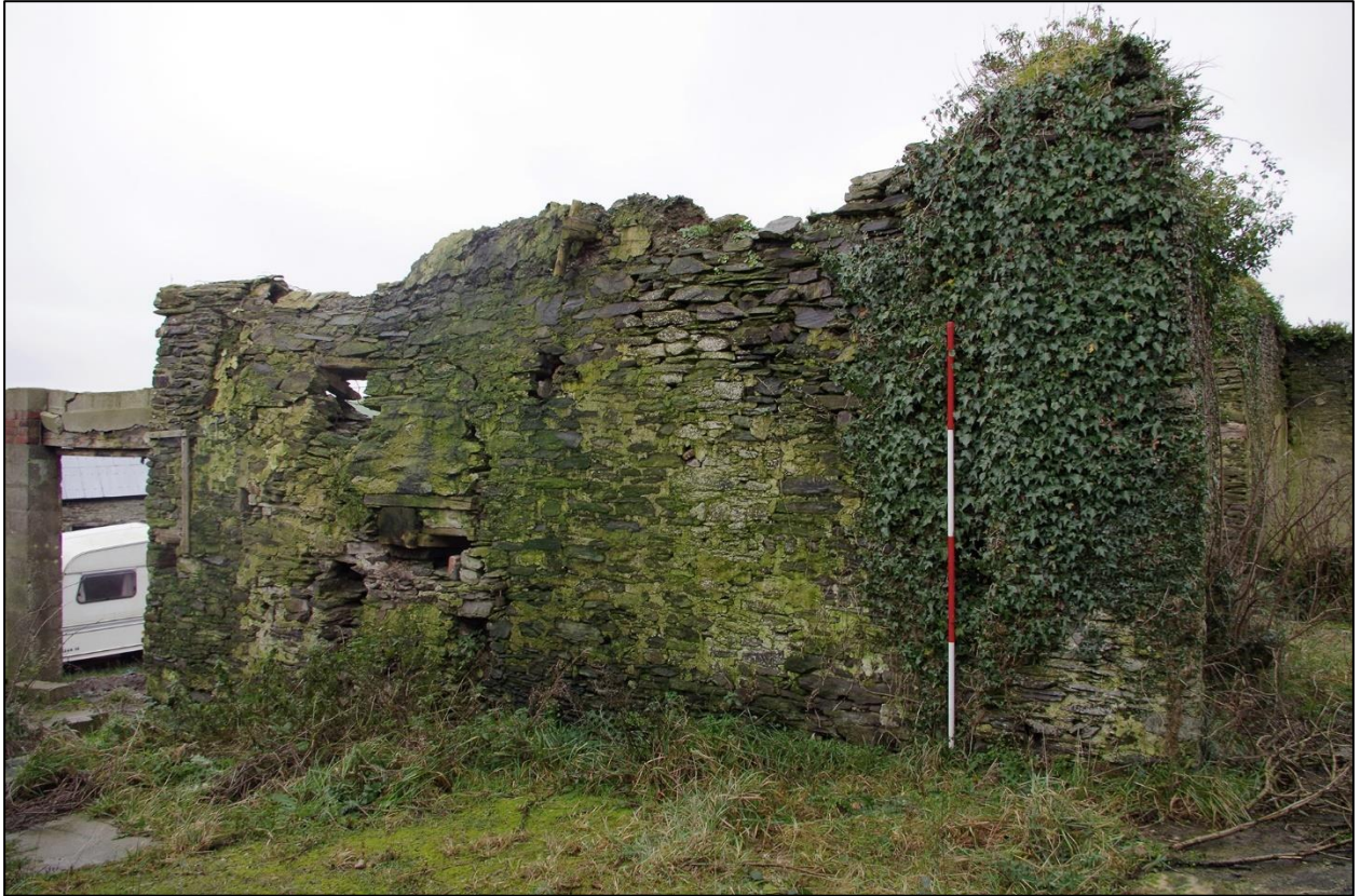
41. THE WESTERN INTERIOR WALL OF B2A. (WITH 2M SCALES). TAKEN FROM THE NORTH EAST.
