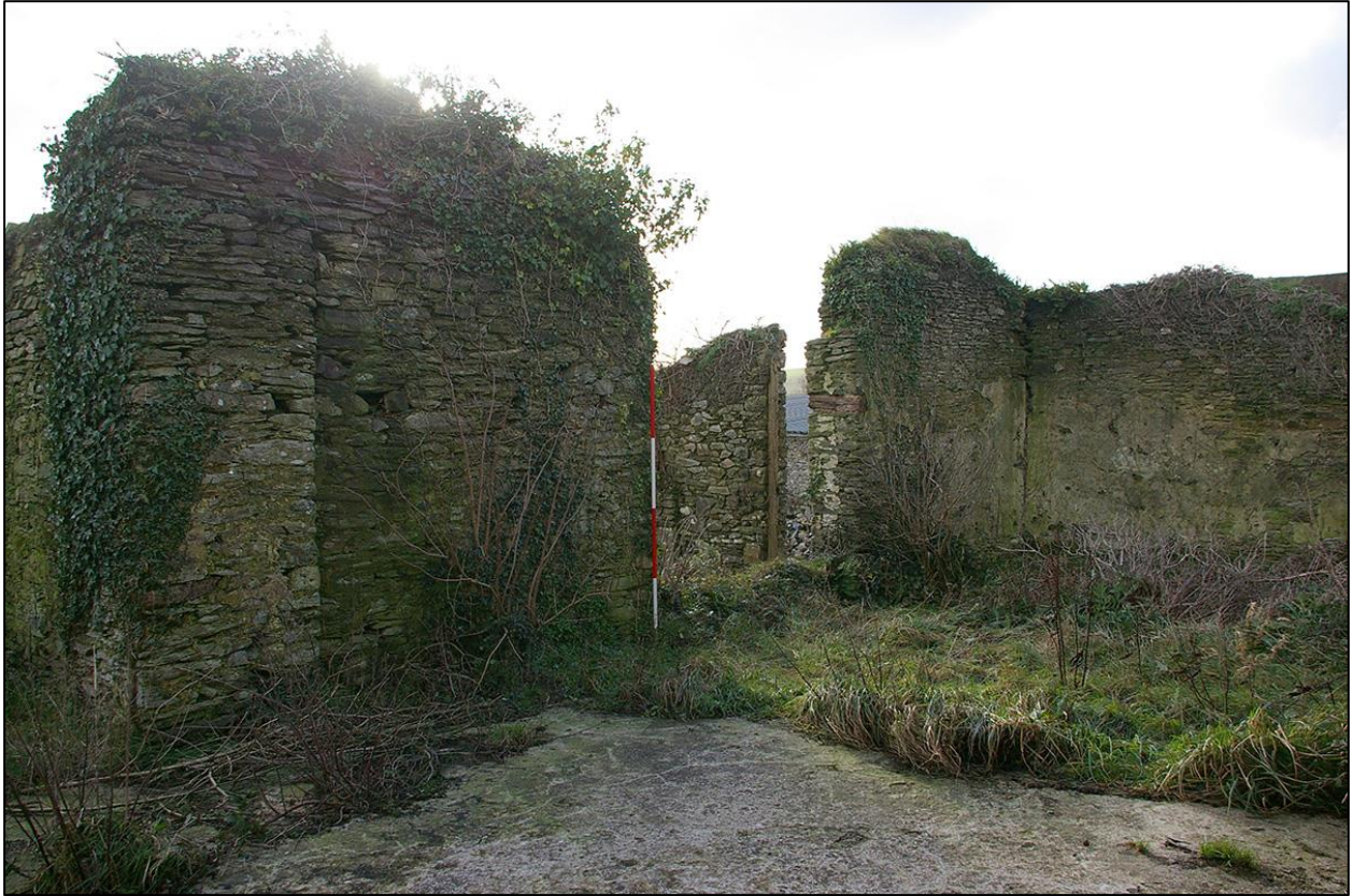
21. THE SOUTHERN WALL OF B2A; SHOWING THE STURCTURAL PILLAR ADDED LATER TO SUPPORT NEW ROOF FRAMES. (WITH 2M SCALES). TAKEN FROM THE NORTH NORTH WEST.
