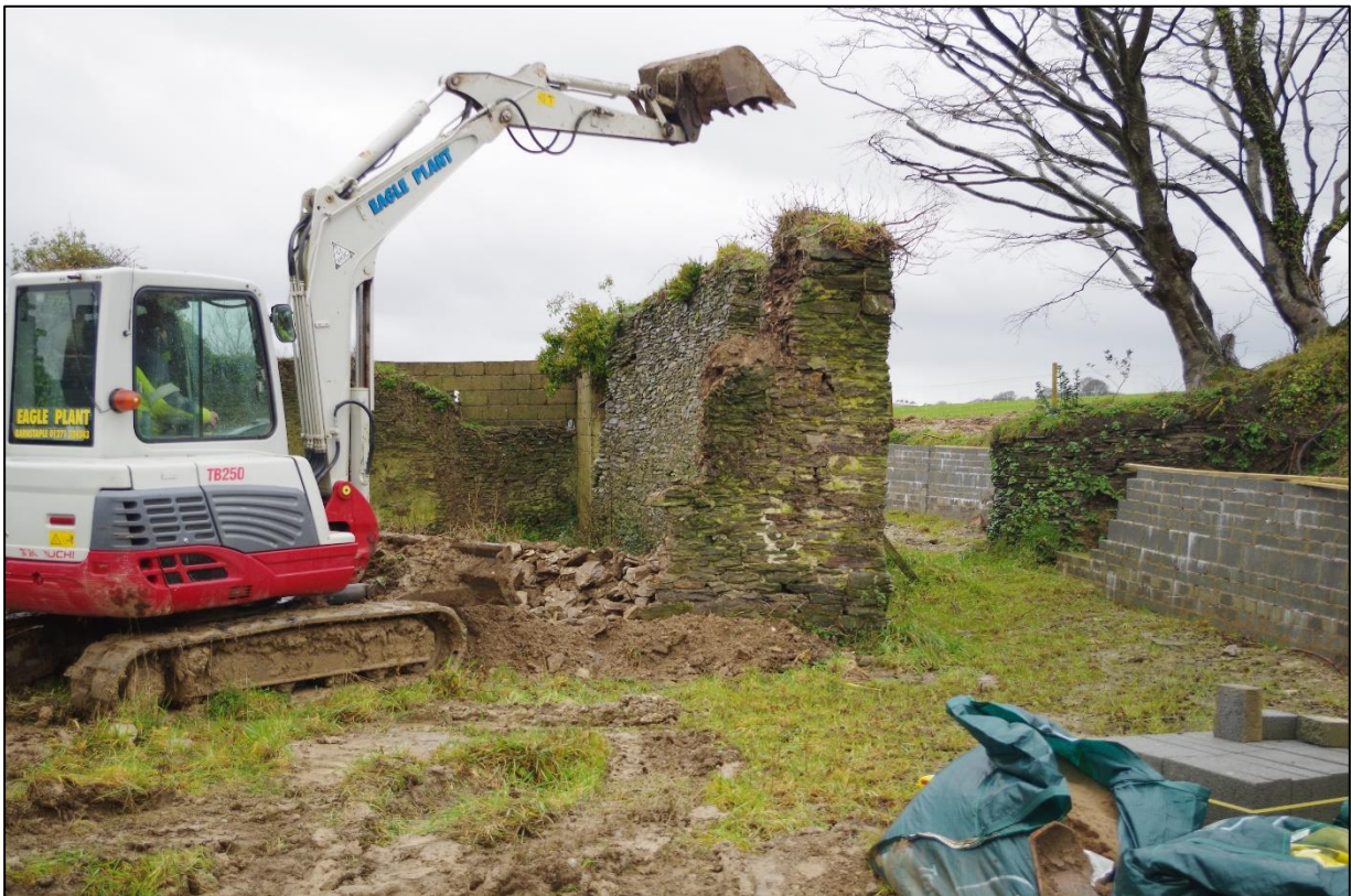
4. BEGINNING OF DEMOLITION WORKS ON THE EASTERN WALL OF B2A. TAKEN FROM THE EAST.
