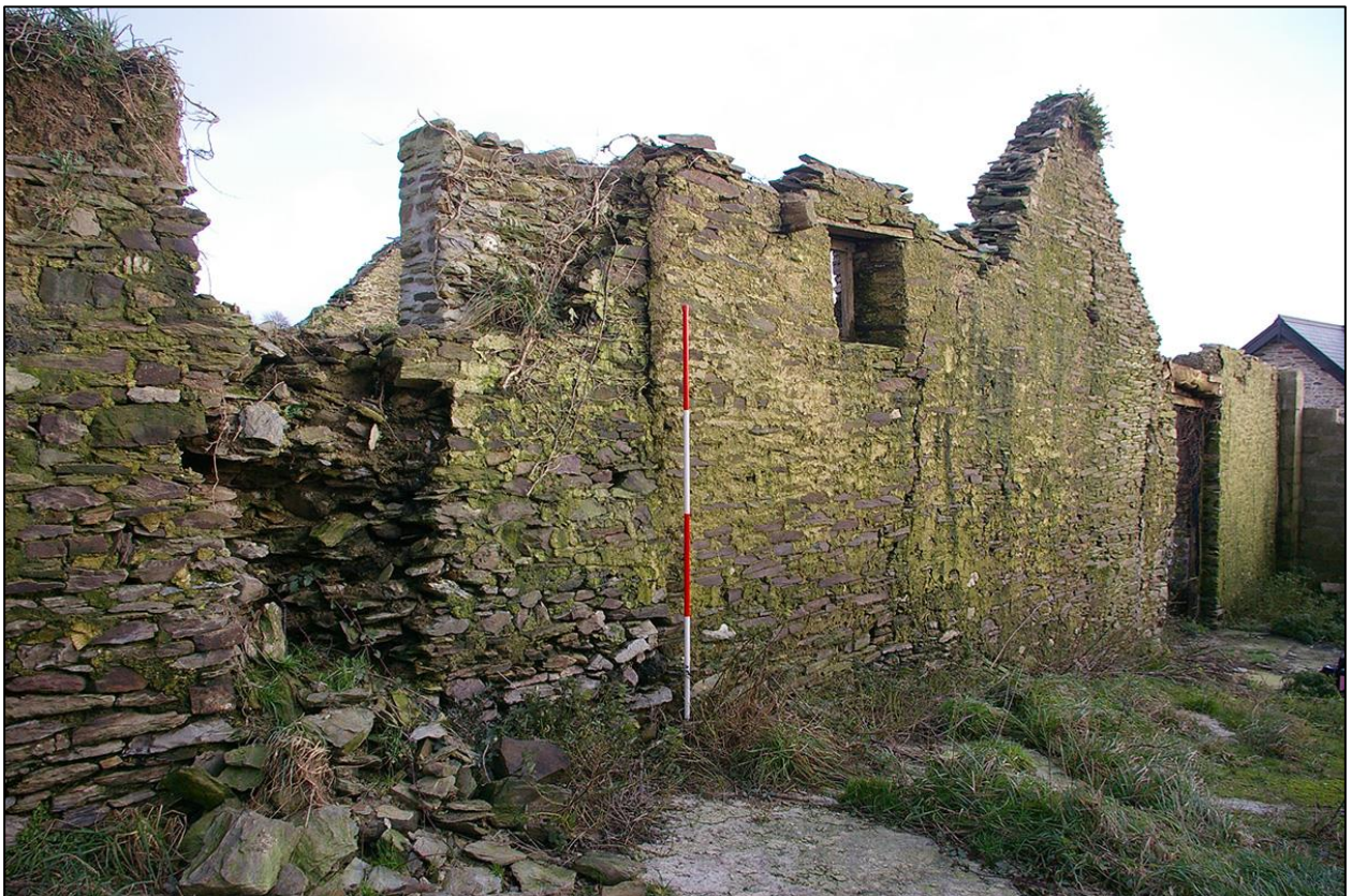
30. B2A LOOKING DOWN TOWARDS B2B AND SHOWING THE GABLED END OF THE STABLES B4. (WITH 2M SCALES). FROM THE NORTH WEST.
