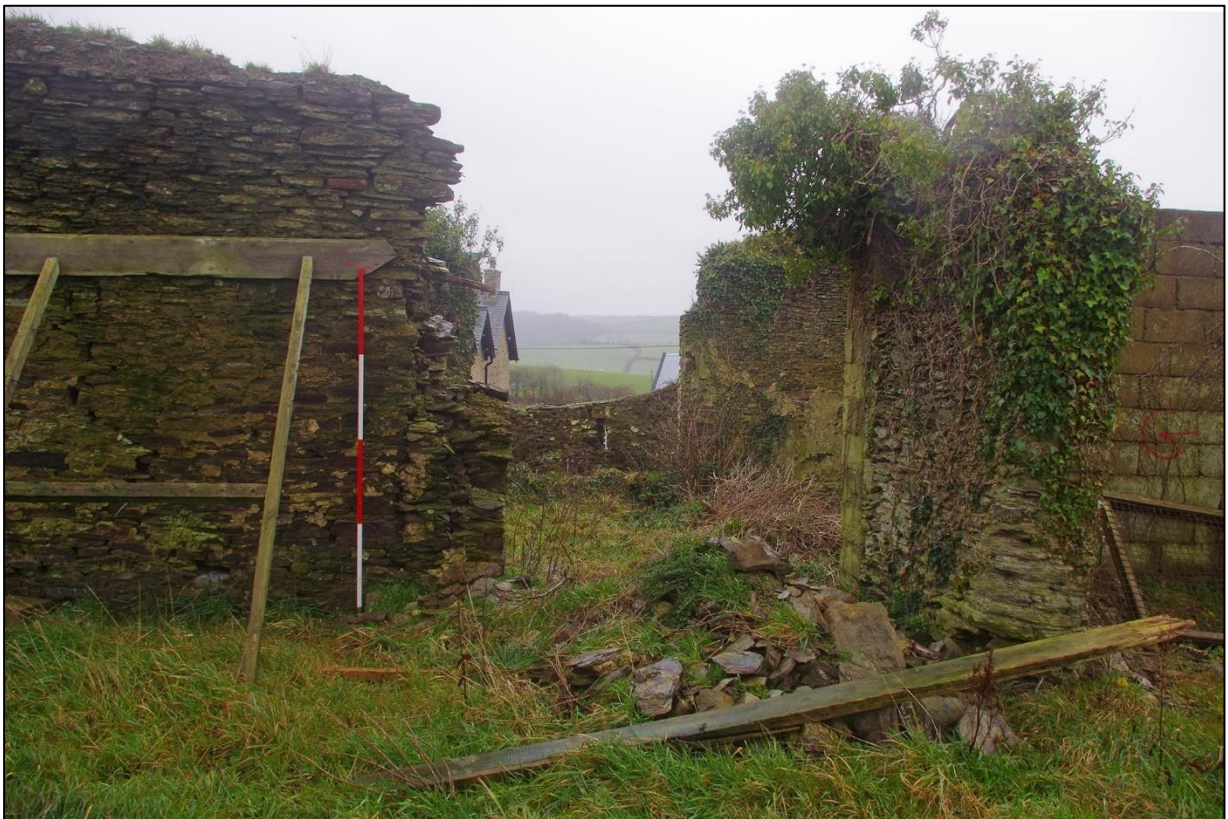
13. BUILDING 2A; LOOKING AT THE NORTHERN OUTER WALL (WITH 2M SCALES). TAKEN FROM THE NORTH.
