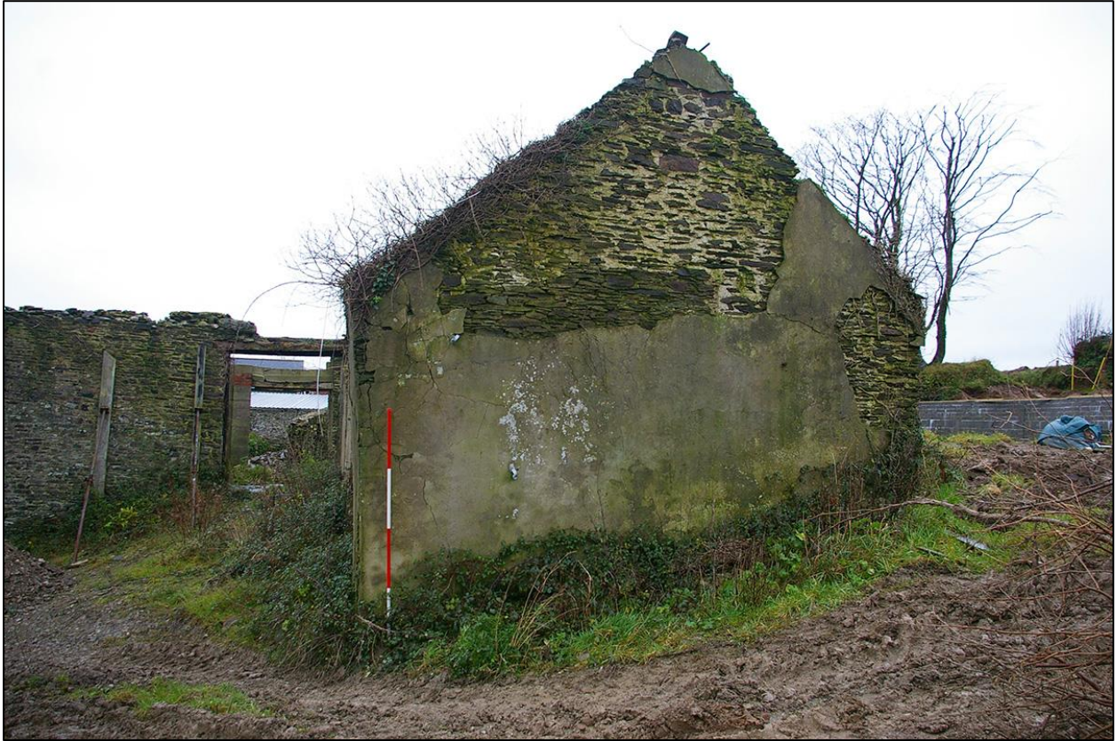
59. THE PLASTERED EASTERN GABLED END OF THE STABLES. (WITH 2M SCALES). TAKEN FROM THE EAST.
