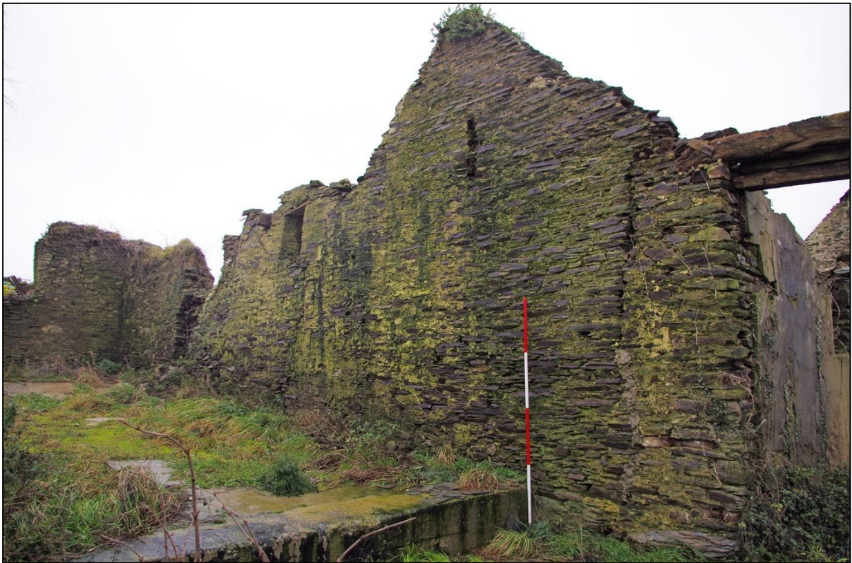
32. VIEW OF B4 THE STABLES AND THE STEP ONTO THE FORMER THRESHING FLOOR. (WITH 2M SCALES). FROM THE SOUTH WEST.
