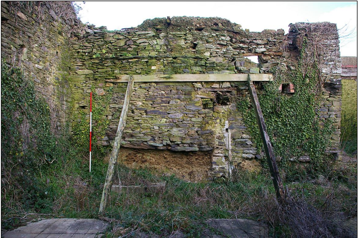
45. WESTERN FORMER EXTERIOR WALL OF B2b SHOWING WEATHERED SLATE RAIN COURSE AND THE BEDROCK FOUNDATIONS. TAKEN FROM THE WEST.
