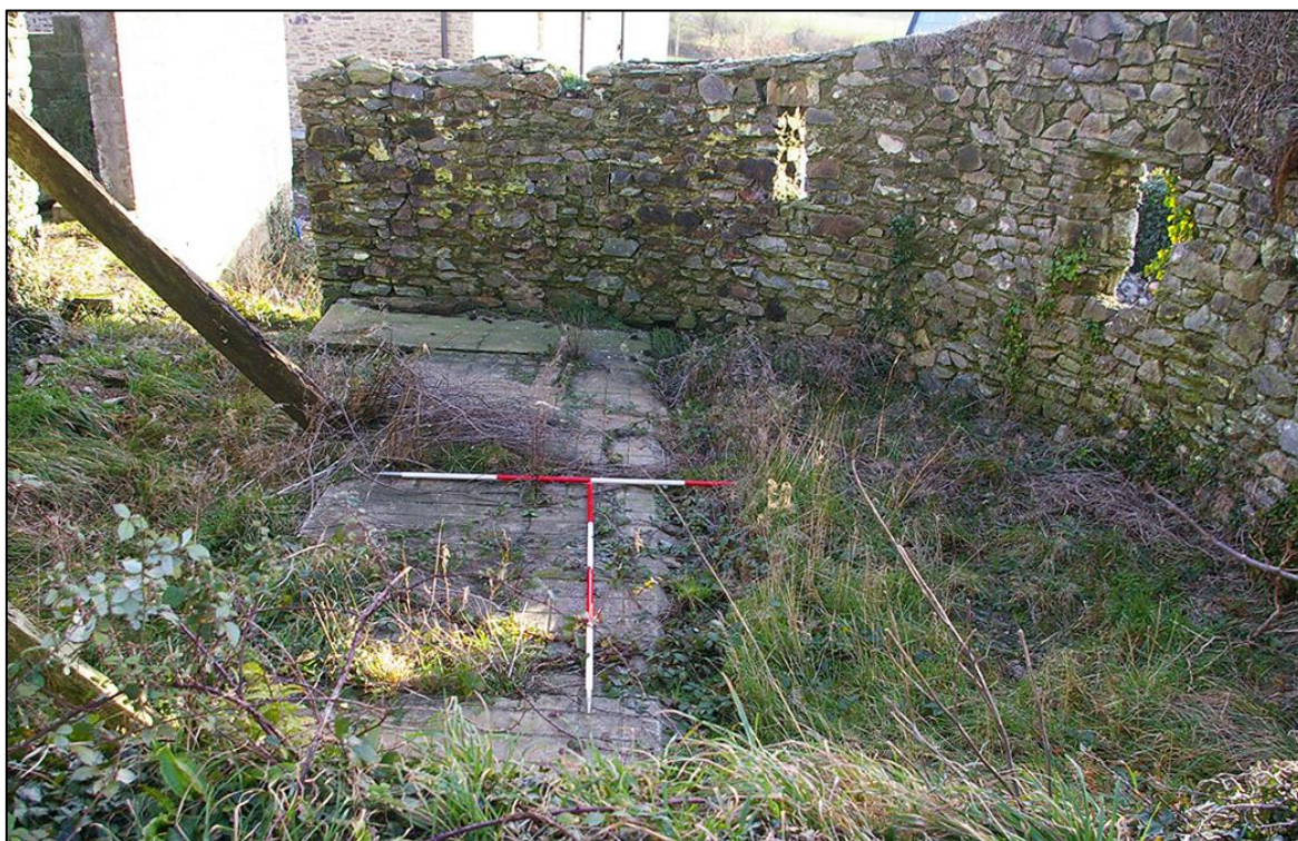
FIGURE 15: B3, VIEWED FROM ABOVE, FROM THE THRESHING DOOR OF B2A, SHOWING THE CURVING OUTER SOUTH WALL; FORM THE NORTH (WITH 2M SCALES).
