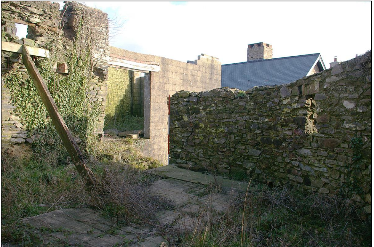
57. INSIDE B3 SHOWING THE MACHINE FLOORS AND GULLEYS; LOOKING INTO B2B. (WITH 2M SCALES). TAKEN FROM THE EAST.
