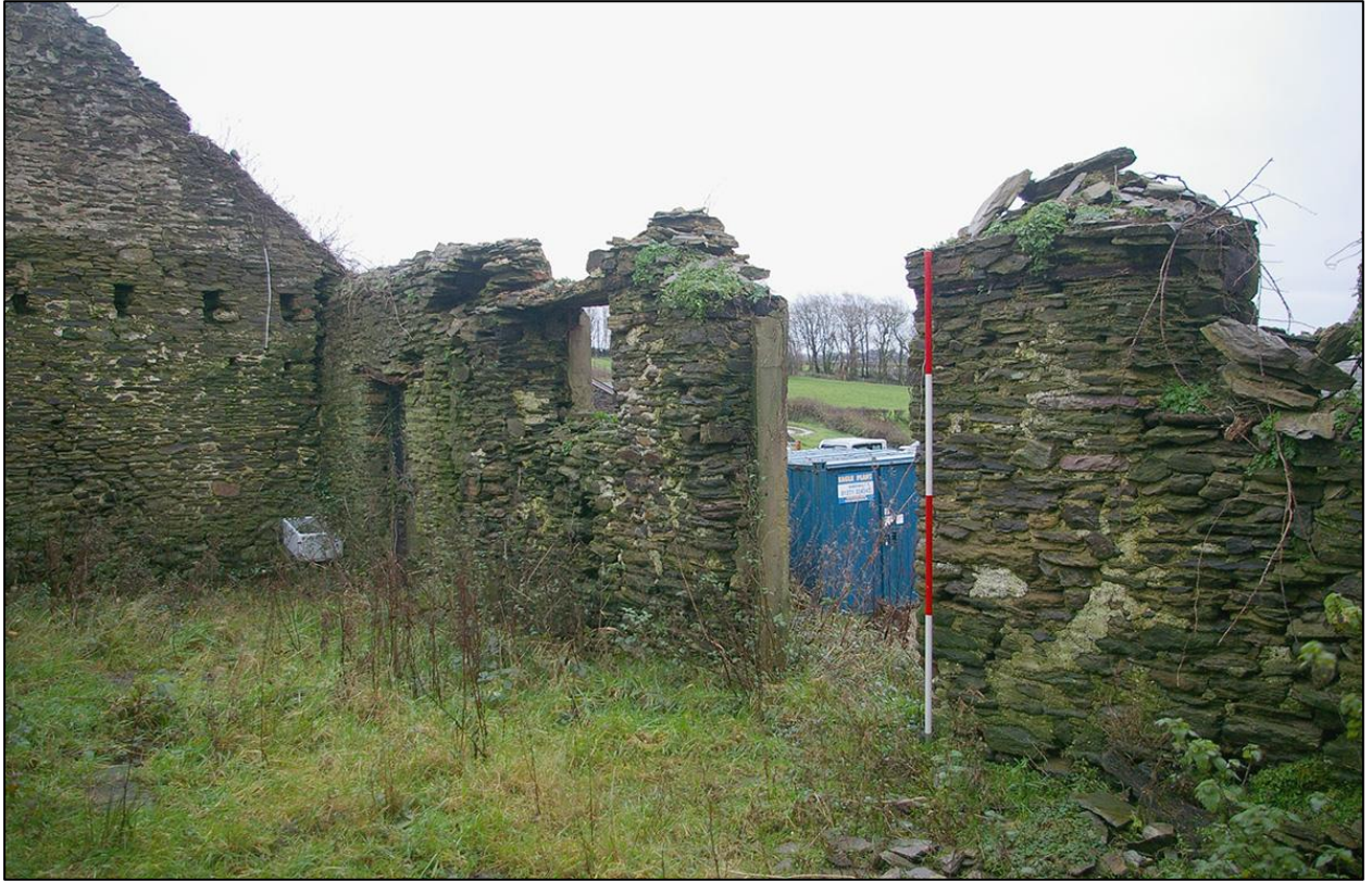
65. EASTERN GABLED END OF B4 SHOWING DOORWAYS AND WINDOW OPENINGS. (WITH 2M SCALES). TAKEN FROM THE WEST.
