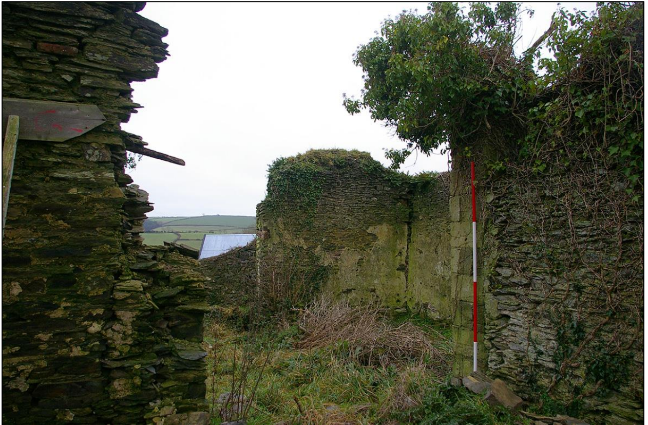
12. BUILDING 2A; SOUTH WESTERN CORNER, LOOKING DOWN THE OUTER WALL (WITH 2M SCALES). TAKEN FROM THE WEST.
