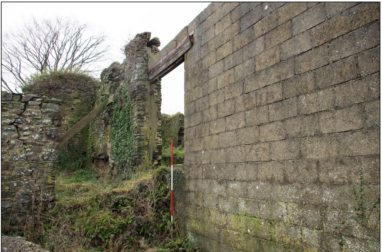
46. THE LATER ADJUSTED WESTERN CONCRETE BLOCK EXTERIOR OF B2b, AND OPENING INTO B3. (WITH 2M SCALES). TAKEN FROM THE SOUTH.
