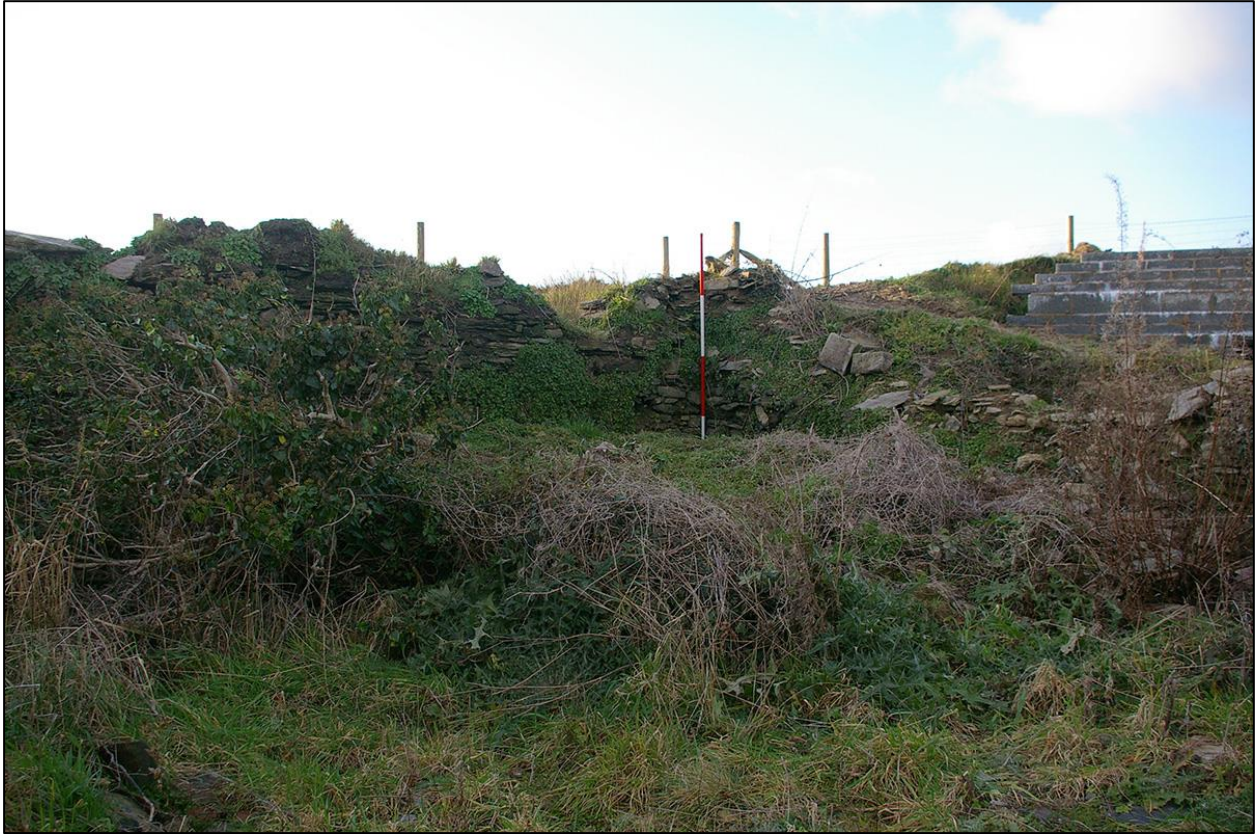
3. BUILDING 1 AND ITS RUINOUS WESTERN WALL, WITH COLLAPSED WINDOW OPENING. TAKEN FROM THE SOUTH EAST.
