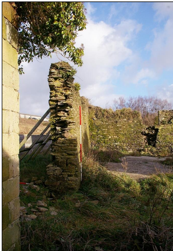
24. B2A NORTHERN WALL, SUPPORTED BY TIMBER FRAMES DUE TO ITS INSTABILITY. (WITH 2M SCALES). TAKEN FROM THE WEST.
