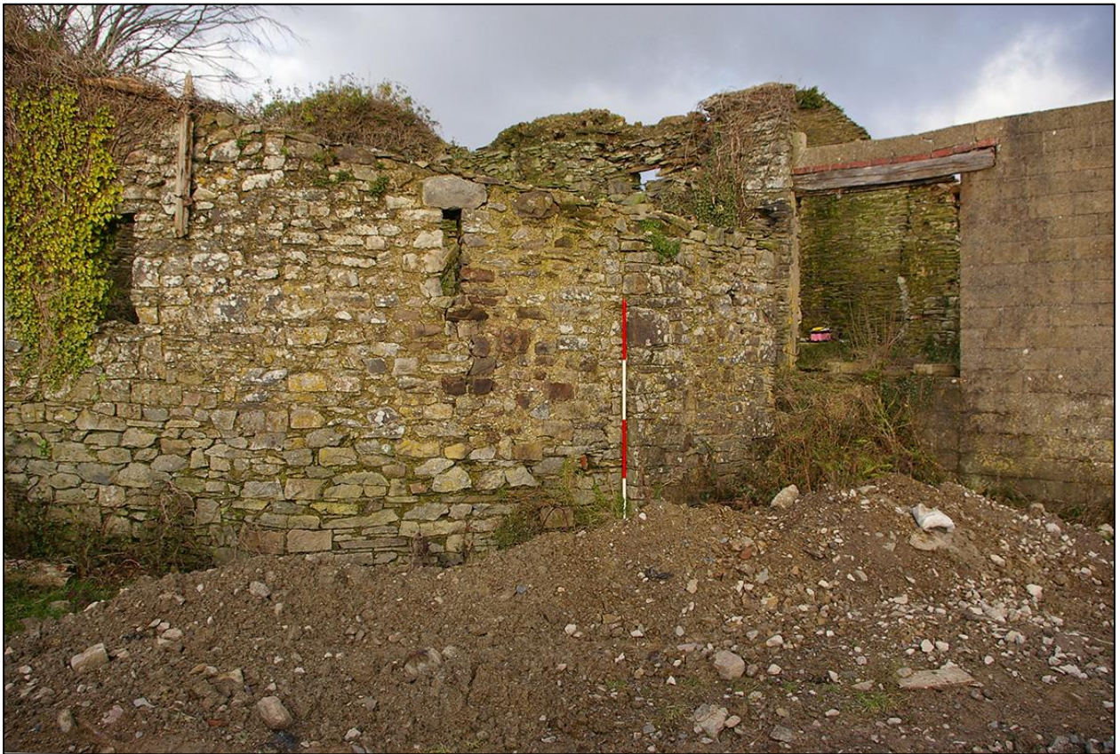
56. EXTERNAL WALLS OF B3 LOOKING IN TO B2B. (WITH 2M SCALES). TAKEN FROM THE SOUTH WEST.
