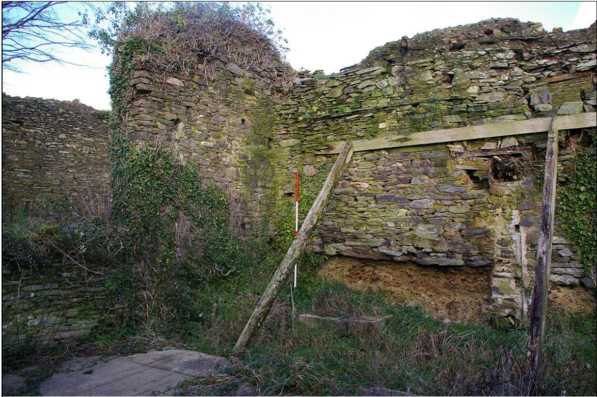
FIGURE 18: VIEW OF B2A AN 18 TH CENTURY THRESHING BARN, ABUTTING THE EARLIER HEAVY SLATE WALLING OF B2B, WITH SLAB WEATHERING COURSE; FROM THE SOUTH-WEST (2M SCALE).
