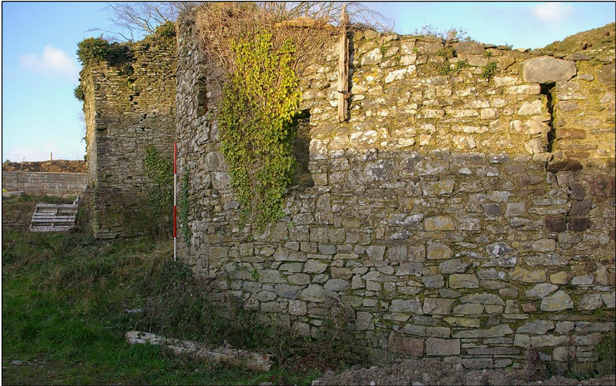
54. EXTERNAL WALLS OF B3 SHOWING THE SMALL WINDOWS. (WITH 2M SCALES). TAKEN FROM THE SOUTH.
