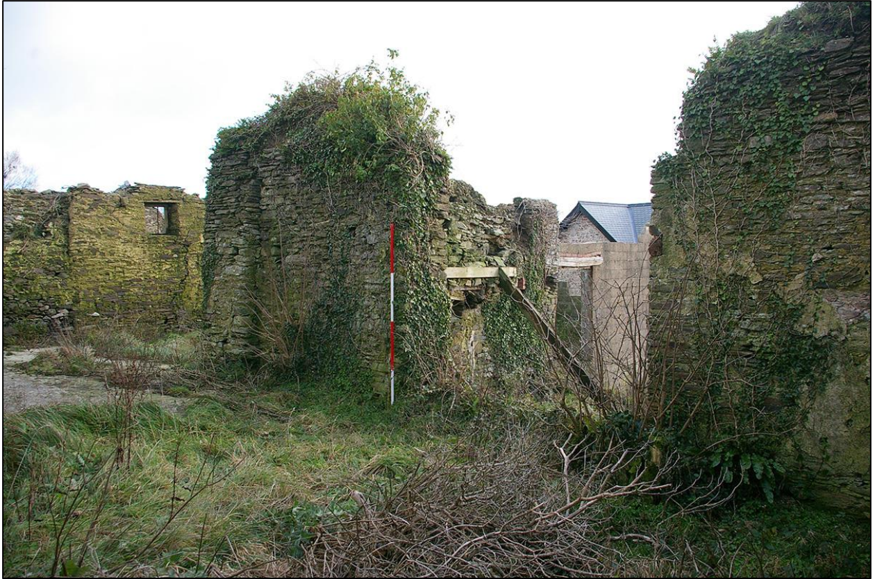
19. BUILDING 2A LOOKING INTO B3 AND FORCED OPENINGS FOR THRESHING (WITH 2M SCALES). TAKEN FROM THE SOUTH WEST.
