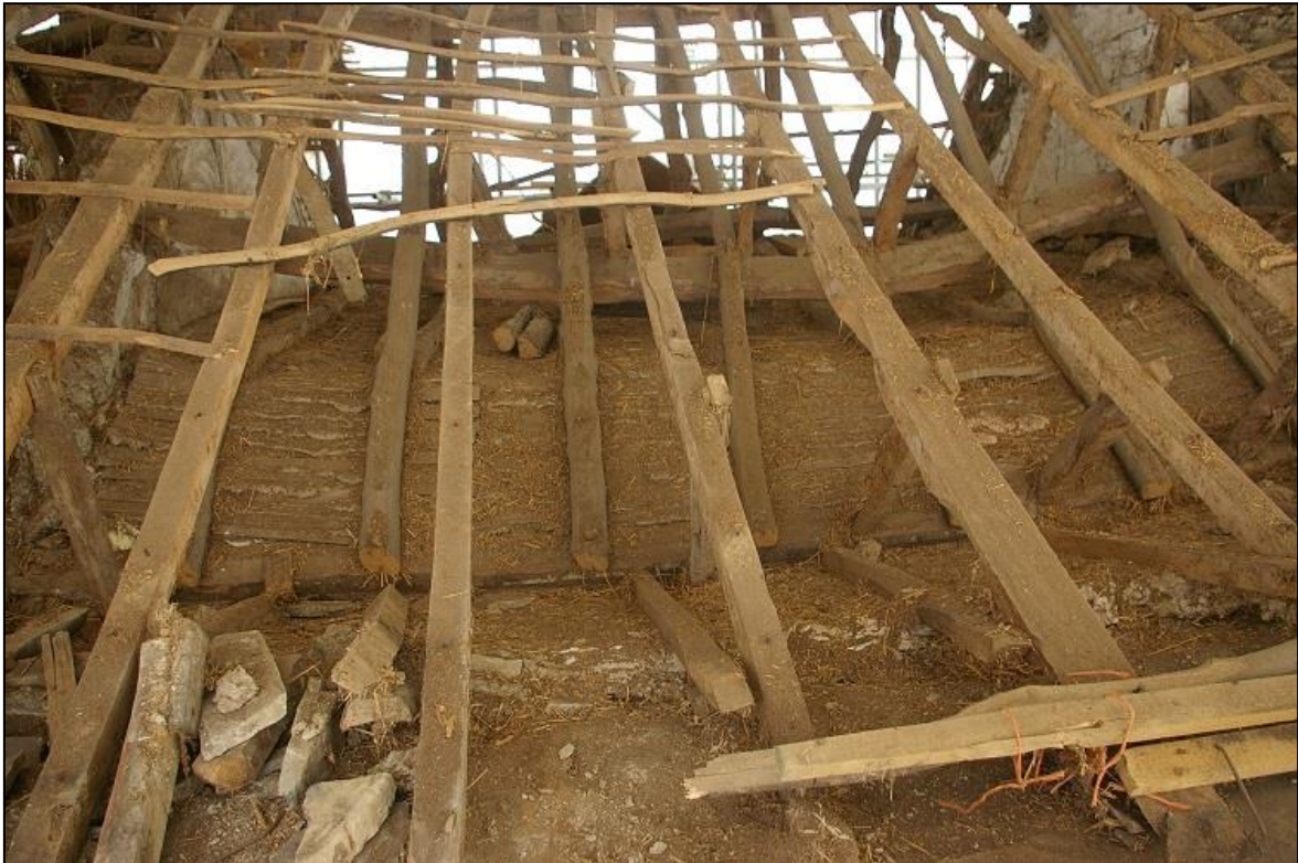
FIGURE 9: BAY 4 OF THE ROOF, WHICH HAS RETAINED ITS 17 TH CENTURY INSERTED VAULT AND PLASTER FRIEZE, AS CAN BE SEEN THE CHAMBER WAS ORIGINALLY OPEN TO THE ROOF, HENCE THE PLASTERED AND PAINTED APEXES; FROM THE SOUTH.
