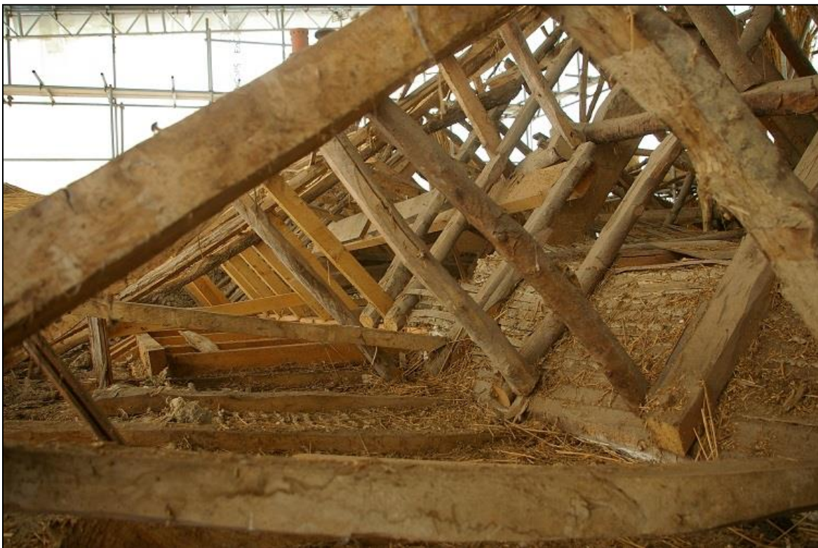
53. VIEW ALONG BAY 3-1 OF THE ROOF, FROM THE EAST END, SHOWING HOW THE LATER ROOF PROJECTS OUT TO THE RAISED FRONT WALL FROM THE OLDER ROOF LINE; FROM THE EAST-SOUTH-EAST.
