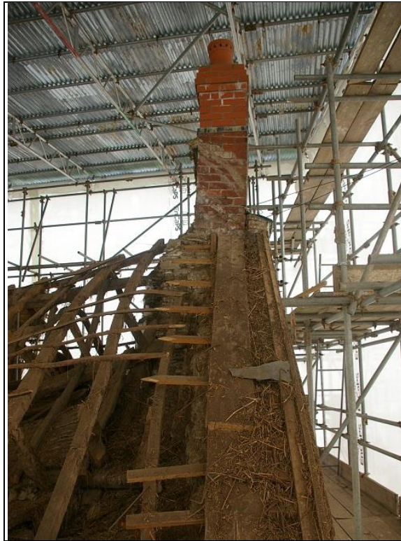
35. THE EASTERN GABLE END STACK, SHOWING THE SHAFT REBUILT IN THE POST MEDIEVAL PHASE, LIKELY THE 19 TH CENTURY, BUT THE UPPER SECTION AGAIN REPLACED IN THE LAST TEN YEARS; FROM THE SOUTH.
