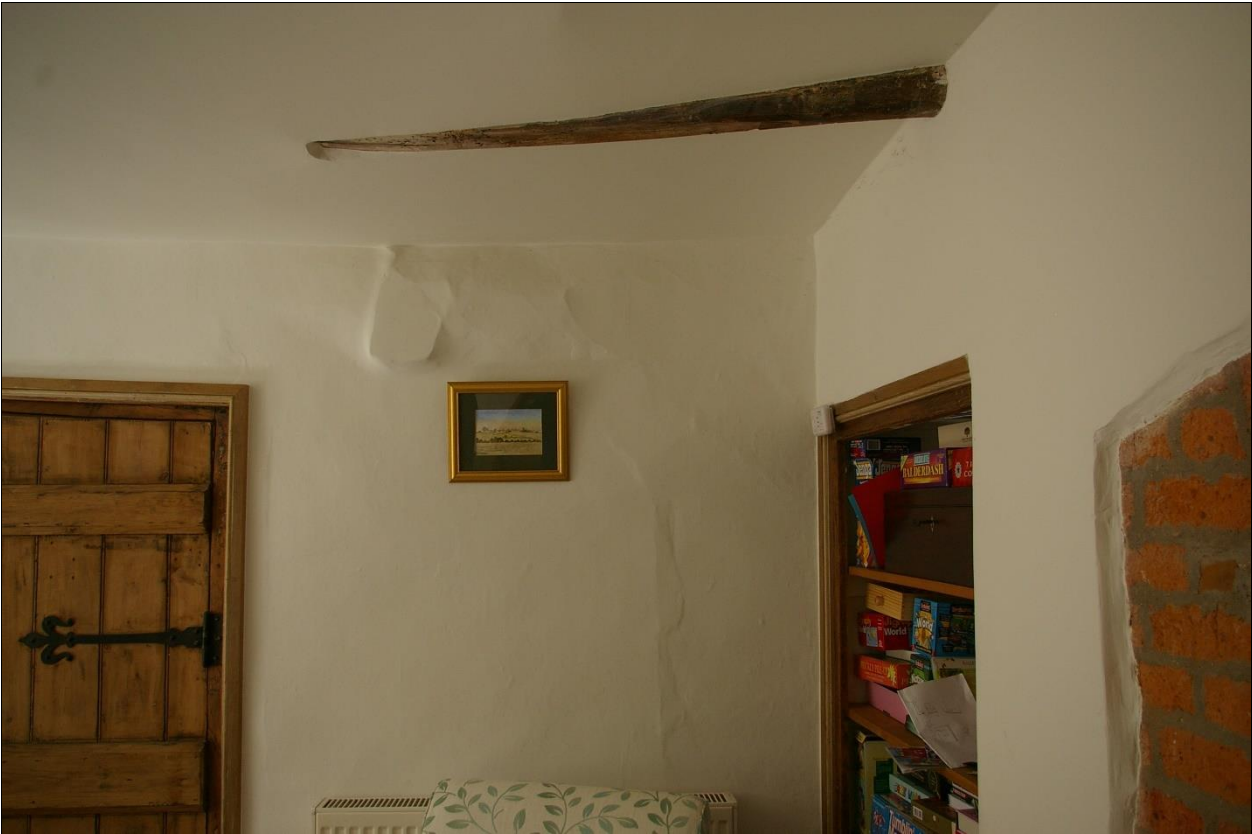
8. SCARRING SEEN IN THE WEST WALL OF ROOM 3, WITH TRUNCATED CEILING BEAM, ASSOCIATED WITH A BRACE TO THE CEILING AND A CHANGE IN FLOOR HEIGHT ON THE FIRST FLOOR, A STAIR (?) FROM THE FORMER OPEN HALL; FROM EAST.
