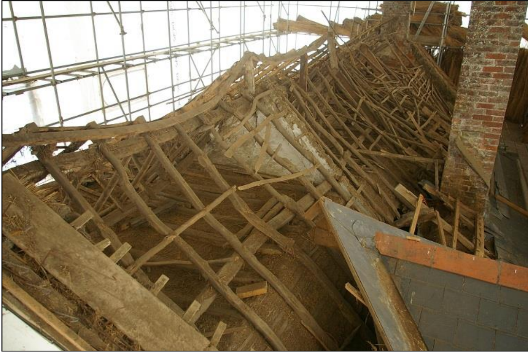
60. THE NORTH SIDE OF BAY 4; FROM THE EAST GABLE; FROM THE EAST-NORTH-EAST, SHOWING THE HIGHLY FRAGILE SUSPENDED VAULTED CEILING OVER ROOM 9.
