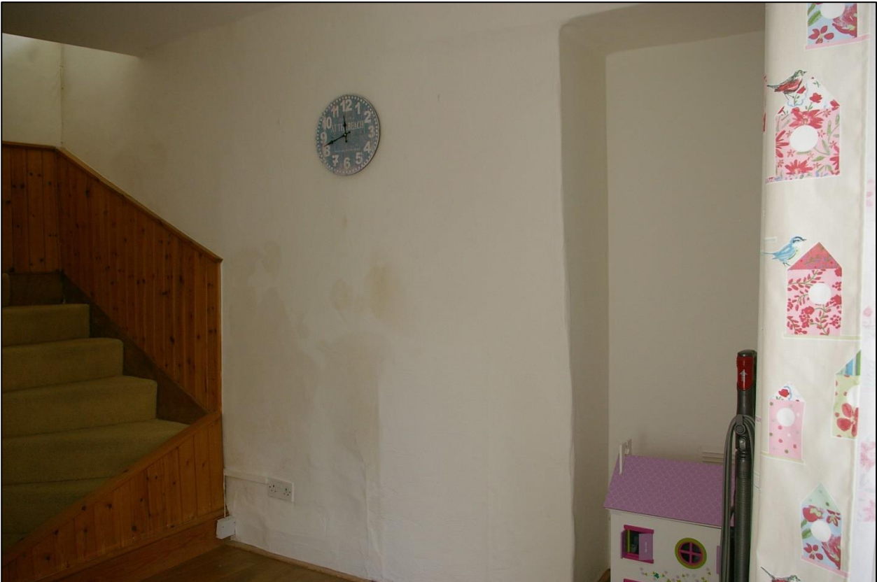
10. THE EAST GABLE STACK IN ROOM 4, WITH WINDER STAIR INSERTED TO THE NORTH END; FROM THE SOUTH-WEST.
