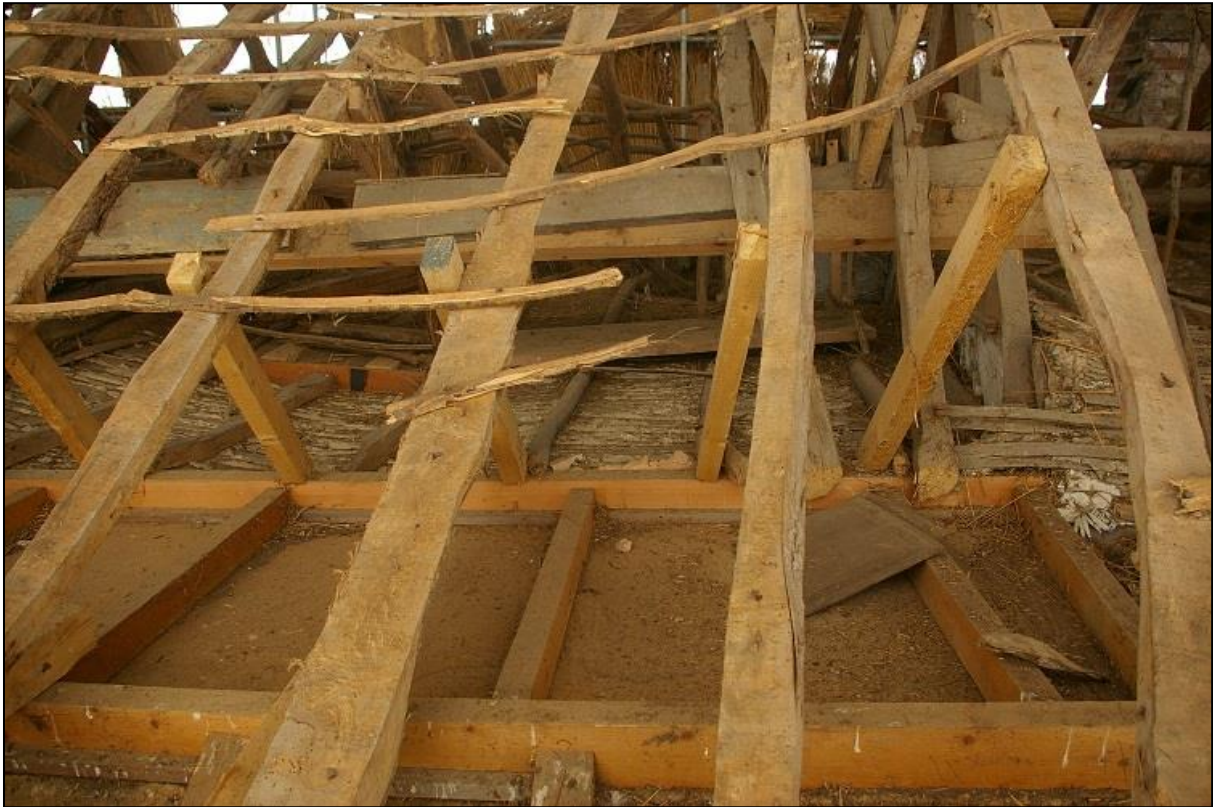
46. BAY 2 OF THE ROOF (TO THE CENTRE) FROM THE SOUTH, SHOWING A LATER FLAT CEILING.
