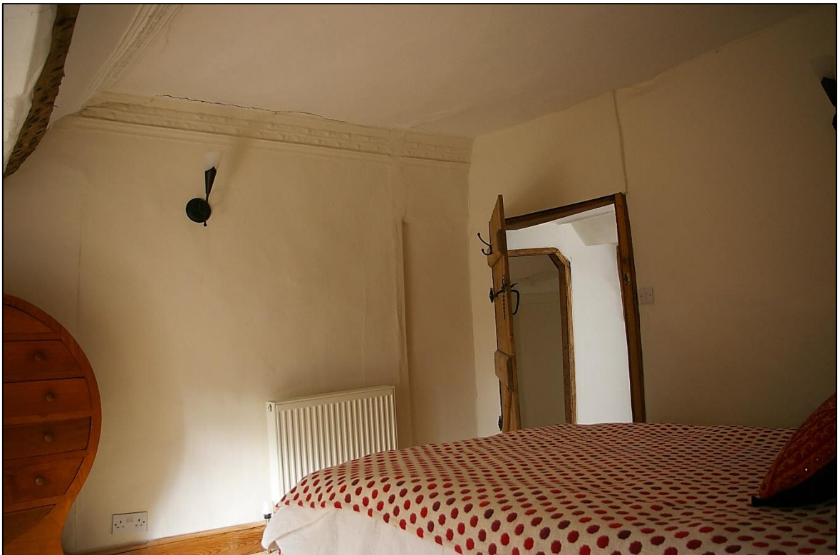
FIGURE 12: THE WEST WALL OF ROOM 9, WITH PLASTER CORNICE TRUNCATED BY THE COB PARTITION TO THE STAIRS AND WITH THE GOOD BLOCKED DOORWAY TO ROOM 12; FROM THE SOUTH-EAST.
