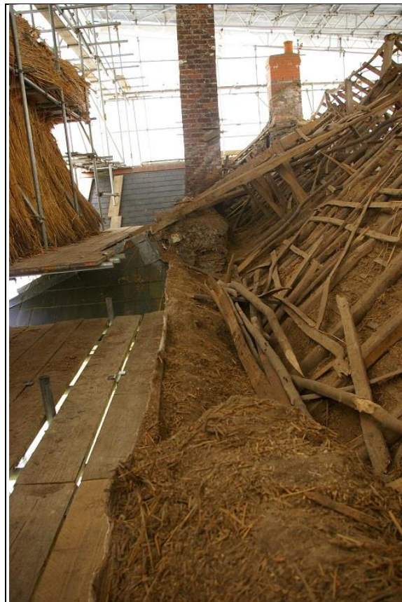
51. LOOKING ALONG THE NORTH SIDE OF THE ROOF, FROM THE WEST GABLE END, SHOWING THE PROFILE OF THE LATERAL STACK AND SMALL SURVIVING SECTION OF SECONDARY ROOF COVERING PROJECTING OVER THE RAISED COB WALL; FROM THE WEST.
