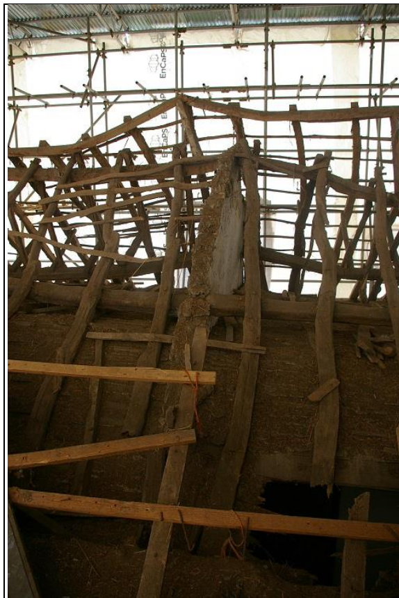
55. TRUSS 3 FROM THE NORTH, SHOWING IT PLASTERED OVER AND SEALED ON THE WEST FACE; FROM THE NORTH-NORTH-WEST.
