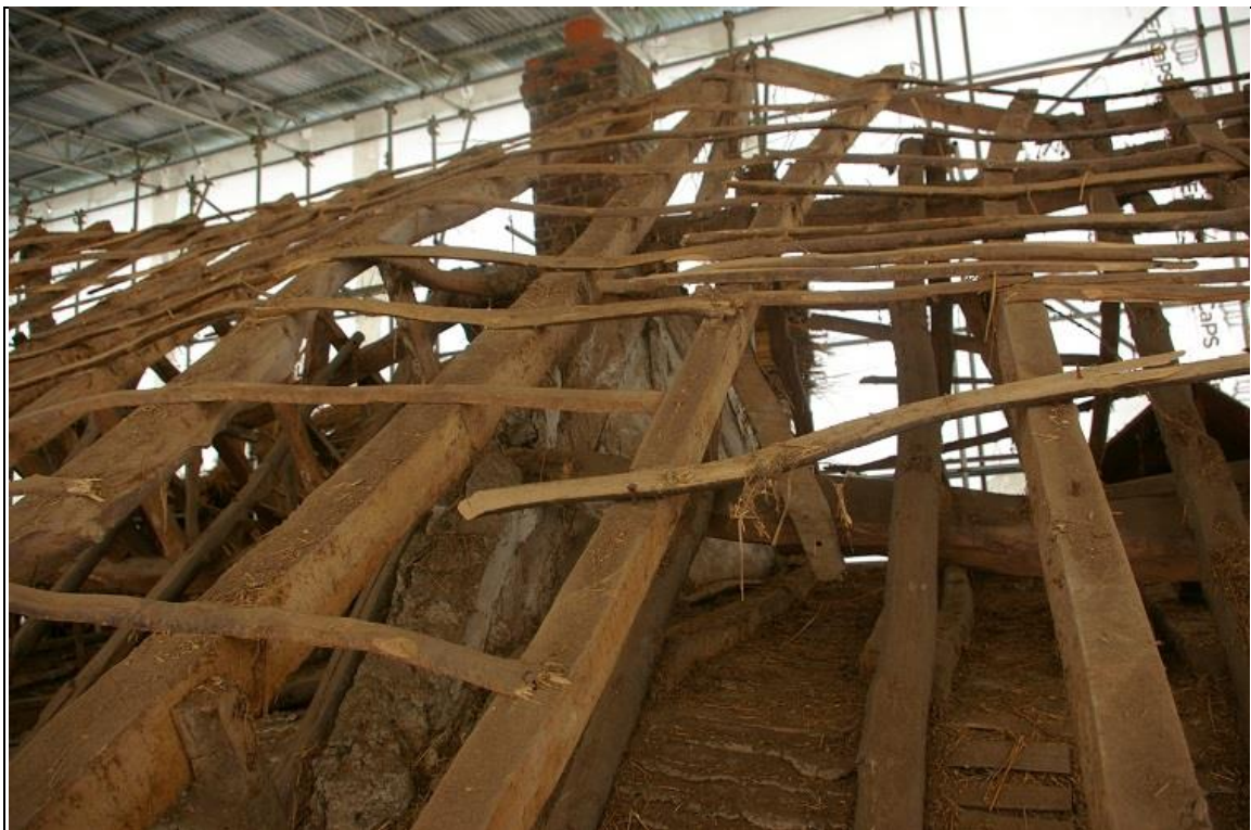
57. TRUSS 3 FROM SOUTH SIDE, THE EAST FACE; FORM THE SOUTH-SOUTH-EAST, SHOWING THE EXPOSED TIMBERS WHITEWASHED AND THE INFILL PARTITION SEALING THE APEX, SUPPORTED ON A KINGPOST CENTRAL POST/BRACE.
