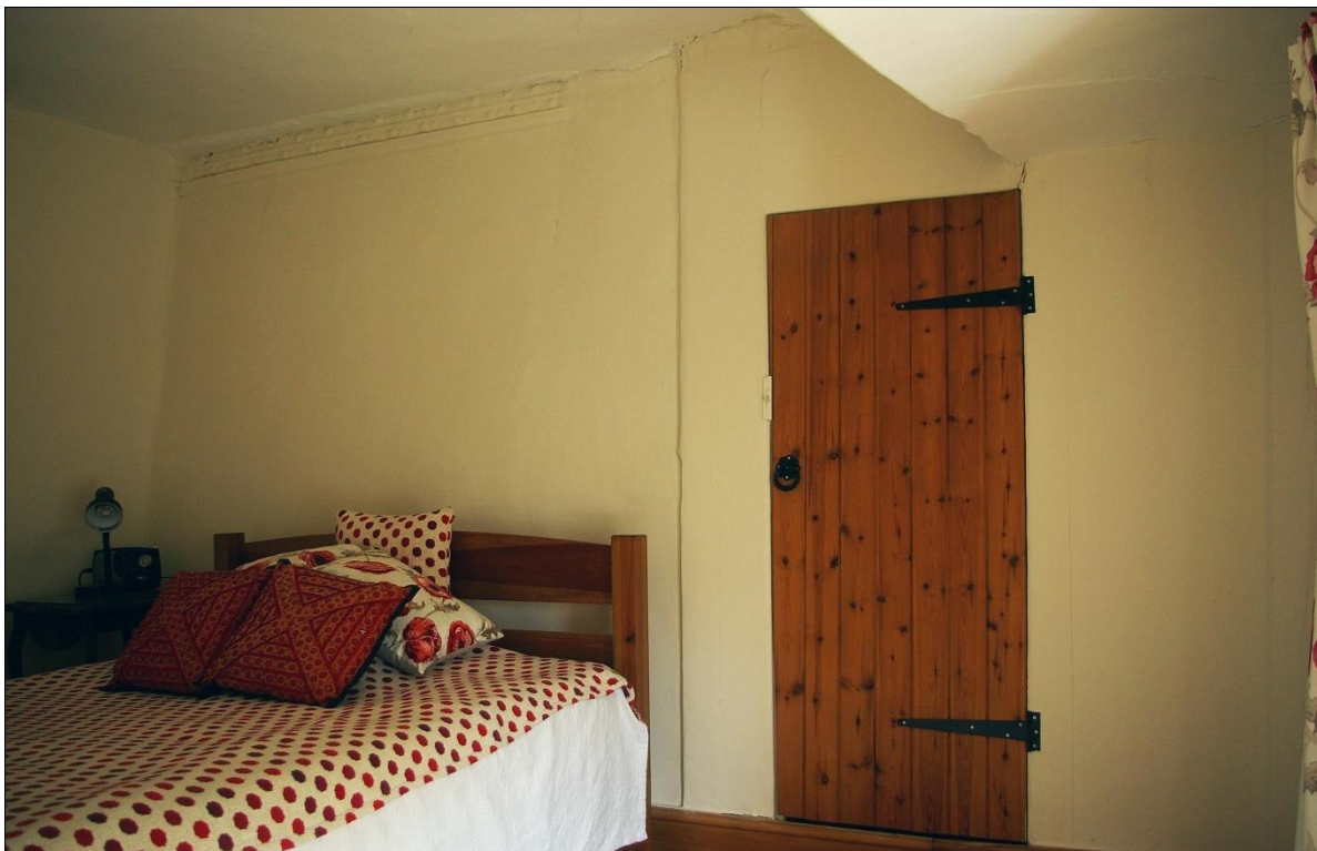
20. THE EAST WALL OF ROOM 9, WITH TRUNCATED CORNICE TO CUPBOARD AND TO COB PARTITION; FROM THE SOUTH-WEST.
