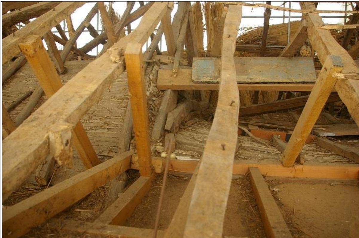
45. TRUSS 1, SHOWING IN DETAIL THE FACE PEGGED COLLARS AND DIFFERENCES IN HEIGHTS BETWEEN THE LATHE CEILINGS OF BAY 1 AND BAY 2: FROM THE SOUTH SIDE.
