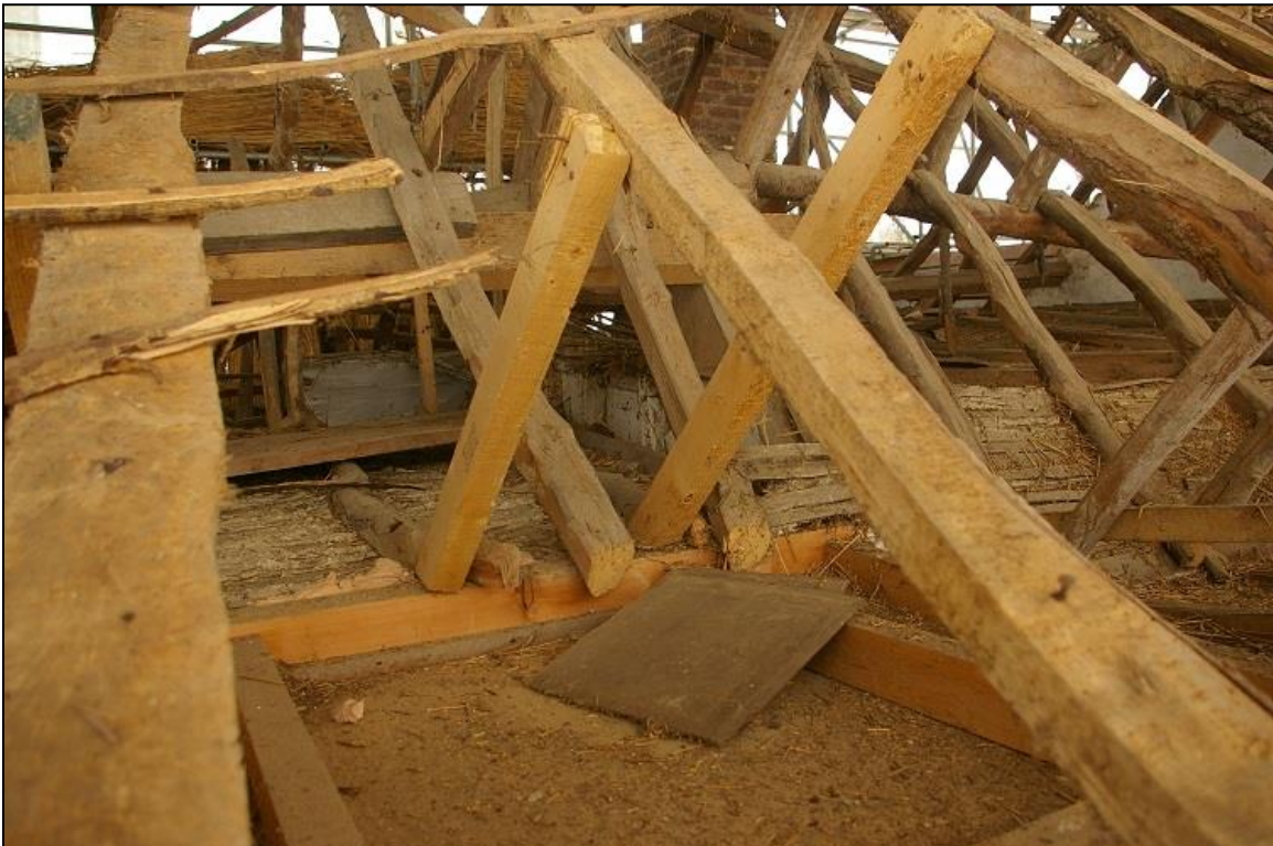
47. VIEW INTO THE ROOF OVER BAY 2, SHOWING THE WHITEWASH ON THE LOWER PART OF TRUSS 2 AND THE INFILL PARTITION, SUGGESTING A HIGHER PREVIOUS CEILING OVER BAY 2; FROM THE SOUTH-SOUTH-WEST.
