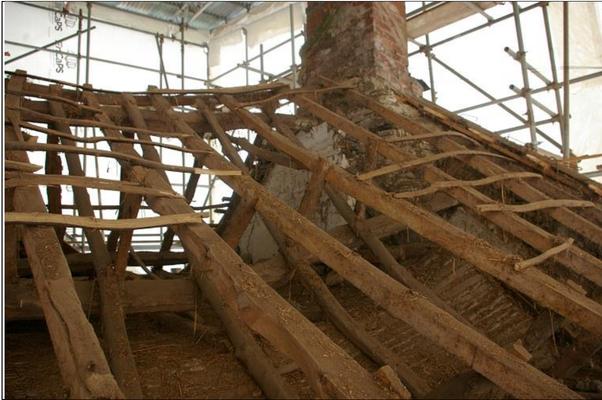
58. THE EAST GABLE STACK ADDED TO THE BUILDING RANGE, WITH PLASTERED APEX OF ORIGINAL TRUSS SURVIVING WITHIN THE BAY; FROM THE SOUTH SIDE OF THE ROOF; FORM THE SOUTH-WEST.
