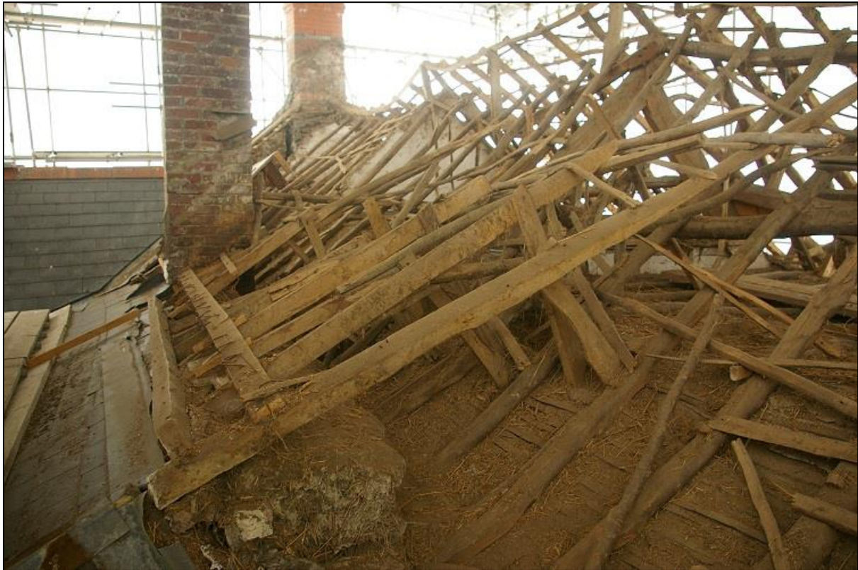
50. THE NORTH SIDE OF BAY 3, WITH THE REAR LATERAL STACK AND A SECTION OF SURVIVING LATER ROOF, PROJECTING OFF THE OLDER STICK RAFTERS; FROM THE WEST-NORTH-WEST.
