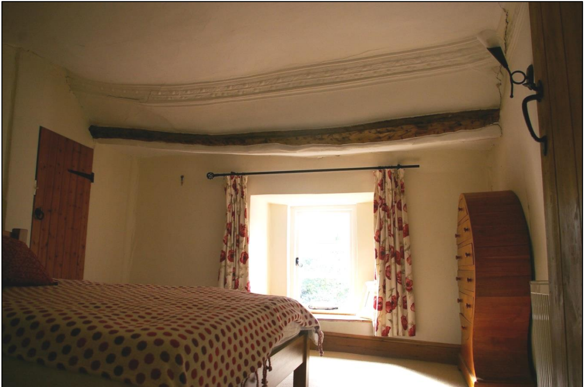
FIGURE 11: THE SOUTH WALL AND FAILING PURLIN AT THE EAVES IN ROOM 9, WITH FINE PLASTER CORNICE; FROM THE NORTH-WEST.
