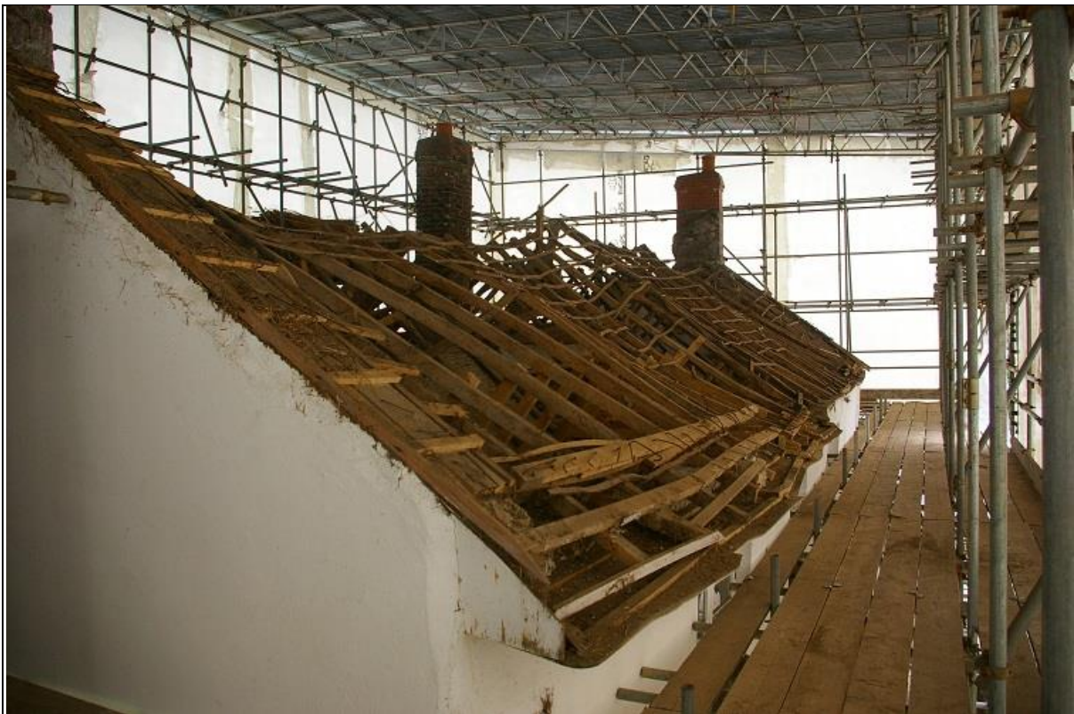
30. WESTACOMBE COTTAGE, WITH THE THATCH STRIPPED OFF; VIEWED FROM THE CORNER OF THE SCAFFOLDING; FROM THE WEST-SOUTH-WEST, SHOWING THE FRONT OF THE COTTAGE.
