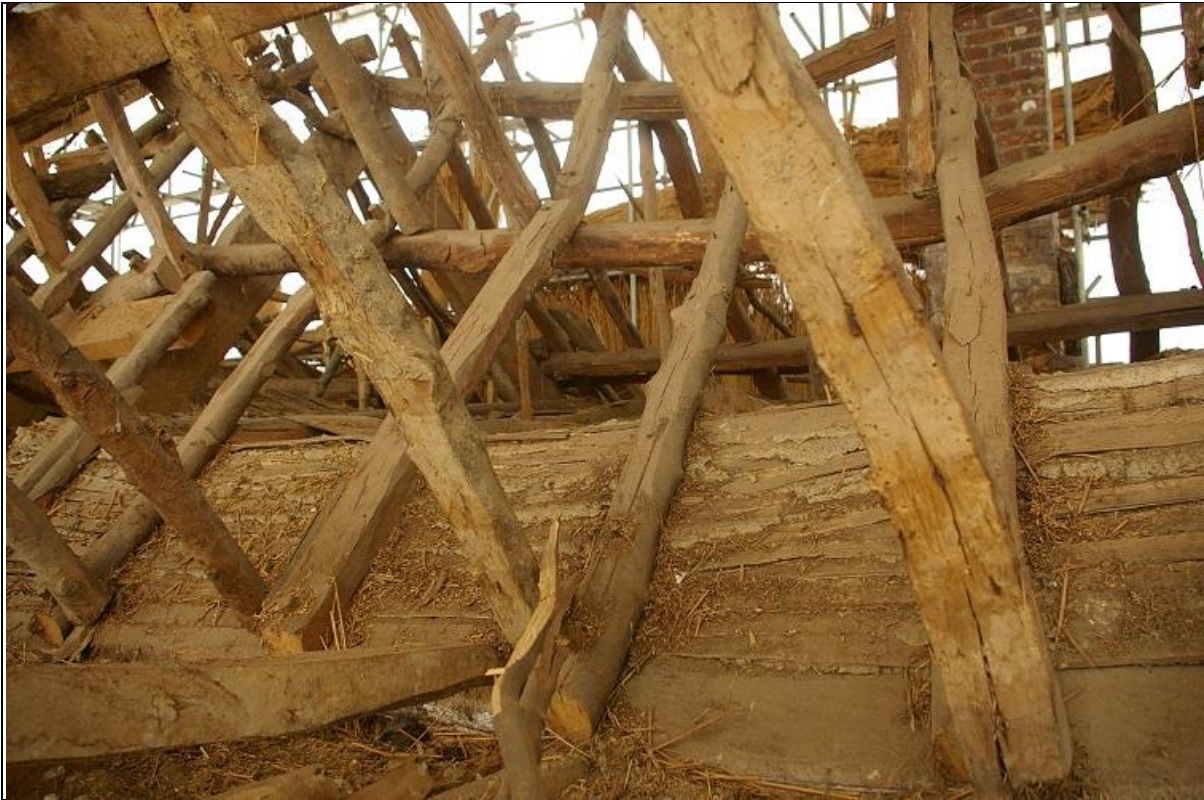
52. BAY 3, FROM THE SOUTH, PHOTO TAKEN FROM WITHIN THE ROOF, SHOWING THE STICK RAFTERS AND ROUGH PURLINS OF THE OLDER, INNER ROOF STRUCTURE; FROM THE SOUTH-EAST.
