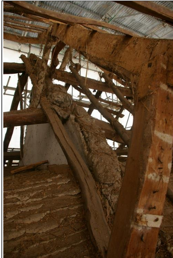
56. TRUSS 3; FROM THE SOUTH SIDE; FORM THE SOUTH-SOUTH-WEST SHOWING THE SEALED SIDE, COVERED BY LIME HAIR PLASTER, WITH COB BENEATH.
