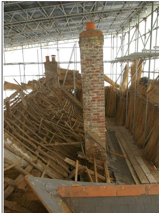
34. THE REAR LATERAL STACK, REBUILT IN POST-MEDIEVAL PHASE, LIKELY THE 19 TH CENTURY IN BRICK AND LIME MORTAR; FROM THE EAST.
