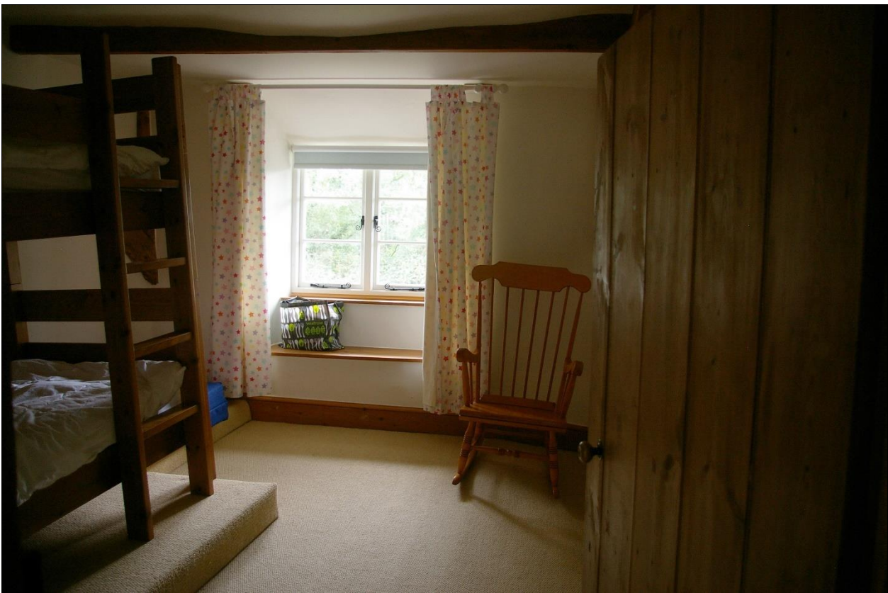
24. ROOM 13, WITH REPLACED PURLIN AND RAISED FLOOR OVER FORMER HALL AND POSSIBLE STAIR FABRIC, LEFT WITHIN CEILING VOID; FROM THE NORTH-NORTH-WEST.
