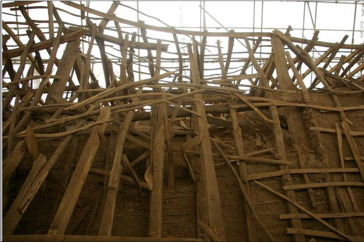
44. BAY 2 OF THE WESTACOMBE ROOF (IN THE CENTRE); FROM THE NORTH SIDE.
