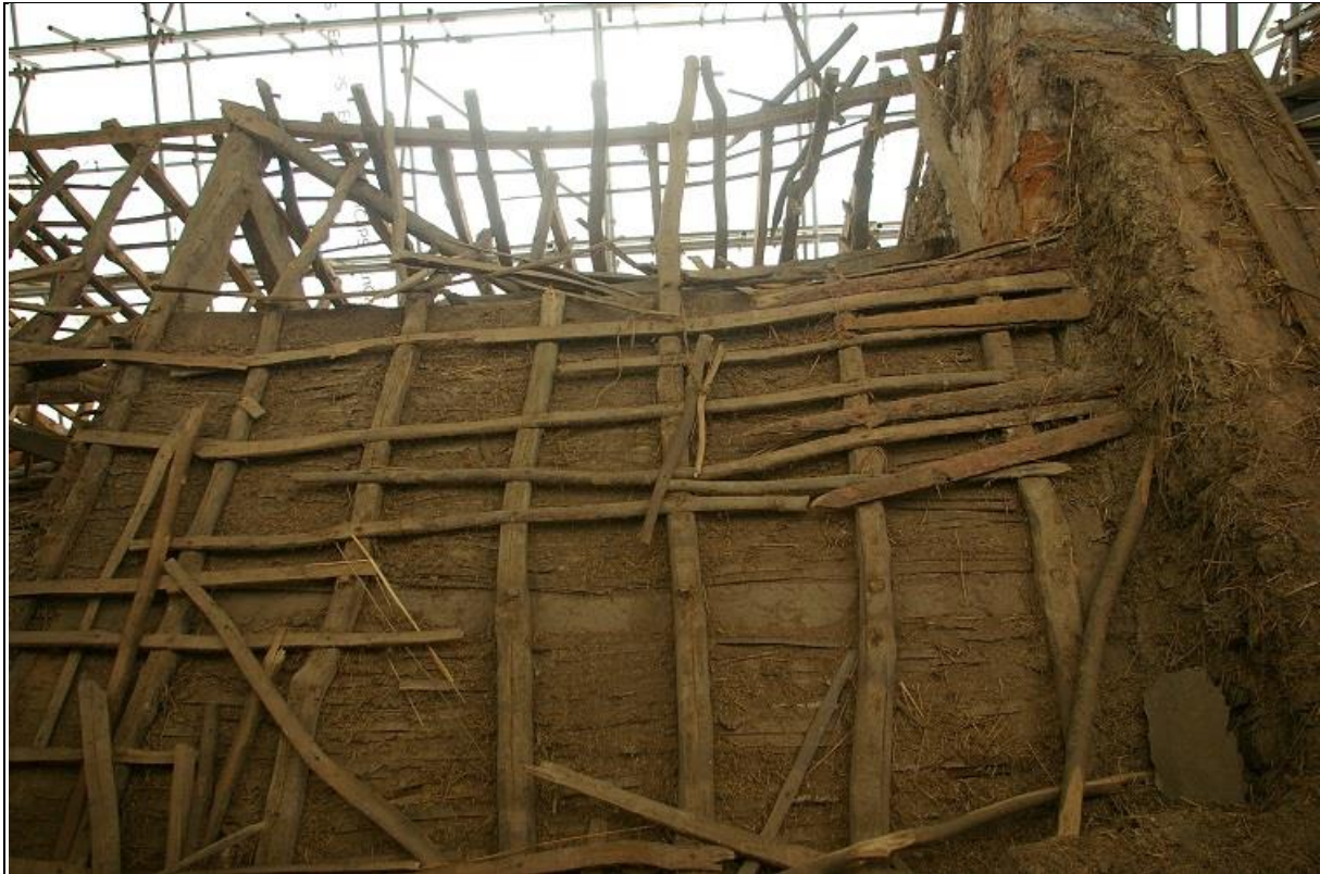
39. THE NORTH SIDE OF BAY 1 OF THE ROOF (AT THE WEST END); FROM THE NORTH.
