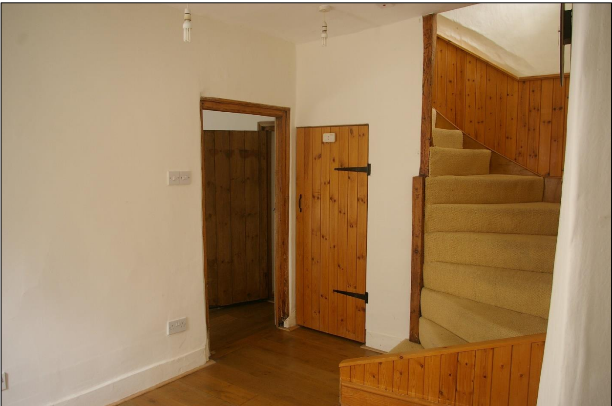
11. ROOM 4, THE THICK COB PARTITION AND WINDER STAIR, WITH BLOCKED DOORWAY BENEATH TO KITCHEN BLOCK; FROM THE SOUTH-EAST.
