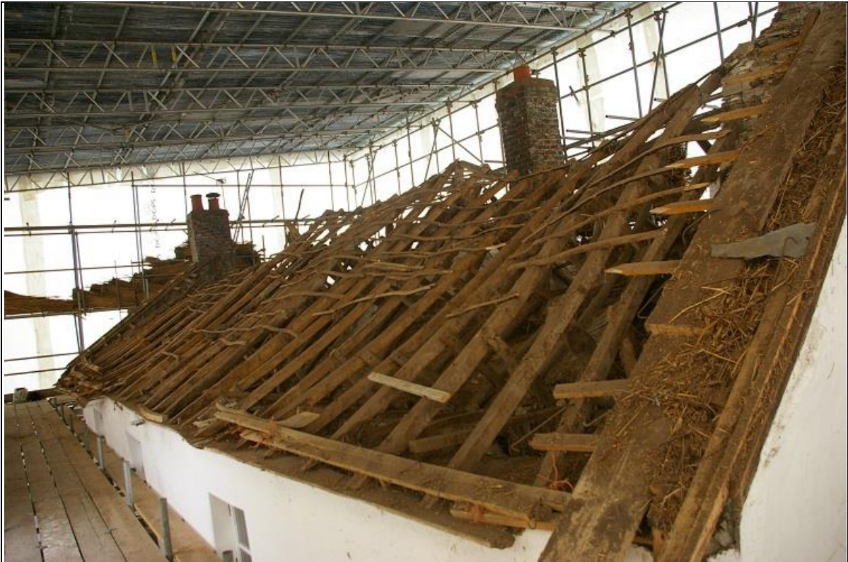
31. WESTACOMBE COTTAGE, WITH THE THATCH STRIPPED OFF; VIEWED FROM THE CORNER OF THE SCAFFOLDING; FROM THE EAST-SOUTH-EAST, SHOWING THE FRONT OF THE COTTAGE.
