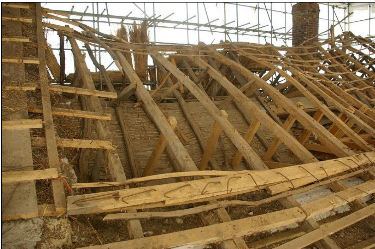
40. THE SOUTH SIDE OF BAY 1 (AT THE WEST END OF THE ROOF); FROM THE SOUTH-WEST.
