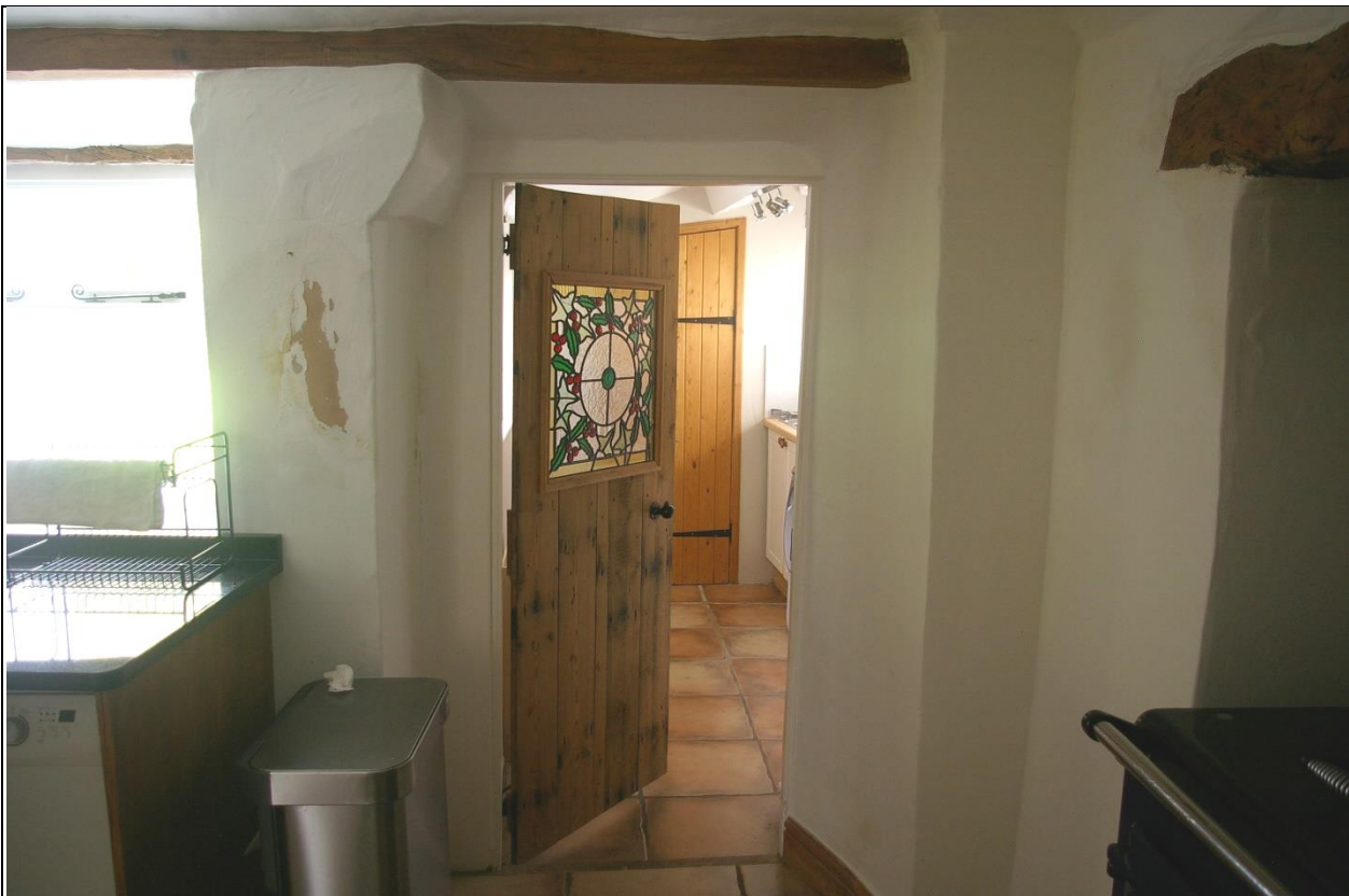
15. ROOM 5, LOOKING INTO ROOM 6, WITH LARGE FORCED OPENING AND INSERTED TIMBER LINTEL CARRIED ON CRUDE CORBEL; FROM THE SOUTH.
