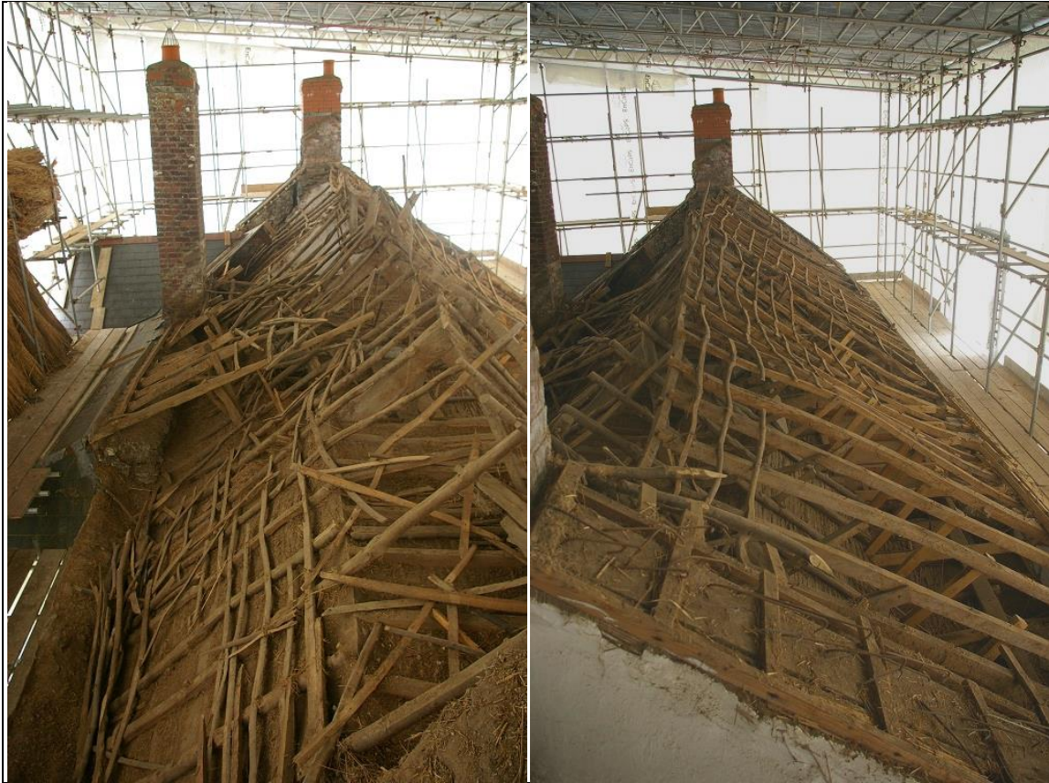
28. LEFT: WESTACOMBE ROOF, STRIPPED OF THATCH FROM THE WEST END, NORTH SIDE. 29. RIGHT: WESTACOMBE ROOF, STRIPPED OF THATCH FROM THE WEST END, SOUTH SIDE.
