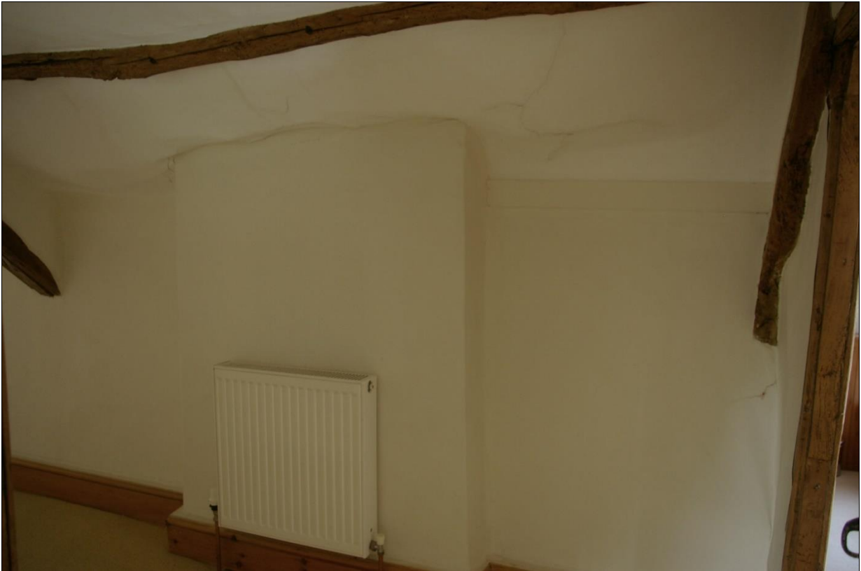
23. ROOM 11, THE NARROWER UPPER PART OF THE LATERAL STACK, SEEN WITHIN THE CORRIDOR BUT DESIGNED TO HEAT THE NEW FLOORED ROOM ON THE FIRST FLOOR; FROM THE SOUTH-EAST.
