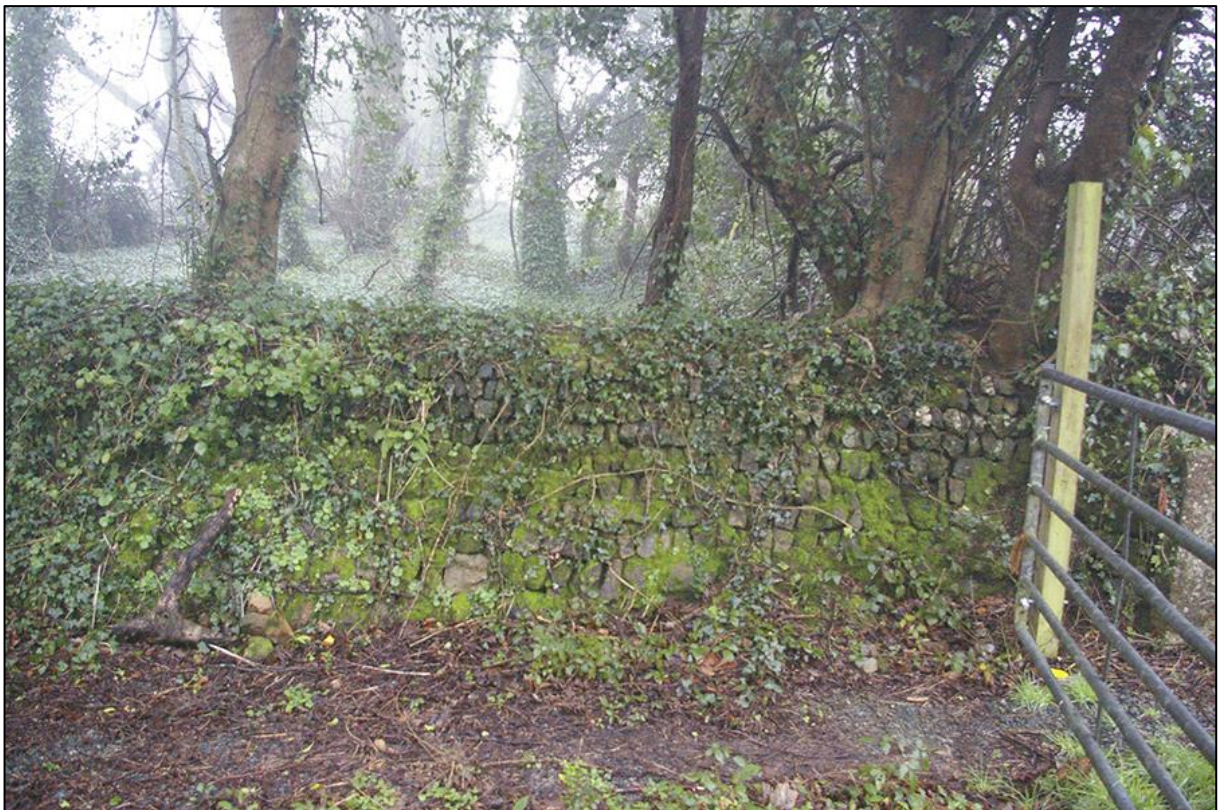
2. BOUNDARY WALL BESIDE SITE ENTRANCE WITH HIGHER GROUND BEYOND; VIEWED FROM THE SOUTH-WEST (NO SCALE).
