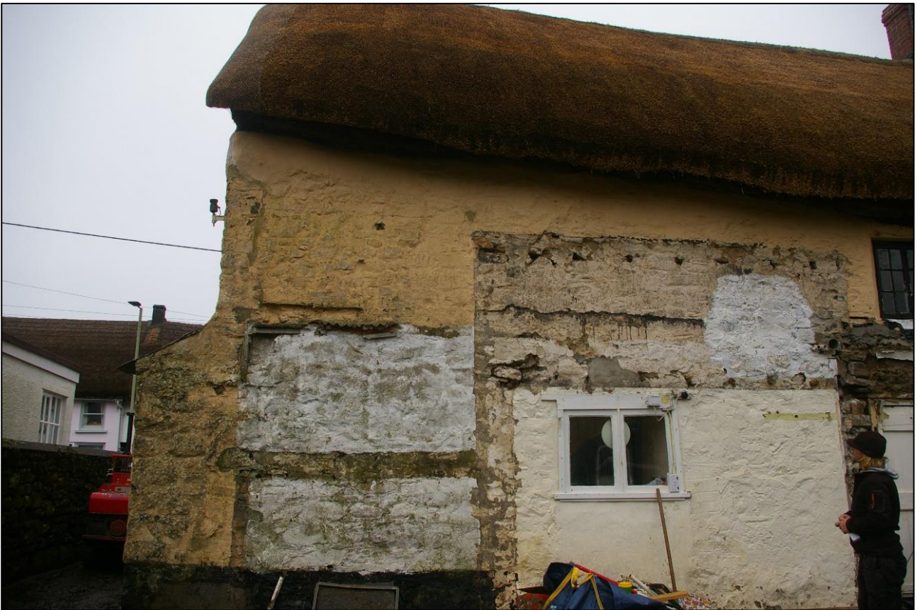
10. DETAIL OF THE EXTERNAL SOUTH ELEVATION OF SYCAMORE COTTAGE, TO THE WEST END, SHOWING THE SURVIVING STUB OF DEMOLISHED WEST END OF THE HISTORIC STRUCTURE; VIEWED FROM THE SOUTH.
