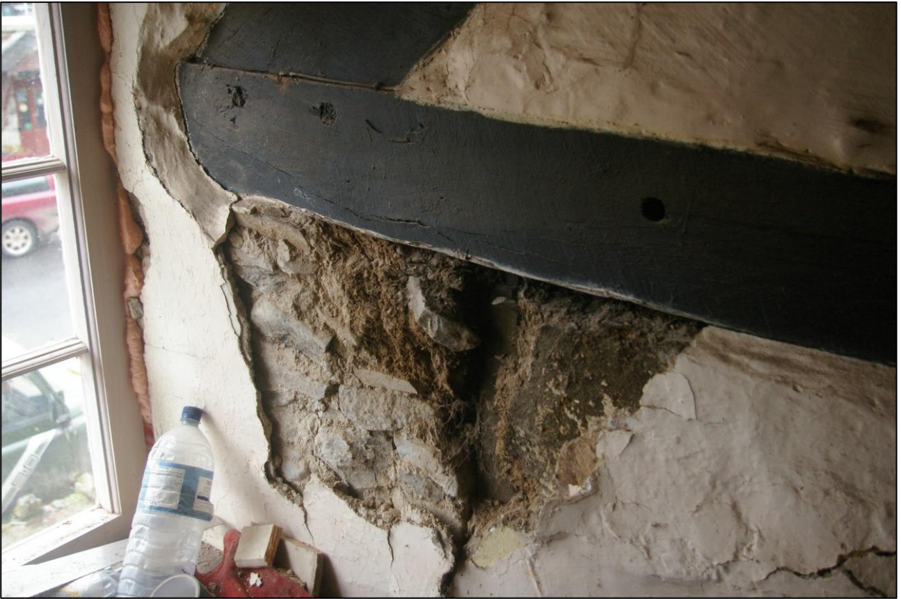
33. R3, DETAIL OF THE SMOKE BLACKENED COB TO THE WALL BETWEEN R3 AND R4, WITH DETAIL OF THE ROOF TRUSS; VIEWED FROM THE SOUTH-WEST.
