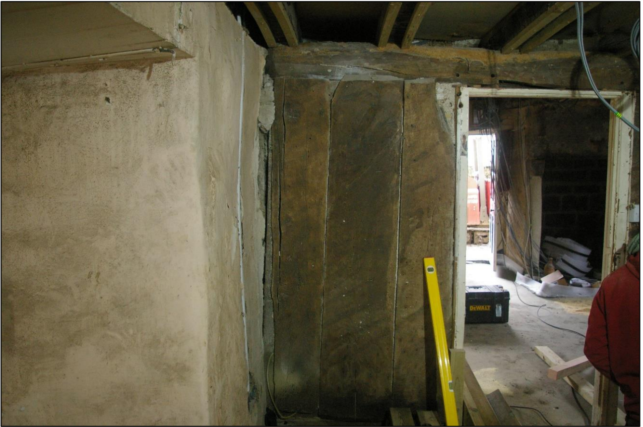
19. R2, DETAIL OF THE SOUTH END OF THE PARTITION WALL BETWEEN R1 AND R2; VIEWED FROM THE EAST.
