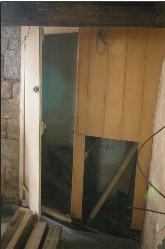
28. R2, DETAIL OF THE RECENT PARTITION BETWEEN R2 AND THE SOUTH-WEST STAIRCASE; VIEWED FROM THE WEST.
