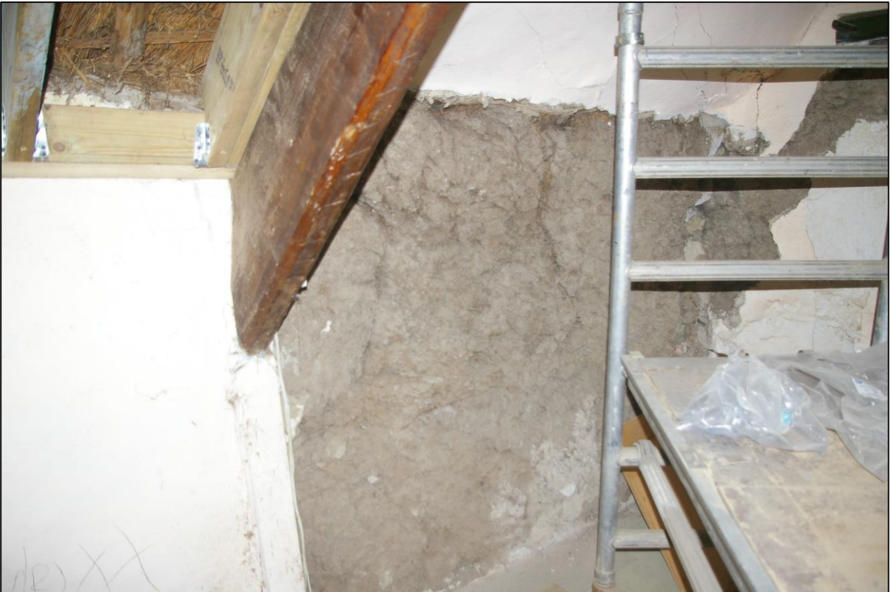
37. R4, THE FOOT OF THE TRUSS AND DETAIL OF THE COB WALL IN THE NORTH-EAST CORNER; VIEWED FROM THE SOUTH-WEST.
