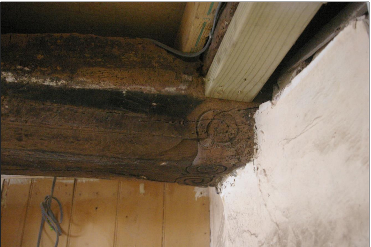
20. R2, DETAIL OF THE SCROLLWORK AT THE SOUTHERN END OF THE OVOLO- AND FILLET-MOULDED BEAM; VIEWED FROM THE WEST.
