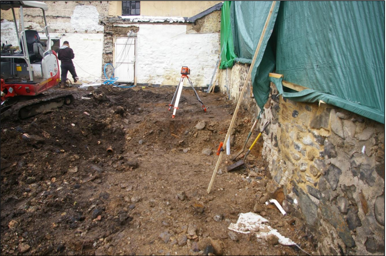
1. AREA 01 FOLLOWING REMOVAL OF MODERN STRUCTURES; VIEWED FROM THE SOUTH (NO SCALE).
