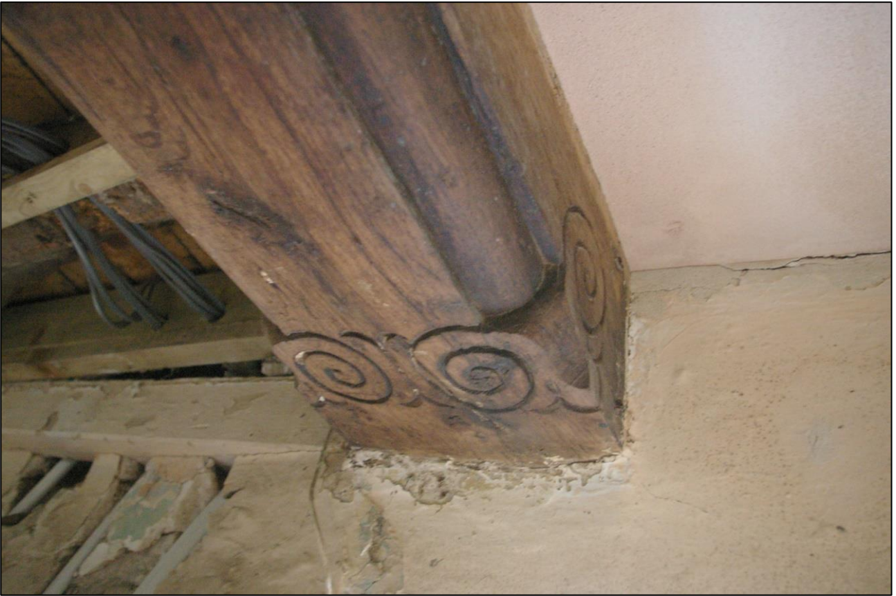
23. R2, DETAIL OF THE SCROLLWORK AT THE NORTHERN END OF THE OVOLO- AND FILLET-MOULDED BEAM; VIEWED FROM THE SOUTH-WEST.
