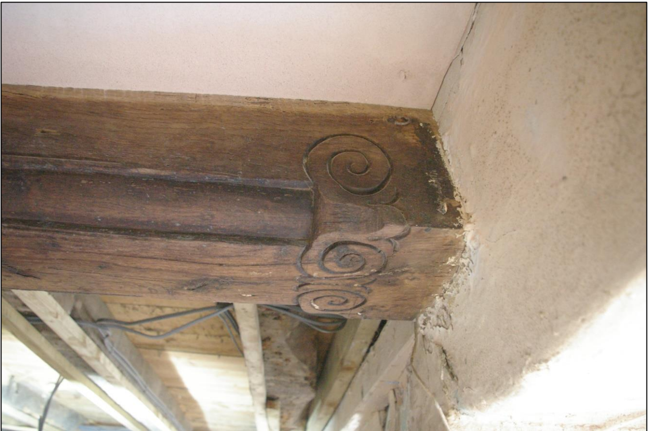
22. DETAIL OF THE SCROLLWORK AT THE NORTHERN END OF THE OVOLO- AND FILLET-MOULDED BEAM; VIEWED FROM THE EAST.
