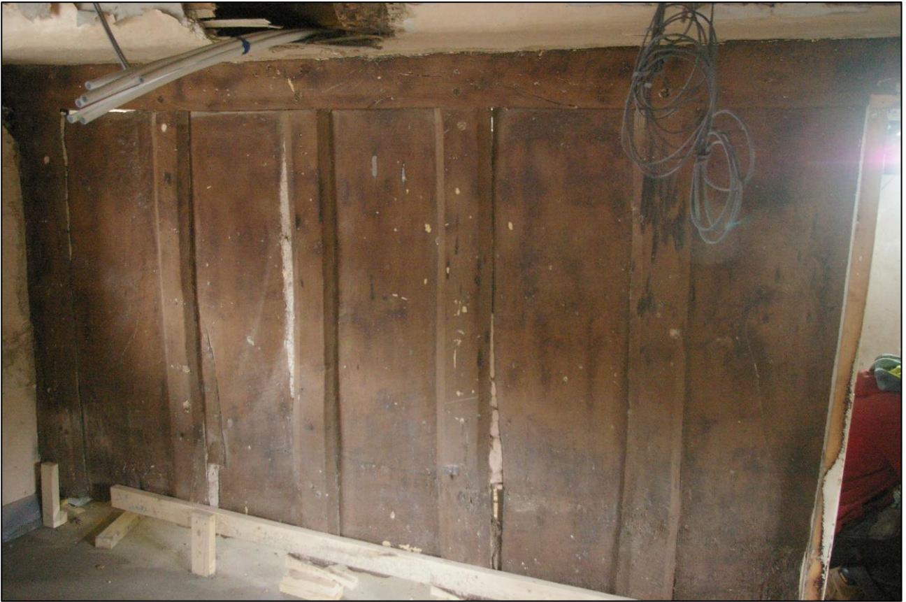
15. R1, DETAIL OF THE PLANK AND MUNTIN SCREEN PARTITION BETWEEN R1 AND R2; VIEWED FROM THE SOUTH-WEST.
