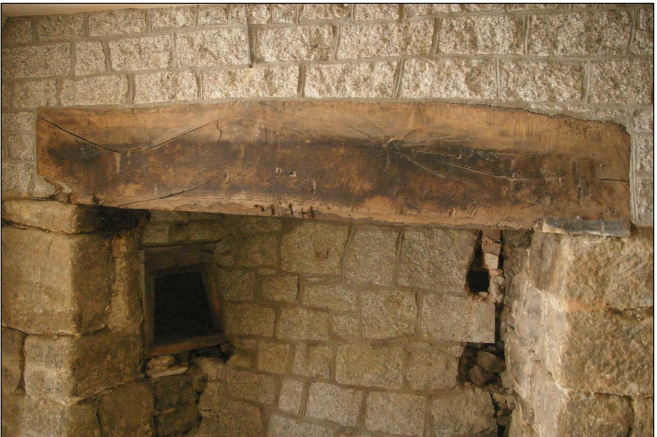
26. R2, DETAIL OF THE LINTEL AND BLOCKING TO THE FIREPLACE IN THE EAST GABLE WALL; VIEWED FROM THE SOUTH-WEST.
