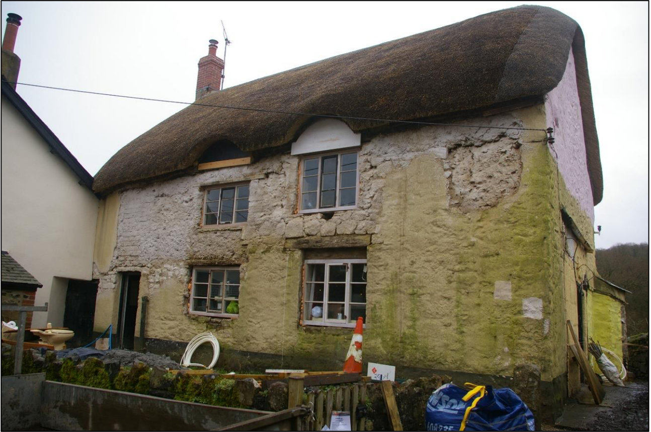
6. NORTH EXTERNAL ELEVATION OF SYCAMORE COTTAGE DURING REMEDIAL WORKS; VIEWED FROM THE NORTH-WEST.
