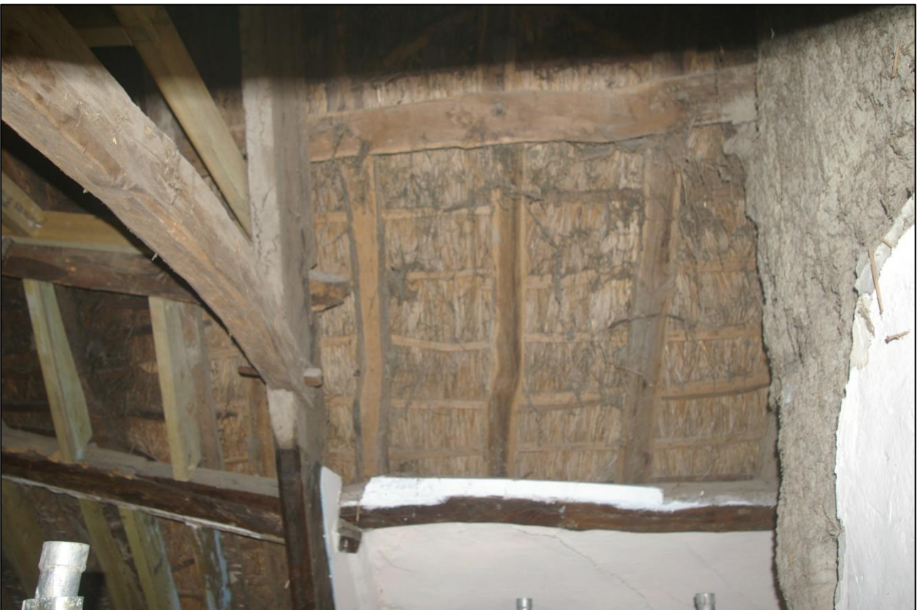
38. R4, DETAIL OF THE THATCHED ROOF, WHICH IS NOT SMOKE-BLACKENED; VIEWED FROM THE SOUTH.
