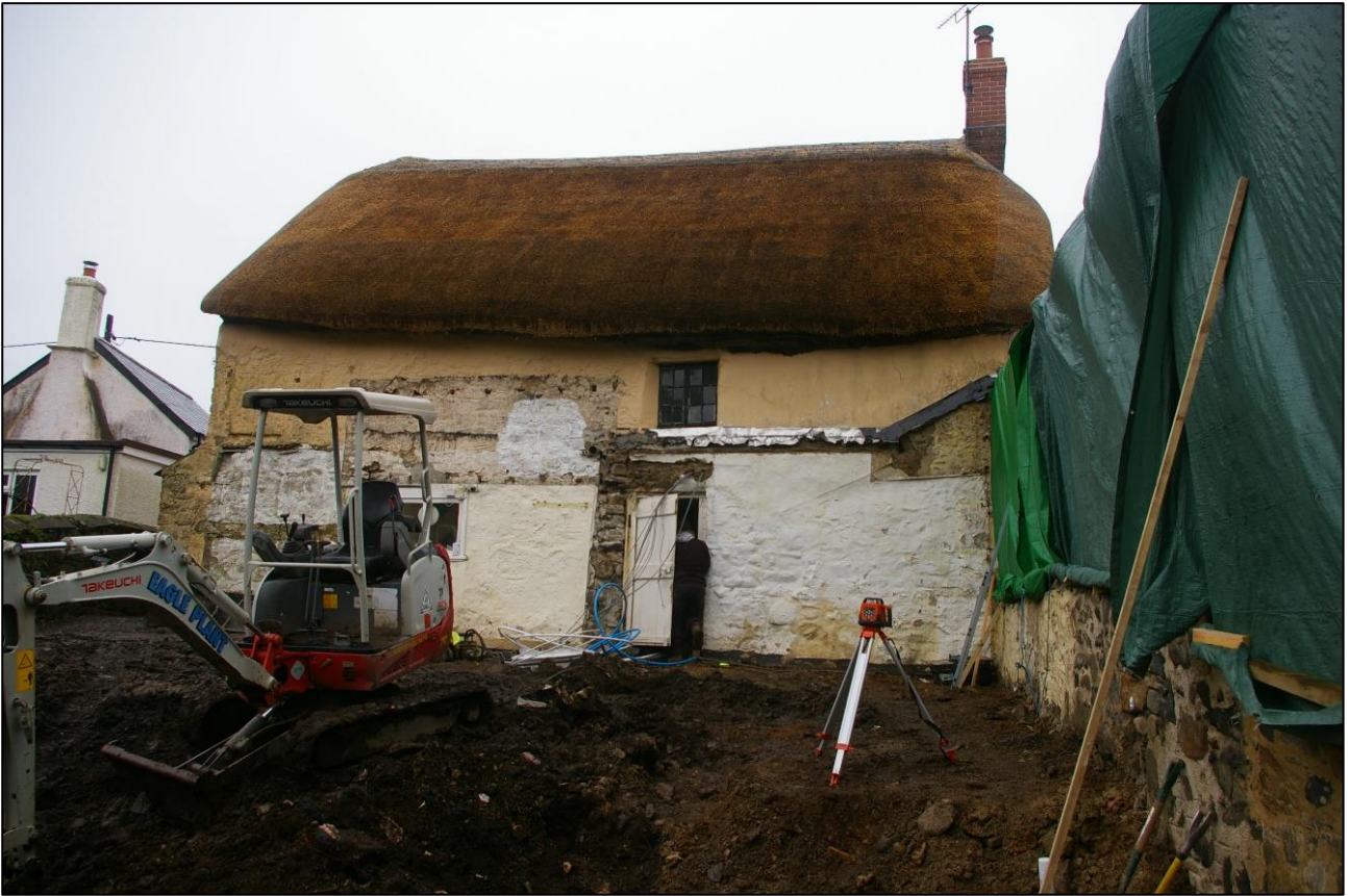
9. EXTERNAL SOUTH ELEVATION OF SYCAMORE COTTAGE SHOWING THE SCARRING FROM THE FORMER OUTBUILDINGS/EXTENSION; VIEWED FROM THE SOUTH.
