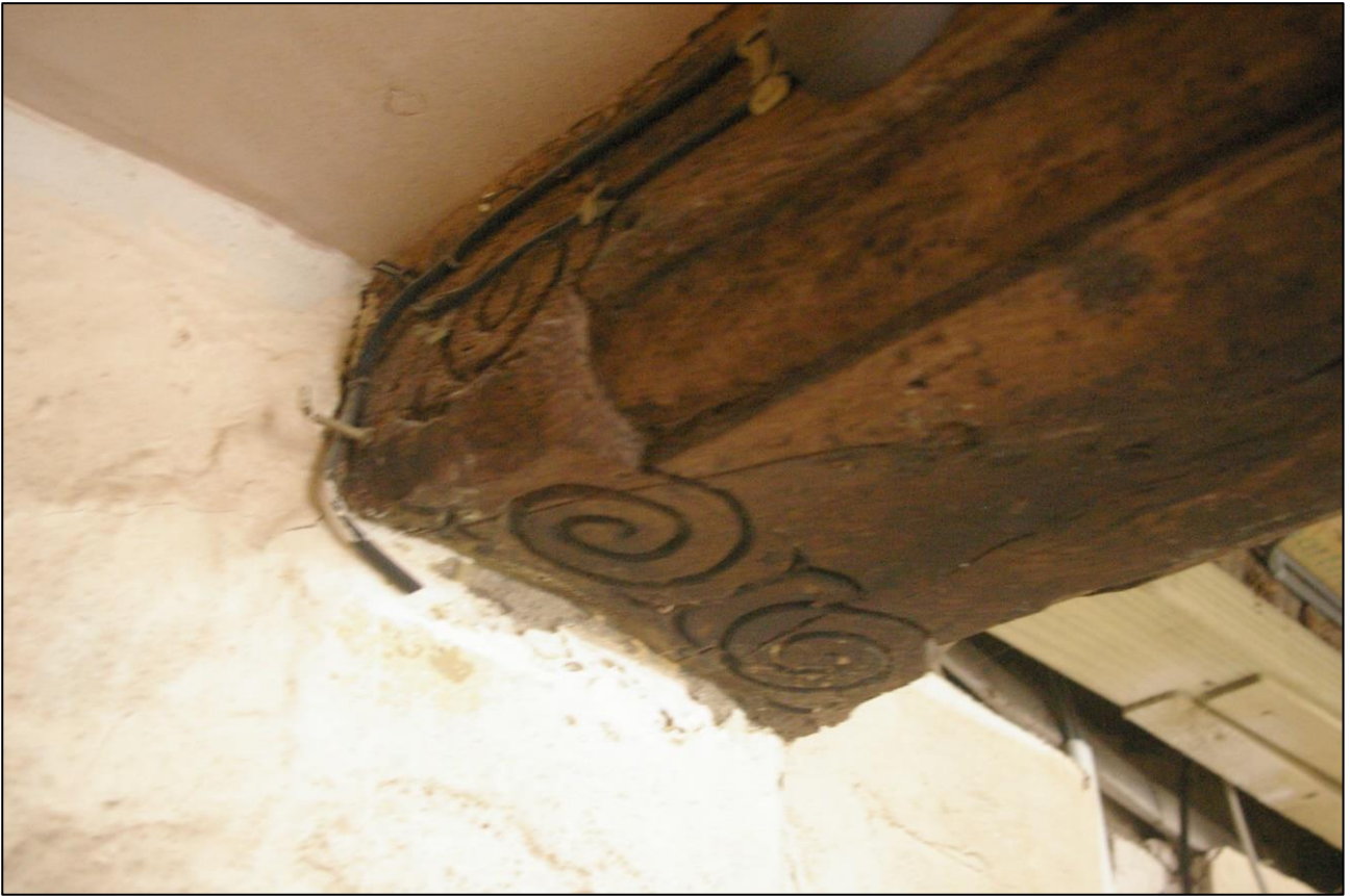
21. R2, DETAIL OF THE SCROLLWORK AT THE SOUTHERN END OF THE OVOLO- AND FILLET-MOULDED BEAM; VIEWED FROM THE NORTH-EAST.
