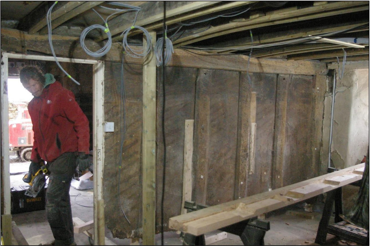
17. R2, DETAIL OF THE PLANK AND MUNTIN SCREEN PARTITION BETWEEN R1 AND R2; VIEWED FROM THE SOUTH-EAST.
