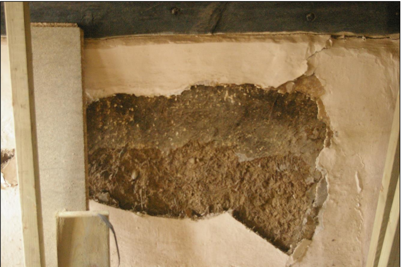
32. R3, DETAIL OF THE SMOKE BLACKENED COB WALL BELOW THE TRUSS BETWEEN R3 AND R4; VIEWED FROM THE SOUTH-WEST.
