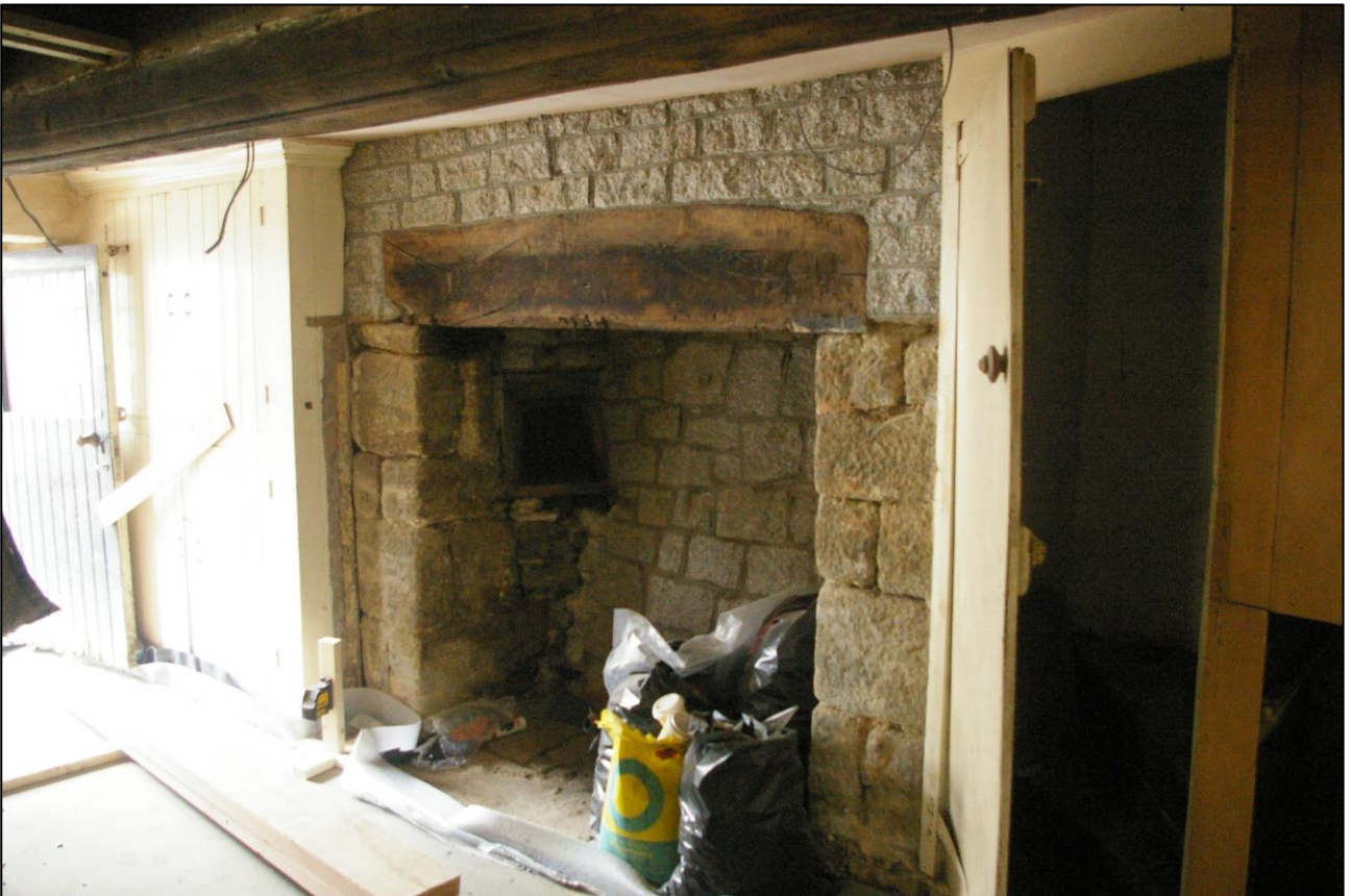
24. R2, DETAIL OF THE FIREPLACE IN THE EAST GABLE WALL OF R2; VIEWED FROM THE SOUTH-WEST.
