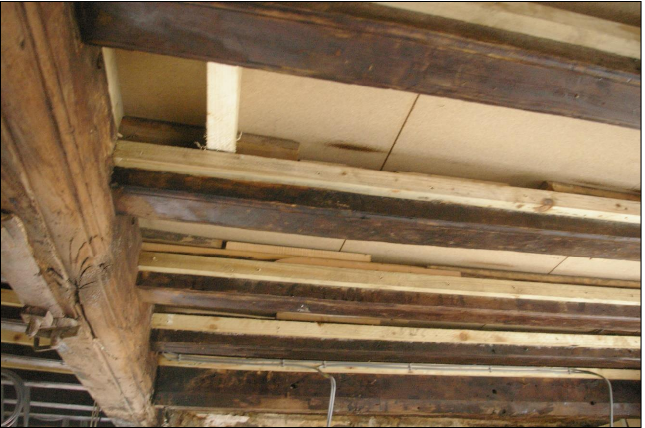
13. R1, DETAIL OF THE CHAMFERED BEAM TO THE CEILING; VIEWED FROM THE SOUTH-EAST.
