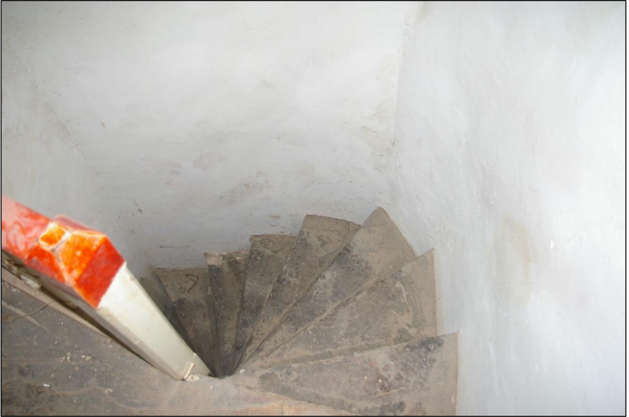
29. DETAIL OF THE SPIRAL STAIRCASE IN THE SOUTH-WEST CORNER OF R2; VIEWED FROM THE WEST.
