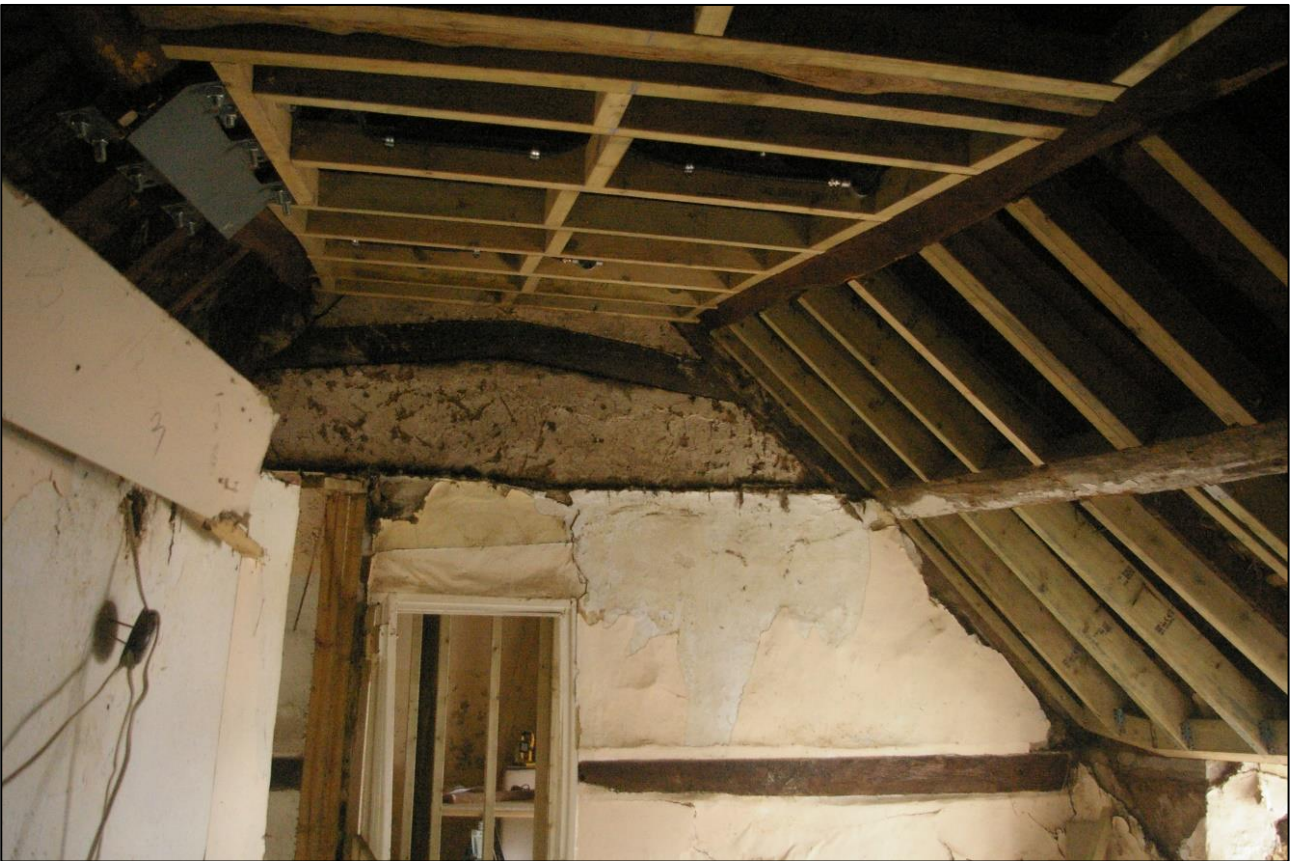
34. R4, DETAIL OF THE WALL SEPARATING R4 FROM R5; VIEWED FROM THE EAST.
