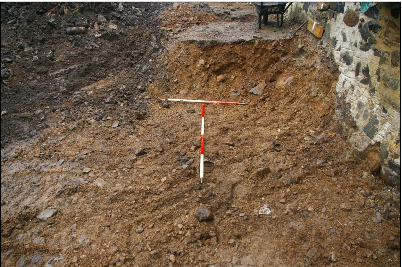
2. AREA 01 FOLLOWING INITIAL SITE STRIP; VIEWED FROM THE SOUTH (1M & 2M SCALES).
