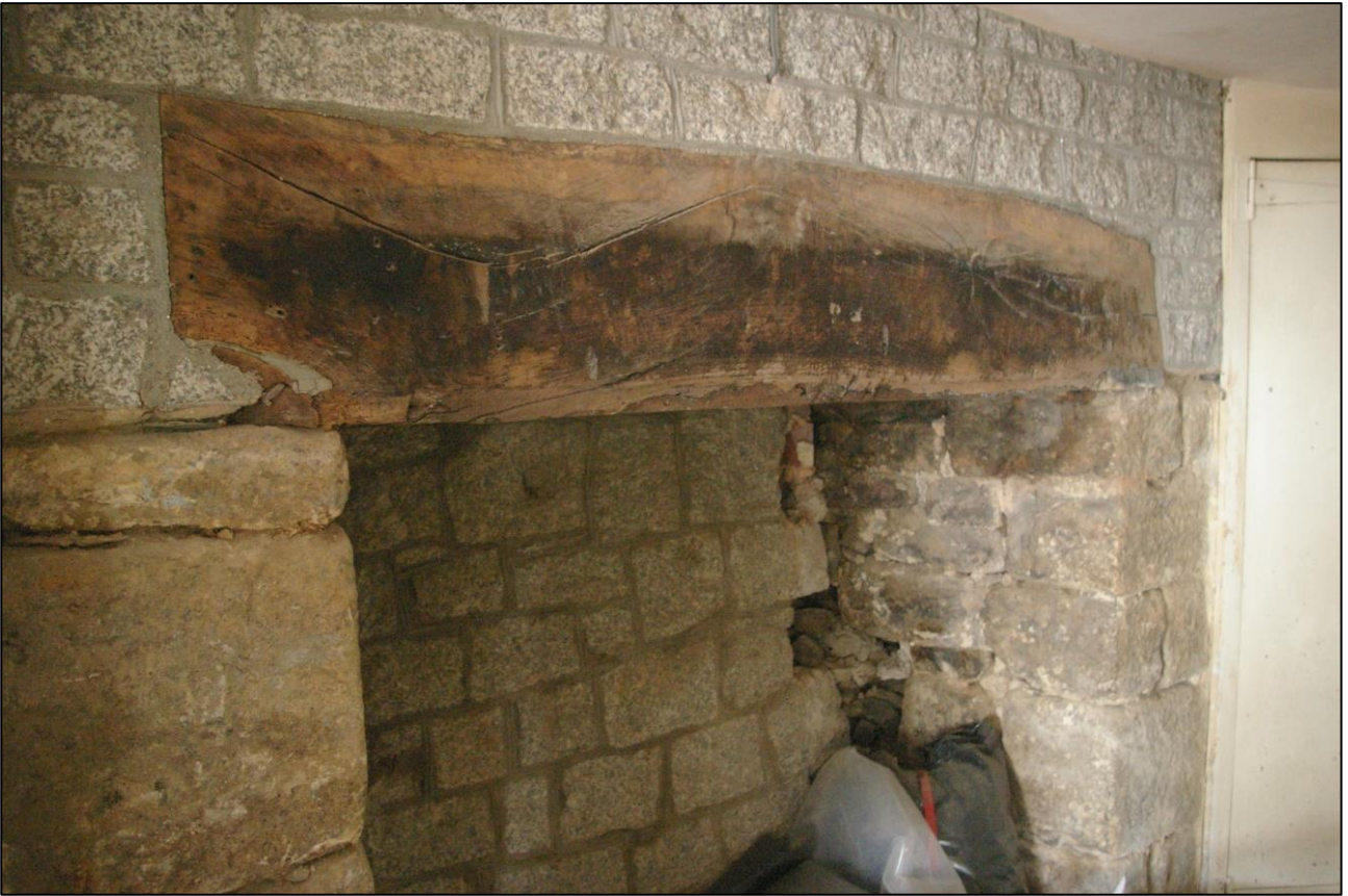
27. R2, DETAIL OF THE LINTEL AND BLOCKING TO THE FIREPLACE IN THE EAST GABLE WALL; VIEWED FROM THE NORTH-WEST.
