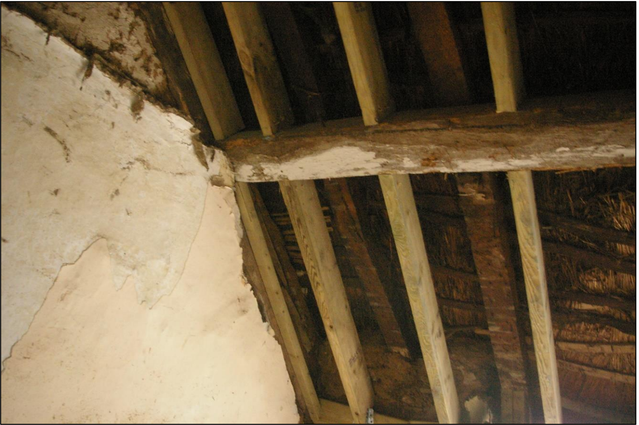
35. R4, DETAIL OF THE NORTH PITCH OF THE ROOF STRUCTURE SHOWING THE THATCH; VIEWED FROM THE SOUTH-EAST.
