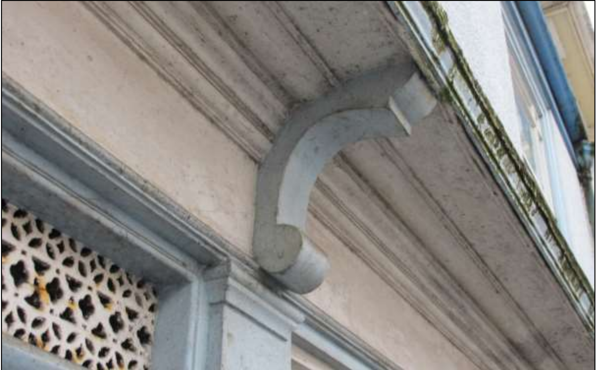
FIGURE 4: DETAIL OF THE 19 TH CENTURY CORNICE WITH SUPPORT BRACKET AND SURVIVING CAST IRON GRILLE ABOVE SHOP DOOR.
