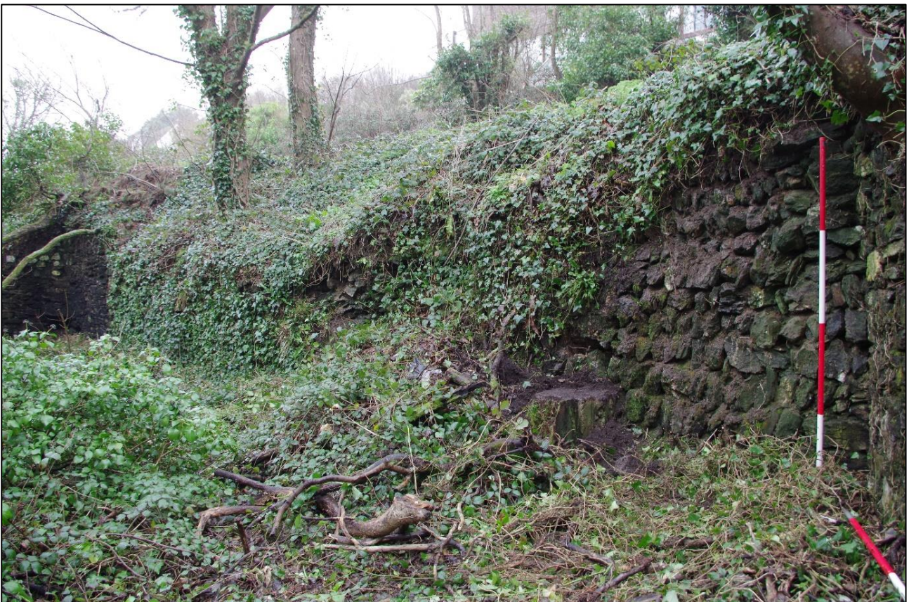
8. RUBBLE RETAINING WALL TO ROAD AT REAR OF WET DRESSING FLOOR; VIEWED FROM THE WEST (SCALE 2M).
