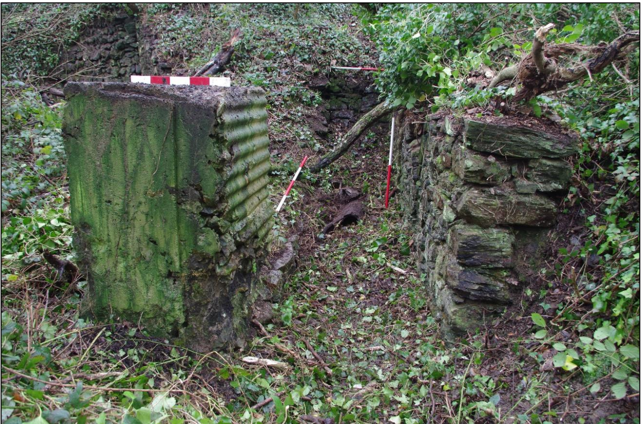
2. VIEW ALONG WATER WHEEL PIT 2 FROM THE NORTH-WEST. NOTE THE CORRUGATED IRON AND TIMBER IMPRESSIONS IN THE CAST CONCRETE DRIVESHAFT STAND TO THE LEFT (SCALES 2M, 1M AND 0.5M).
