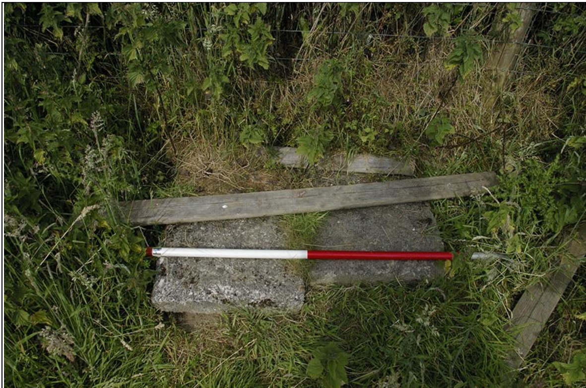
30. DETAIL OF CONCRETE PLINTH AT NORTH-EAST BOUNDARY F2; VIEWED FROM THE WEST-SOUTH-WEST (1M SCALE).
