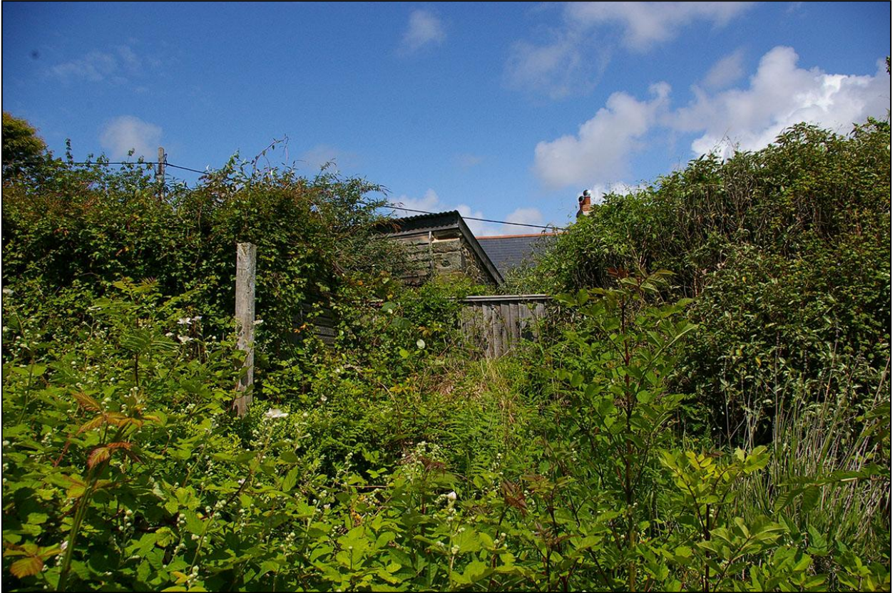
THE BACK OF THE CIDER BARN AND FURTHER TIMBER SHEDS, AS WELL AS A GLIMPSE OF THE ROOF OF THE ADJACENT HOUSE; FROM THE SOUTH.
