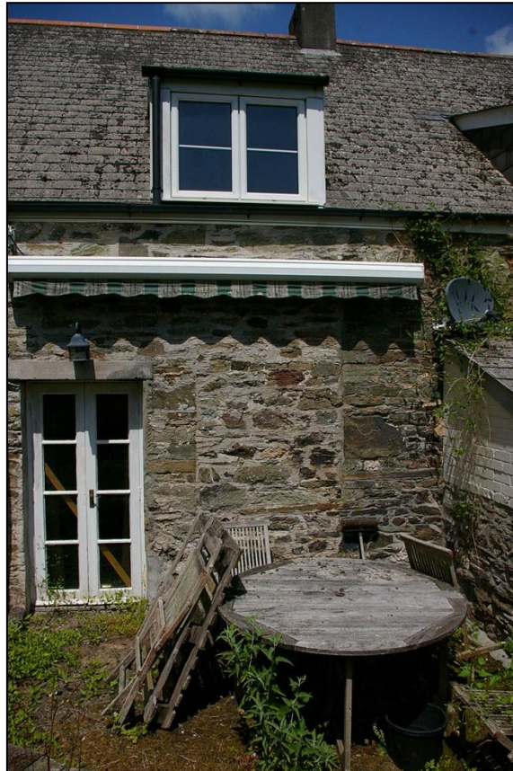
THE BLOCKED DOORWAY IN THE SOUTH ELEVATION OF THE COTTAGE IN THE SOUTH-EAST CORNER, SHOWING GOOD DRESSED REVEALS; FROM THE SOUTH.
