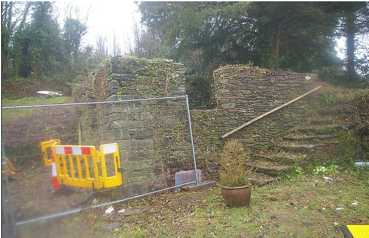
THE EAST WALL OF THE DETACHED MEDIEVAL BLOCK, SHOWING A LENGTH OF EARLY REBUILDING AND ONE MODERN REPAIR, WITH THE LATER 20 TH CENTURY GARDEN STEPS; FROM THE SOUTH-EAST.
