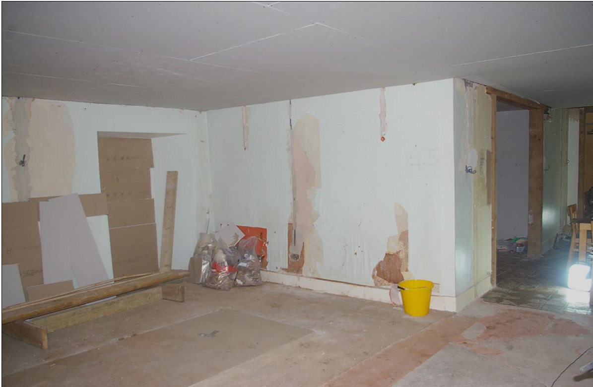
ROOM 3, IN THE FARMHOUSE, THE MAIN SITTING ROOM, WITH BOARDED OVER FRENCH-STYLE PATIO DOORS TO THE GARDEN; FROM THE NORTH-EAST.
