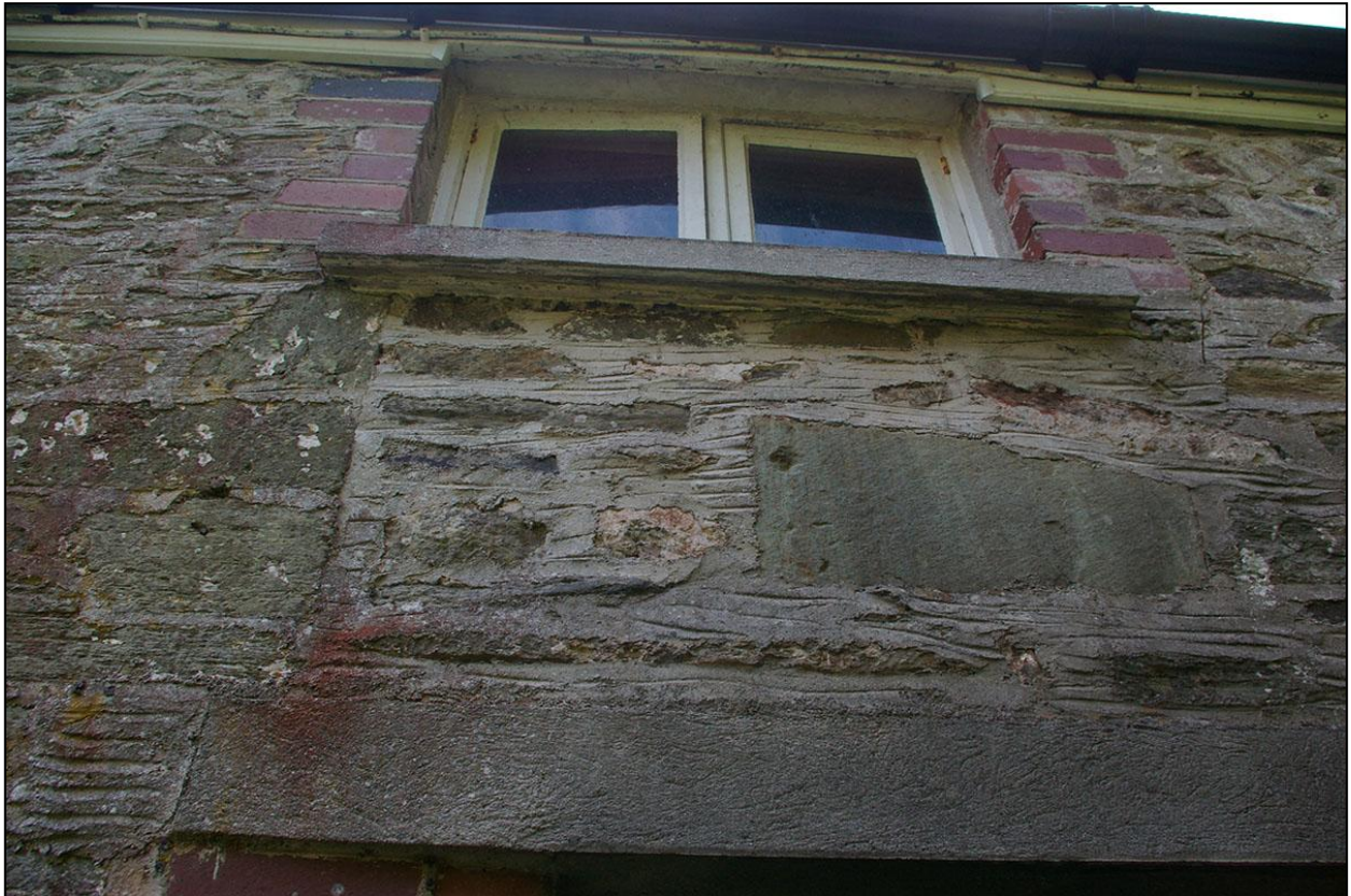
THE SMALL BLOCKED WINDOW WITH BRICK REVEALS SET INTO A LARGER OPENING, A LOADING DOOR ABOVE THE FORCED DOORWAY TO THE FRONT OF THE ATTACHED COTTAGE; FROM BELOW (NORTH-EAST).
