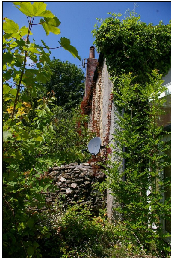
VIEW ALONG THE BACK OF THE FARMHOUSE, SHOWING HOW IT IS ALMOST TOTALLY OBSCURED BY OVERGROWTH; FROM THE EAST.
