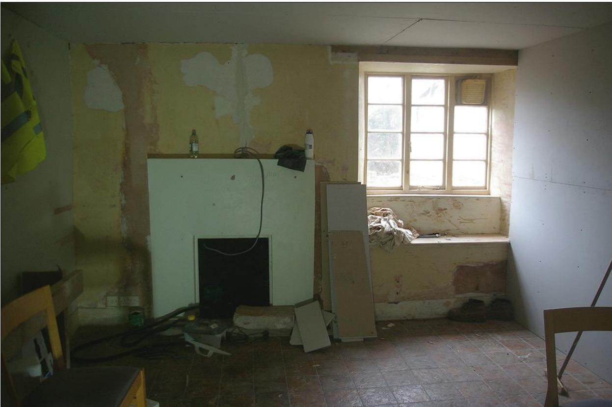
THE MODERNISED KITCHEN FIREPLACE AND GOOD 19 TH CENTURY WINDOW, ROOM 2B; FROM THE NORTH.
