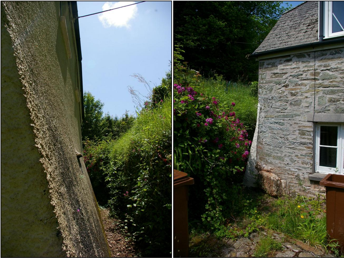
LEFT: THE WEST GABLE END OF THE COTTAGE, SHOWING HEAVY BUTTRESS AND FORCED WINDOWS SET HIGH IN APEX; FROM THE NORTH. RIGHT: VIEW OF THE SOUTH-WEST CORNER OF THE COTTAGE, SHOWING BRICK RENDERED BUTTRESS SUPPORTING THE WEST GABLE; FROM THE SOUTH-EAST.
