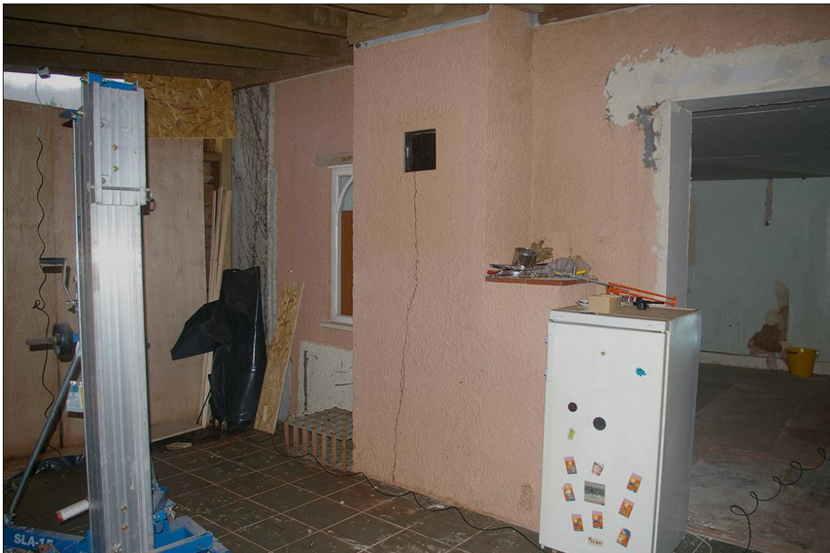
THE MODERN BOXY STACK SERVING THE SITTING ROOM FIREPLACE, ENCLOSED WITHIN THE CONSERVATORY; FROM THE NORTH-EAST.
