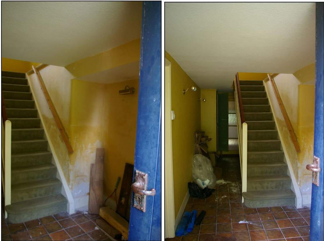
LEFT: INTO THE ENTRANCE HALLWAY AND STAIRS, ROOM 1, SHOWING HOW THIS DOOR HAS BEEN FORCED UP AGAINST THE PARTY WALL TO THE COTTAGE, WHICH HAS A LARGE BLOCKED DOORWAY WITHIN IT; FROM THE NORTH-EAST.
