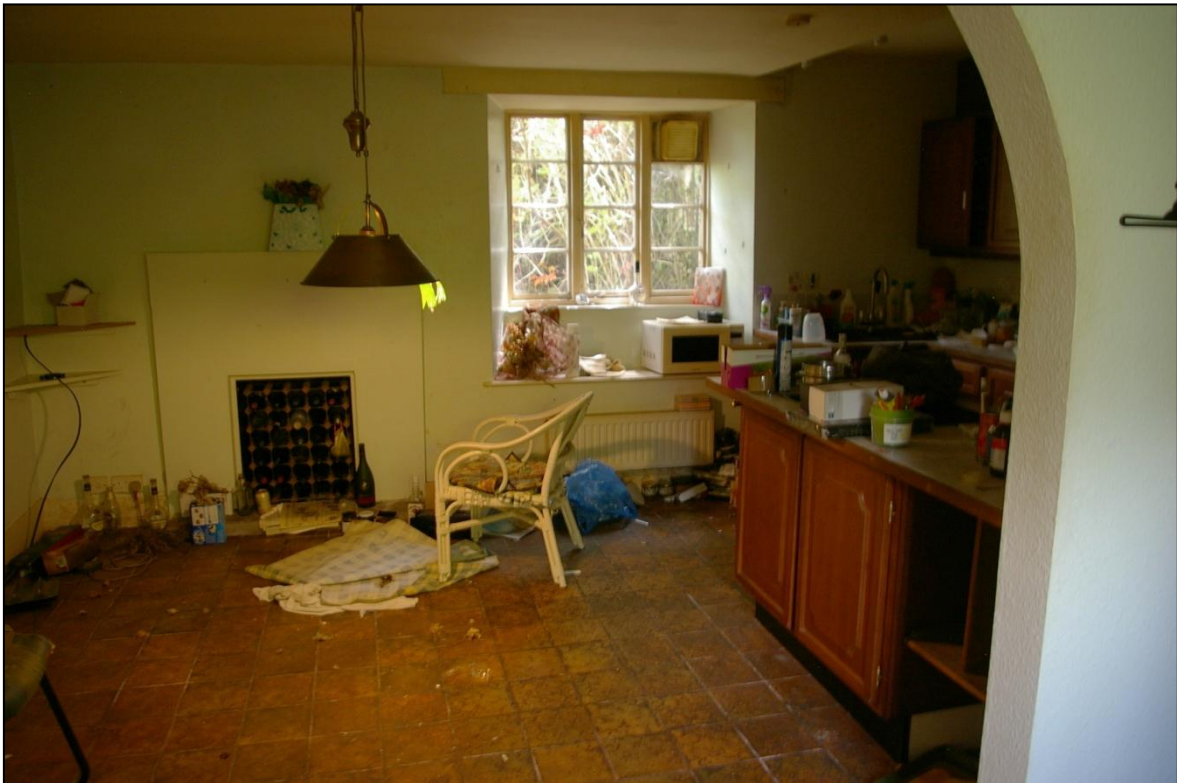
FIGURE 16: VIEW OF THE FITTED KITCHEN, WITH THE THREE LIGHT 19 TH CENTURY CASEMENT AND WINDOW SEAT, BLOCKED FIREPLACE ON THE REAR WALL, MODERN QUARRY TILED FLOOR, BOARDED OUT CEILING; FROM THE NORTH-NORTH-EAST.
