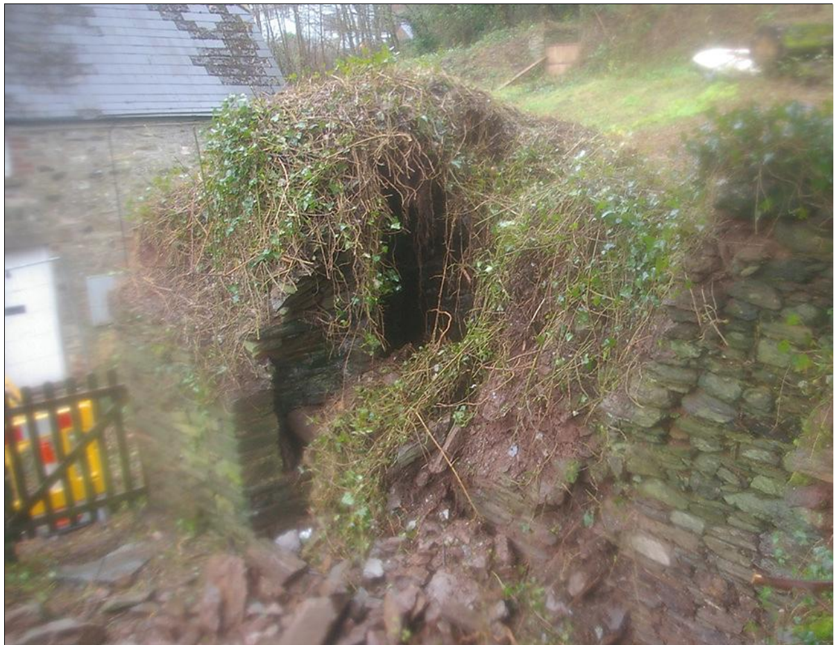
DETAILED VIEW INTO THE OVEN AND SHOWING THE ANGLED TAPERING PROFILE OF THE FORMER OPEN HEARTH; FROM THE NORTH-EAST.
