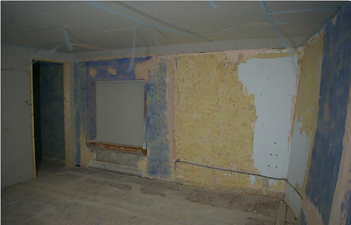
ROOM 9, BEDROOM 1, TO THE SOUTH OF THE BUILDING, SHOWING THE BATTERED AND ANGLED FRAGMENT OF EARLIER WALL TO THE SOUTH-EAST CORNER; FROM THE SOUTH-WEST.
