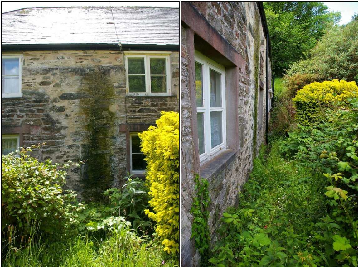
LEFT: DETAIL WITHIN THE RUINED WALL INCORPORATED INTO THE BUILDING SHOWING A POTENTIAL SET OF RAGGED LARGE SLAB QUOINS AND ALSO A POTENTIAL BLOCKED OPENING AT GROUND FLOOR; FROM THE NORTH.
