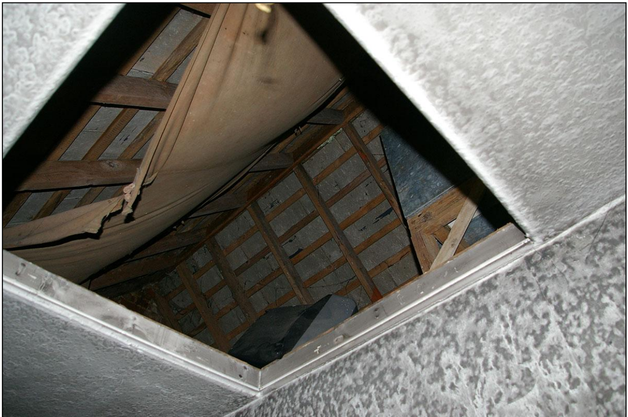
VIEW UP INTO THE LOFT, SHOWING THE MODERN COMMON RAFTER REPLACEMENT ROOF; FROM BELOW (NORTH-WEST).
