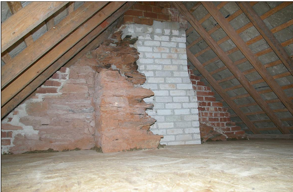
THE STACK TO THE WEST END OF BATSON HALL FARM; WITH FRAGMENTARY REMAINS RISING TO ONE AND A HALF STOREYS, THE STONWORK PATCHED IN BRICKWORK IN LIME MORTAR, THEN IN LATER BRICKWORK IN CEMENT AND IN CONCRETE BLOCK, INDICATING 19 TH AND SEVERAL PHASES OF 20 TH CENTURY REMODELLING.
