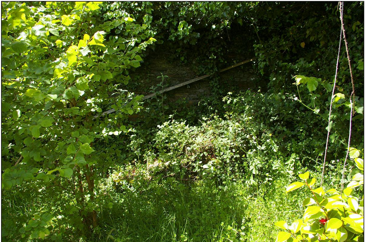
THE EAST WALL OF THE SQUARE BLOCK LARGELY OBSCURED BY IVY BUT ALSO WITH THE SET OF SATE GARDEN STEPS RISING ALONGSIDE IT; FROM THE EAST.
