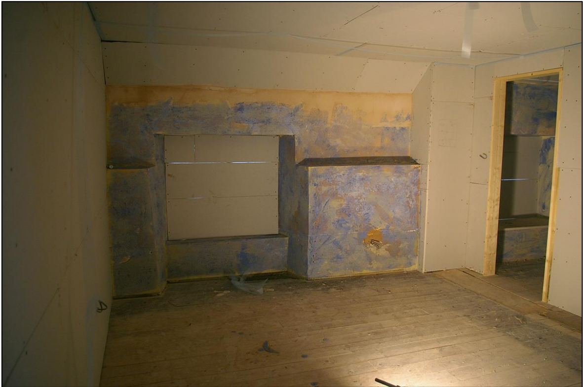
FIGURE 18: BEDROOM 2, ROOM 8, SHOWING THE MEDIEVAL WALL FRAGMENT SURVIVING TO THE NORTH WALL; FROM THE SOUTH-WEST.
