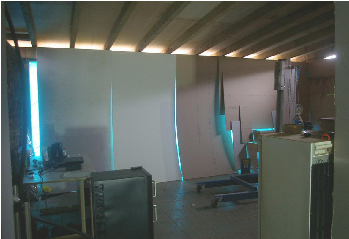
THE CONSERVATORY, WHICH HAS BEEN BOARDED OUT FOR SECURITY AND DUE TO PARTIAL COLLAPSE; FROM THE WEST-NORTH-WEST.
