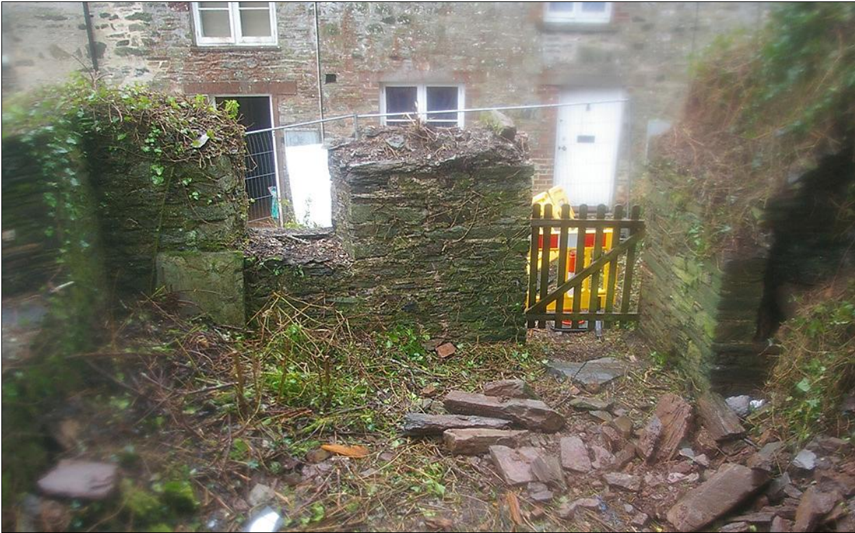
THE SOUTH WALL OF THE DETACHED BLOCK, WITH WINDOW AND DOOR, SHOWING THE INNER VERNACULAR CHARACTER FACE OF THE WALL, SO DIFFERENT FROM THE OUTER DRESSED AND FACED STONEWORK, FROM THE NORTH.
