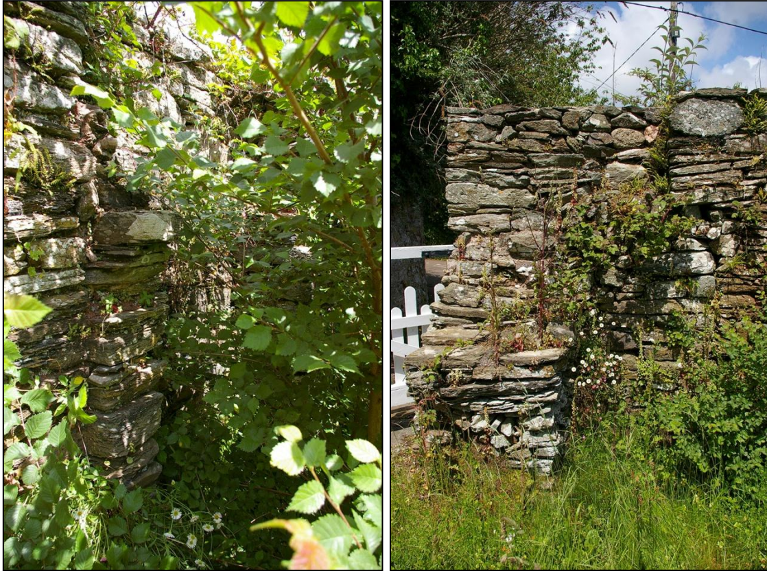
LEFT: VIEW OF THE RAISED FLAT BUILT PILASTERS AND PADSTONE WHICH WOULD HAVE CARRIED A STONE OR WOOD CORBELLED BRESUMMER OVER A LARGE OPEN FIREPLACE; FROM THE SOUTH-WEST.
