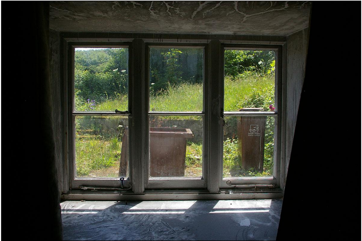
DETAIL OF THE GOOD 19 TH CENTURY THREE LIGHT CASEMENT WINDOW CW3; FROM THE NORTH.
