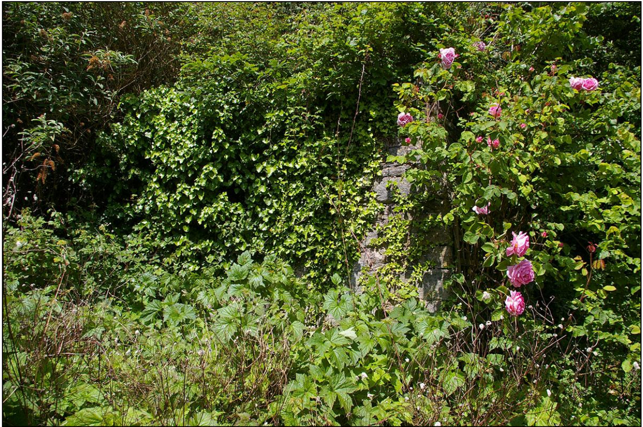
THE SOUTH-EAST CORNER OF THE SQUARE BLOCK, SHOWING ITS GOOD SHAPED BLOCK QUOINS; FROM THE SOUTH-EAST.
