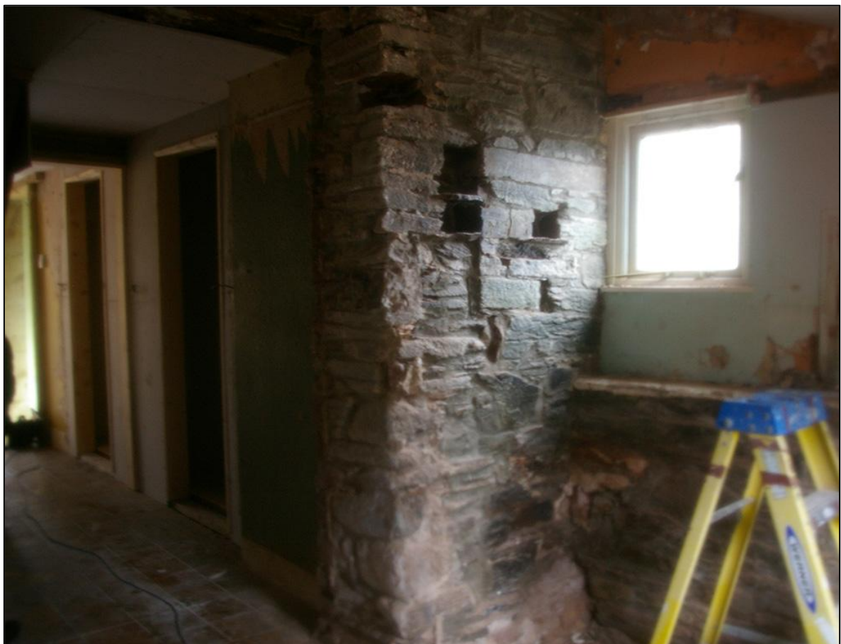
FIGURE 21: THE SHORT LENGTH OF GOOD DRESSED AND FACED MEDIEVAL STONEMWORK, WITH ABUTTING HEAVY SLATESTONE RUBBLE AROUND OPENING AND PUTLOG HOLES, REWORKED AS DOVE HOLES, WITHIN THE PROJECTION ON THE SOUTH ELEVATION OF THE FARMHOUSE, NOW ENCLOSED WITHIN THE OUTSHUT; FROM THE SOUTH-WEST.
