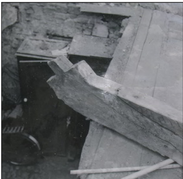
Figure 22: Foot of roof timber after removal.
