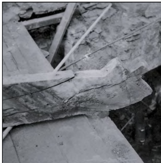
Figure 23: Foot of roof timber after removal.
