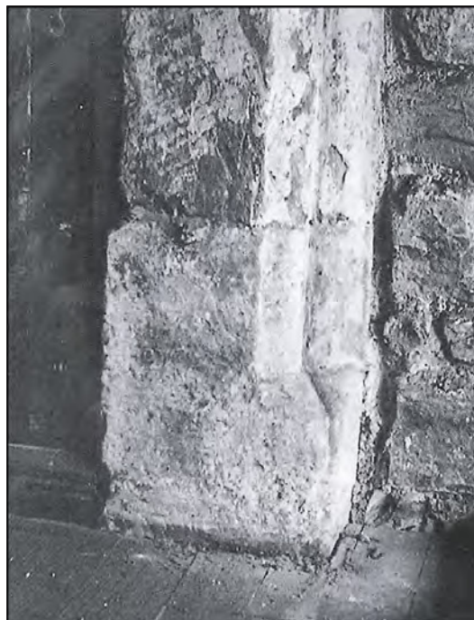
Figure 29: Foot of the left-hand jamb of the first floor front fireplace.
