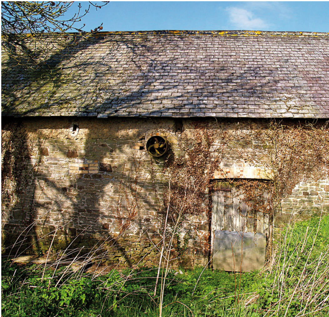
[19] The centre of the north wall, showing the man-sized doorway to the threshing floor, with the driveshaft and belt drive for an external source of power.
