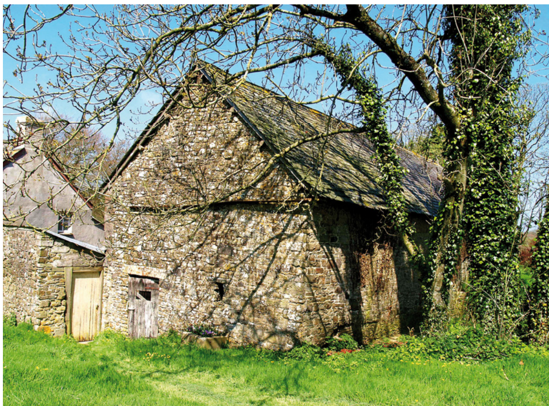
[20] The southern gable end of the barn. This is all stone rubble, and this end includes a calf-house.
