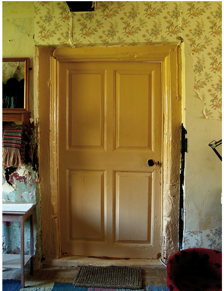
[12] The 17th century oak doorframe from the cross passage to the hall/ dining room. It contains an 18th century fielded-panel door.
