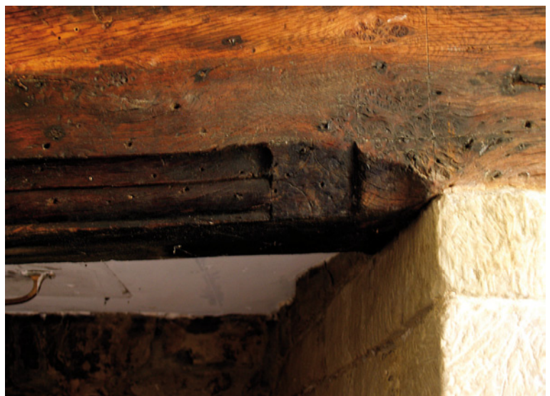
[14] Detail of the 17th century parlour fireplace showing the stop to the moulding on the oak lintel.
