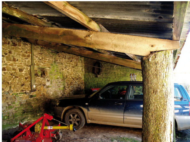
[38] The inside of the cartshed looking west from the barn end towards the end of the house. the rear wall to left includes a keeping place. The capentry is rather rudimentary.
