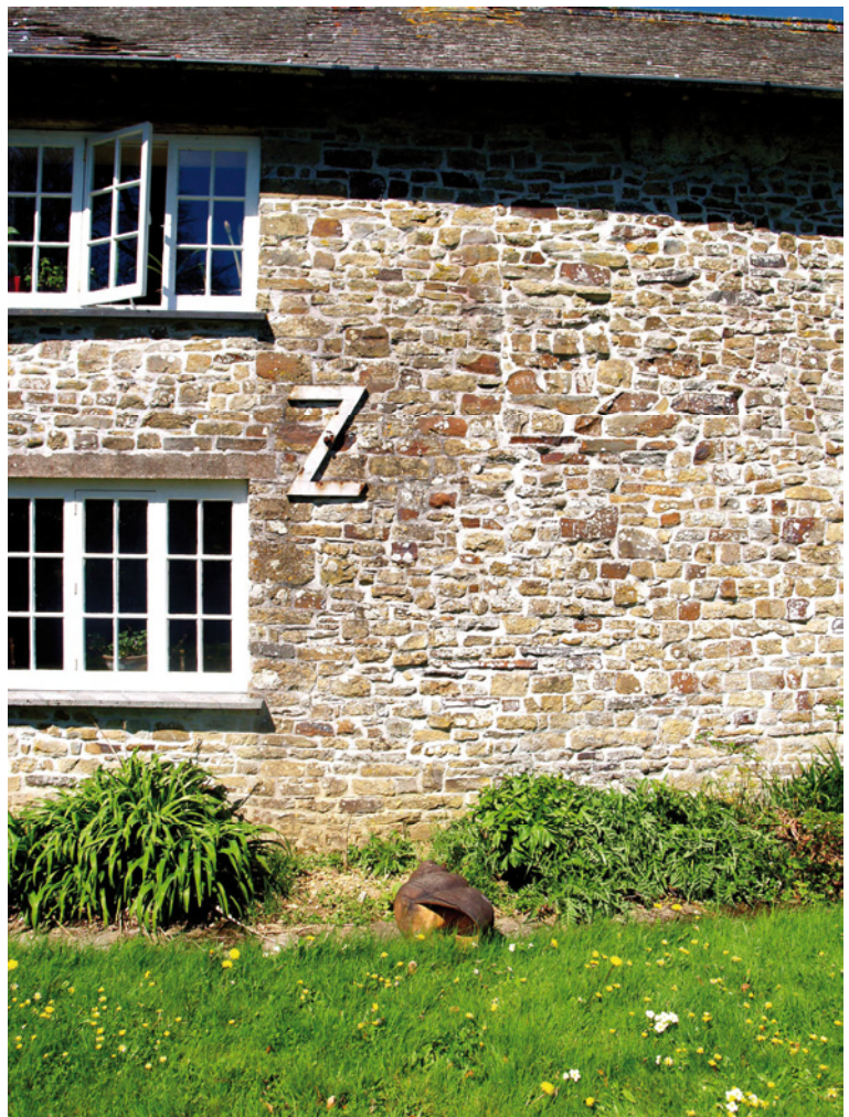
[9] Detail of the south front showing the vertical butt join in the masonry between the two eastern first floor windows. Notice too the Z-shaped plate of the c1880 tie-rod.
