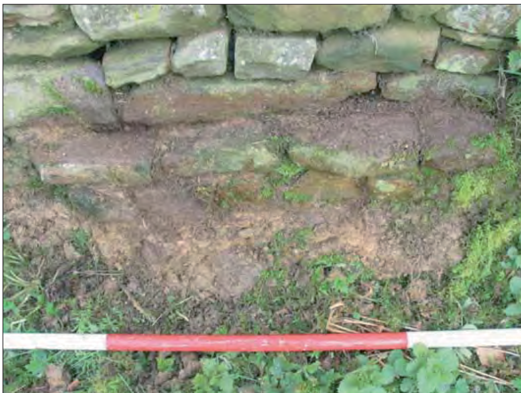
Plate 6: Detail of the rear north wall of the former stable showing the projecting base, viewed from the north.
