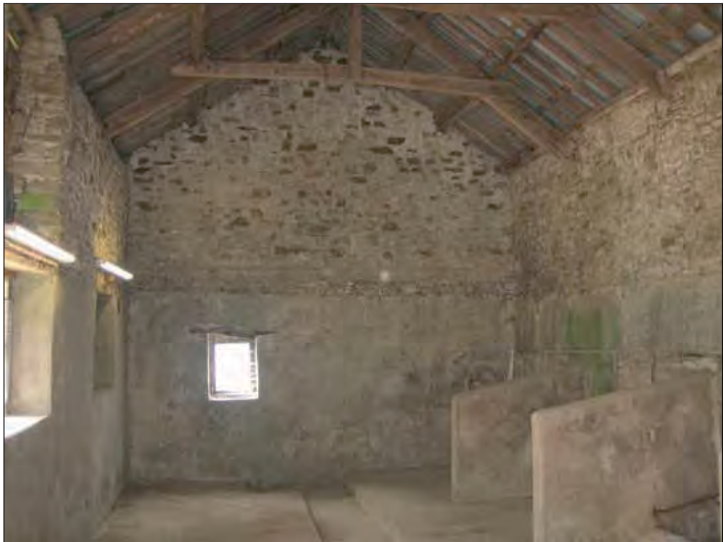
Plate 2: The interior west end of the former stable before the removal of the modern concrete.
