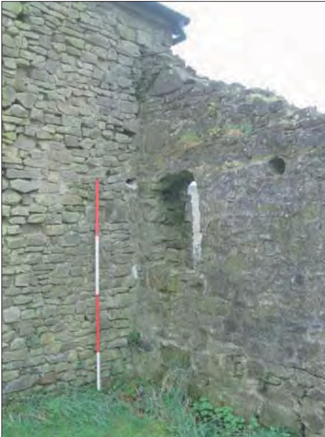
Plate 5: Western corner of the north wall of the stable abutting the west wall of the former shippon, viewed from the north.
