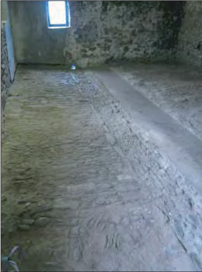
Plate 3: The interior west end of the former stable showing the cobbled floor and drain.
