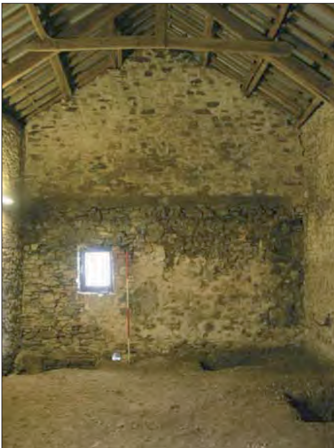
Plate 4: The interior west wall of the former stable after removal of the cobbled floor, showing brick repair to window reveal.
