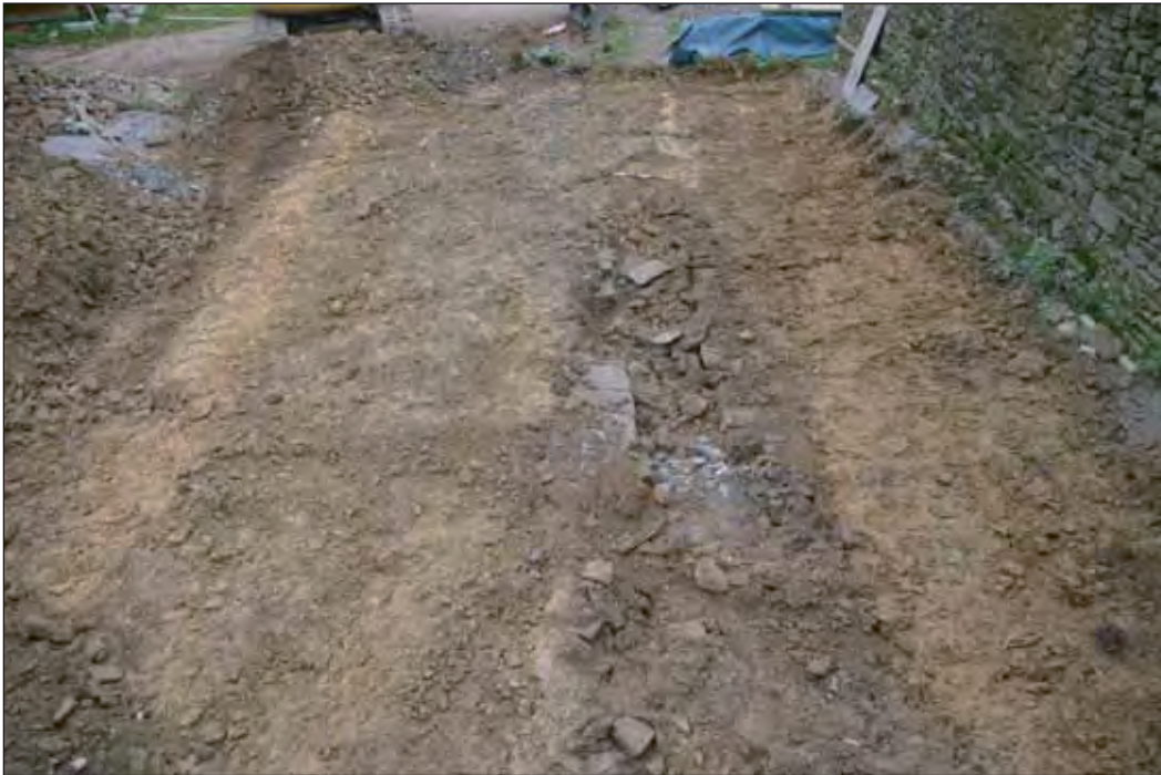
Plate 7: Stripped area of former shippon showing the orange soil indicating the position of the former rear wall and the former position of drain [508].
