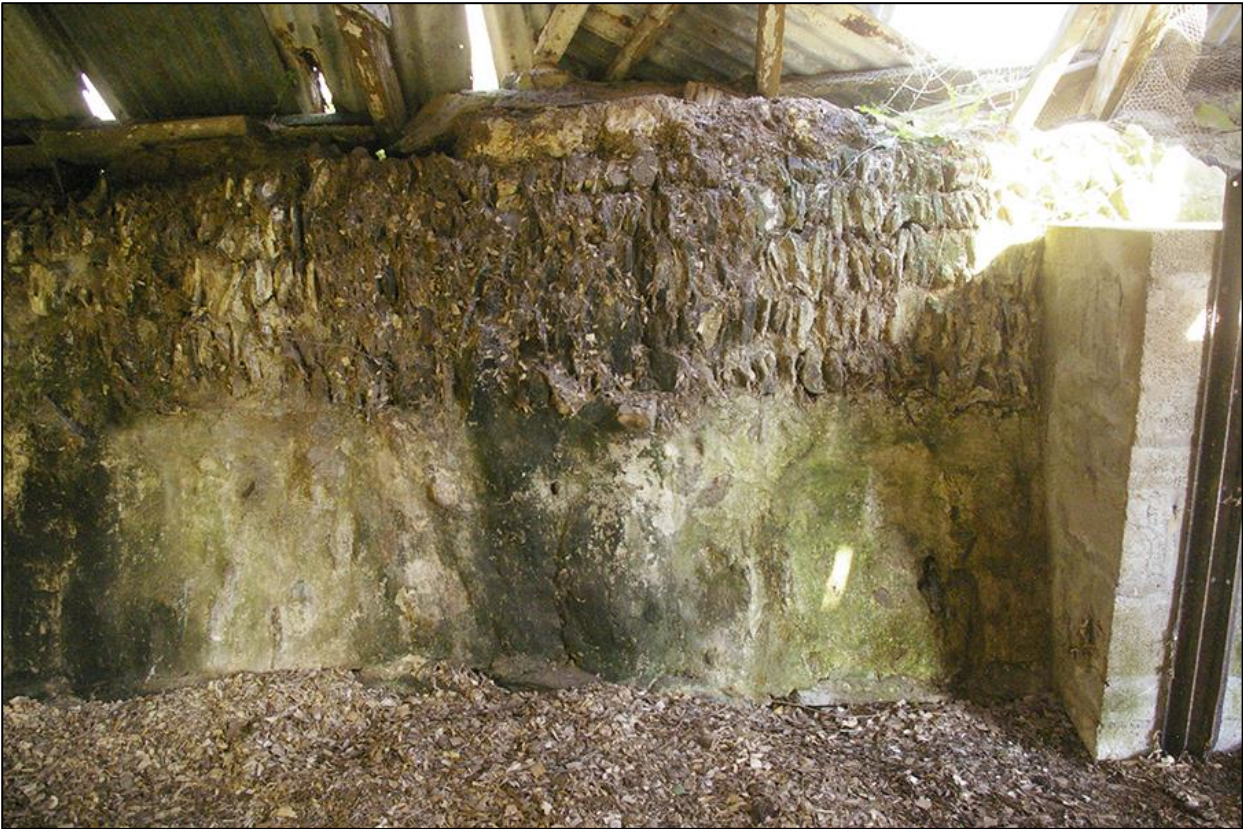
17. DETAIL OF THE MODIFIED FIELD BOUNDARY, PLASTERED/RENDERED WHERE IT FORMS PART OF THE STRUCTURE; VIEWED FROM THE SOUTH (NO SCALE).
