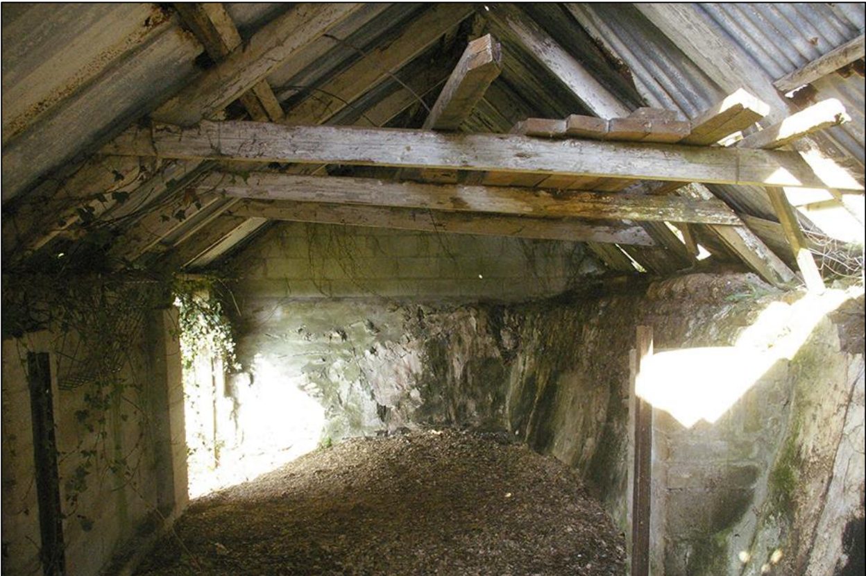
16. DETAIL OF THE ROOF STRUCTURE OVER THE WEST CELL OF THE STRUCTURE; VIEWED FROM THE EAST (NO SCALE).
