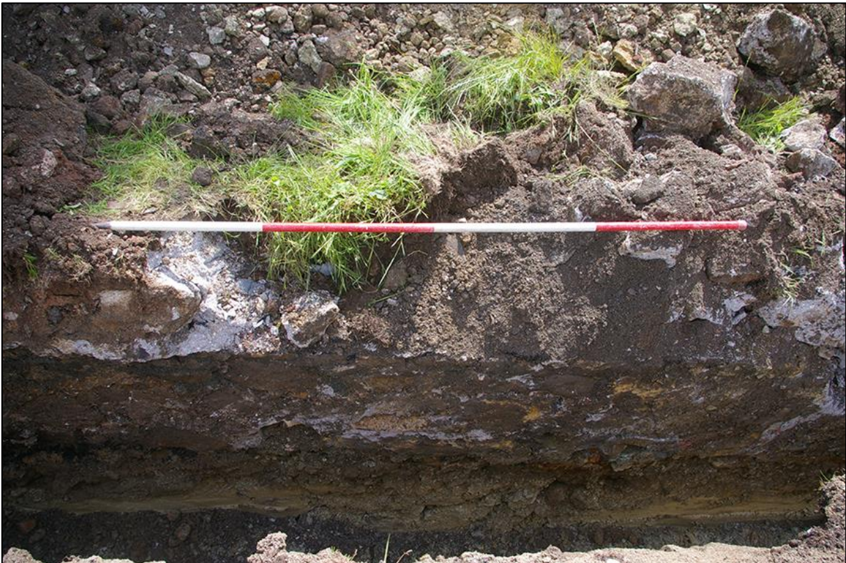
61. WALL {148}/{149} WITH REPAIR {147}, NORTH FACING ELEVATION; VIEWED FROM THE NORTH (2M SCALE).
