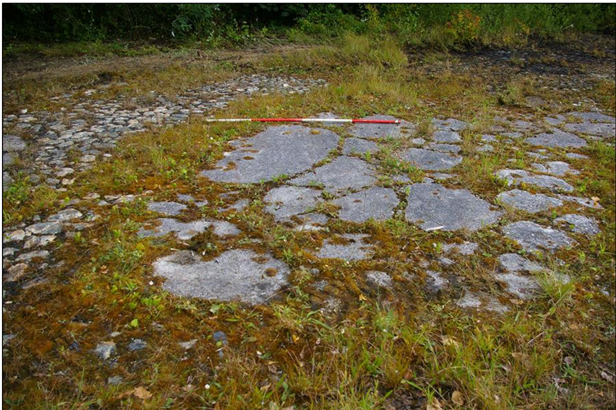
16. DETAIL OF COBBLE SURFACE (103) AND CONCRETE REPAIRS (100), SOUTH-WEST CORNER TO MIDDLE; VIEWED FROM THE SOUTH (2M SCALE).
