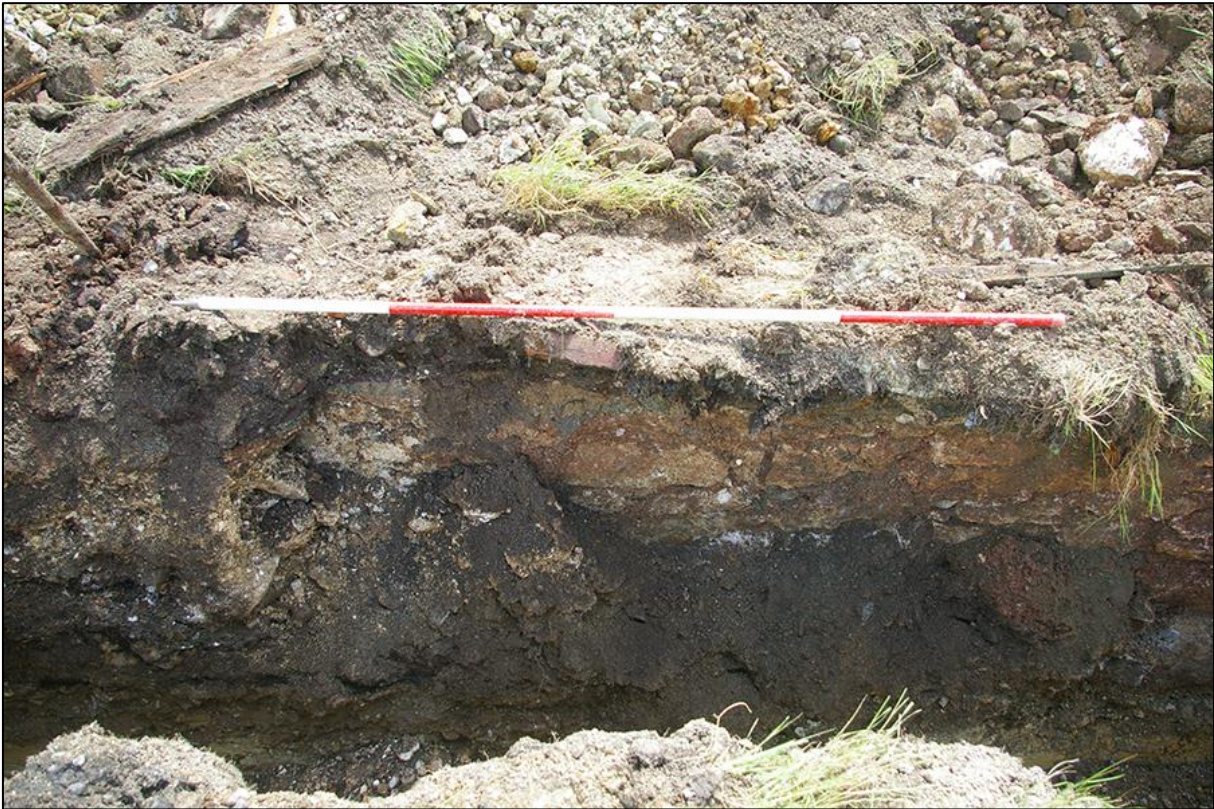
62. DETAIL OF WALL {148}/{149} WITH REPAIR {147}, NORTH FACING ELEVATION; VIEWED FROM THE NORTH (2M SCALE).
