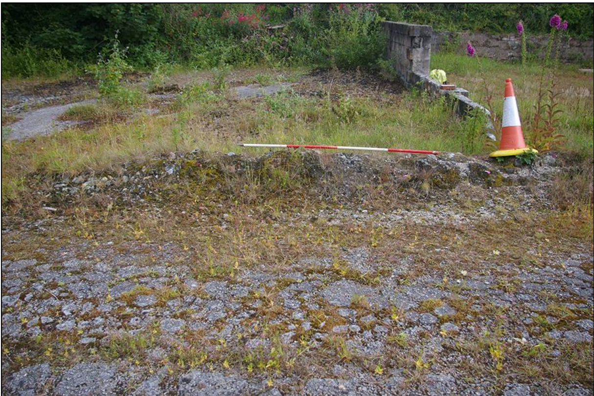
20. DETAIL OF COBBLE SURFACE (103) AND CONCRETE REPAIRS, SOUTH-EAST CORNER; VIEWED FROM THE SOUTH (2M SCALE).
