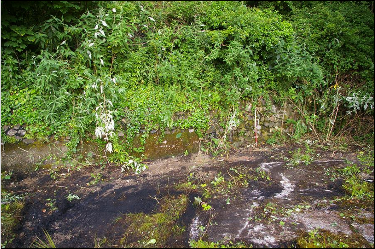
23. DETAIL OF STONE WALL FORMING CURRENT WEST SITE BOUNDARY; VIEWED FROM THE EAST (1M SCALE).
