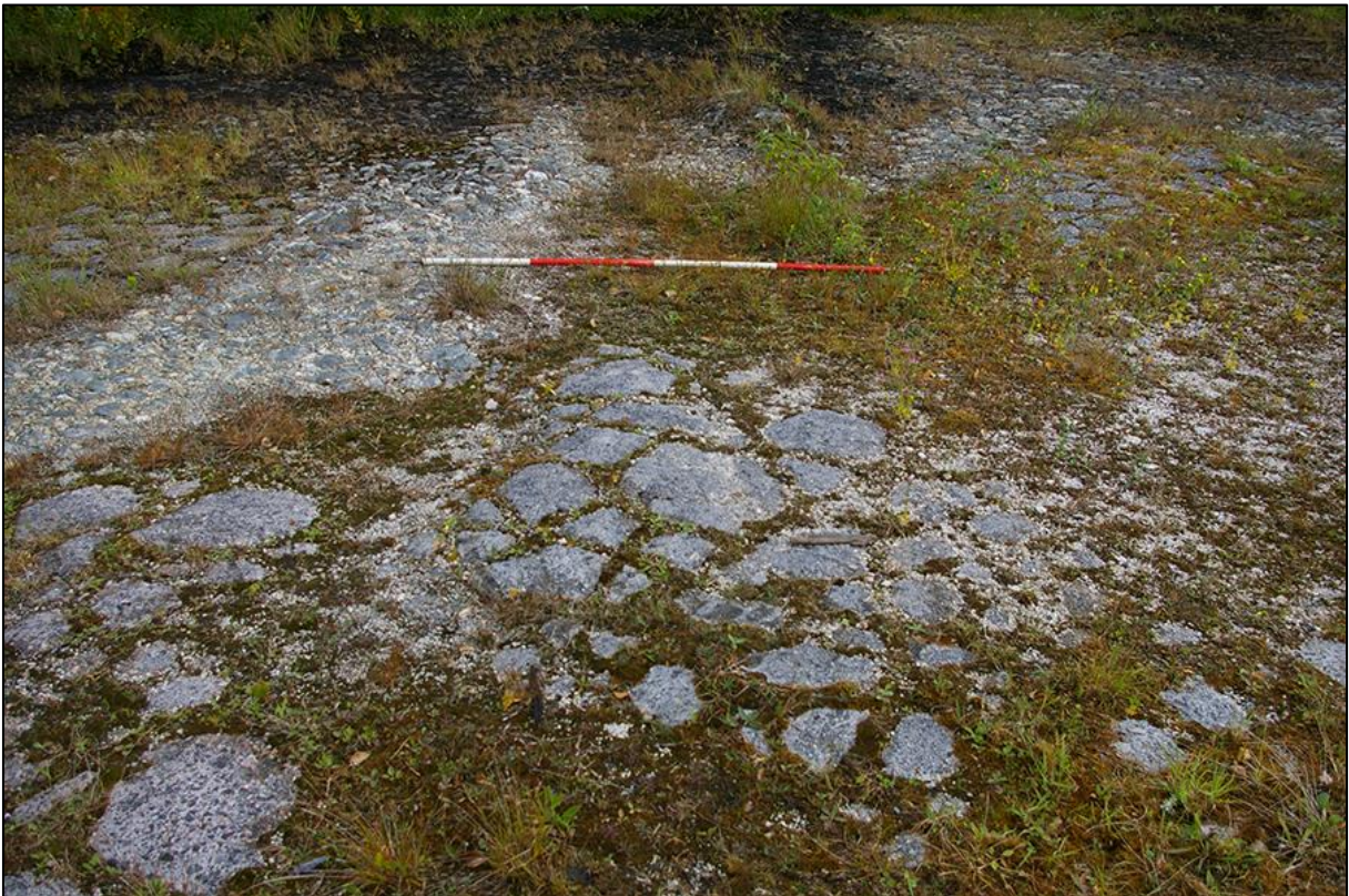
18. DETAIL OF COBBLE SURFACE (103) AND CONCRETE REPAIRS, MIDDLE; VIEWED FROM THE SOUTH (2M SCALE).
