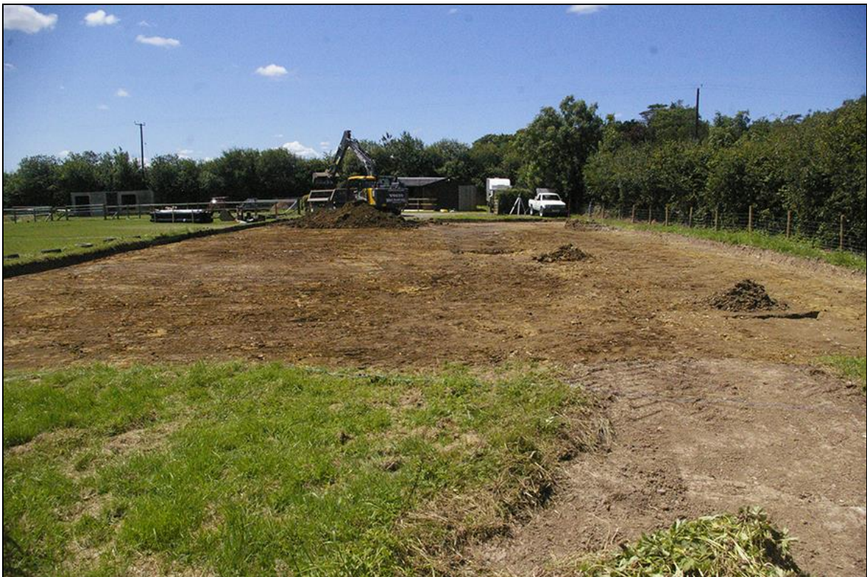
FIGURE 3: SITE SHOT, MID-EXCAVATION, SHOWING DITCHES [103] (RIGHT) AND [106], VIEWED FROM THE NORTH-EAST (NO SCALE).
