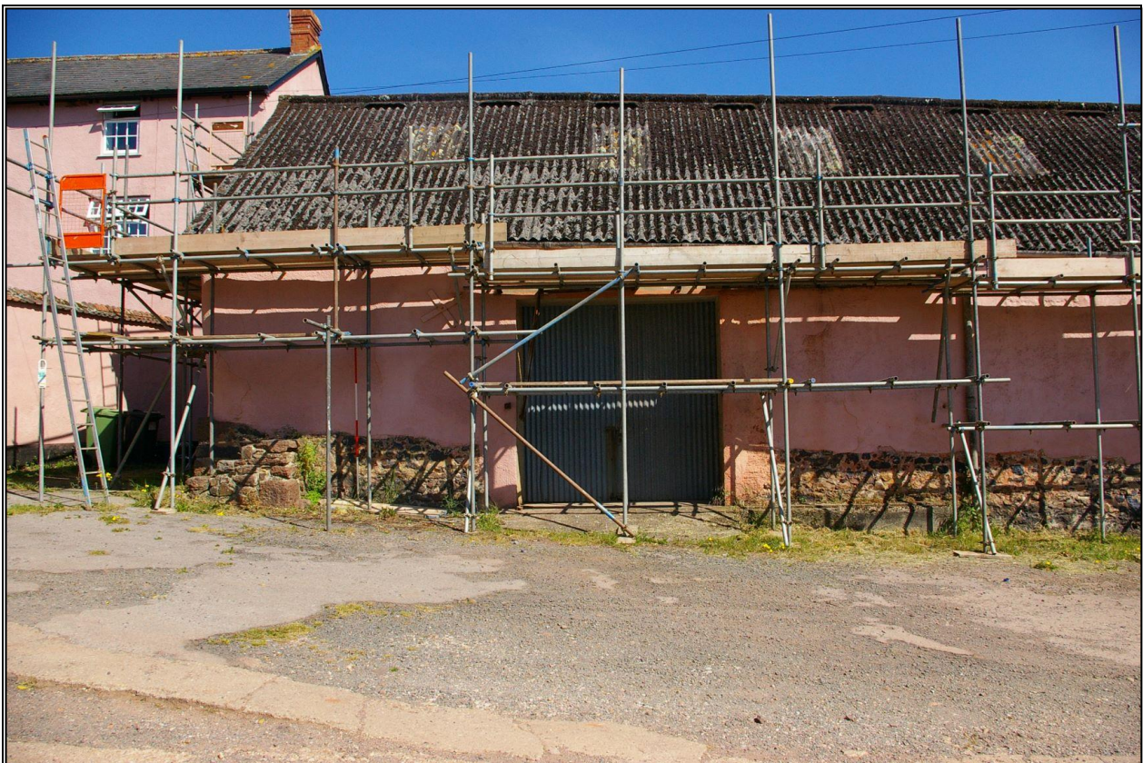
4. THE WESTERN END OF THE BARN (B1.1), WITH LARGER, BUT ALTERED THRESHING OPENING, WITH 2M SCALE; FROM THE SOUTH.
