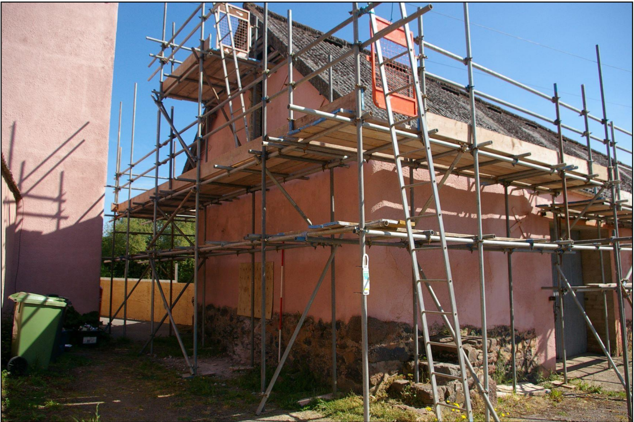
1. THE WEST GABLE ELEVATION OF THE MAIN BARN (B1.1) WITH 2M SCALE; FROM THE SOUTH-WEST.
