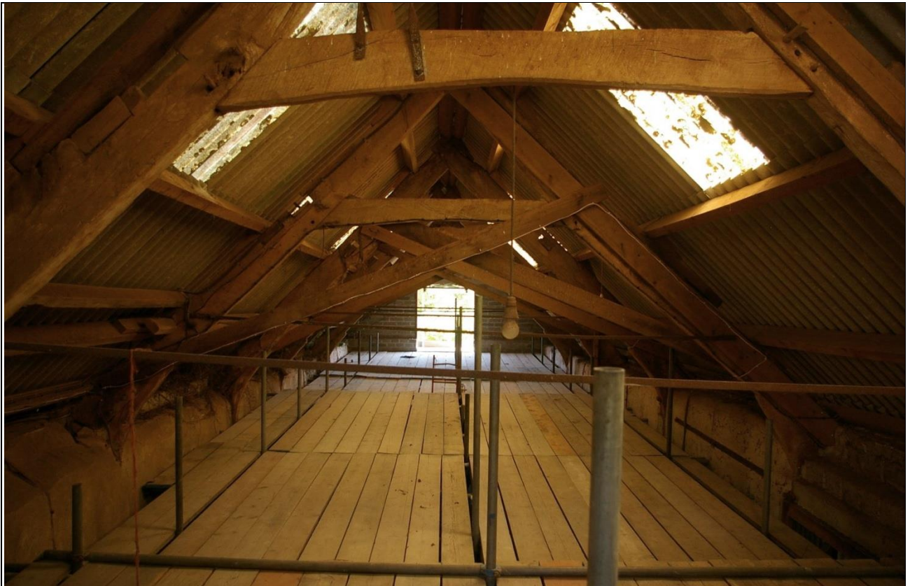
27. THE JOINTED CRUCK ROOF OF THE BARN, B1.1; FROM THE WEST, BAY 1, SHOWING THE DIFFERENT TRUSS TYPE FOR TRUSS 1 AND 2.
