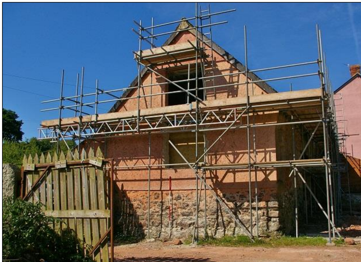
FIGURE 8: THE EAST REBUILT AND RENDERED GABLE OF THE BARN, WITH 2M SCALE; FROM THE EAST-NORTH-EAST.
