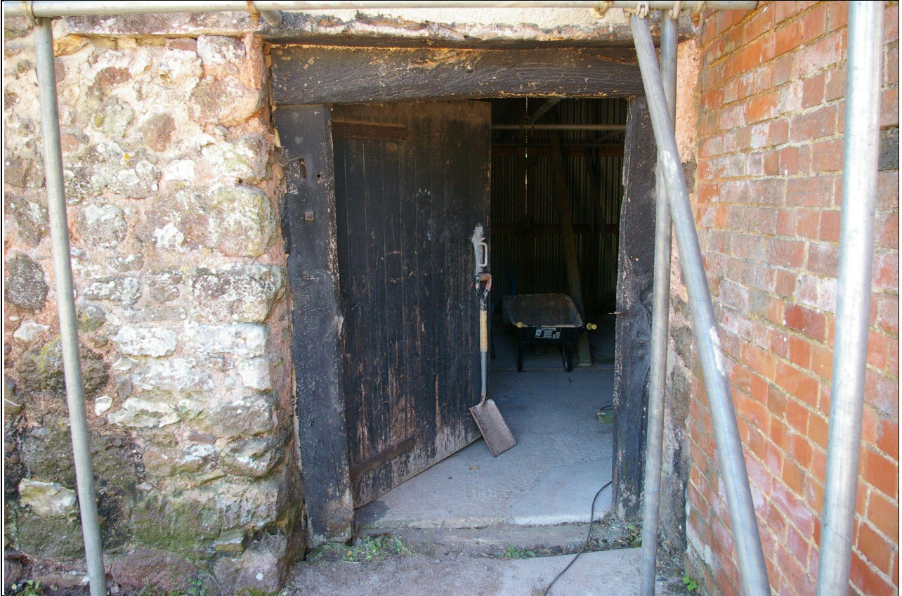
24. LARGE WEATHERED OAK LINTEL, OVER OPENING REDUCED IN SIZE, WITH INFILL OF RUBBLE STONE, WITH A RESET DOORFRAME, WITH VERY FINE CHAMFERED JAMBS, BUT CRUDELY CHAMFERED ROUGH LINTEL, WITH CHARRING FROM A FIRE AND DIFFERENT LEVELS OF WEATHERING, FORMING A WINNOWING DOOR FOR THRESHING; FROM THE
