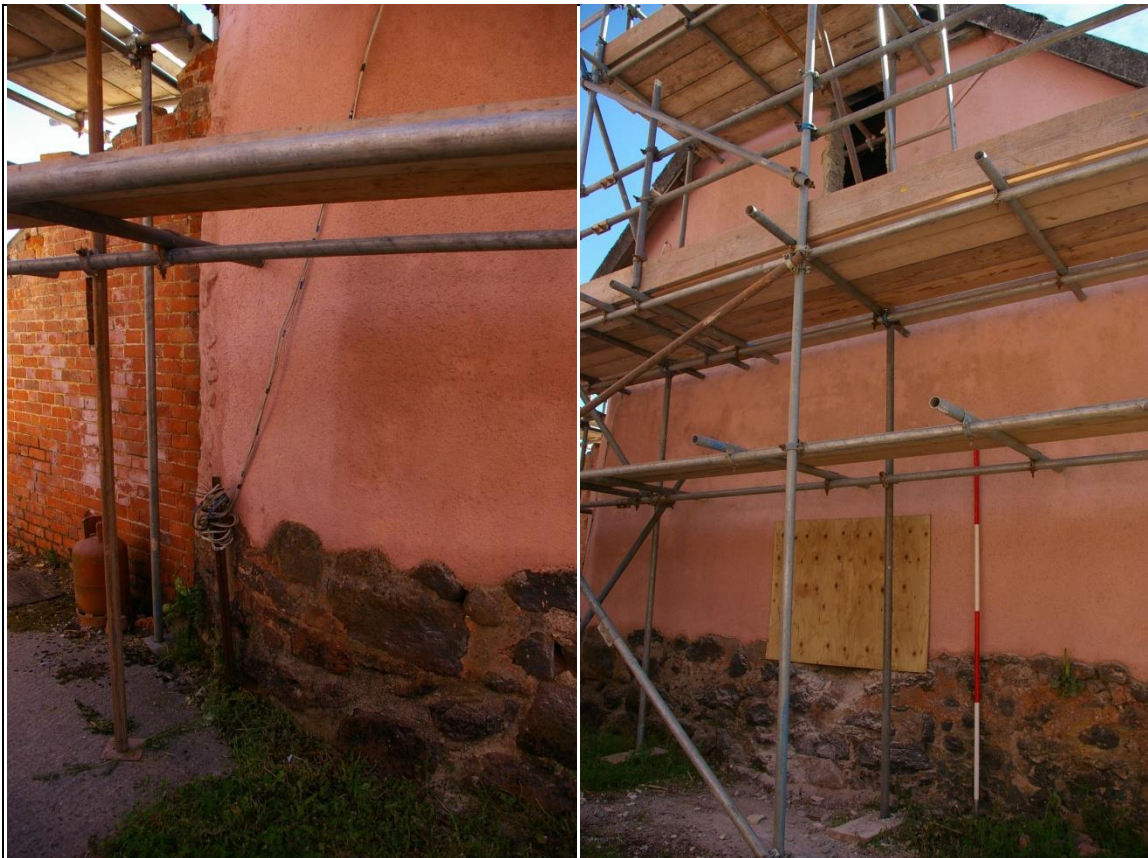
22. LEFT: THE NORTH-WEST CORNER OF THE BARN, RELIEVED AND REBUILT IN RENDERED STONE RUBBLE, ABUTTED BY THE BRICK OUTSHUT B1.3; FROM THE SOUTH-WEST.
