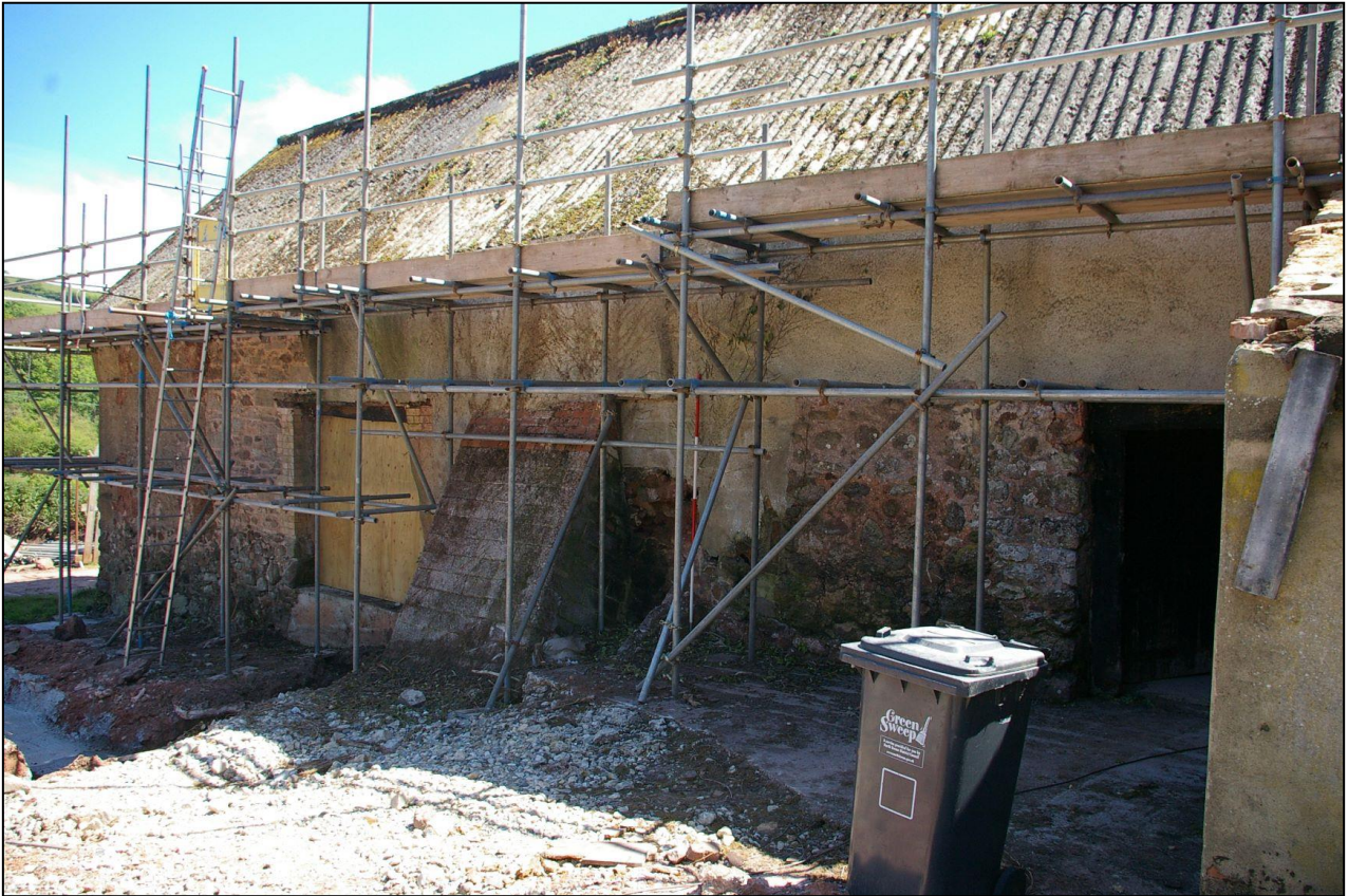
17. THE NORTH ELEVATION OF B1.1, THE MAIN BARN, WITH 2M SCALE; FROM THE NORTH-WEST.
