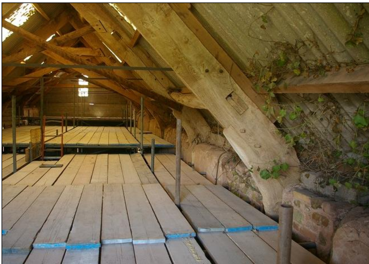
FIGURE 16: DETAIL OF PART OF THE ROOF OVER B1.1, THE JOINTED CRUCKS, SHOWING THE SHAPED FOOT PEGGED TO THE CRUCK BLADE AND ONE OF THE SURVIVING HEAVY PURLINS; FROM THE EAST.
