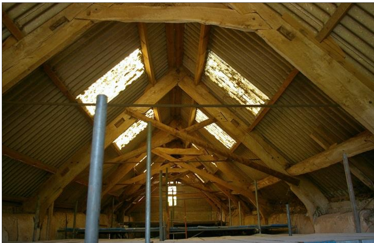
FIGURE 10: THE ROOF OVER B1.1 IS OF FIVE JOINTED CRUCK TRUSSES; SOME OF THESE HAVE LATER SCISSOR BRACES ATTACHED; THERE IS ONE ADDITIONAL MODERN A-FRAME TO THE WEST END.
