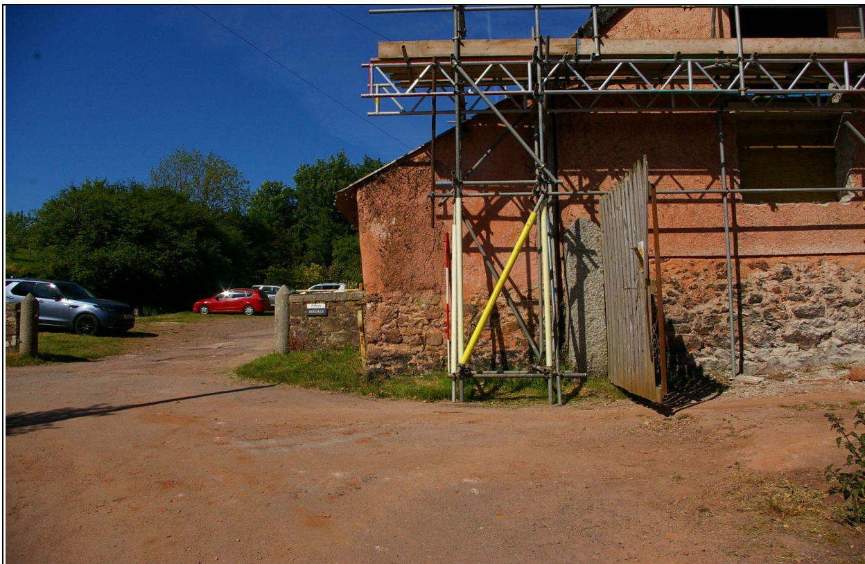
11. THE EQUIPMENT SHED (B1.2), WHERE IT ABUTS THE MAIN BARN (B1.1), WITH 2M SCALE; FROM THE EAST.
