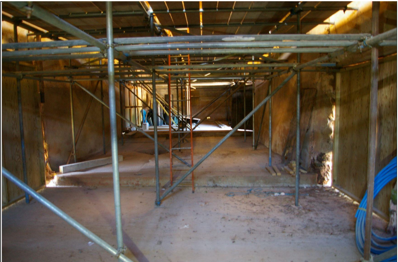
25. THE INTERIOR OF THE MAIN BARN B1.1, WITH IN SITU SCAFFOLDING; FROM THE EAST.
