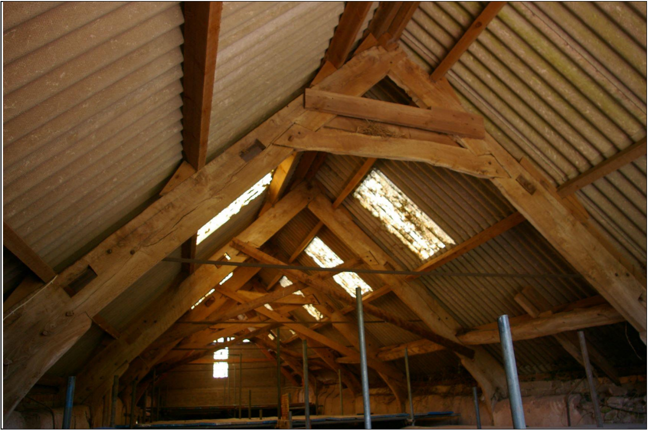
26. THE JOINTED CRUCK ROOF STRUCTURE OF B1.1, THE MAIN BARN; FROM THE SOUTH-EAST CORNER, BAY 6.
