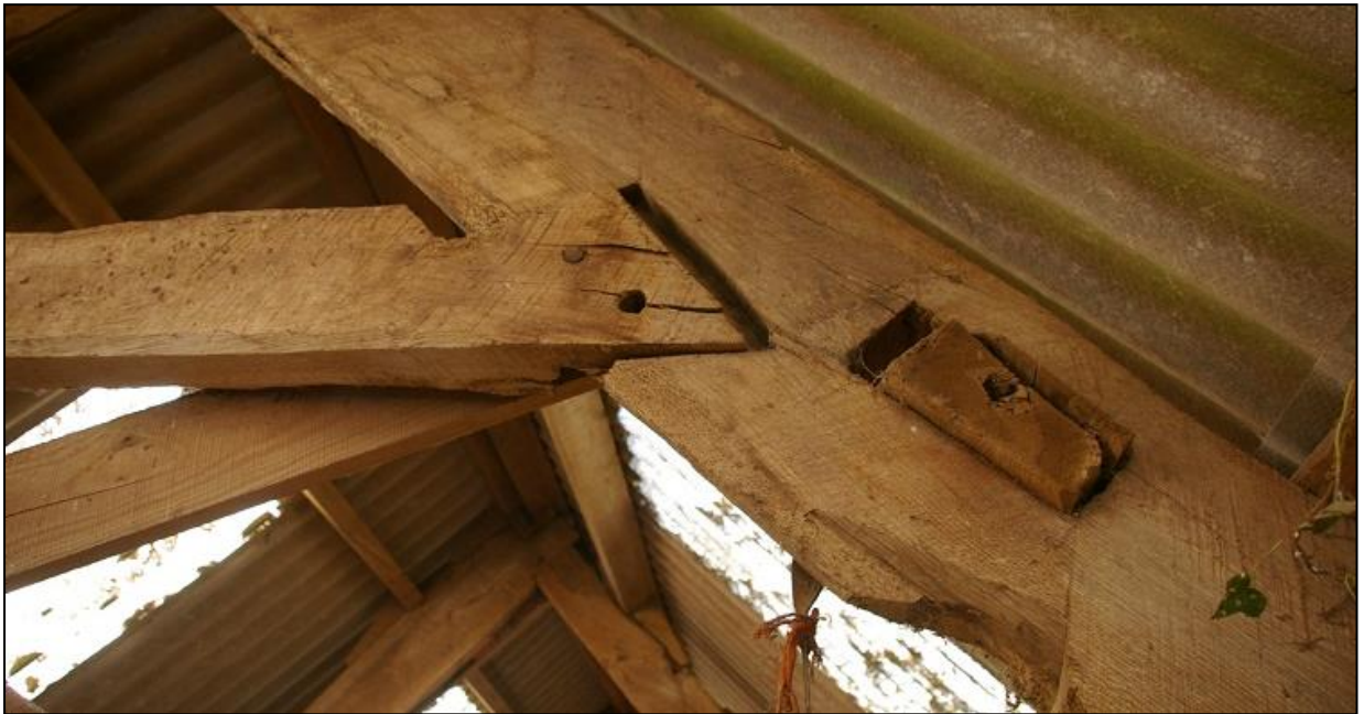
FIGURE 14: DETAIL OF ONE OF THE DOVETAILED COLLAR JOINTS AND THREADED PURLINS SOCKETS; FROM THE EAST.
