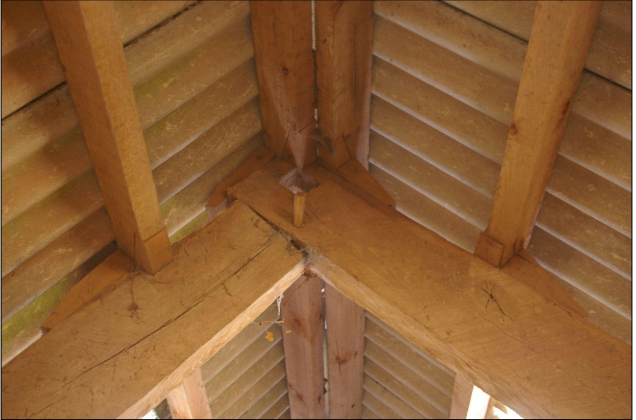
28. UNALTERED RIDGE, SHOWING THE RIDGE POLE WAS ORIGINALLY THREADED; FROM THE WEST, TRUSS 4.
