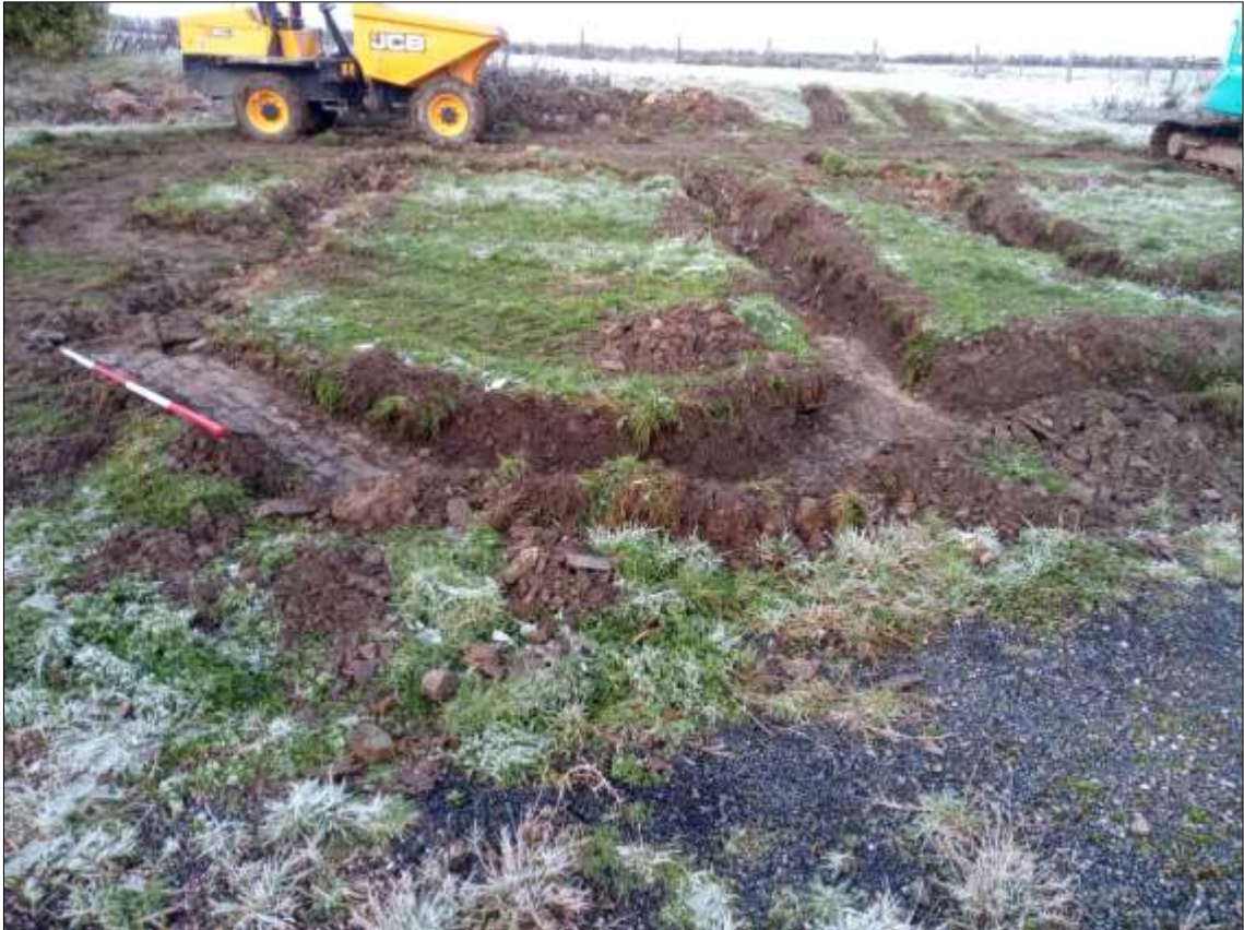
FIGURE 9: PLAN OF SOUTH-WEST CORNER OF SITE, WITH COBBLES (109), (110) AND CONCRETE REPAIR; FROM THE SOUTH (2M SCALE).
