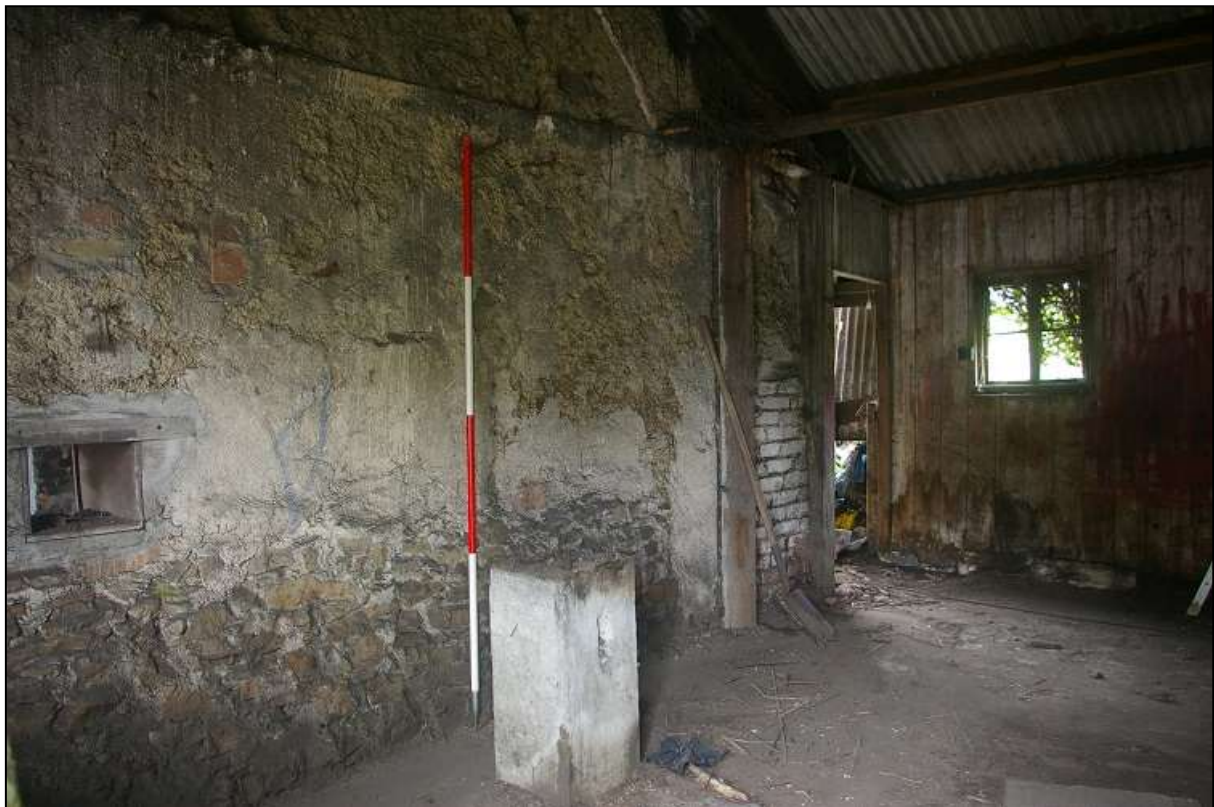
FIGURE 8: ROOM 1B INTERIOR OF THE EXTENSION TO THE OLD FORGE, FROM THE SOUTH-WEST (2M SCALE).
