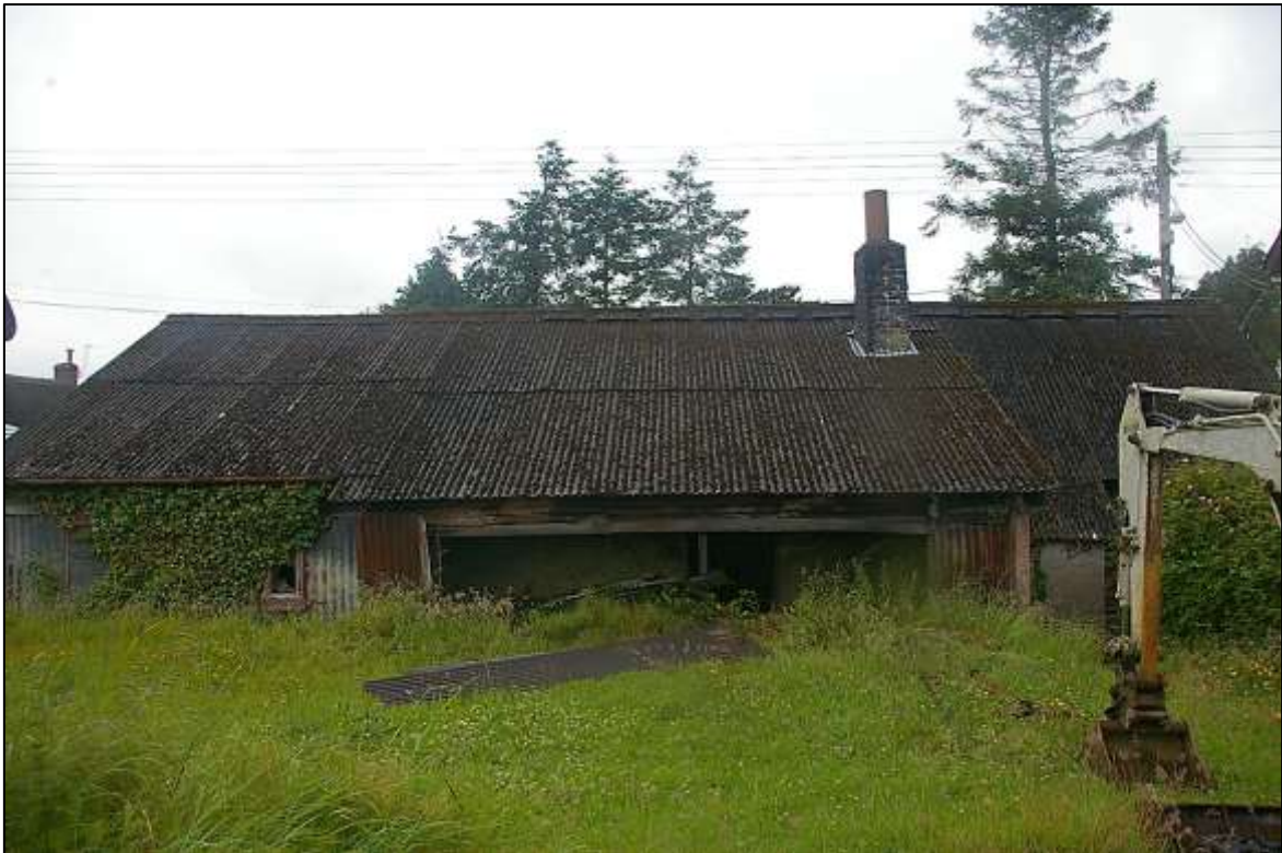
1. THE REAR, EAST ELEVATION OF THE OLD FORGE BUILDING, SHOWING THE VERANDA AND REAR BRICK STACK TO THE FORGE; FROM THE EAST.
