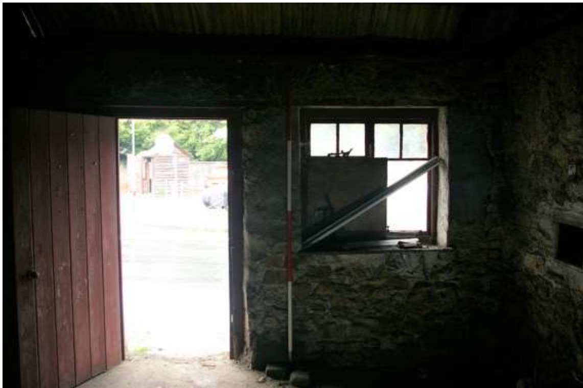
24. THE SOUTH END OF THE WEST WALL, WITH 2M SCALE; FORM THE EAST.
