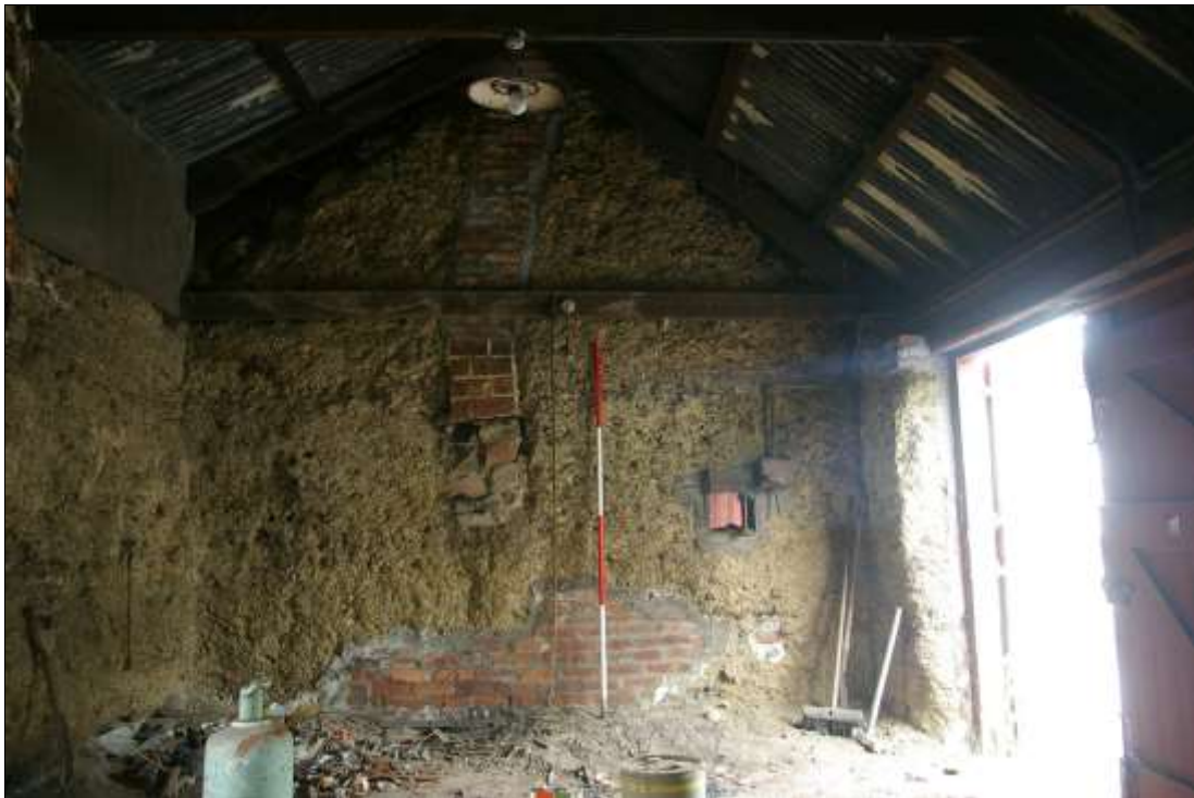
10. THE INTERIOR FACE OF THE SOUTH GABLE, WITH 2M SCALE; FORM THE NORTH.
