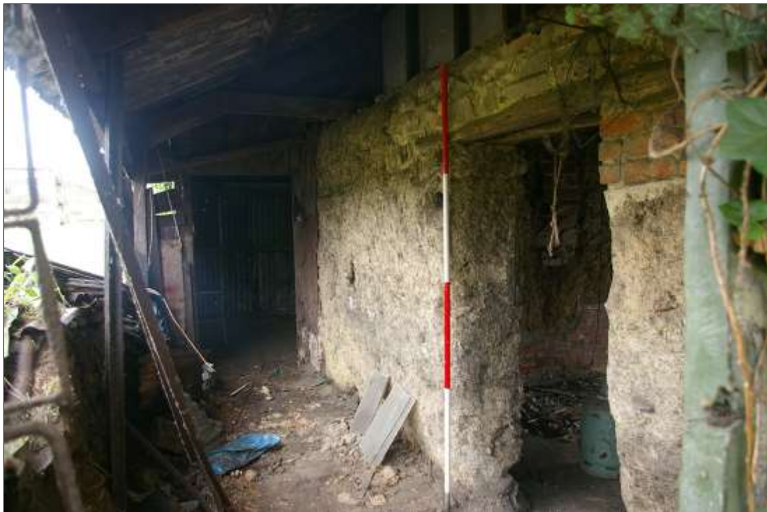
20. THE VERANDA AND EXPOSED COB WALL WITHIN, WITH 2M SCALE (D2) AND (D5); FROM THE NORTH-EAST.
