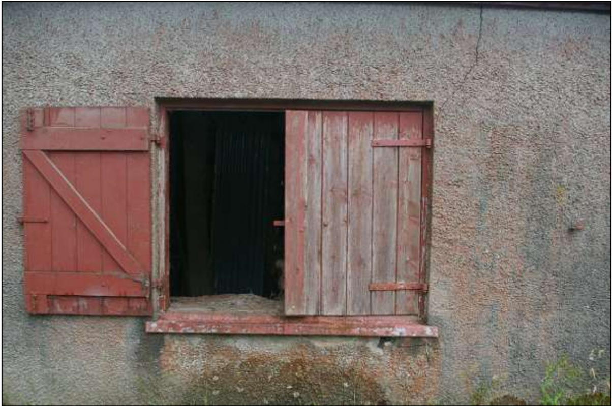
4. THE HATCH W1 IN THE FRONT WEST WALL OF THE BUILDING; FROM THE WEST.
