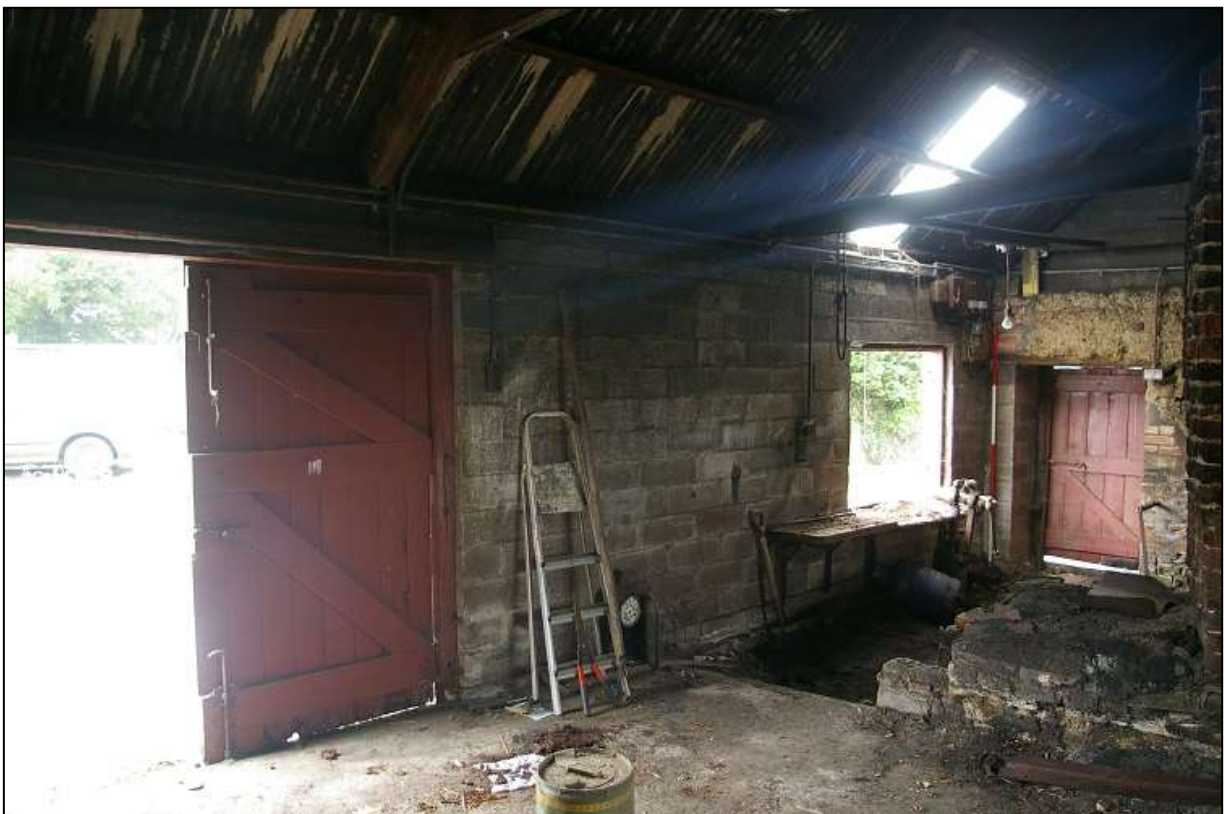
FIGURE 7: THE INTERIOR OF THE OLD FORGE, ROOM 1A, WITH 2M SCALE; FROM THE SOUTH-EAST.
