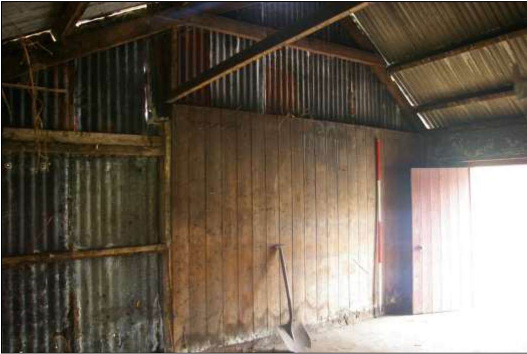
21. THE BOARDED AND CORRUGATED STRUCTURE WHICH FORMS R1B, WITH 2M SCALE; FROM THE NORTH-EAST.
