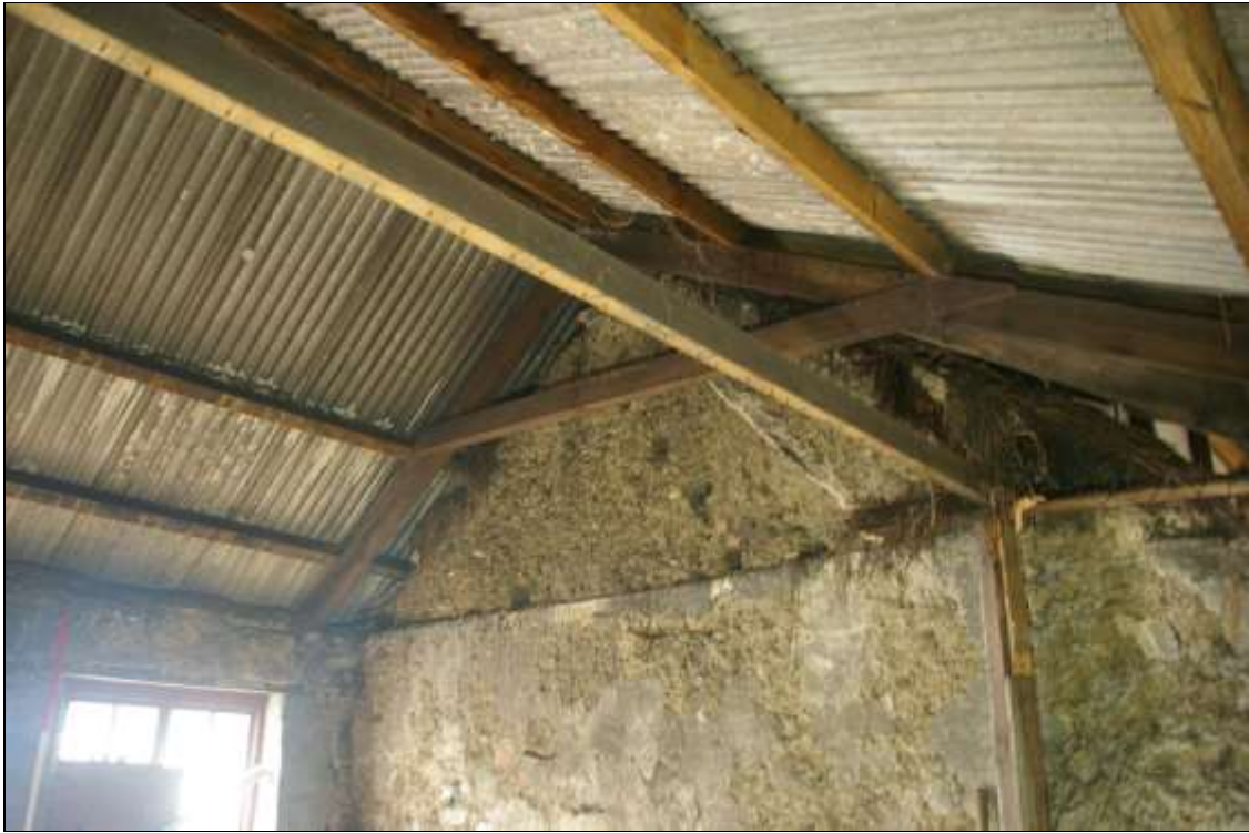
25. ROOFLINE SCAR OF FORMER OUTSHUT TO COB GABLE WITHIN R1B; FROM THE SOUTH-EAST.
