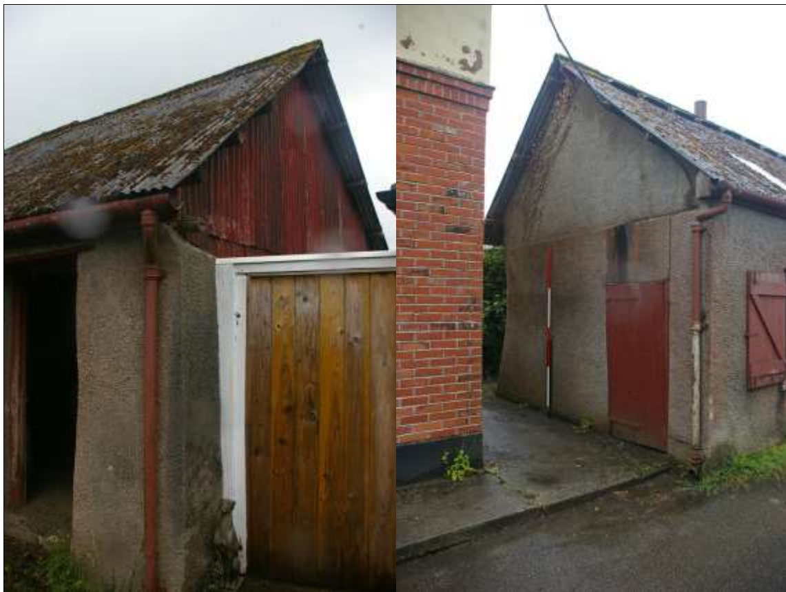
2. LEFT: THE SOUTH GABLE OF THE EXTENSION, WITH CORRUGATED SHEETING C 1940S; FROM THE SOUTH-WEST. 3. RIGHT: THE NORTH GABLE, RENDERED, WITH D3, 2M SCALE; FROM THE NORTH-WEST.
