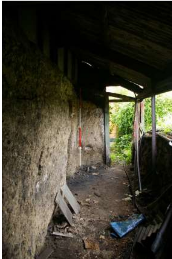
19. THE LATERAL STACK, WITH 2M SCALE; FROM THE SOUTH, SHOWING THE SLOPING PROFILE OF THE SURVIVING THATCHED ROOF.
