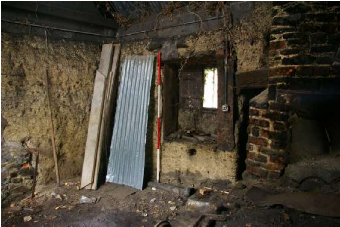
17. THE WINDOW (W2) FROM THE INTERIOR, WITH 2M SCALE; FROM THE SOUTH-WEST.
