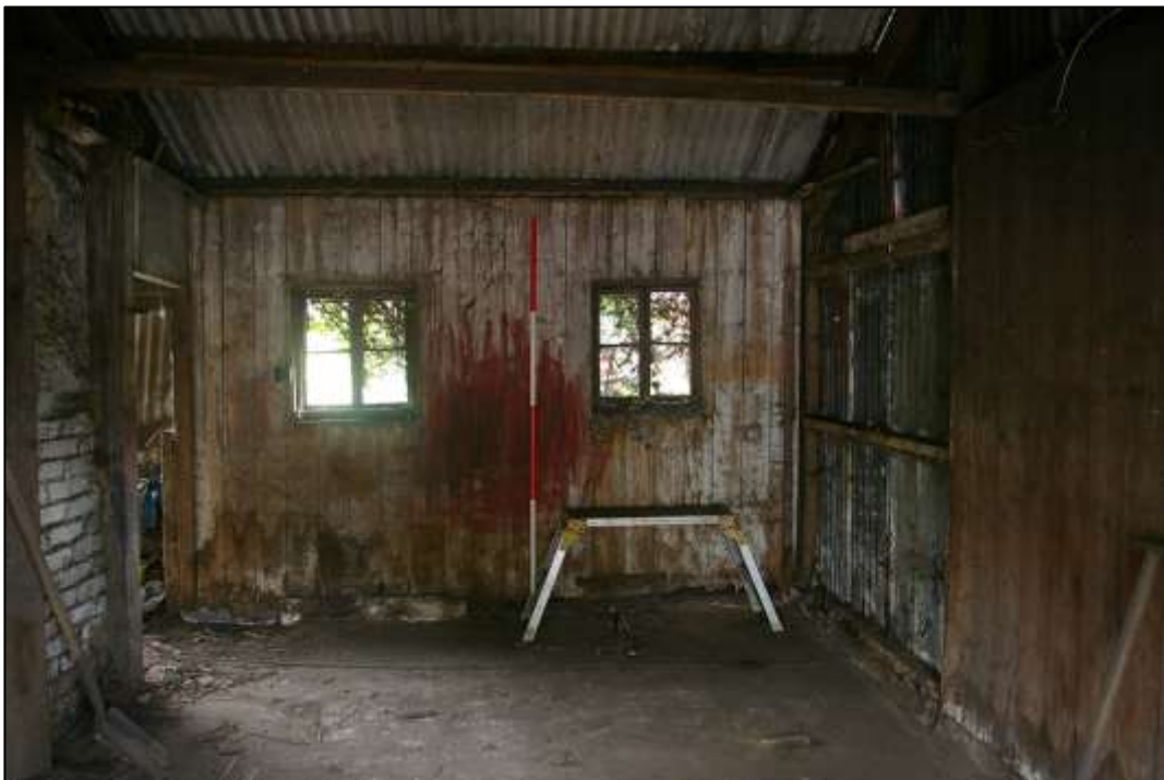
22. THE BOARDED AND CORRUGATED STRUCTURE WHICH FORMS R1B, WITH 2M SCALE; FROM THE WEST.
