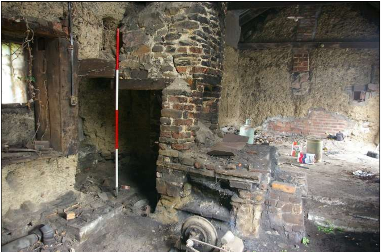
FIGURE 9: THE RELATIONSHIP OF THE FORGE AND EARLIER FIREPLACE IN ROOM 1A; FROM THE NORTH-WEST, WITH 2M SCALE.
