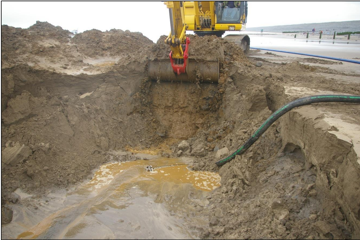
1. TRENCH 01, WORKING SHOT DEMONSTRATING THE LEVEL OF WATER INUNDATION AND SAND 'WASH-OUT' AND COLLAPSE; VIEWED FROM THE SOUTH.
