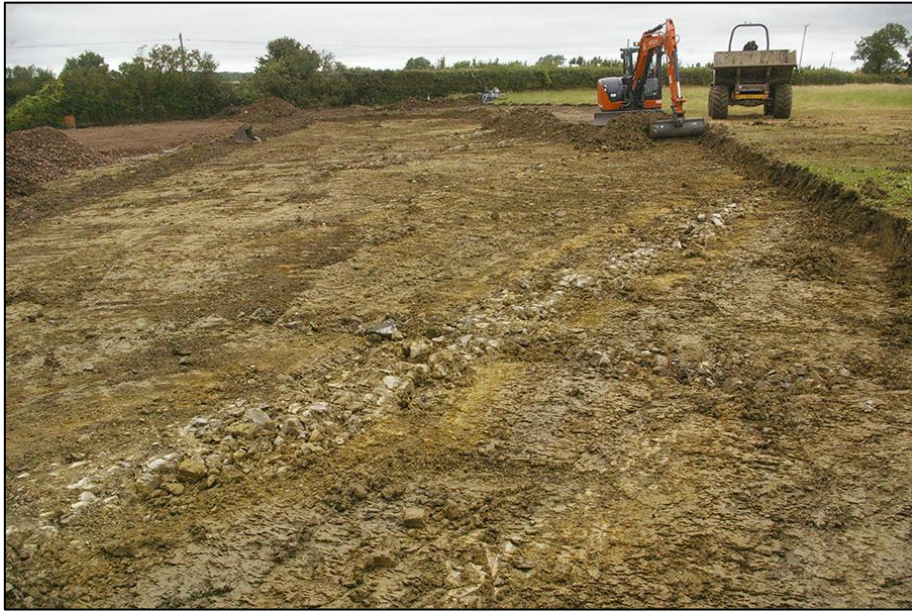
FIGURE 2: EAST HALF OF THE SITE MID-EXCAVATION; VIEWED FROM THE SOUTH-SOUTH-EAST (NO SCALE).
