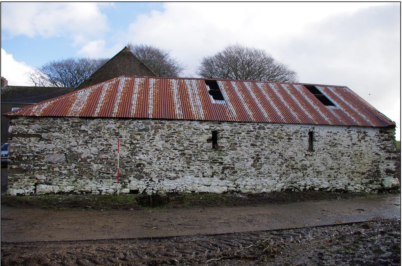
72. THE WEST ELEVATION OF THE SHIPPON; VIEWED FROM THE WEST (SCALE 2M).
