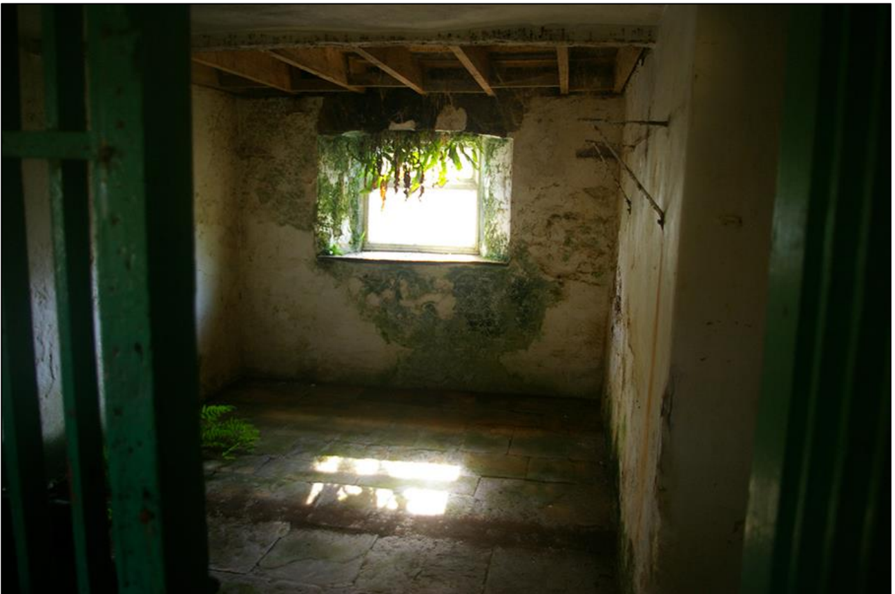
24. R5, DETAIL OF R5C AND ITS FINE SLATE FLAGSTONE FLOOR; VIEWED FROM THE NORTH.
