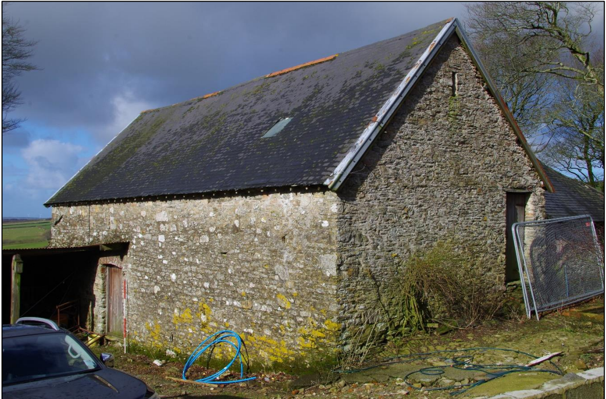
FIGURE 19: THE SOUTH AND EAST ELEVATIONS OF THE THRESHING BARN (B2.1); VIEWED FROM THE SOUTH-EAST.
