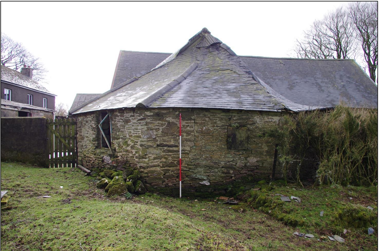
48. THE NORTH ELEVATION OF THE HORSE ENGINE HOUSE; VIEWED FROM THE NORTH (SCALE 2M).
