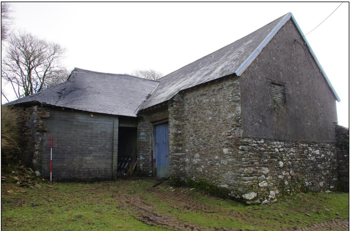
FIGURE 20: THE NORTH AND WEST ELEVATIONS OF THE THRESHING BARN (B2.1) AND HORSE ENGINE HOUSE (B2.2); VIEWED FROM THE WNW (SCALE 2M).
