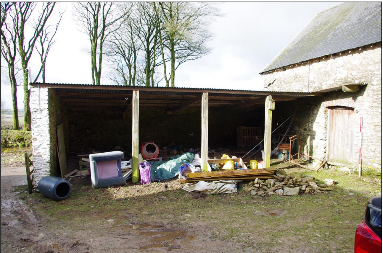
54. THE EAST ELEVATION OF THE CARTSHED; VIEWED FROM THE EAST (SCALE 2M).
