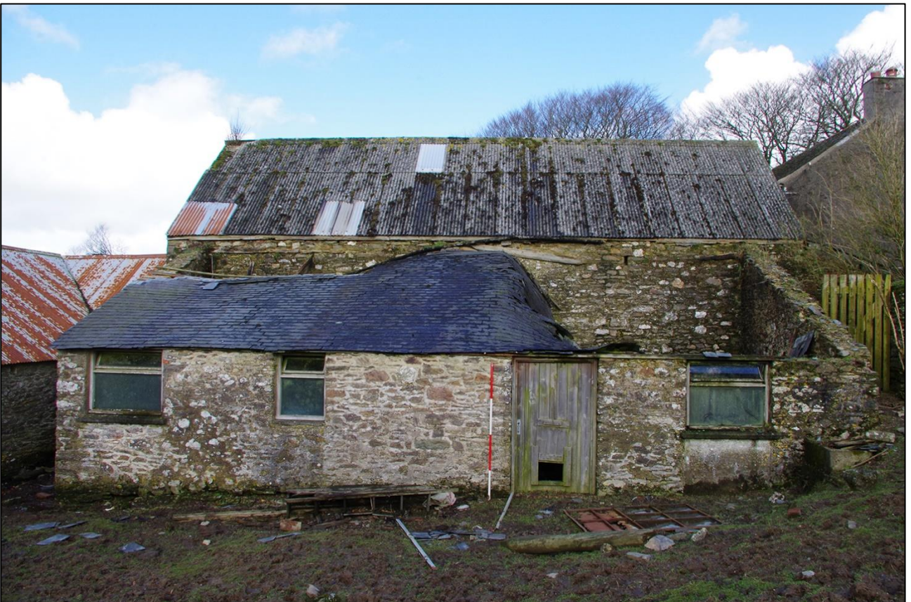
76. THE SOUTH ELEVATIONS OF THE STABLES AND THE MILKING PARLOUR; VIEWED FROM THE SOUTH (SCALE 2M).
