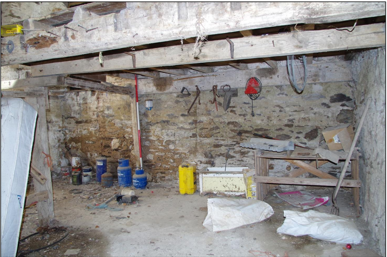
62. THE EAST END OF THE THRESHING BARN, WITH 17 TH CENTURY CHAMFERED ABOVE; VIEWED FROM THE WEST (SCALE 2M).
