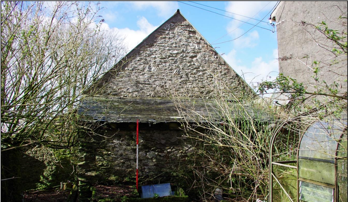
FIGURE 26: THE EAST ELEVATION OF LEAN-TO B3.4, WITH THE GABLE OF B3.1 BEHIND; VIEWED FROM THE EAST (SCALE 2M).
