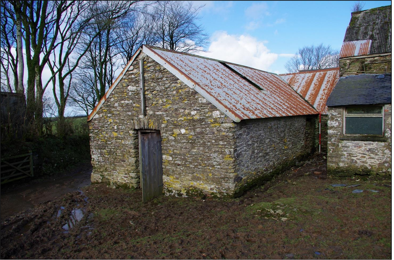
75. THE SOUTH AND EAST ELEVATIONS OF THE SHIPPON; VIEWED FROM THE SOUTH-EAST (SCALE 2M).
