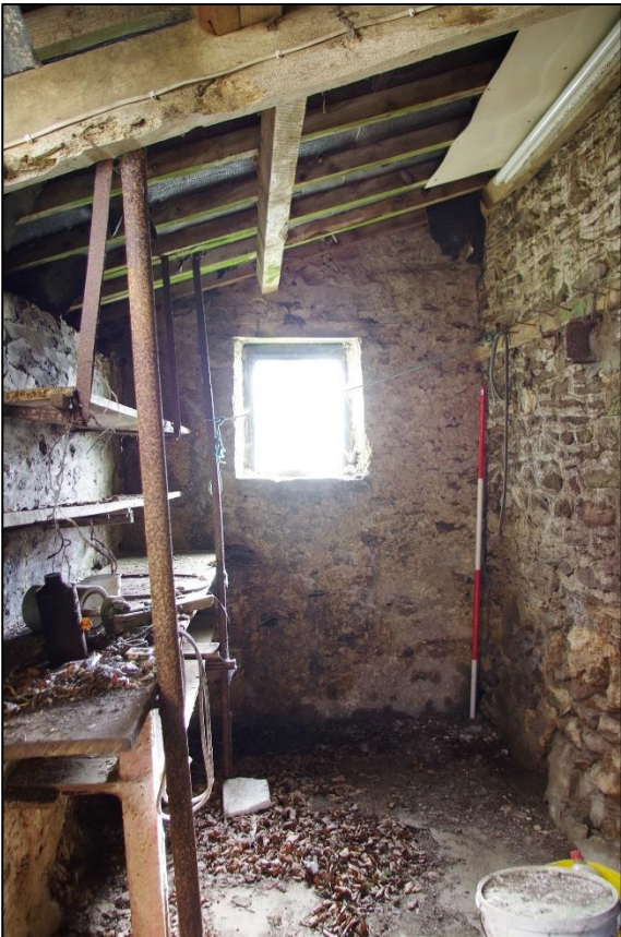
85. THE INTERIOR OF THE TACK ROOM (B3.4); VIEWED FROM THE NORTH (SCALE 2M).
