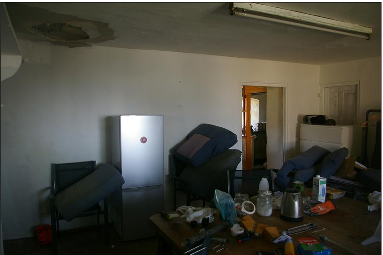
15. R4, THE EAST WALL WITH DOORWAY LEADING THROUGH INTO R5A; VIEWED FROM THE NORTH-WEST.
