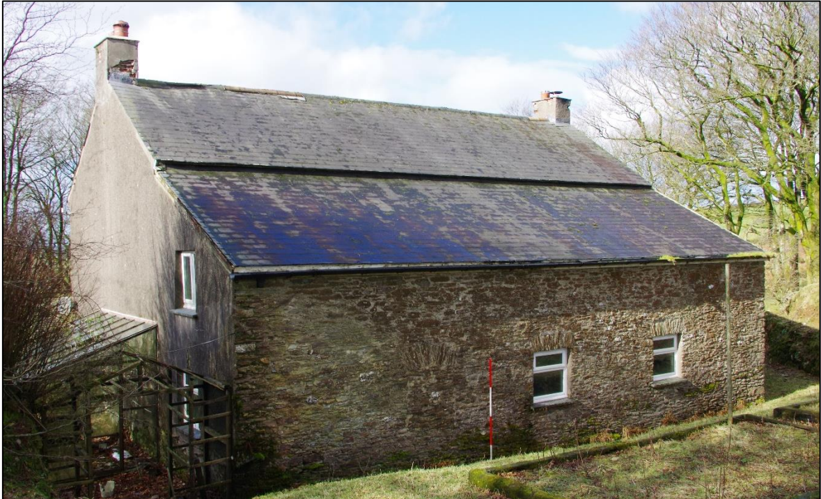
FIGURE 16: THE REAR (EAST) ELEVATION OF THE FARMHOUSE (B1.1); VIEWED FROM THE ESE (SCALE 2M).
