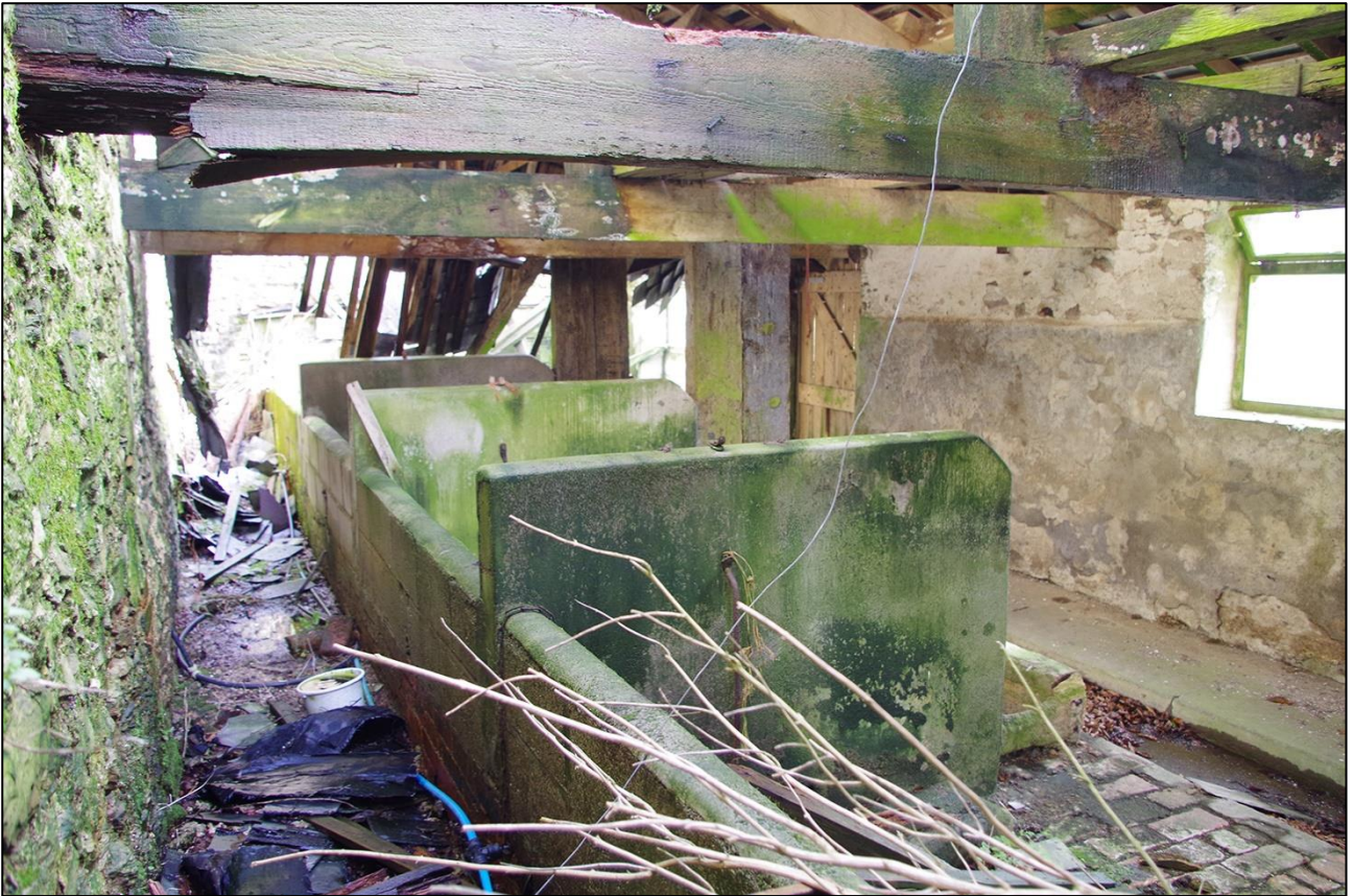
93. THE INTERIOR OF THE MILKING PARLOUR, SHOWING THE CATTLE STALLS; VIEWED FROM THE WNW.
