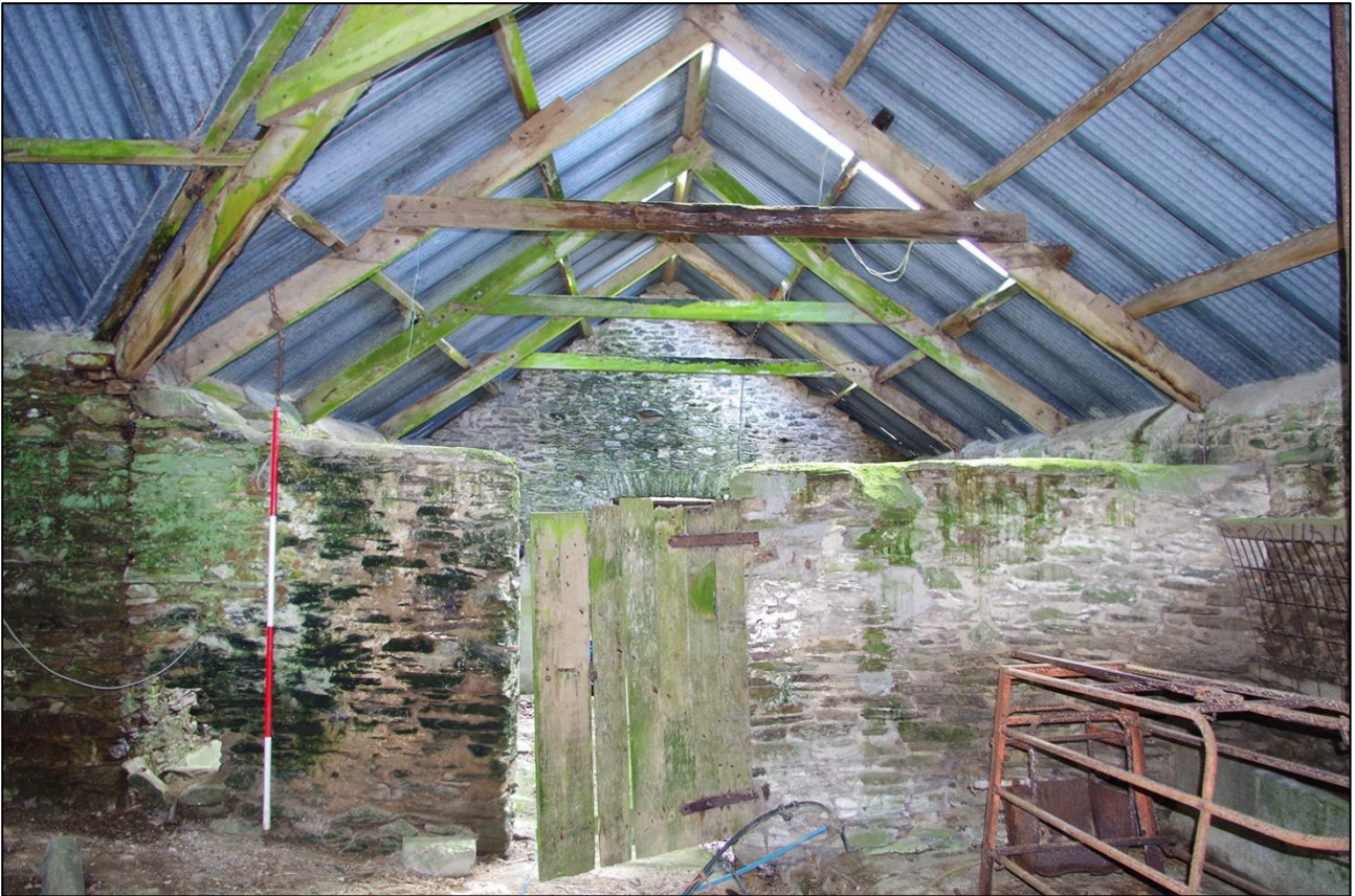
91. THE INSERTED WALL WITHIN THE SHIPPON; VIEWED FROM THE NORTH (SCALE 2M).
