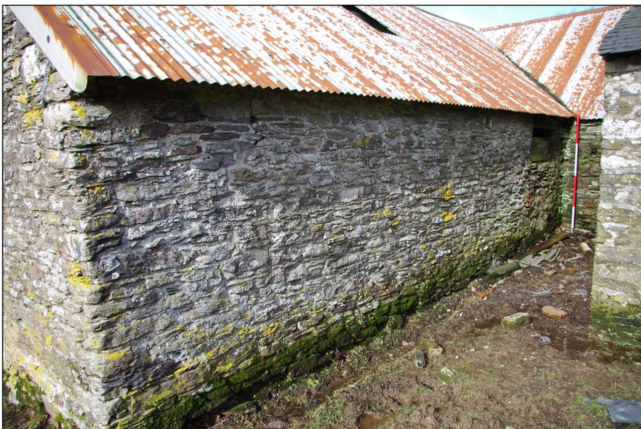
74. THE EAST ELEVATION OF THE SHIPPON; VIEWED FROM THE SOUTH-EAST (SCALE 2M).
