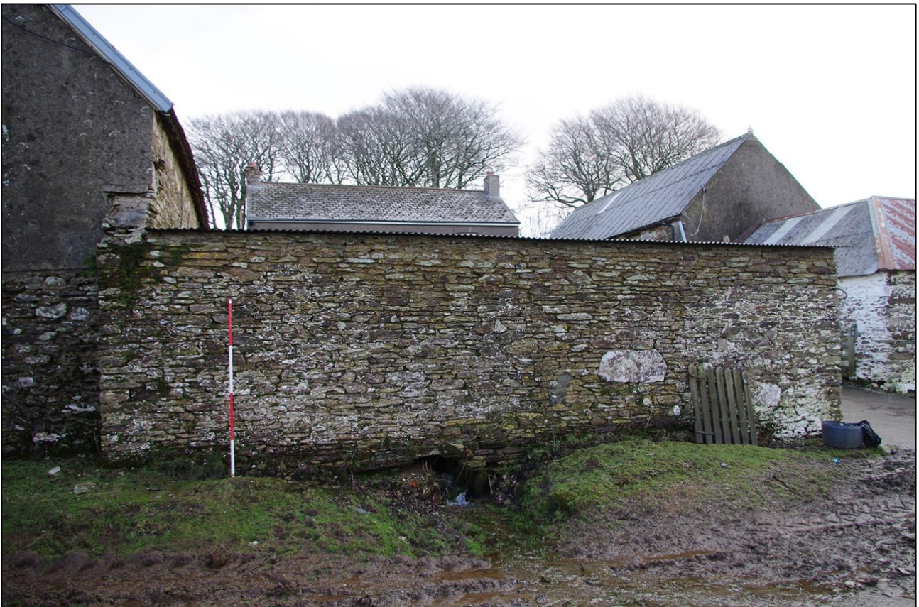
50. THE WEST ELEVATION OF THE CARTSHED; VIEWED FROM THE WEST (SCALE 2M).
