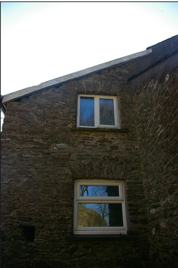
4. THE NORTH ELEVATION OF THE DAIRY ATTACHED TO THE REAR OF THE FARMHOUSE; VIEWED FROM THE NORTH.
