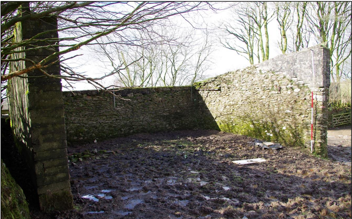
FIGURE 27: THE BARE WALLS OF THE OUTBUILDING B4; VIEWED FROM THE ENE (SCALE 2M).
