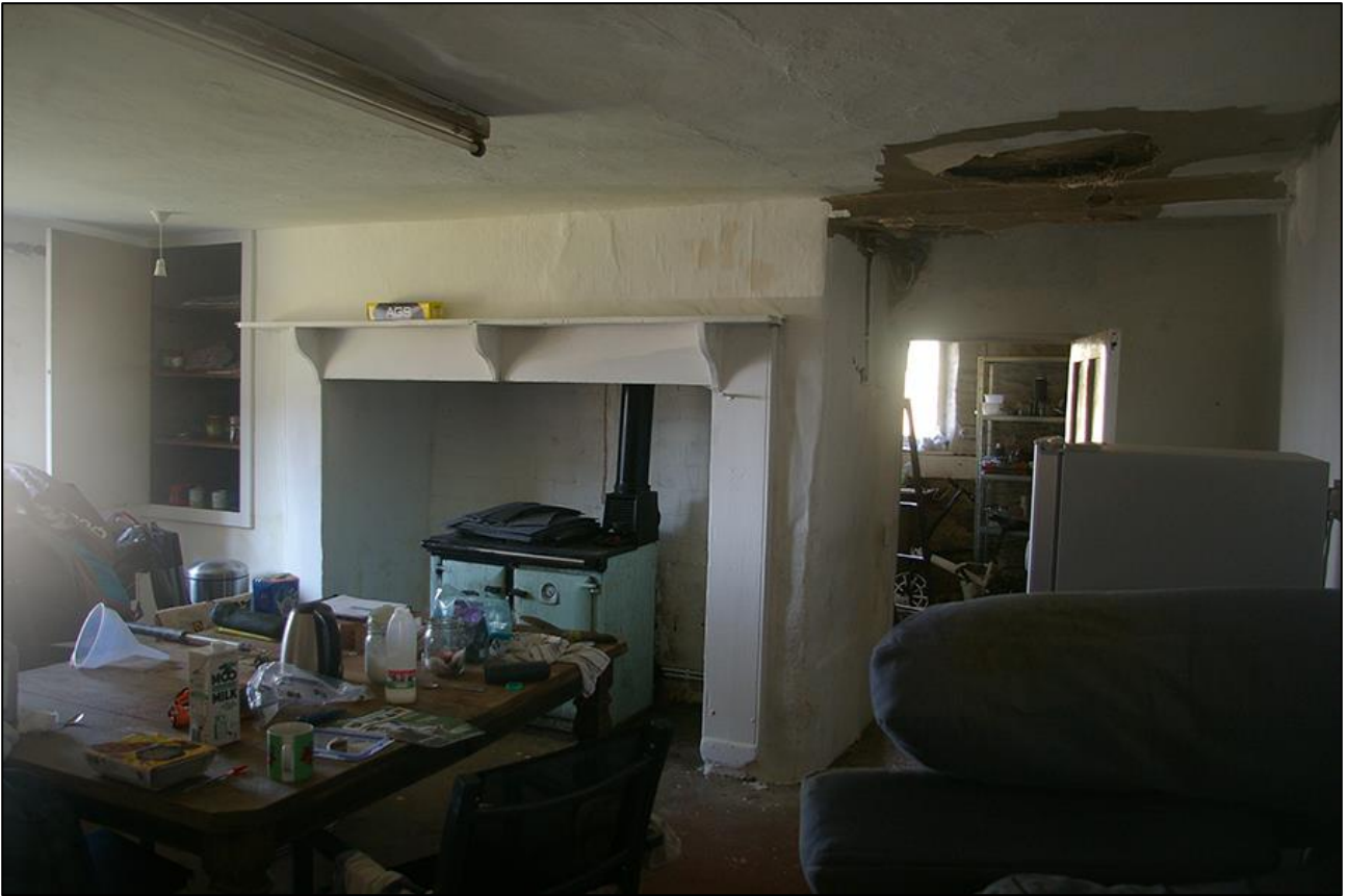
14. R4, THE LARGE HEARTH AND DOOR THROUGH INTO R6; VIEWED FROM THE SOUTH.
