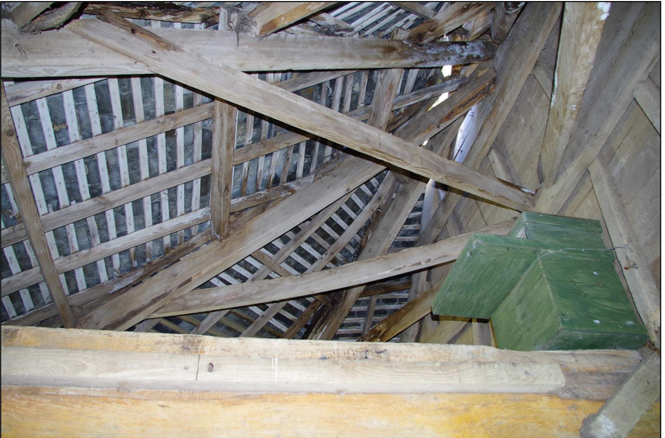
66. THE ROOF STRUCTURE IN THE HORSE ENGINE HOUSE; VIEWED FROM THE WEST.
