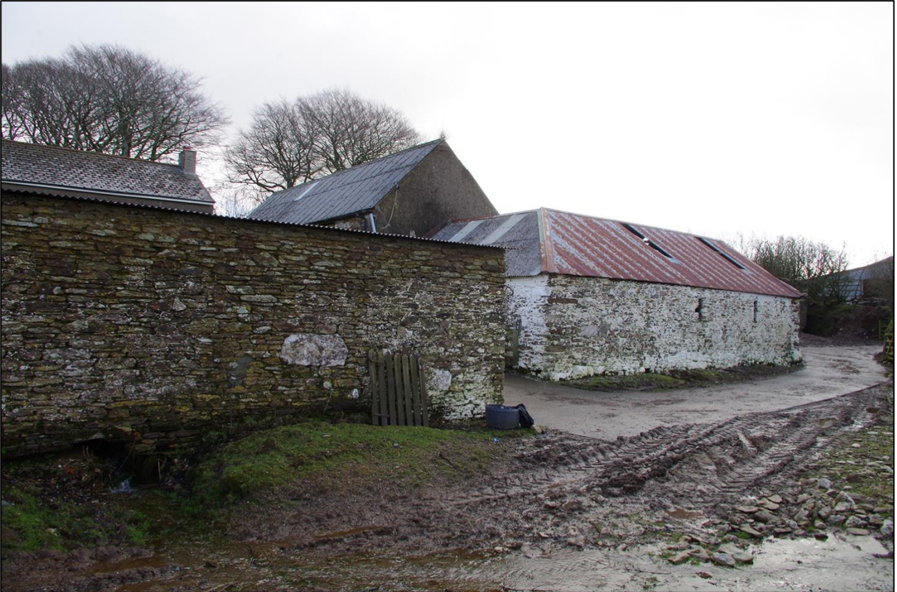
51. THE SOUTH ELEVATIONS OF THE CARTSHED AND SHIPPON; VIEWED FROM THE NORTH-WEST.
