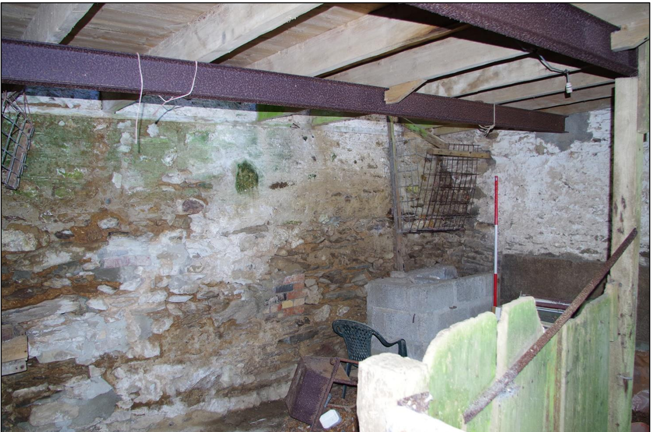
80. THE INTERIOR OF THE STABLES (EAST ROOM); VIEWED FROM THE NORTH-EAST (SCALE 2M).
