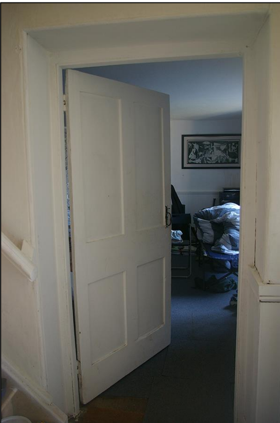
11. R2, DETAIL OF THE DOORWAY LEADING INTO R3; VIEWED FROM THE NORTH.
