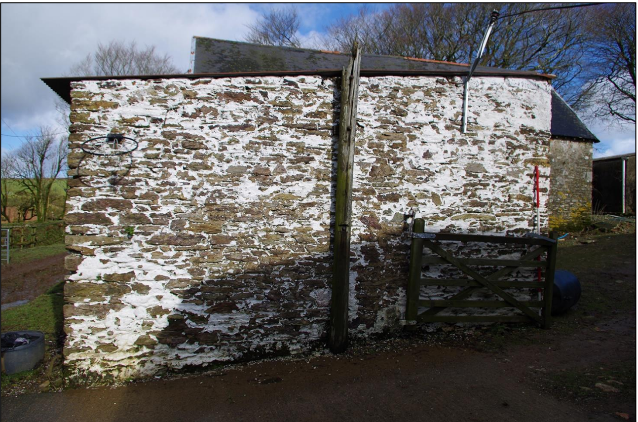
52. THE SOUTH ELEVATION OF THE CARTSHED; VIEWED FROM THE SOUTH (SCALE 2M).
