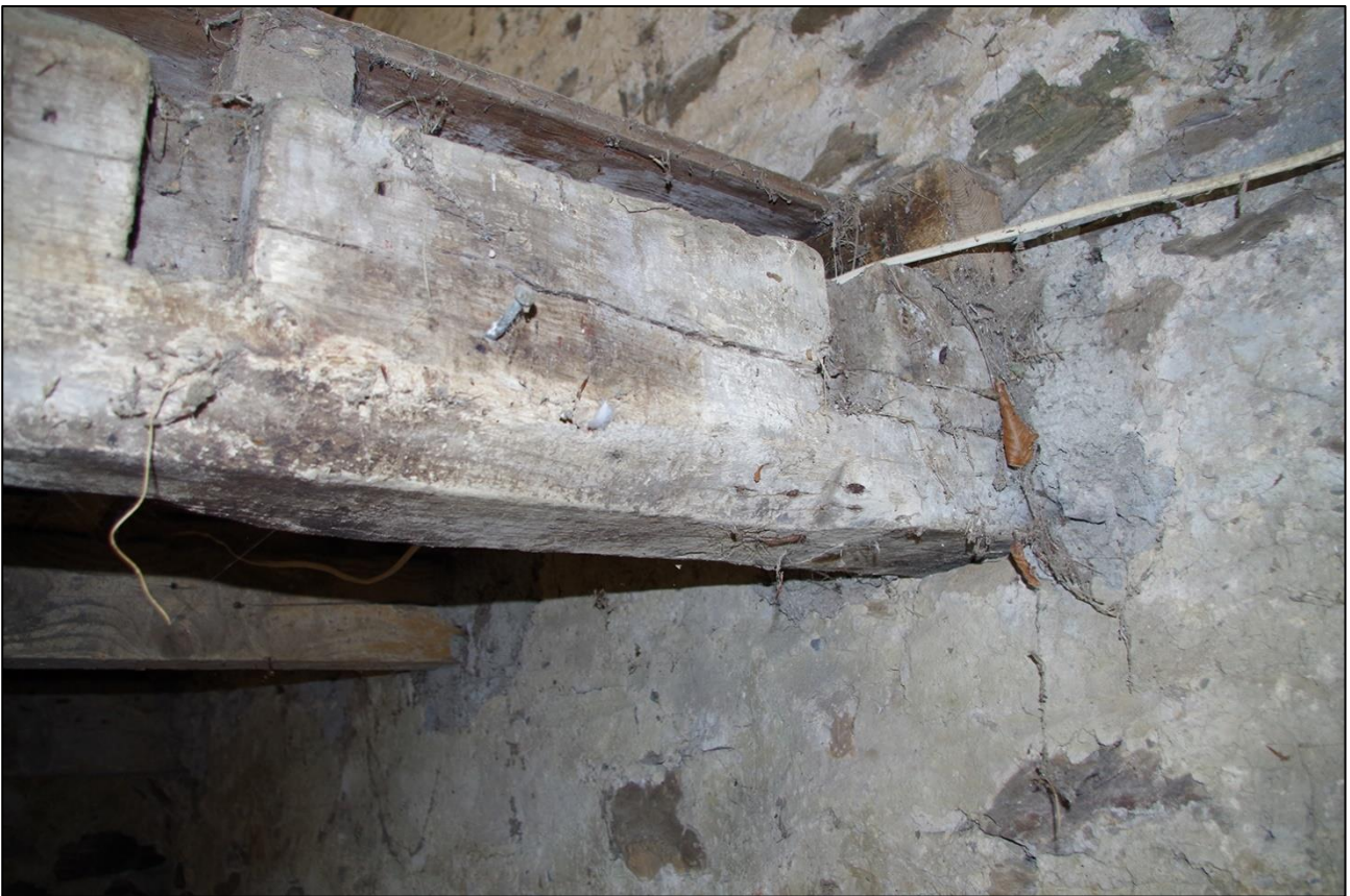
59. DETAIL OF THE RUN-OUT STOP AND DEEP JOIST SOCKETS ON THE RE-USED 17 TH CENTURY BEAM; VIEWED FROM THE NORTH-WEST.
