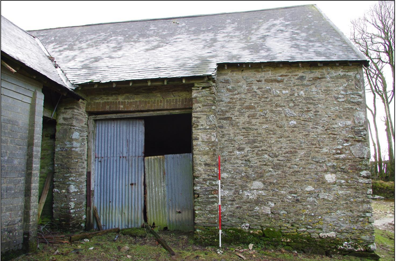
49. THE NORTH ELEVATION AND THRESHING DOORS IN THE THRESHING BARN; VIEWED FROM THE NORTH (SCALE 2M).
