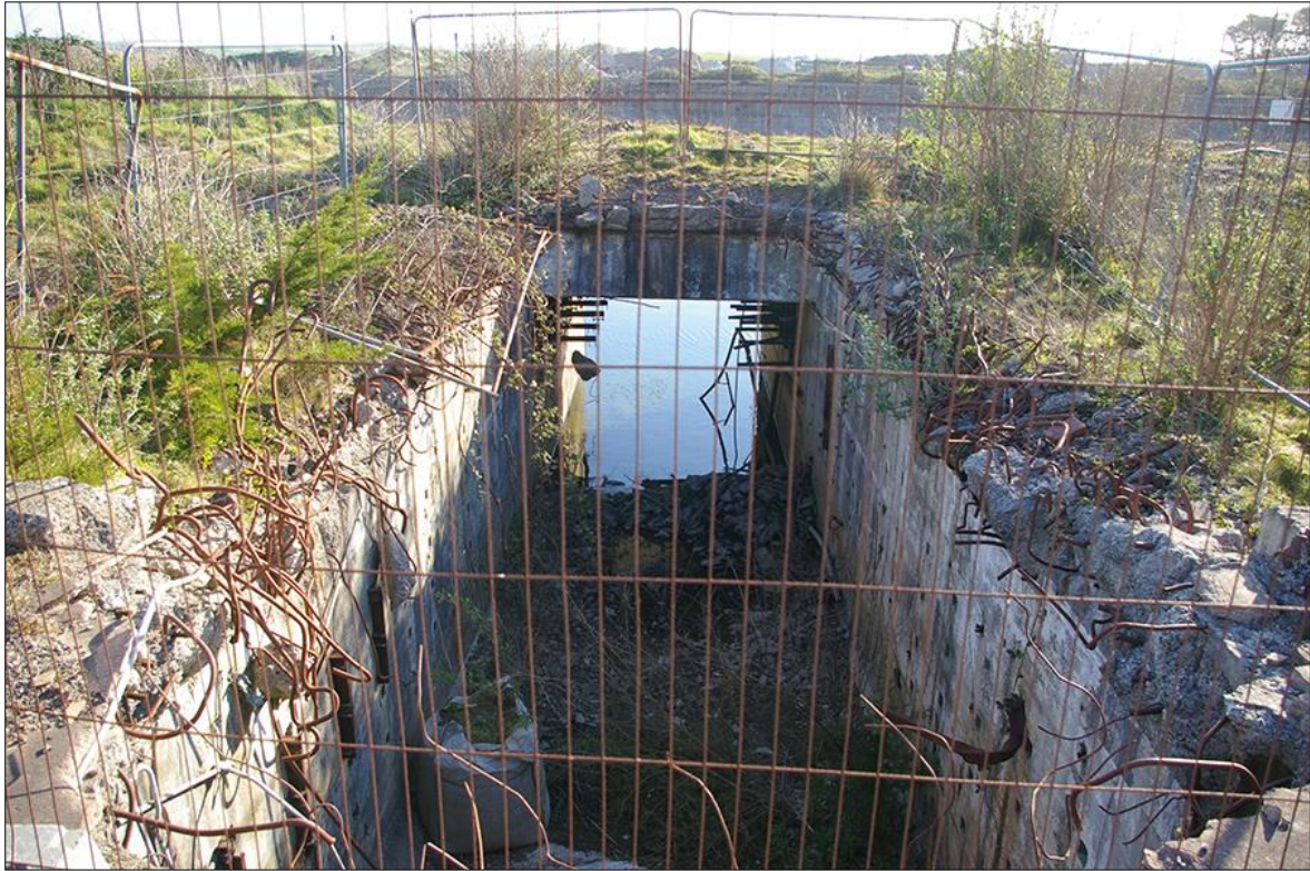
17. DETAIL OF THE ACCESS TUNNEL BETWEEN THE CONTROL ROOM AND OFFICE BLOCK TO THE BOILER- AND TURBINE-HOUSE; VIEWED FROM THE WEST (NO SCALE).
