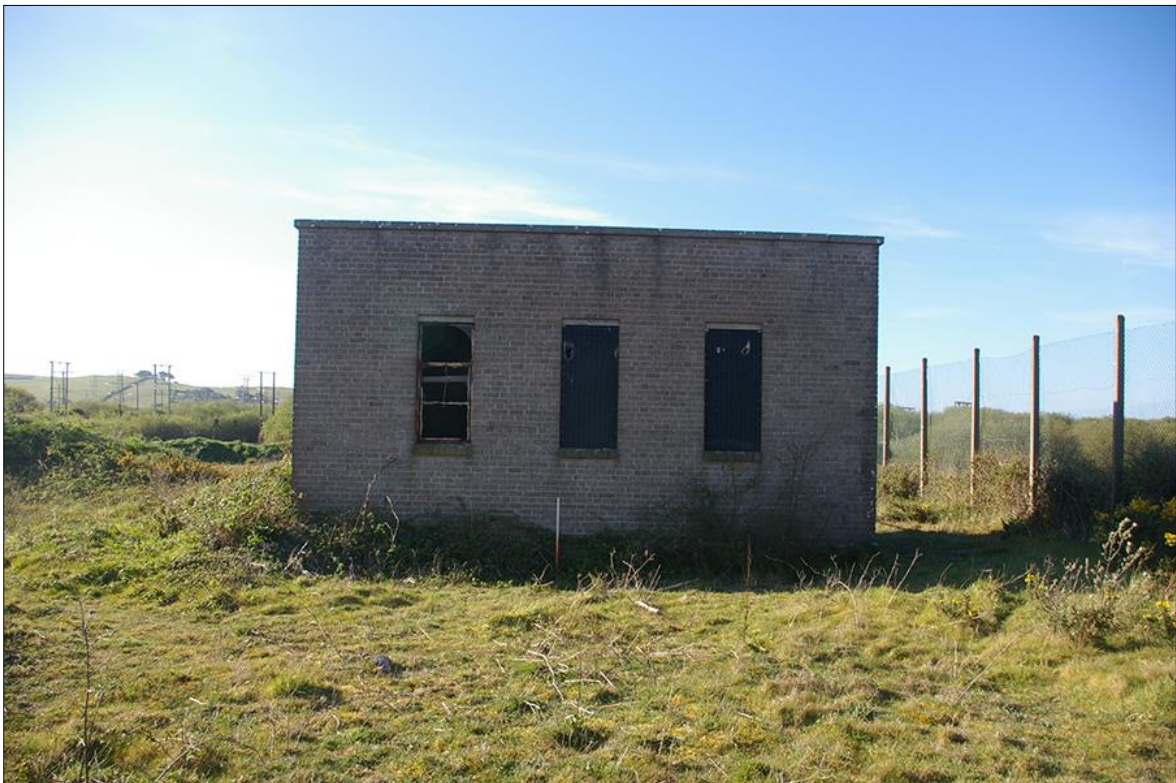
22. NORTH EXTERNAL ELEVATION OF THE PUMP-HOUSE; VIEWED FROM THE NORTH (1M SCALE).
