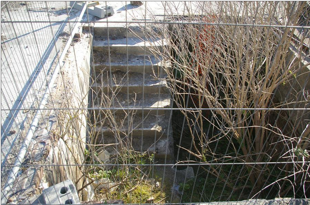
16. DETAIL OF THE SURVIVING STAIRS LEADING TO THE BASEMENT LEVEL OF THE CONTROL ROOM AND OFFICE BLOCK; VIEWED FROM THE WEST (NO SCALE).
