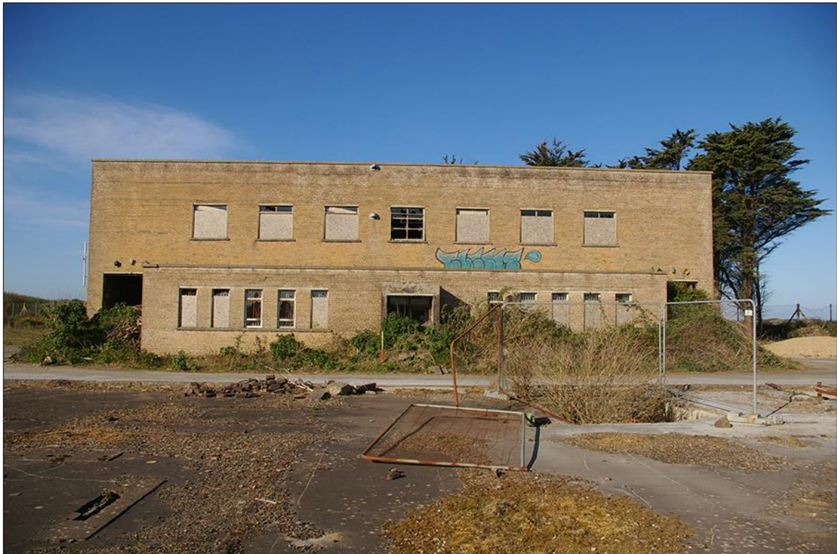
18. EAST EXTERNAL ELEVATION OF THE SWITCH-HOUSE; VIEWED FROM THE EAST (1M SCALE).
