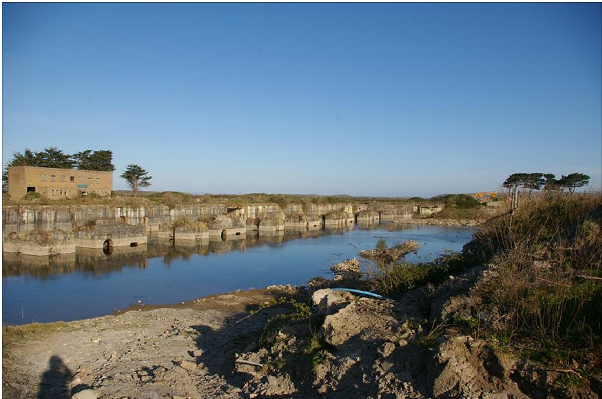
6. VIEW ACROSS THE FLOODED BOILER- AND TURBINE-HOUSE BASEMENT LEVELS; VIEWED FROM THE SOUTH-EAST (NO SCALE).
