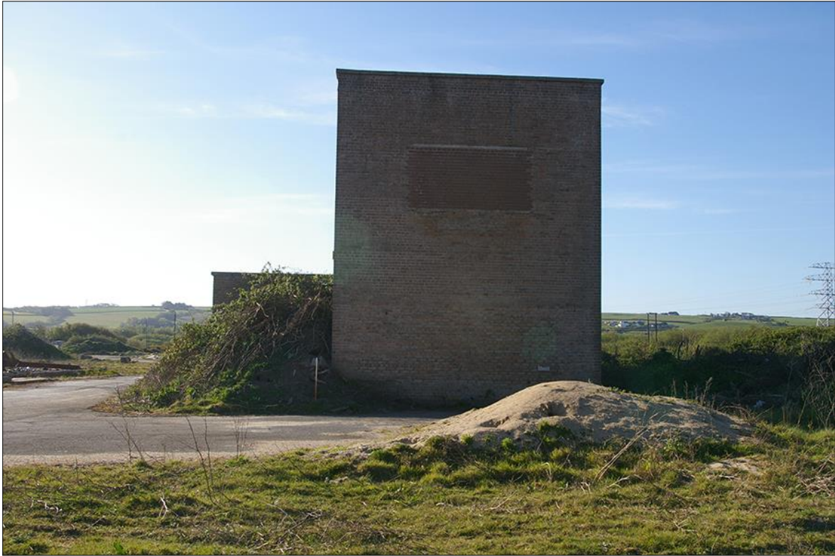
19. NORTH EXTERNAL ELEVATION OF THE SWITCH-HOUSE; VIEWED FROM THE NORTH (1M SCALE).
