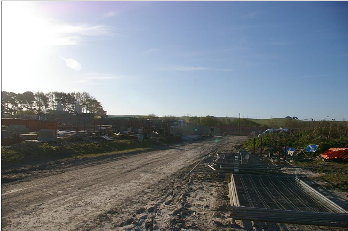
1. VIEW ALONG THE CENTRAL ACCESS ROAD, SHOWING THE CURRENT USE OF THE SITE AS A STORAGE YARD; VIEWED FROM THE NORTH-WEST (NO SCALE).
