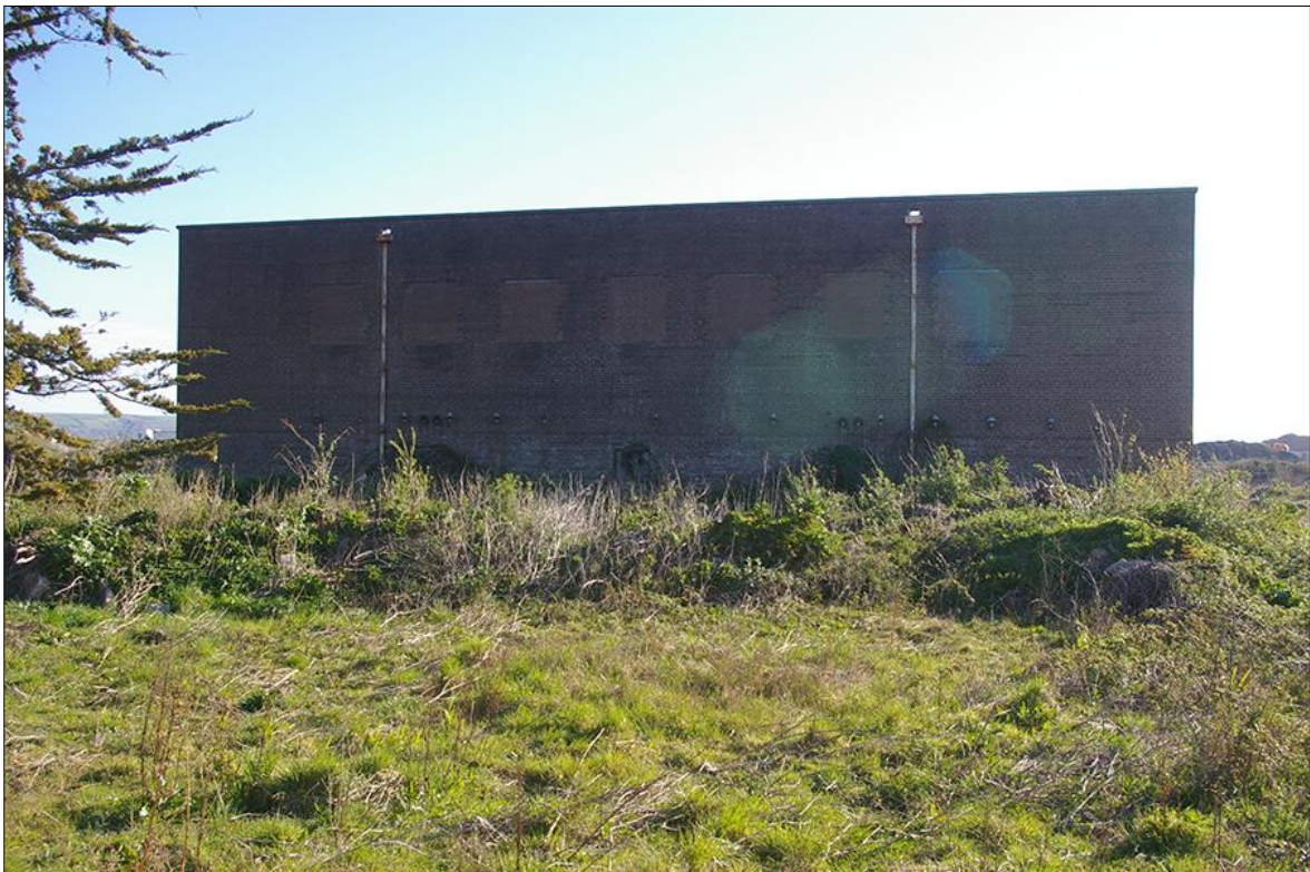
20. WEST EXTERNAL ELEVATION OF THE SWITCH-HOUSE; VIEWED FROM THE WEST (NO SCALE).
