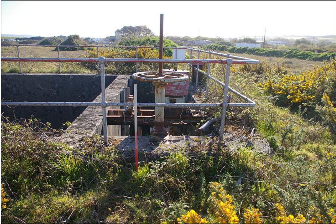
25. DETAIL OF THE SLUICE AT THE SOUTHERN END OF THE PUMP-HOUSE SETTLING TANK; VIEWED FROM THE WEST (1M SCALE).
