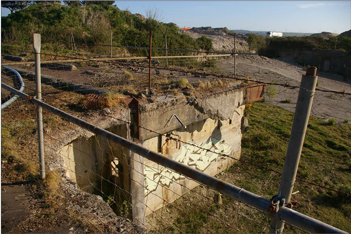
9. DETAIL OF THE FLOODED BOILER- AND TURBINE-HOUSE, DEMONSTRATING THE STEEL FRAME AND CONCRETE CONSTRUCTION; VIEWED FROM THE SOUTH-WEST (NO SCALE).
