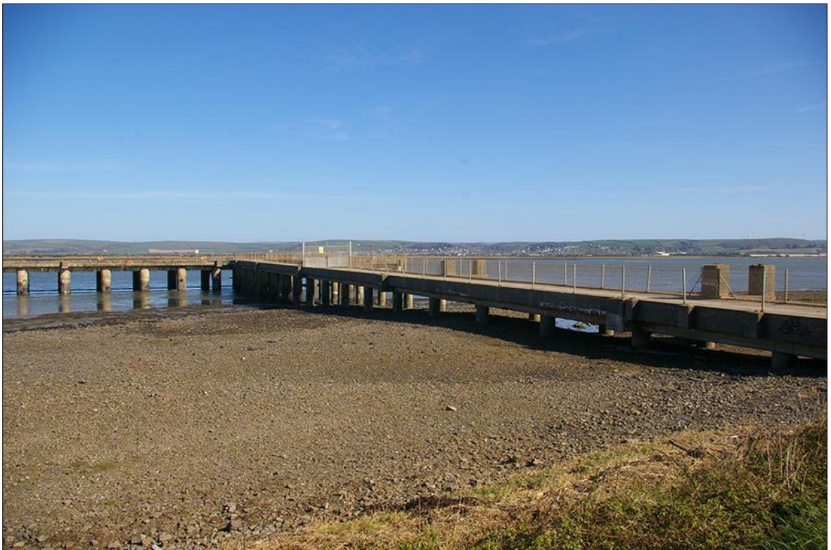
28. DETAIL OF THE SURVIVING JETTY STRUCTURE; VIEWED FROM THE SOUTH-WEST (NO SCALE).
