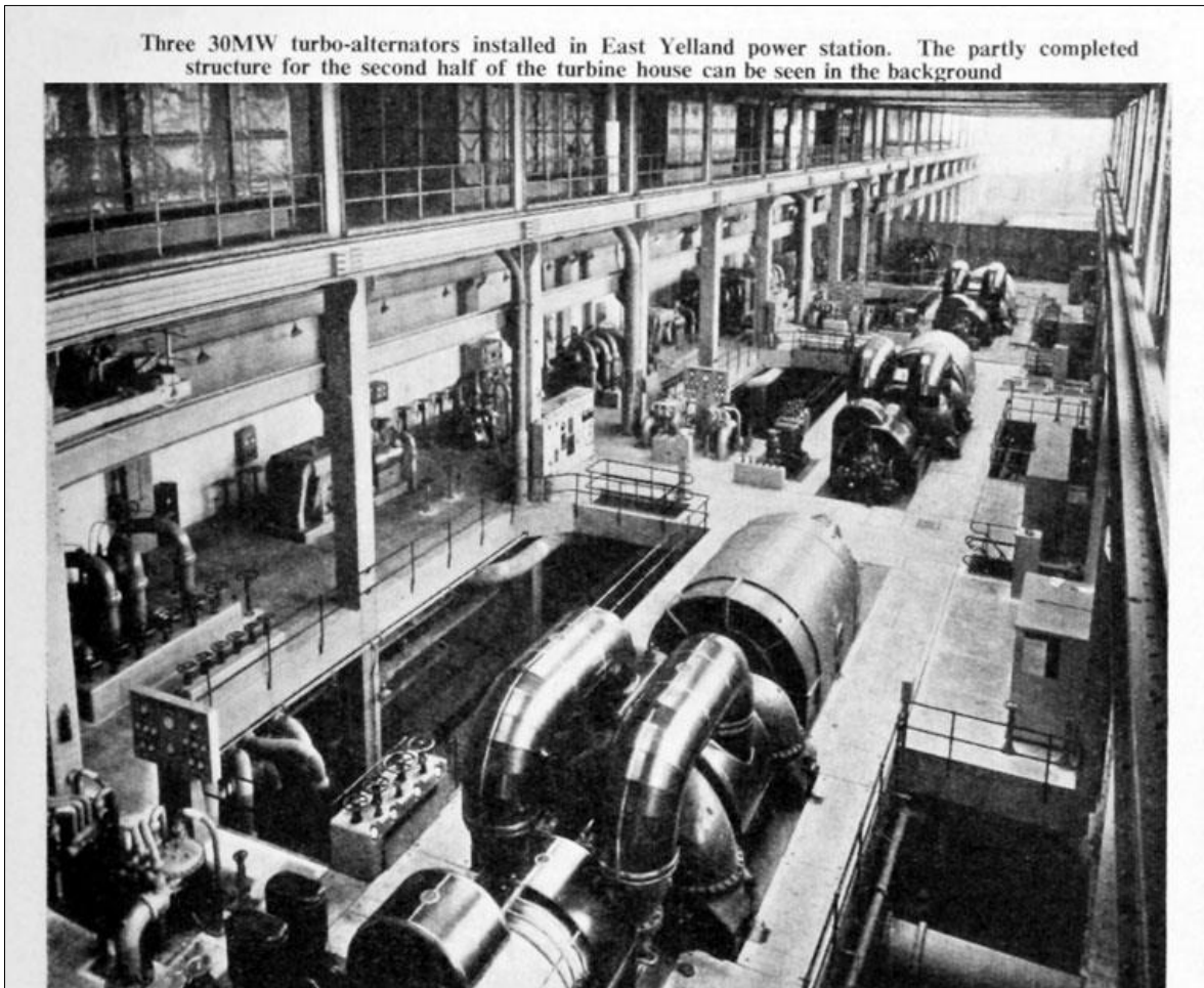
FIGURE 7: DETAIL OF TURBO-ALTERNATORS AT EAST YELLAND POWER STATION (THE ENGINEER 1955).
