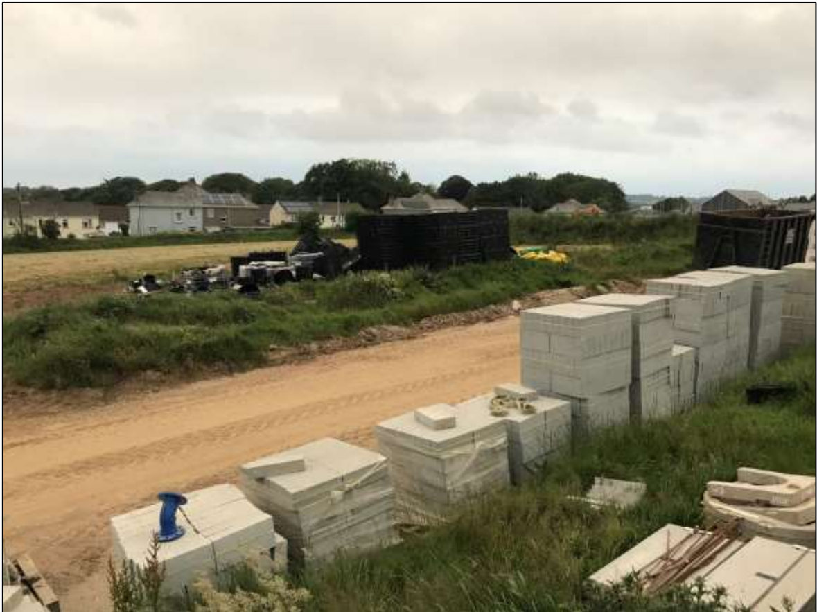
FIGURE 3: VIEW ACROSS THE NORTHERN PART OF THE PHASE 2 SITE; VIEWED FROM THE SOUTH-EAST.
