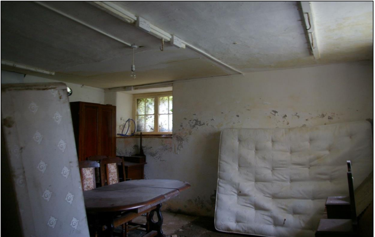
36. R6, WITH WINDOW TO WEST WALL, GOOD FLOOR AND BEAMS AND HOOKS TO CEILING; FROM THE NORTH-EAST.
