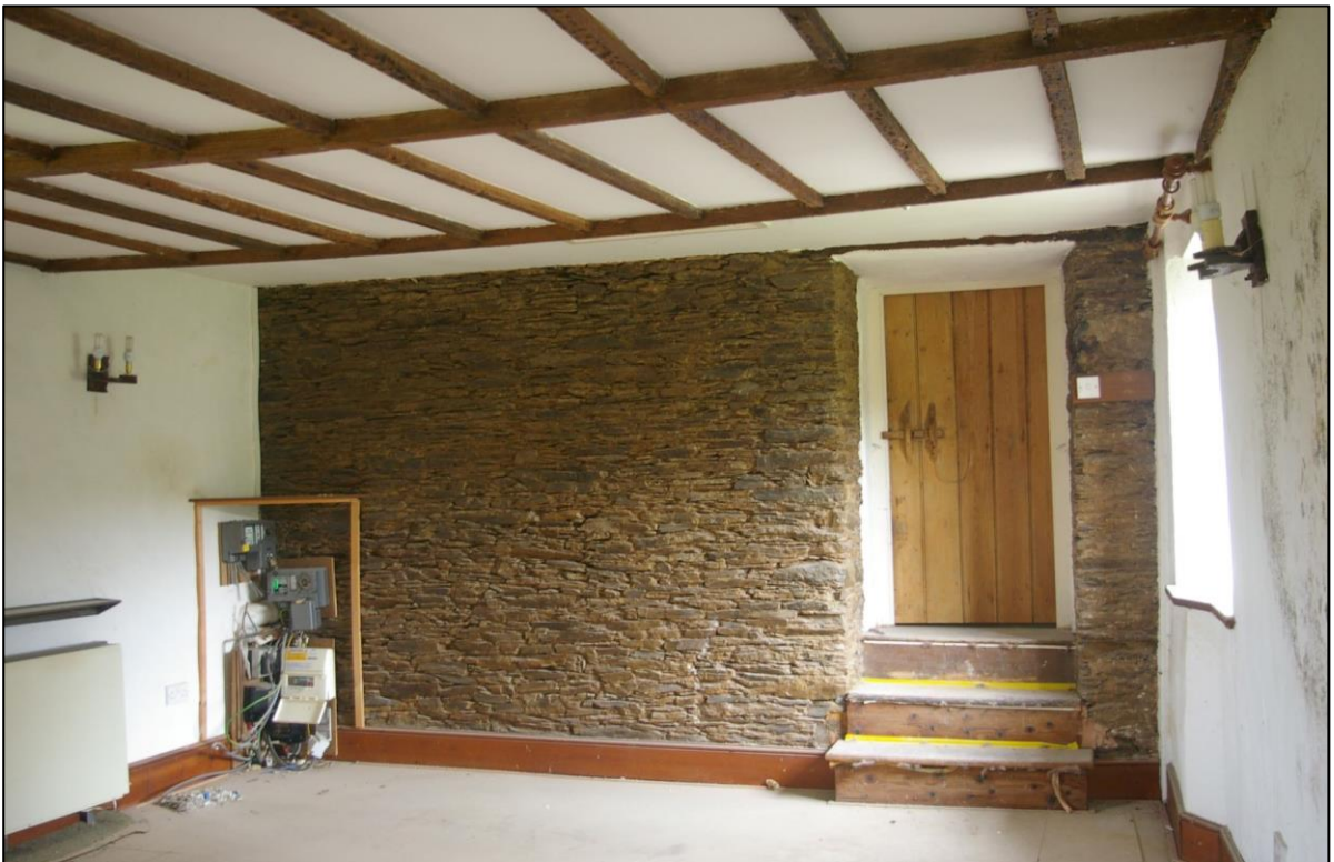
63. ROOM 20, VIEW BACK TO THE REAR WALL OF THE FORMER HALL; FROM THE NORTH-WEST CORNER.
