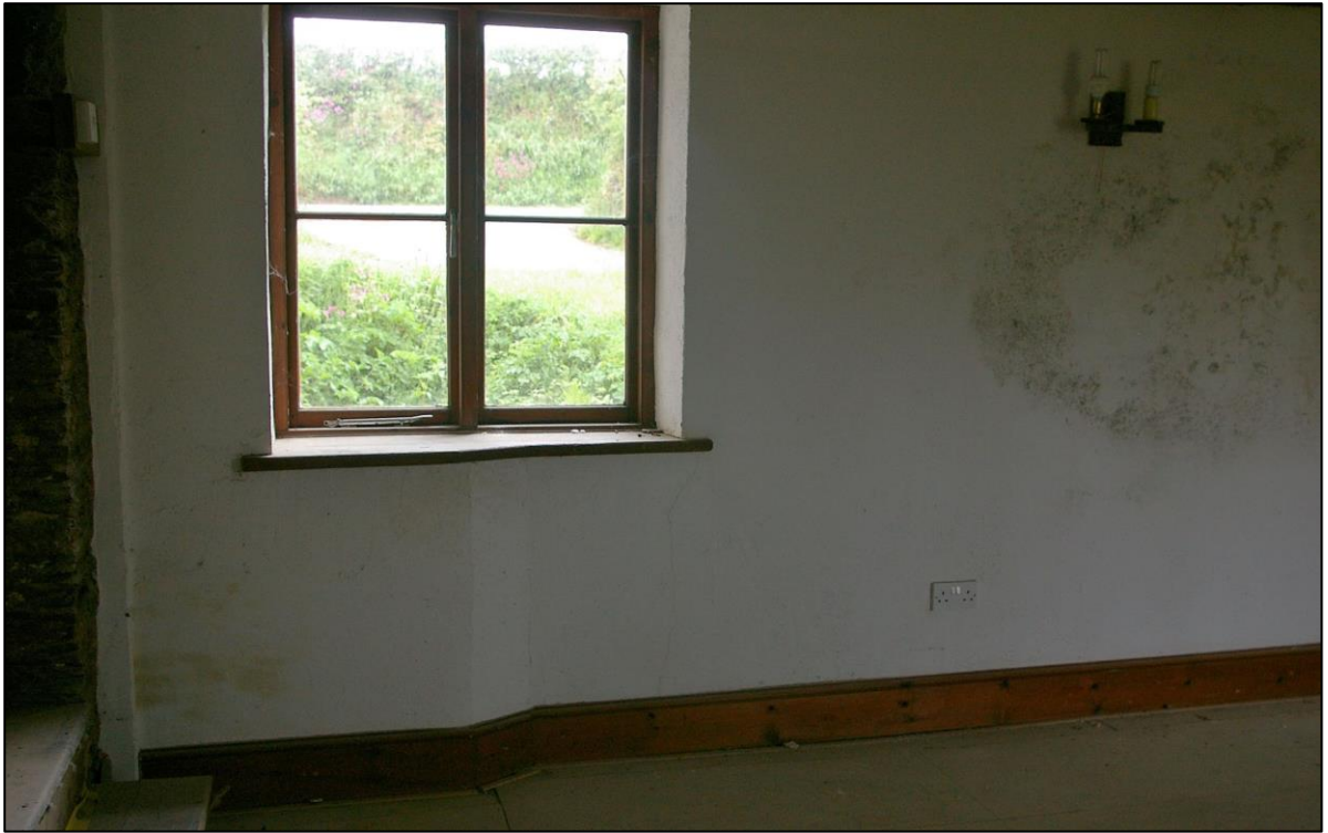
62. ROOM 20, THE WEST WALL WITH THICK SHORT SECTION, FORMERLY OF THE STAIR TURRET; FROM THE SOUTH-EAST.
