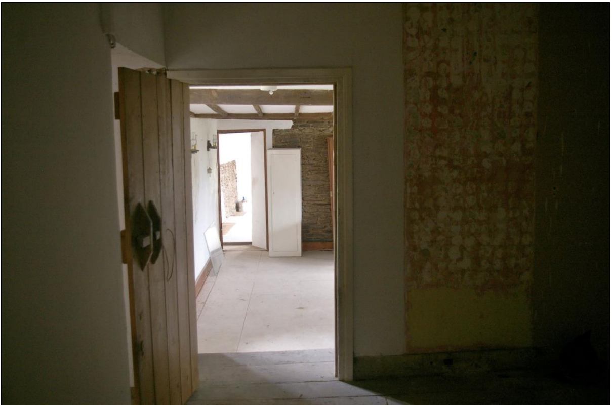
56. ROOM 18, NOW A WINDOWLESS LOBBY LINKING THE RANGES WITH TWO GOOD DOORS; FROM THE SOUTH.
