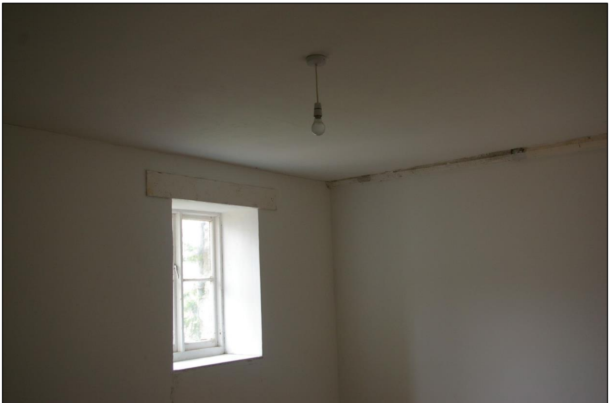
54. ROOM 17, WITH THE MORE RECENT WINDOW AND MOULDED BRACING BEAM; FROM THE SOUTH-WEST.
