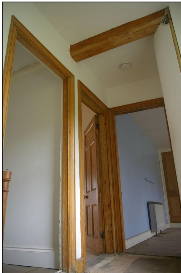
50. VIEW TO THE DOORS AND BEAM BRACING WHERE THE VARIOUS BLOCKS ADJOIN IN R14; FROM THE WEST.
