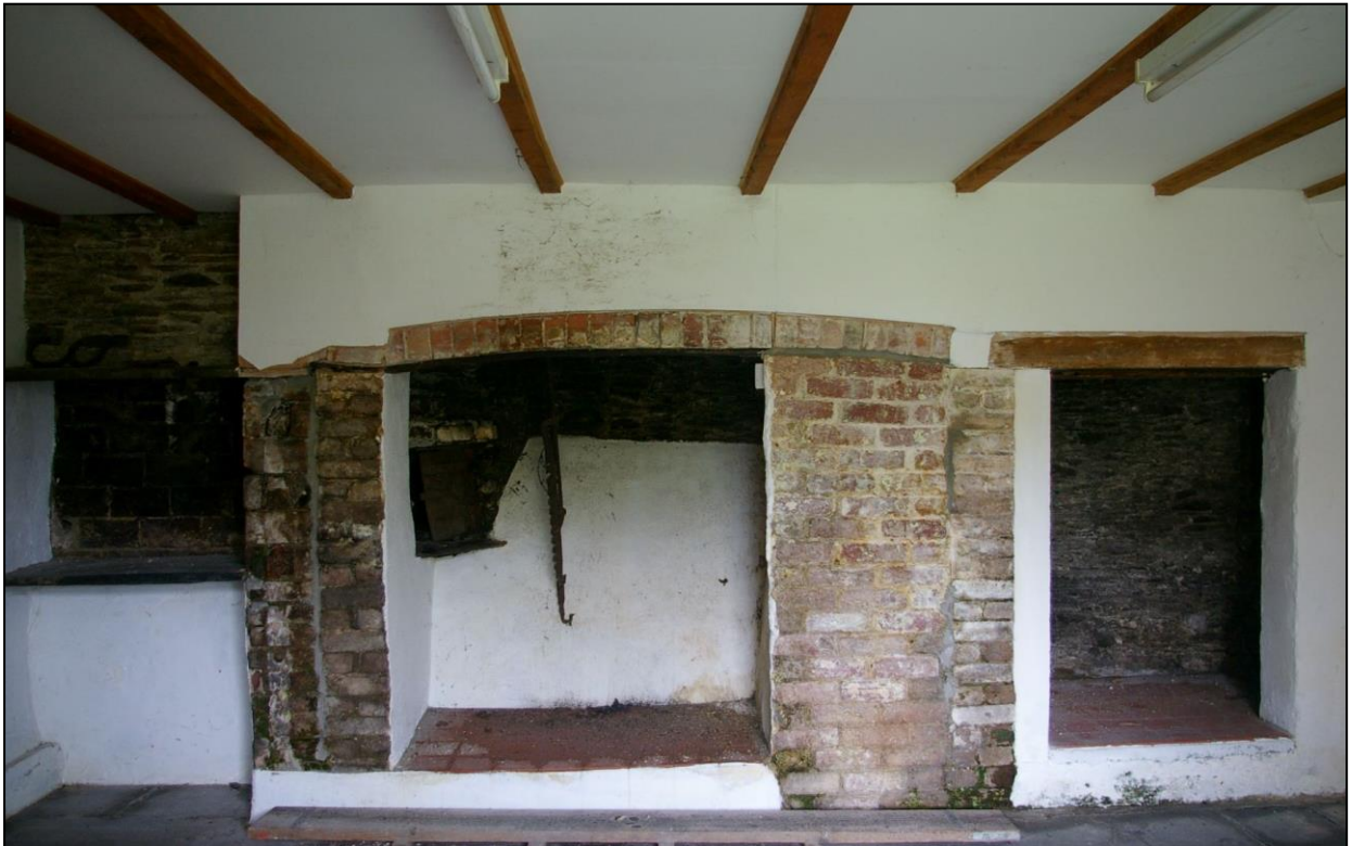
FIGURE 9: THE MUCH-ALTERED LATERAL STACK IN THE REAR WING, ROOM 7; FROM THE EAST.
