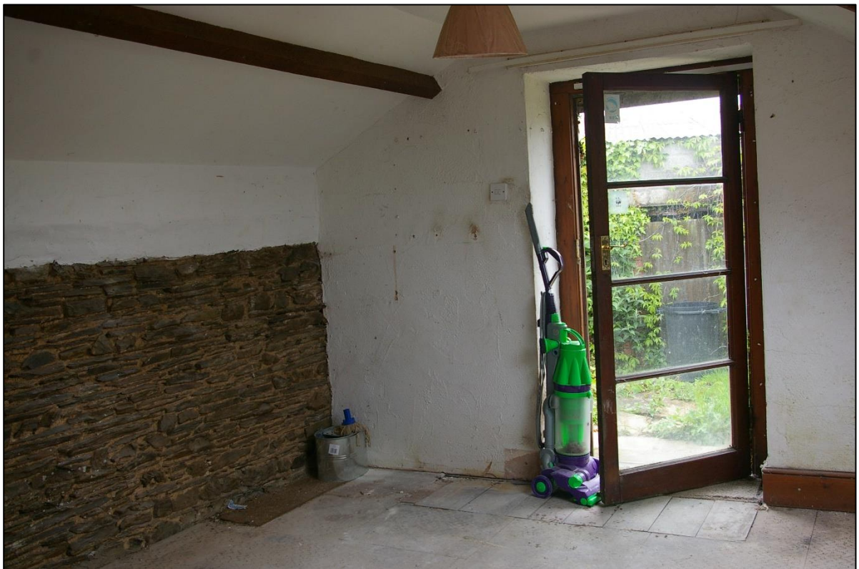
65. ROOM 21, A LOFT OVER AN AGRICULTURAL EXTENSION, NOW A STUDIO/ANNEXE WITH EXTERIOR DOOR, AS TERRACED DEEPLY INTO THE BANK; FORM THE SOUTH-EAST.
