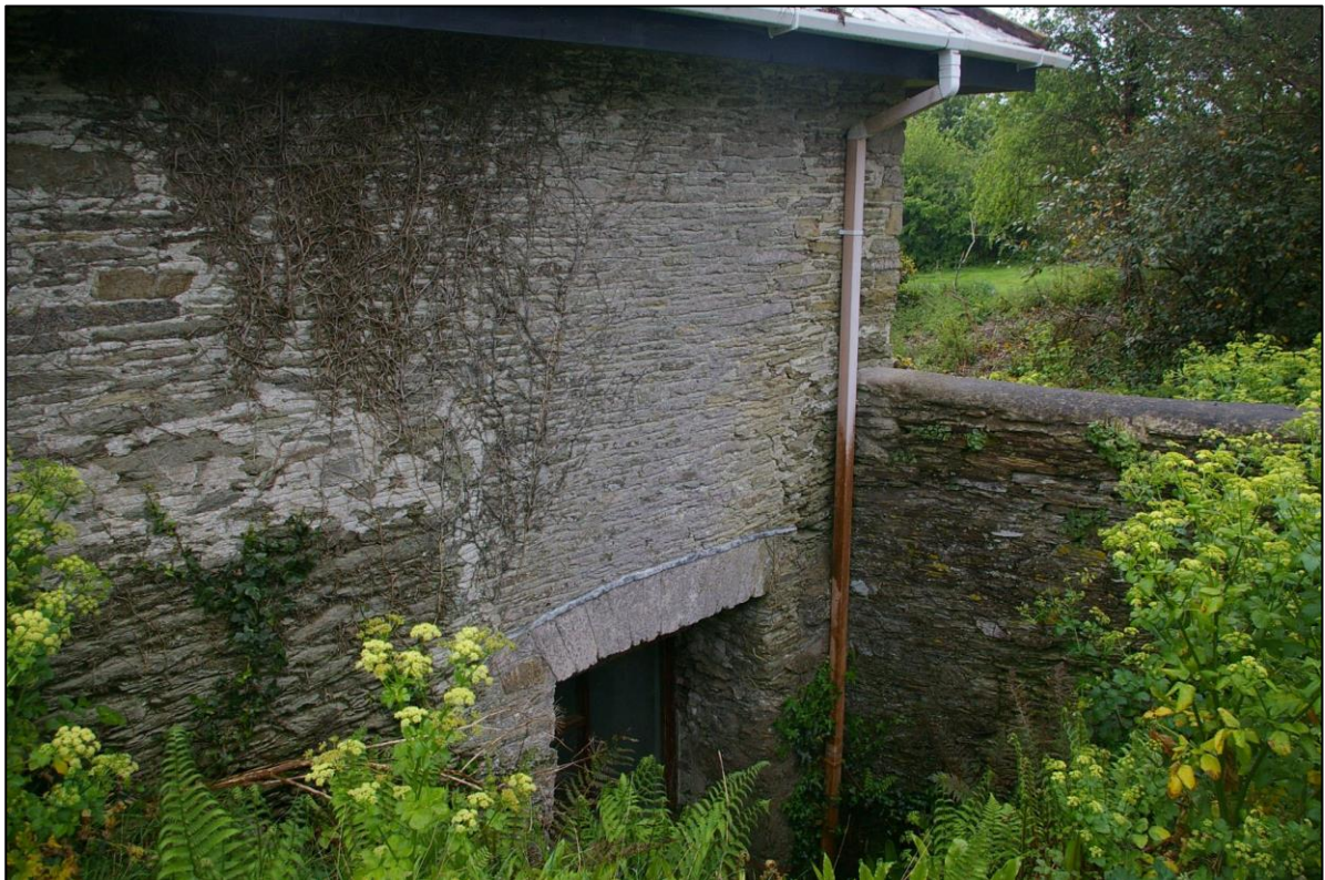
14. THE SOUTH END OF THE WEST WALL OF THE WEST CROSS-WING; FROM THE NORTH-WEST.
