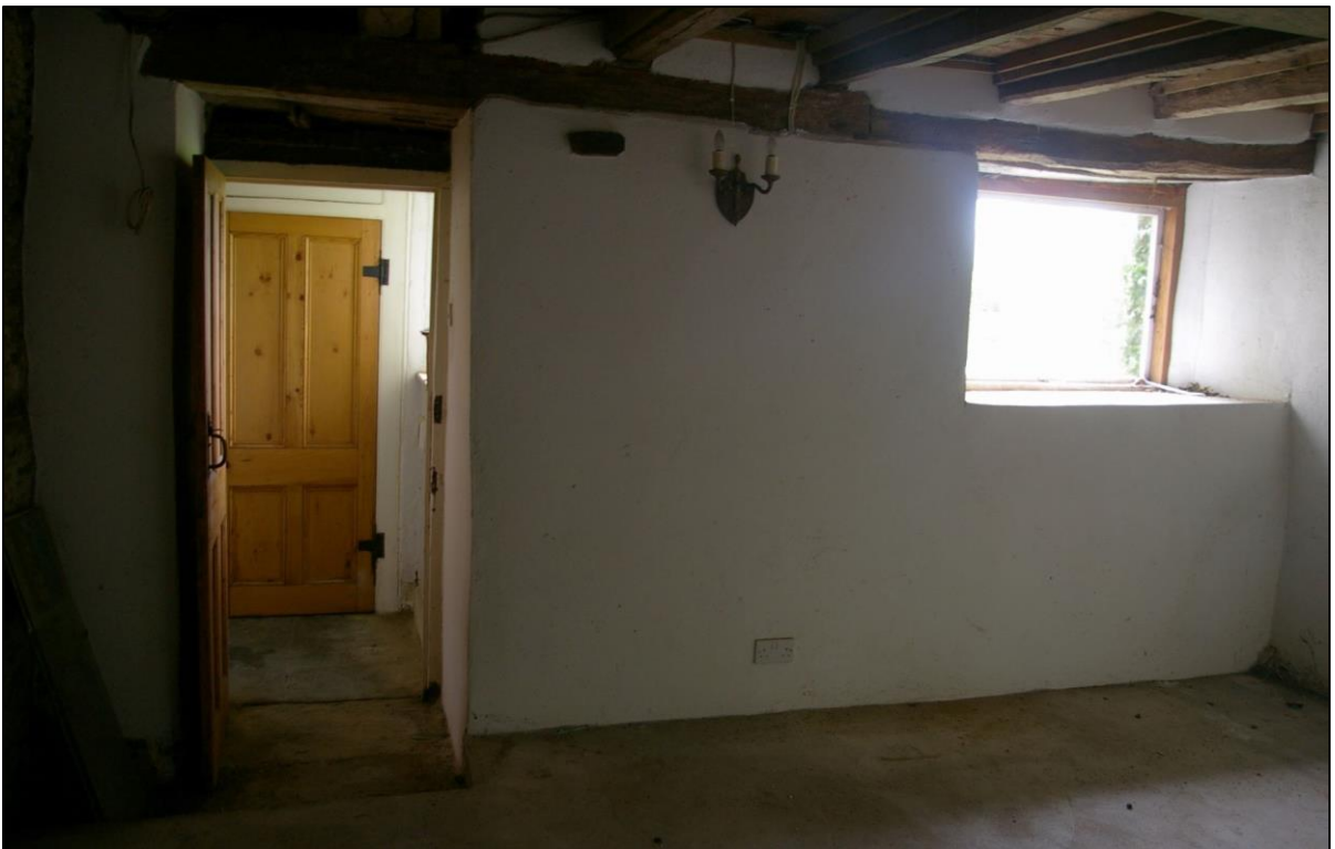
31. R5, THE EAST WALL, WITH BLOCKED OPENINGS AND MODERN WINDOW UNDER THE THICK CHAMFERED BEAM; FORM THE NORTH-WEST.
