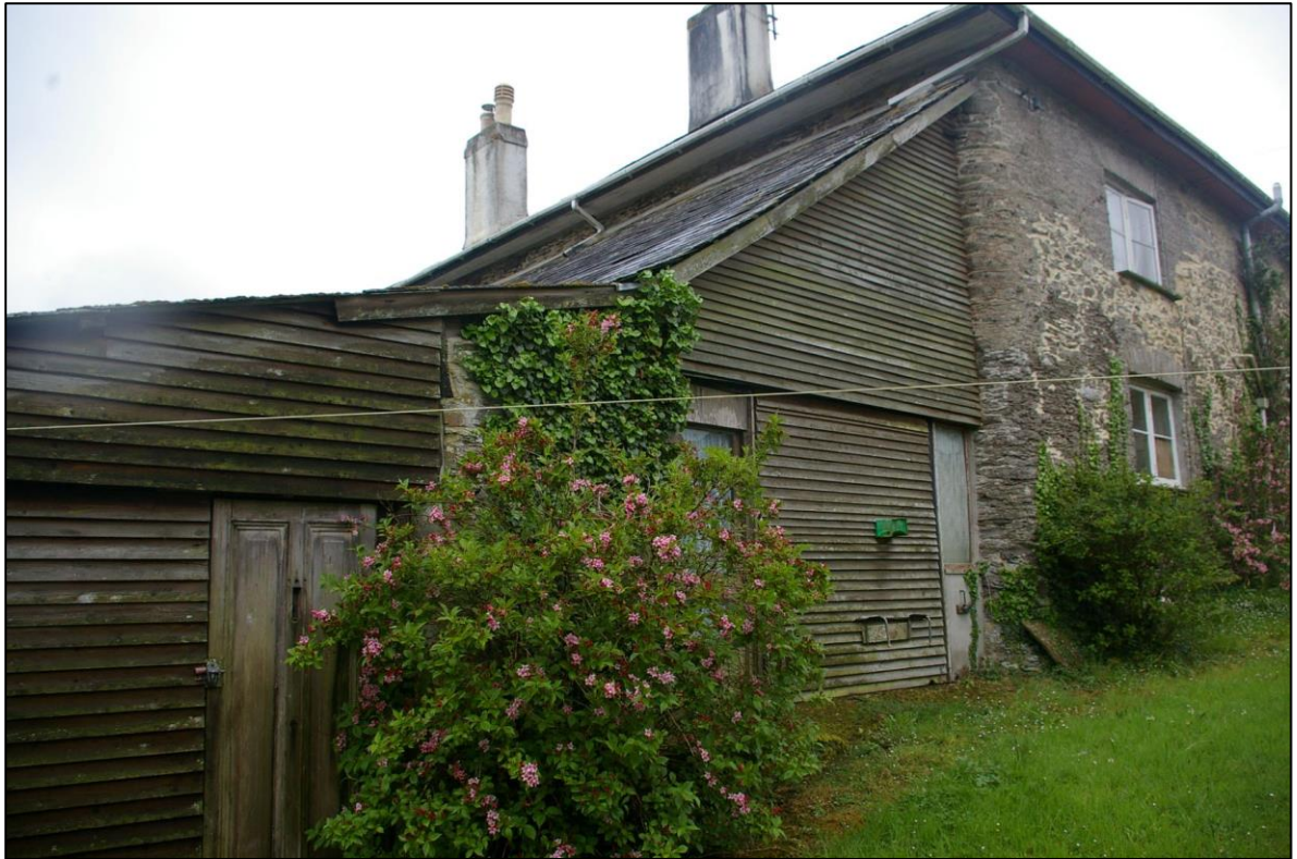
7. OB1, ATTACHED TO THE EAST WALL OF THE HOUSE; FROM THE EAST-NORTH-EAST.
