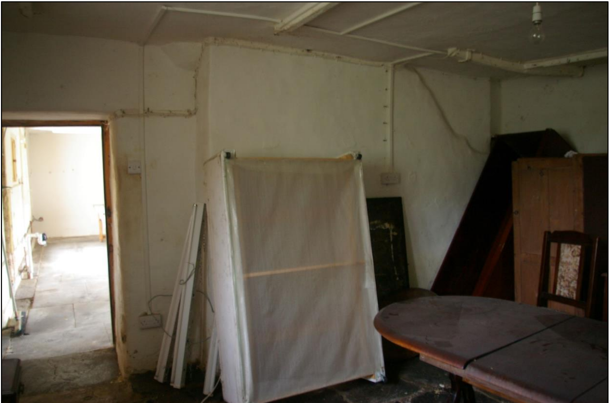
35. R6, THE EAST WALL WITH MASSIVE STACK AND BLOCKED FIREPLACE AND HOOKS TO CEILING; FROM THE NORTH-WEST.
