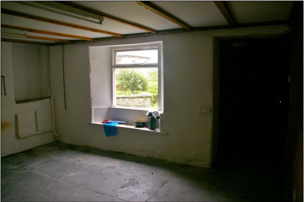
40. R7, THE EAST WALL WITH GOOD WINDOW SEAT AND EXTANT DOOR; FROM THE SOUTH-WEST.
