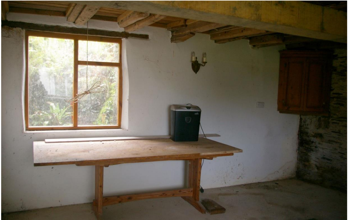
32. THE WEST WALL OF R5, WITH WINDOW IN THE BLOCKED DOORWAY; FROM THE SOUTH-EAST.
