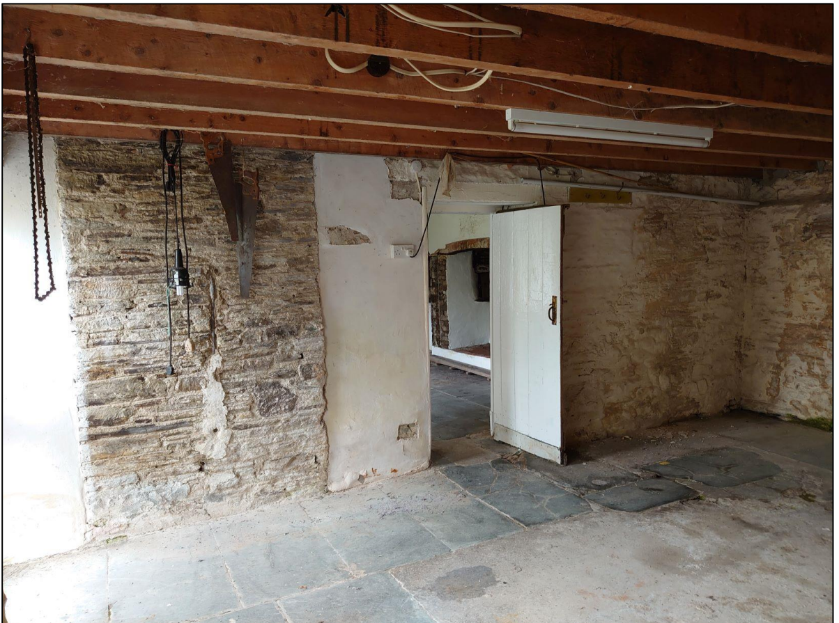
41. R8, THE SOUTH WALL, WITH DOOR LEADING BACK TO R7; FROM THE NORTH-EAST.
