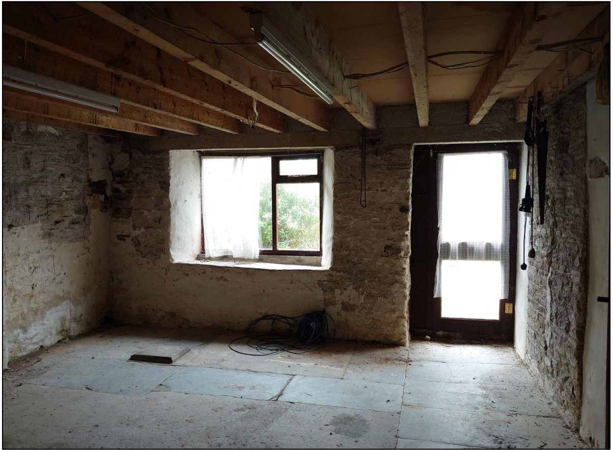
42. R8, WITH PARTS OF A GOOD FLAGSTONE FLOOR AND MODERN DOOR AND WINDOW TO THE EAST WALL; FROM THE SOUTH-WEST.
