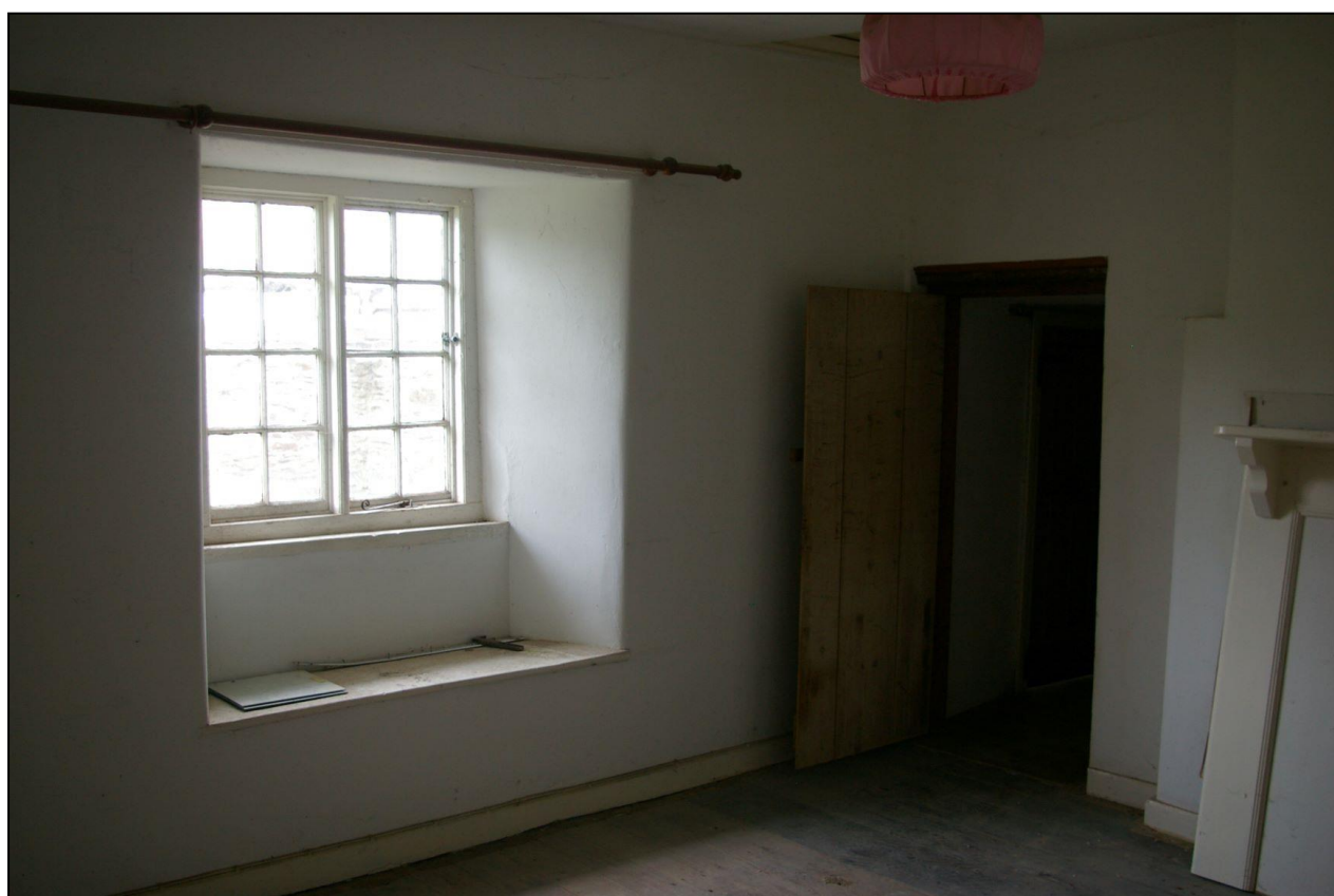
FIGURE 12: ROOM 19, WITH GOOD DOOR AND WINDOW, WITH WINDOW SEAT; FROM THE SOUTH-WEST.
