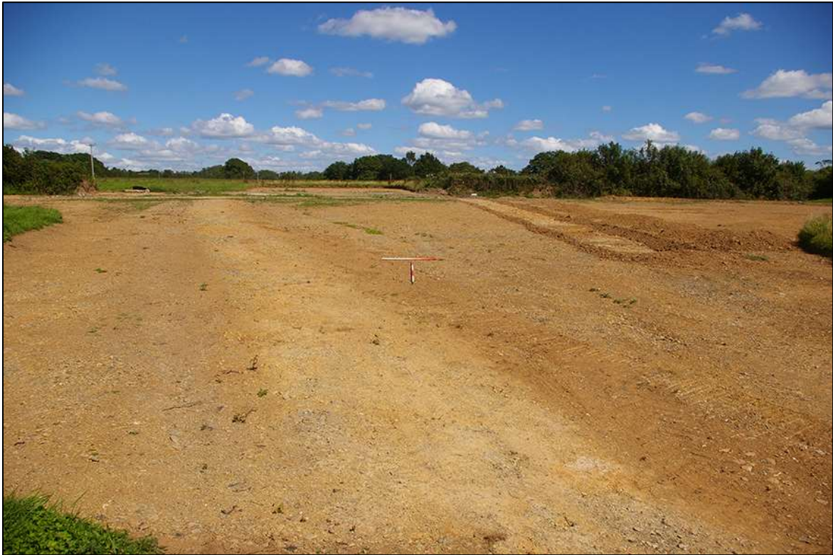
107. VIEW ACROSS THE ALREADY STRIPPED ROAD ACCESS AREA 14; VIEWED FROM THE WEST (1M & 2M SCALES).
