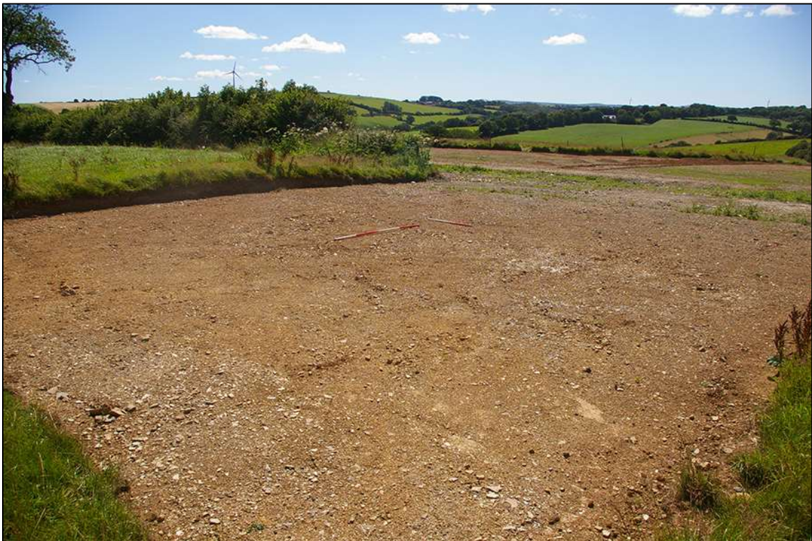
108. VIEW ACROSS THE ALREADY STRIPPED ROAD ACCESS AREA 14; VIEWED FROM THE NORTH-EAST (1M & 2M SCALES).
