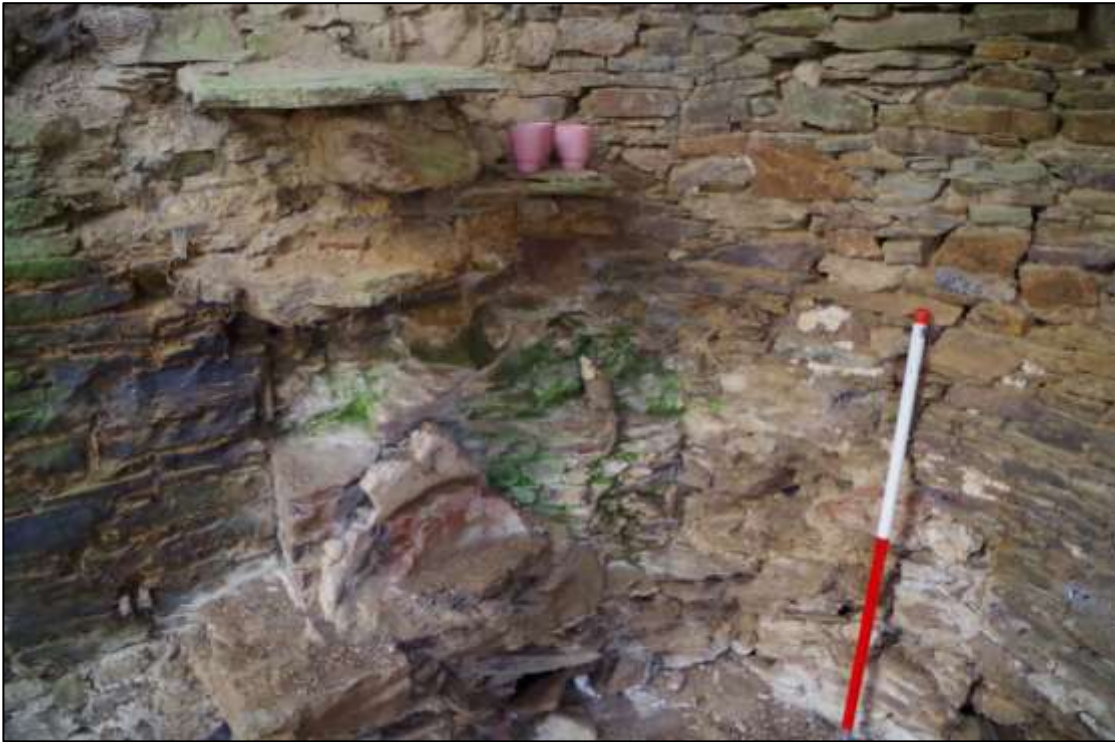
7. DETAIL OF OVEN, WITH SCAR FOR LINTEL FOR FIREPLACE ABOVE, VIEWED FROM THE EAST (1M SCALE).
