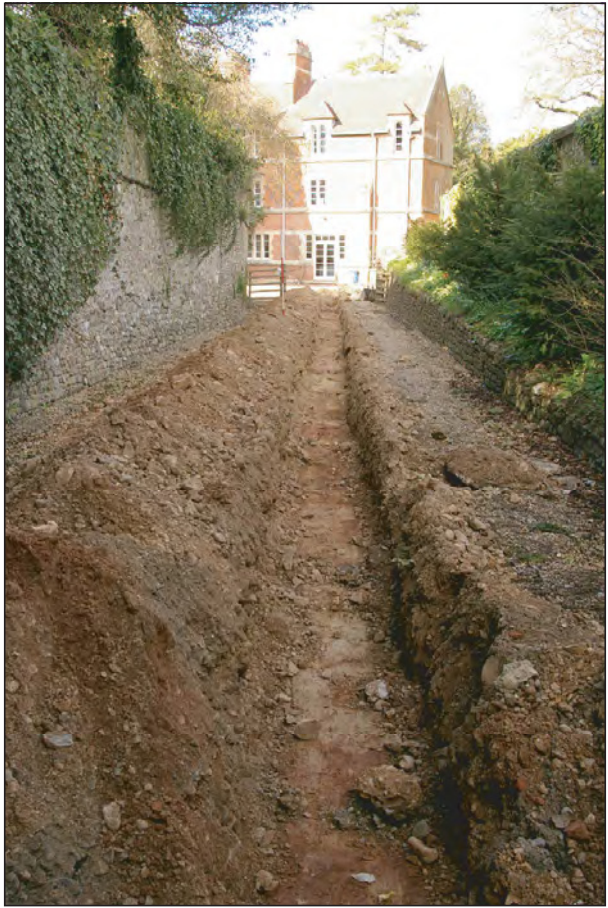
Plate 1: Trench 1, looking north along the drive to the Chanter's House. The wall of St Mary's Churchyard is on the right (2m scale).
