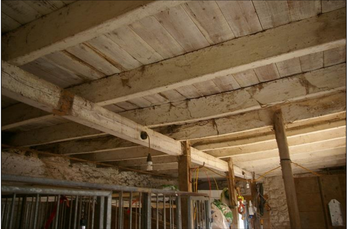
7. THE LOFT FLOOR IN B1A, SHOWING CENTRAL TIMBER BRACING FRAMEWORK FOR RESET STALLS.
