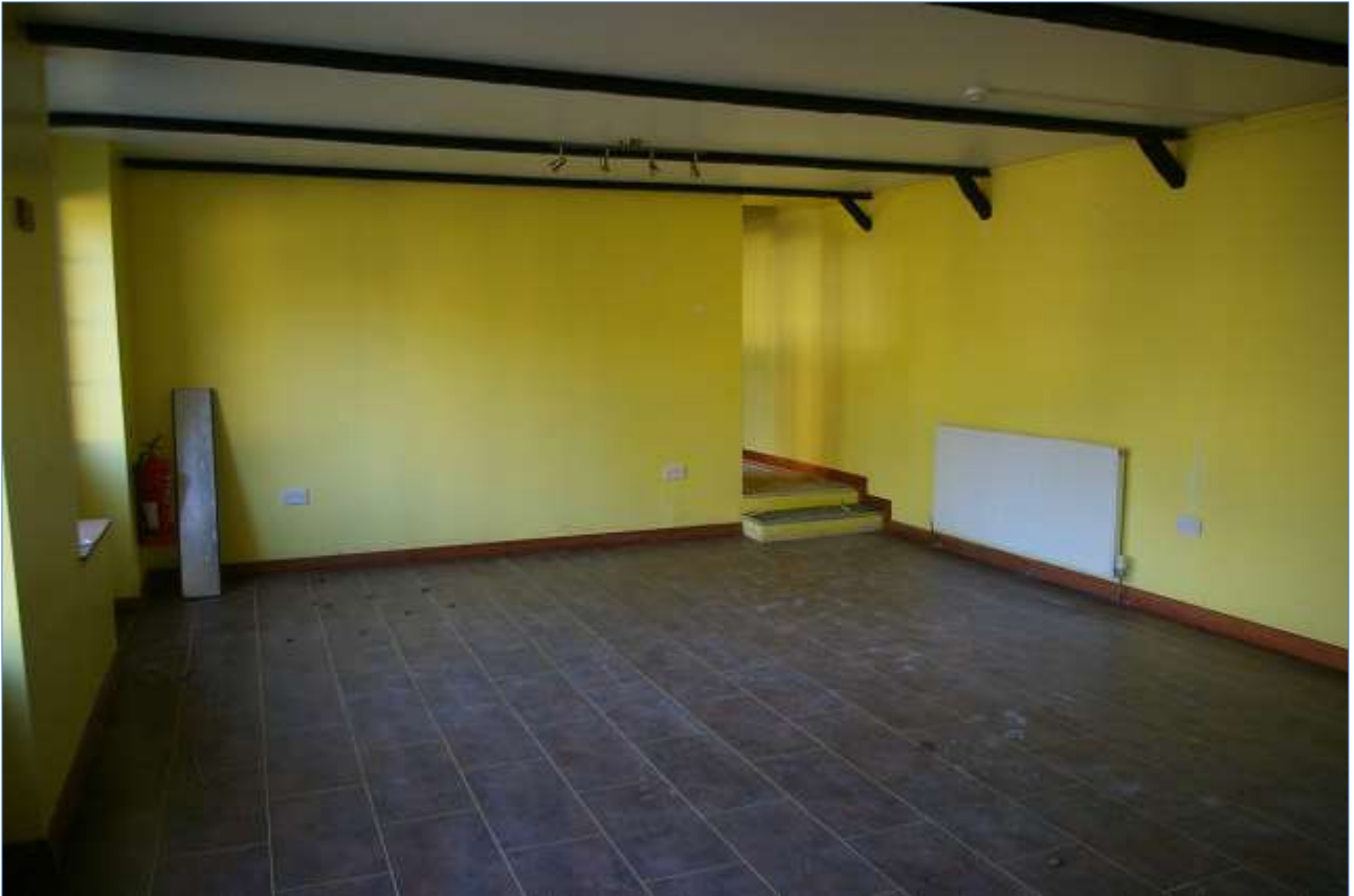
15. THE LARGE LIVING SPACE AT THE SOUTH END OF BLOCK 1, WITHIN 1A, WHERE THERE IS A BLOCKED FIREPLACE IN THE WALL, SHOWING THE MODERNISED CHARACTER; VIEWED FROM THE SOUTH-WEST.
