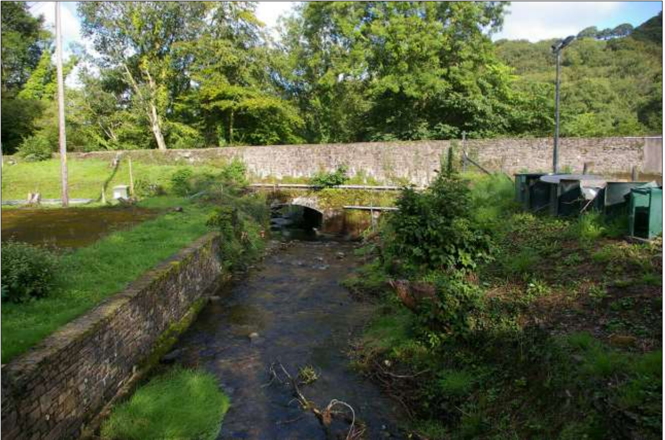
49. THE BRIDGE WHICH CARRIES THE ROAD OVER RIVER, SHOWING HOW THE BANK HAS SLUMPED ON THE NORTH SIDE, BLOCKING THE SECOND ARCH; FROM THE EAST.
