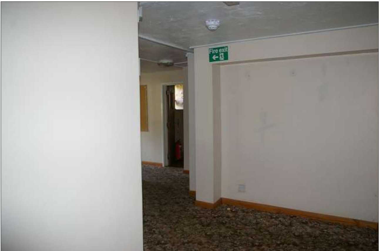
90. THE ODD ANGLES AND LINKING SPACES FORMED BY JOINING THE RANGES TOGETHER; VIEWED FROM THE WSW.
