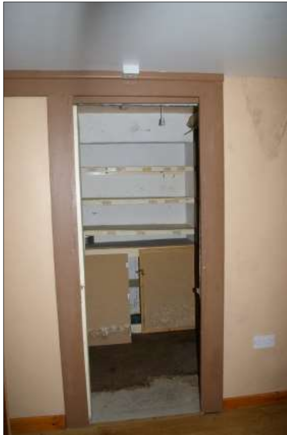
76. THE BLOCKED DOORWAY BETWEEN THE MILL BUILDING AND SERVICE RANGE; VIEWED FROM THE WEST.
