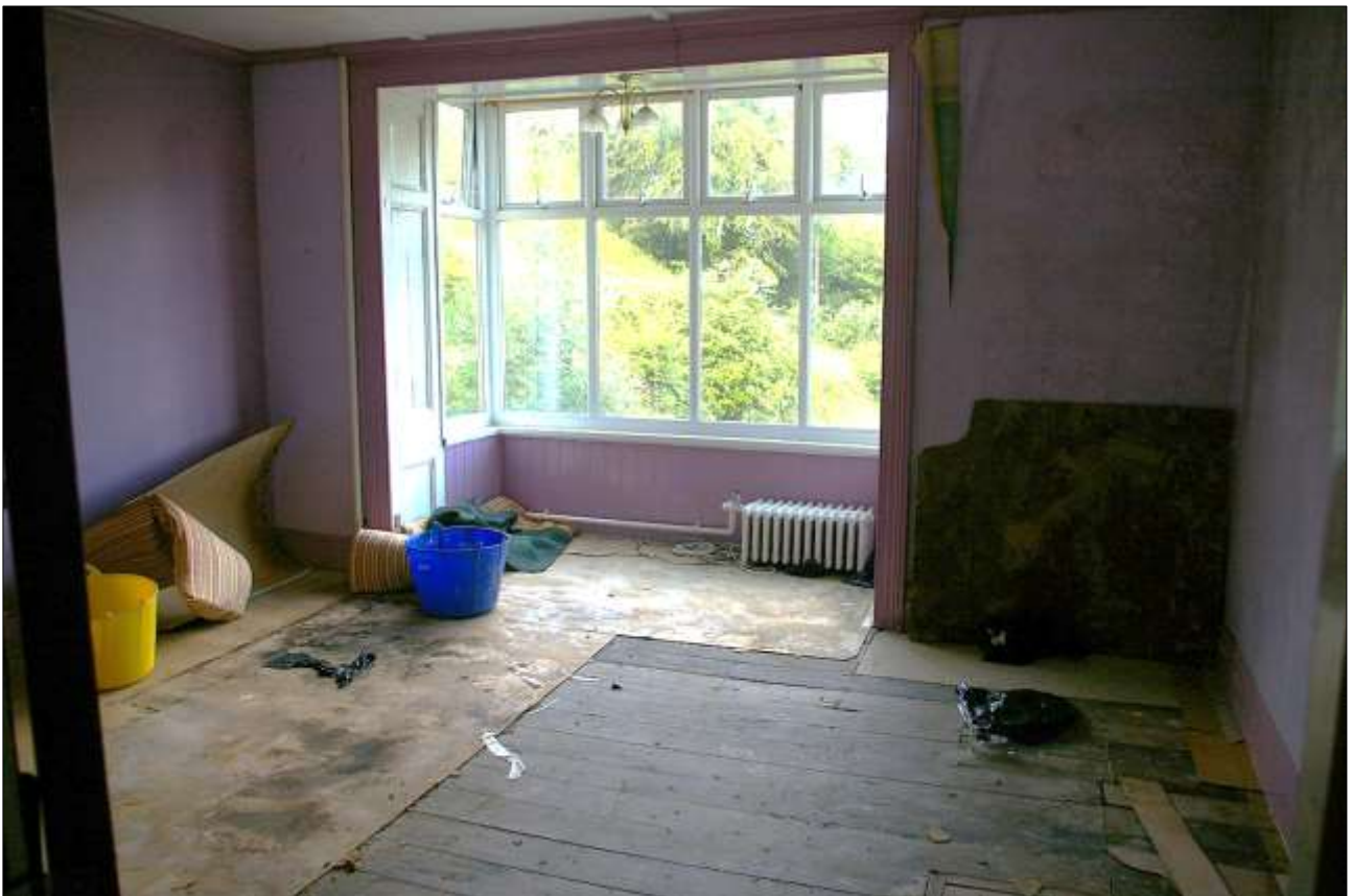
83. ONE OF THE OTHER LARGE FIRST-FLOOR BEDROOMS IN BLOCK 7A; VIEWED FROM THE ENE.
