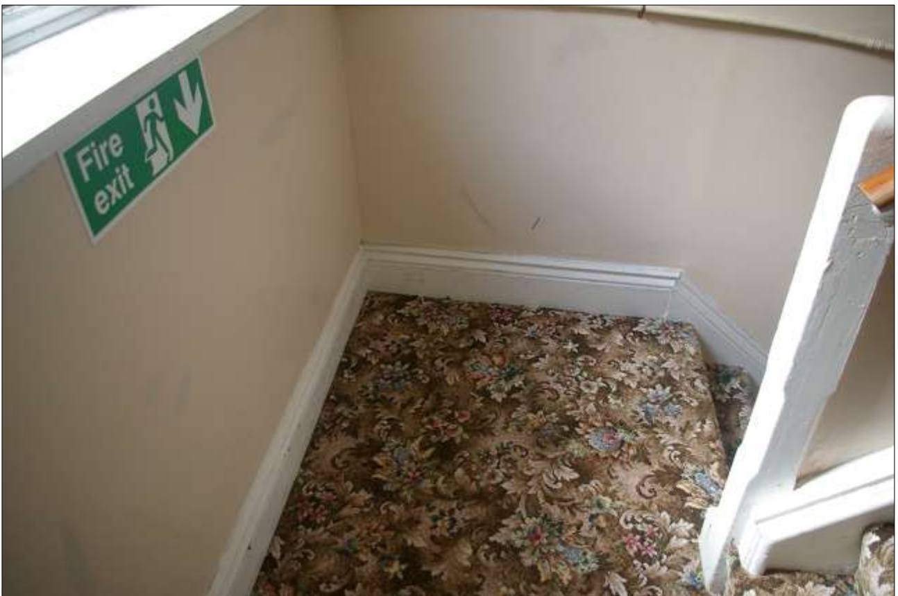
79. DETAIL OF THE SURVIVING SKIRTING BOARDS/STAIR PLATES WITHIN THE ALTERED STAIR AREA IN BLOCK 7A; VIEWED FROM THE NORTH.
