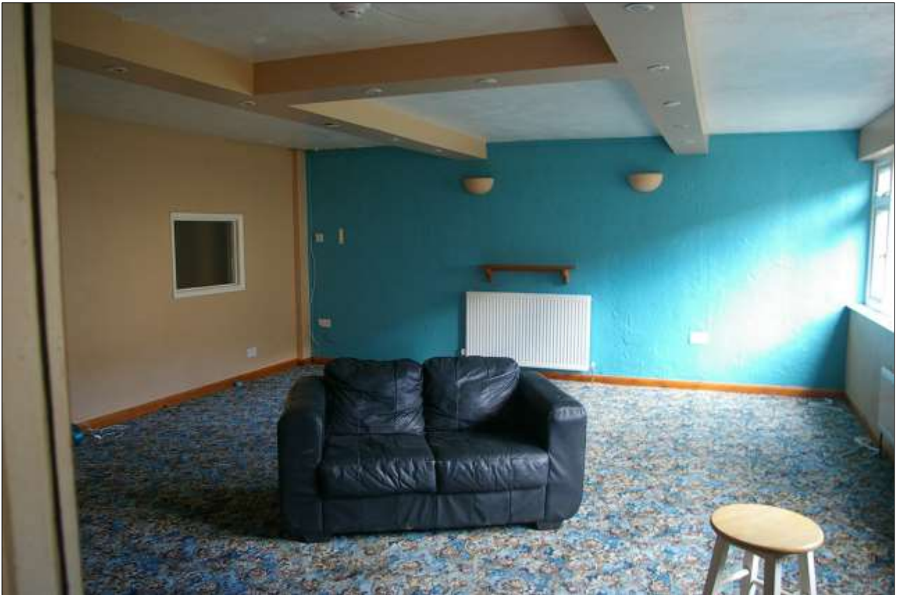
89. THE LARGE MODERN SPACE ON THE GROUND FLOOR CREATED BY INFILLING THE SPACE BETWEEN BLOCK 6 AND BLOCK 7A; VIEWED FROM THE EAST.
