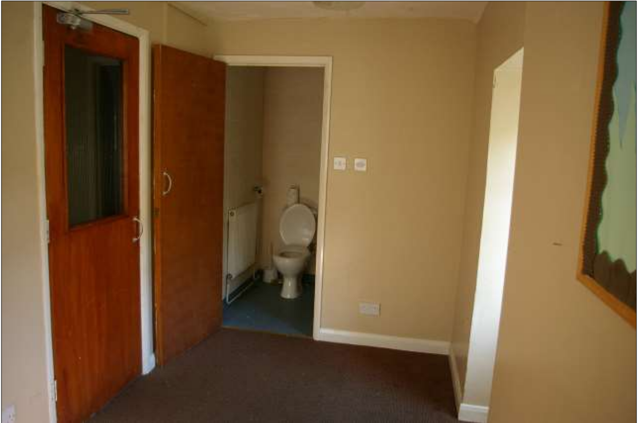
59. ONE OF THE SMALL ROOMS AND BATHROOMS ON THE FIRST FLOOR OF THE MILL, WHICH HAS BEEN DIVIDED UP FOR STAFF ACCOMMODATIONS; VIEWED FROM THE NORTH-EAST.
