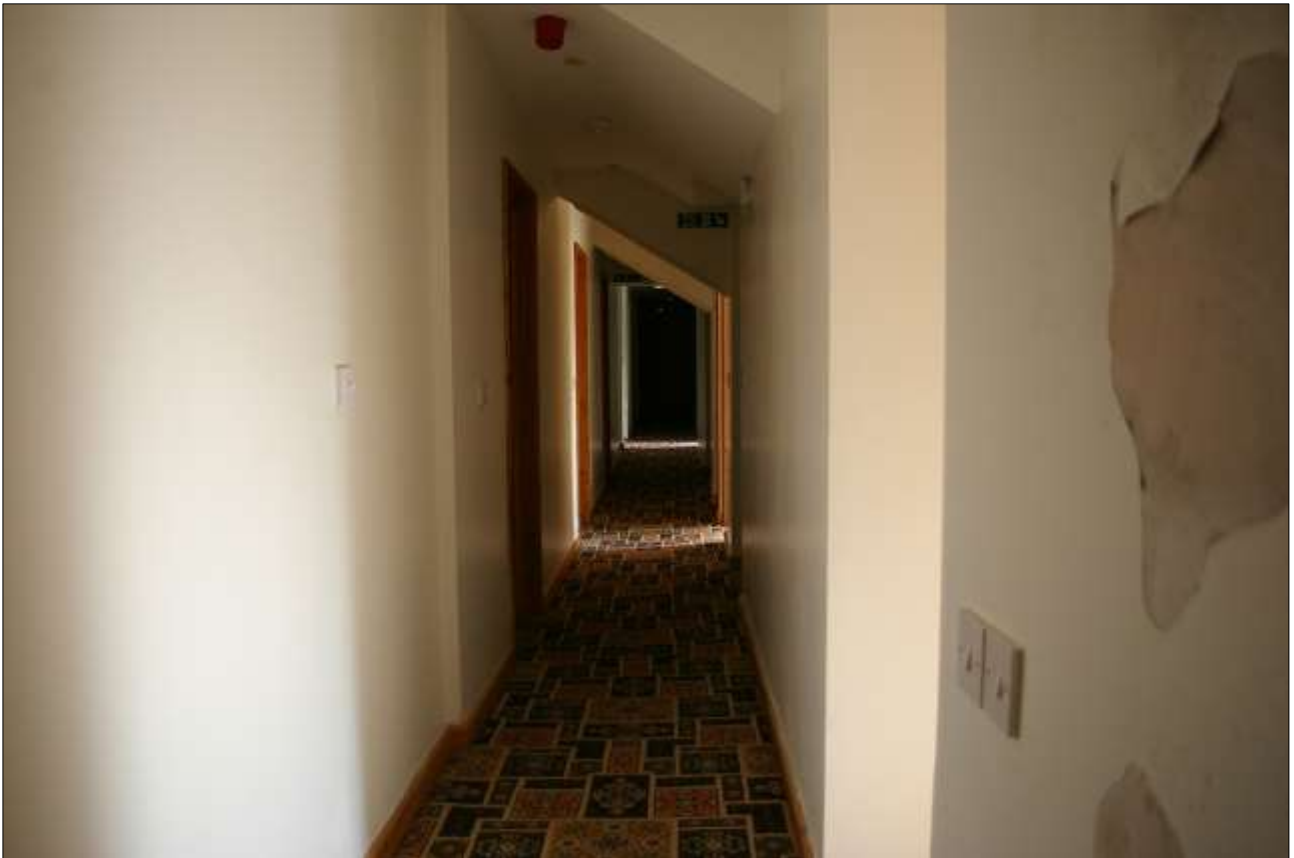
17. FIRST FLOOR CORRIDOR ALONG THE COMBINED FIRST FLOOR OF BLOCK 1; VIEWED FROM THE SOUTH.
