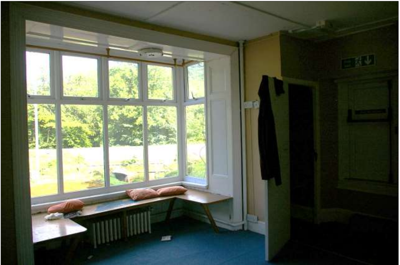
82. ONE OF THE LARGE FRONT WINDOWS ON THE FIRST FLOOR IN BLOCK 7A SHOWING PANELLED SHUTTERS; VIEWED FROM THE SOUTH-EAST.
