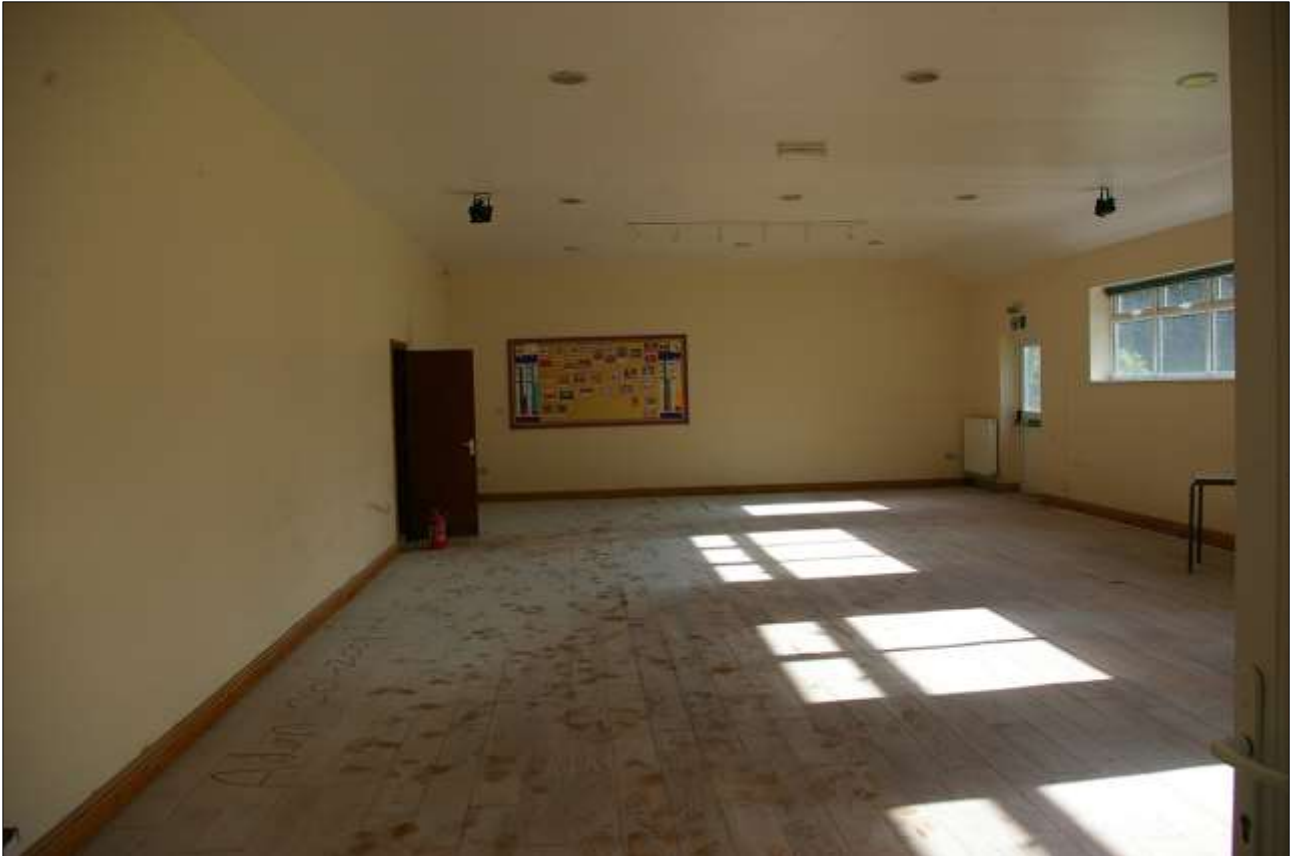
93. THE INTERIOR OF THE MODERN SCHOOL HALL, BLOCK 8; VIEWED FROM THE SOUTH.
