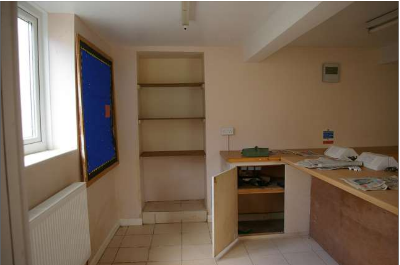
36. THE BLOCKED DOORWAY IN THE EAST WALL OF BLOCK 4A, ON THE GROUND FLOOR; VIEWED FROM THE WEST.
