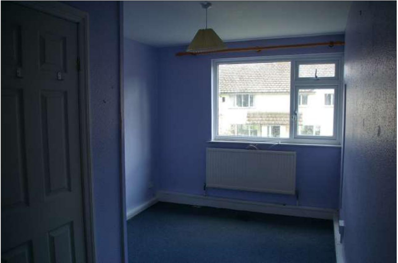
91. ONE OF THE SMALL PURPOSE-BUILT STAFF BEDROOMS IN THE FIRST FLOOR SECTION OF BLOCK 7B; VIEWED FROM THE SOUTH.
