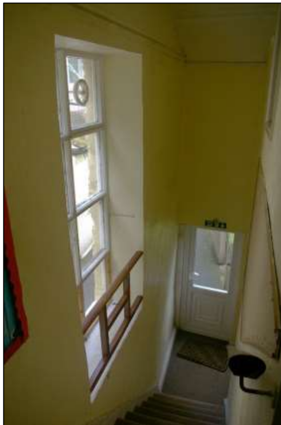
40. THE STAIRS FORCED INTO BLOCK 4A AT ITS SOUTHERN END, LIT BY A TALL WINDOW; VIEWED FROM THE EAST.
