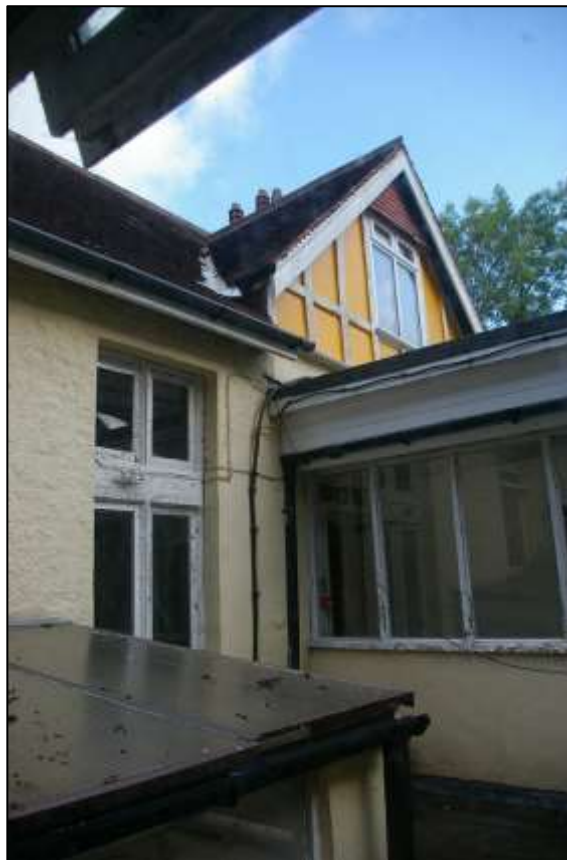
66. THE EAST WALL OF BLOCK 7A AT FIRST FLOOR AND ATTIC LEVEL, WHICH ARE NOT OBSCURED BY ADJOINING STRUCTURES; VIEWED FROM THE SOUTH-EAST.
