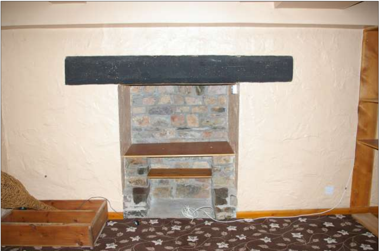
55. BLOCKED OPENING OR FIREPLACE IN THE WEST WALL OF THE MILL; VIEWED FROM THE EAST.
