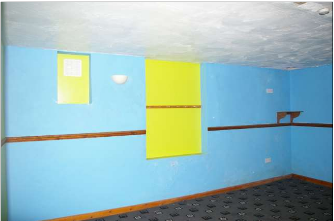
77. THE LARGE GROUND-FLOOR ROOM TO THE EAST OF THE SERVICE RANGE; THE WINDOWS AND FIREPLACE ARE NOW BLOCKED; VIEWED FROM THE NORTH-WEST.
