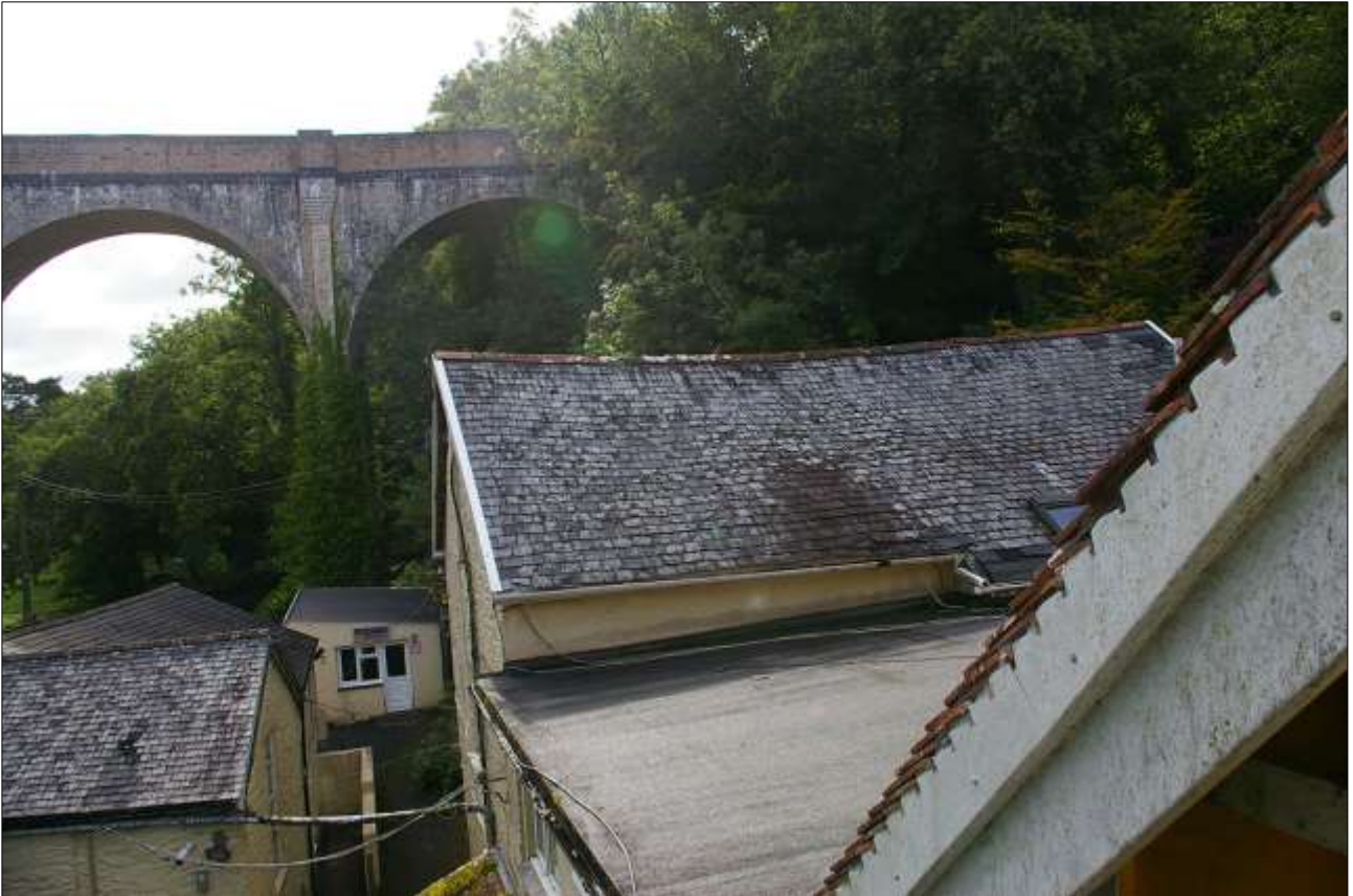
61. VIEW OF THE ROOF OF THE MILL, BLOCK 6; VIEWED FROM THE WEST.
