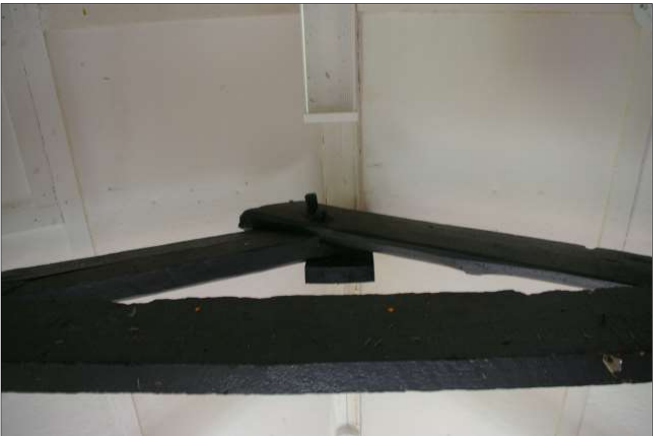
42. PEGS IN THE OVERLAPPING RIDGE OF THE A-FRAME TRUSSES IN BLOCK 4A; VIEWED FROM THE SOUTH.
