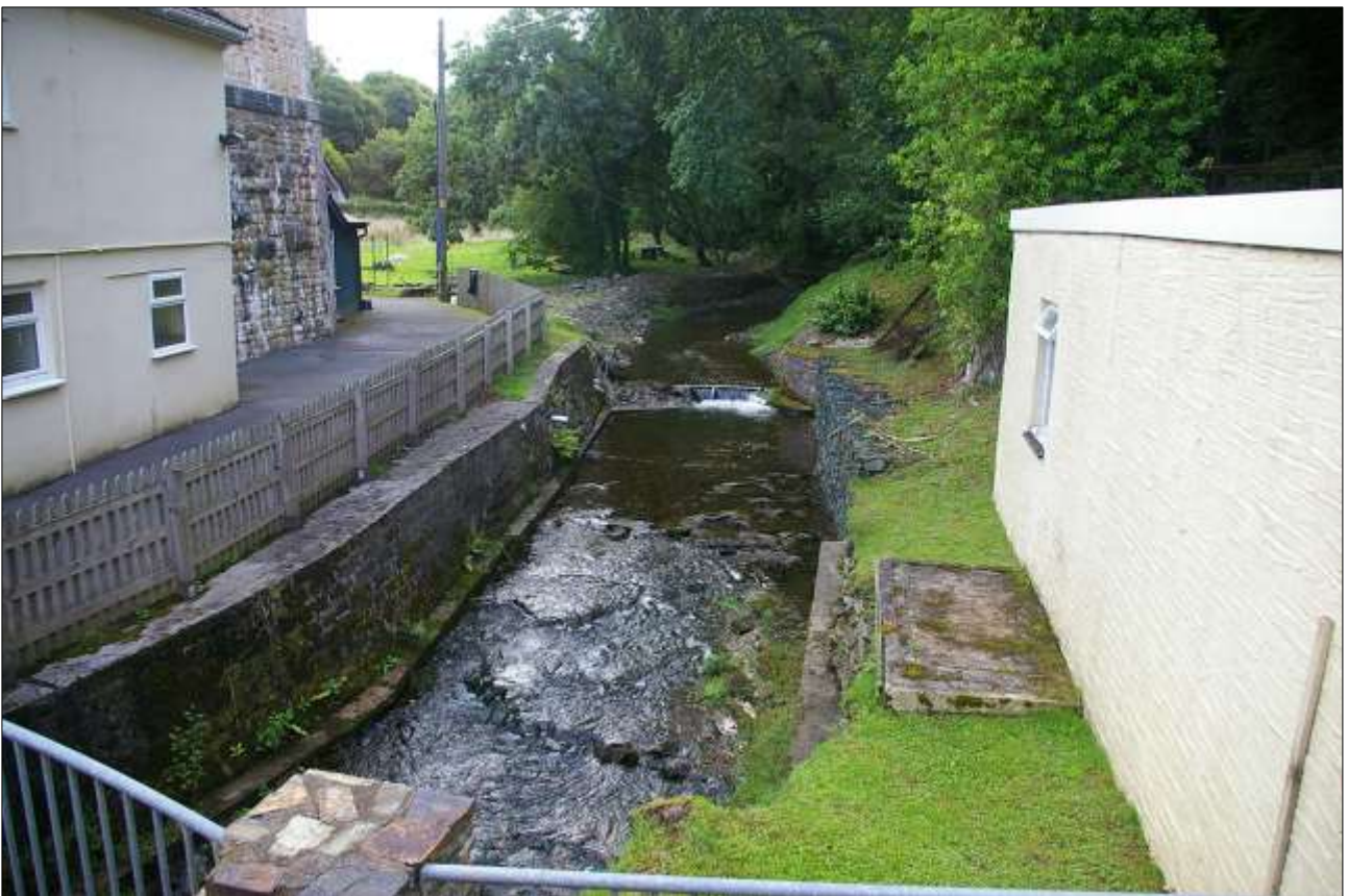
44. THE RIVER WHERE IT RUNS BENEATH THE PIERS OF THE VIADUCT; VIEWED FROM THE WEST.
