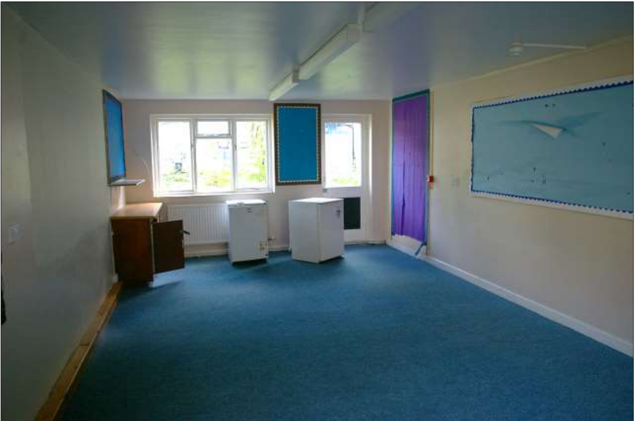
26. ONE OF THE GROUND FLOOR CLASSROOMS IN BLOCK 3; VIEWED FROM THE SSW.
