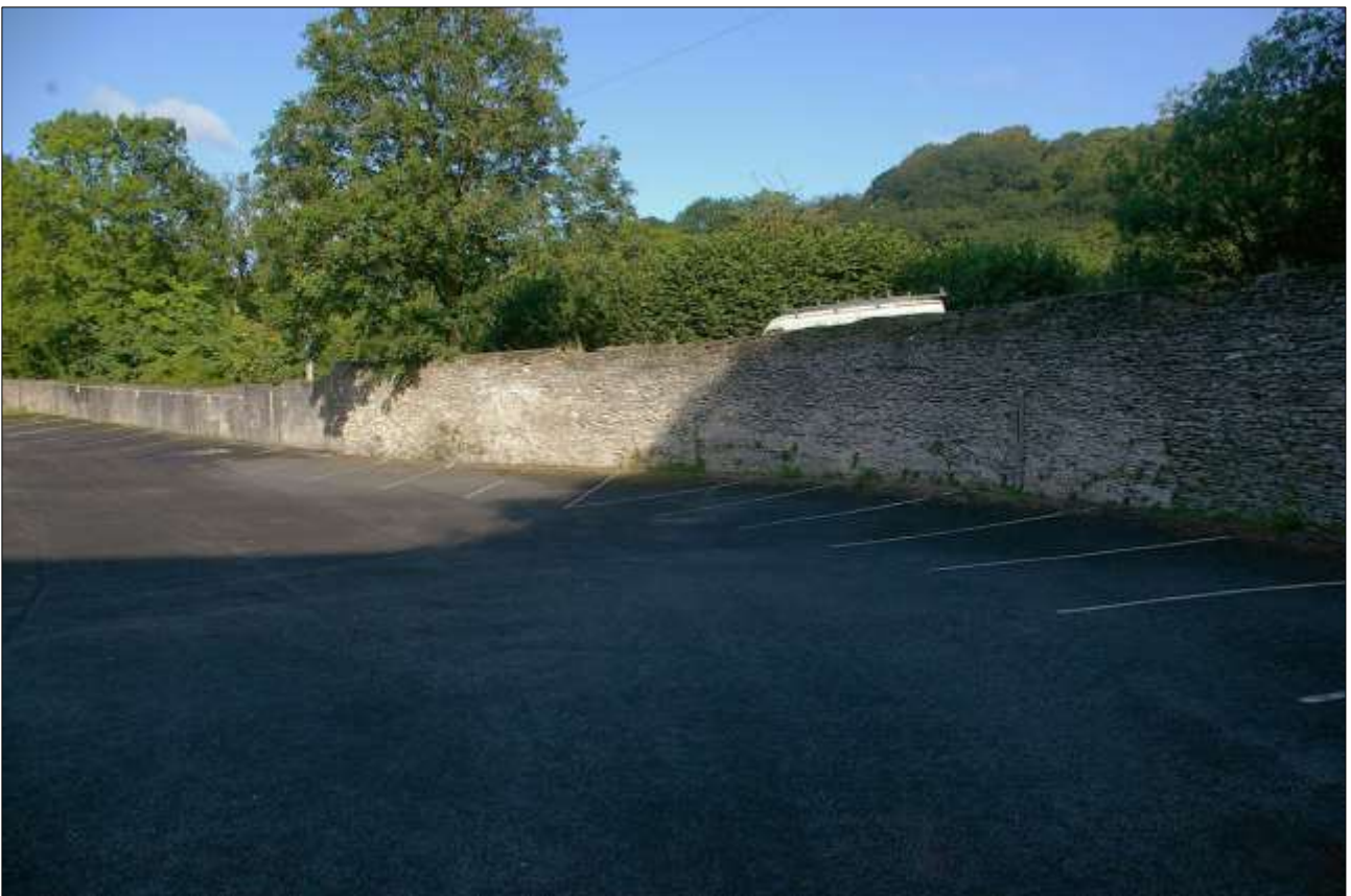
6. DETAILED VIEW OF THE CURVING SLATESTONE RUBBLE PERIMETER WALL THAT ENCLOSED THE FORMER GARDENS; VIEWED FROM THE EAST.
