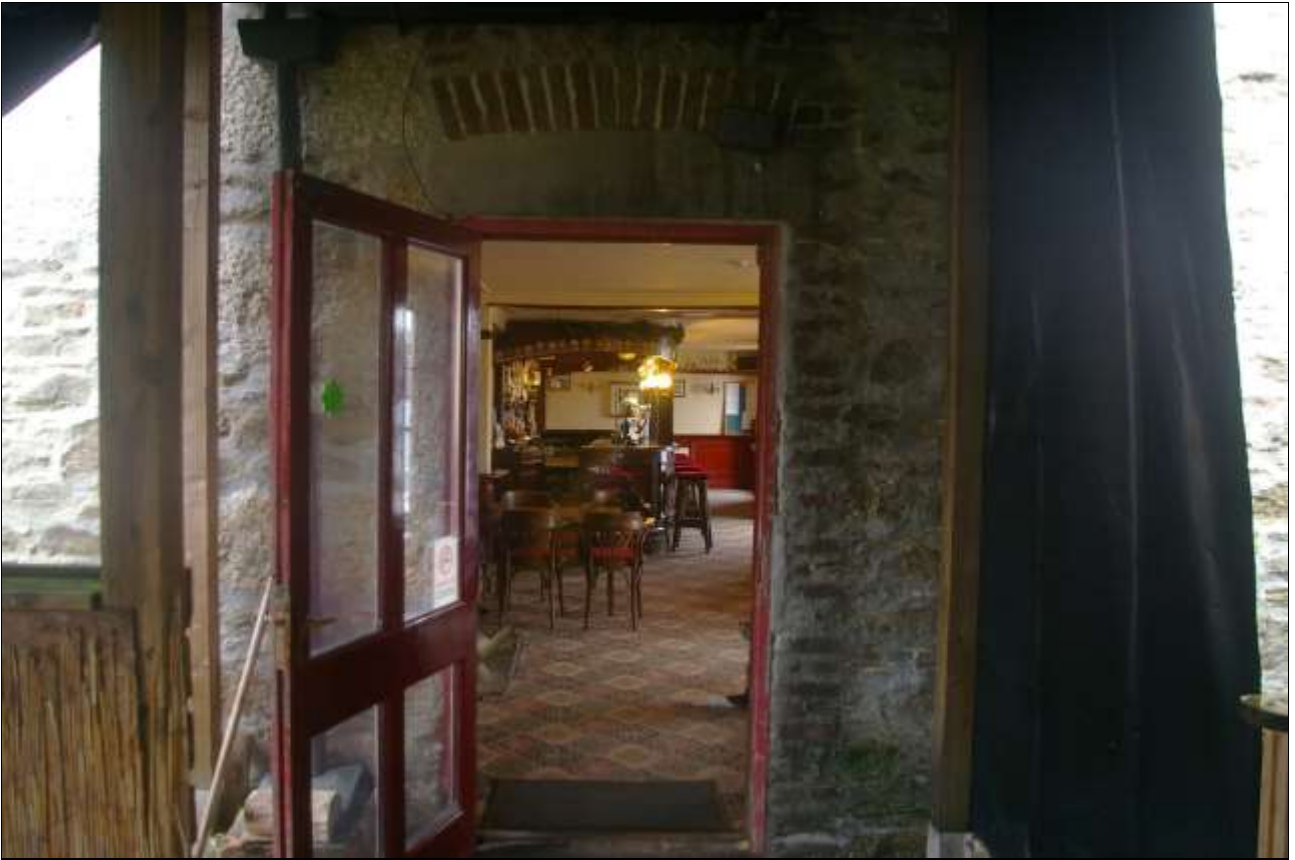
13. VIEW THROUGH D3, THE DOOR FORCED INTO AN EARLIER WINDOW OPENING, HENCE THE HIGHER BRICK SEGMENTAL ARCH AND NEED FOR REPAIR TO THE EAST SIDE; VIEWED FROM THE SOUTH.
