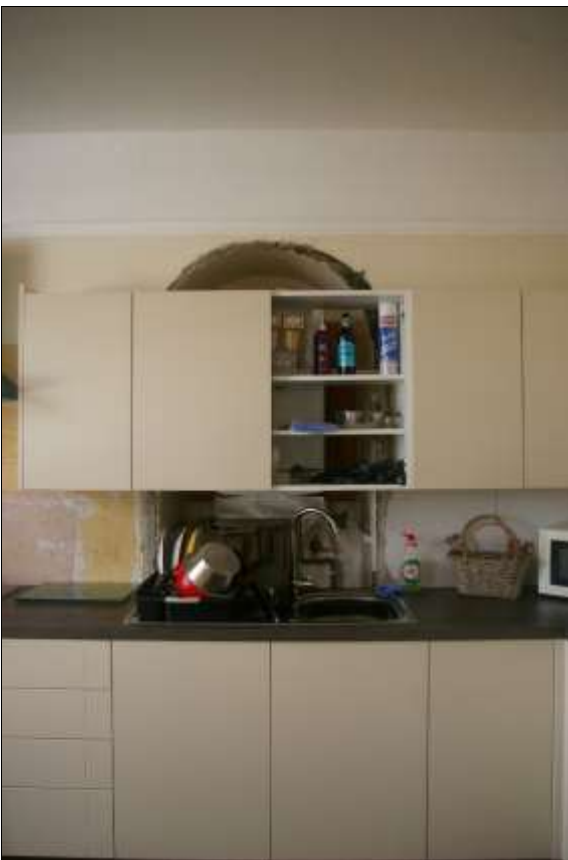
43. R15A, THE BLOCKED OPENING (BO4) IN THE SOUTH WALL; VIEWED FROM THE NORTH.
