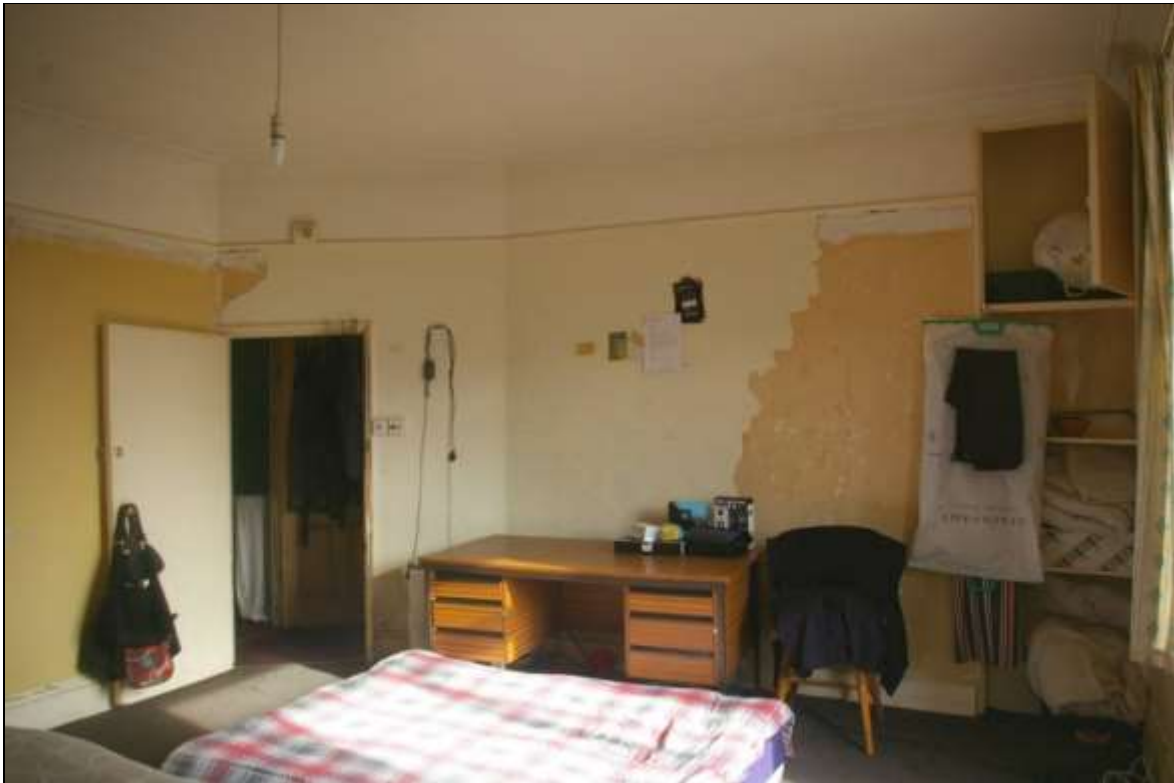
FIGURE 17: R14 WITH THE REEDED CORNICE THAT RESPECTS THE INSERTED PARTITION AND DOOR (LEFT); BLOCKED FIREPLACE (FP4) AND PANELLED CUPBOARD (RIGHT); VIEWED FROM THE SOUTH-WEST.
