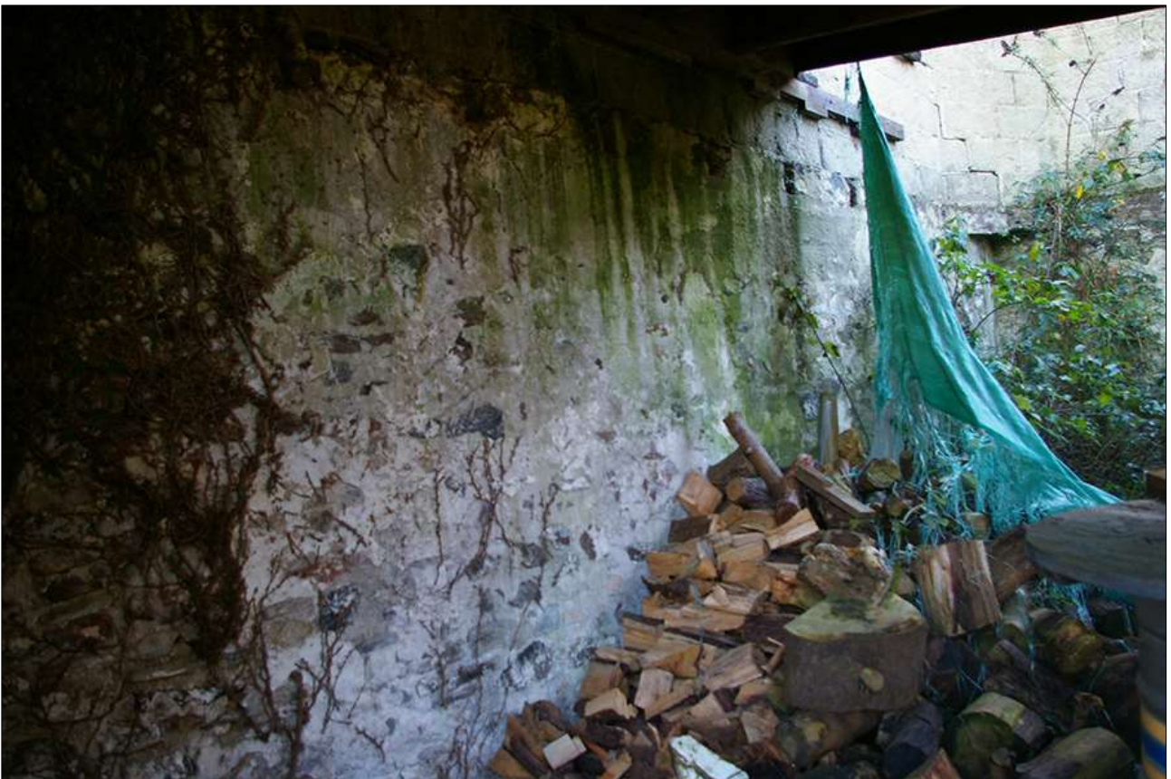
54. DETAIL OF THE INTERNAL EAST ELEVATION OF THE DERELICT OUTBUILDING; VIEWED FROM THE NORTH-WEST.
