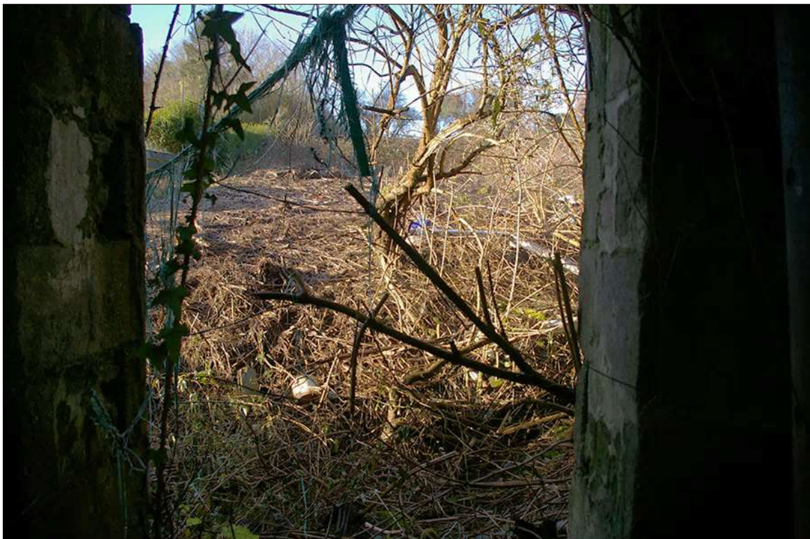
FIGURE 11: VIEW ACROSS THE FIELD FROM THE INTERIOR OF THE DERELICT OUTBUILDING; VIEWED FROM THE EAST.
