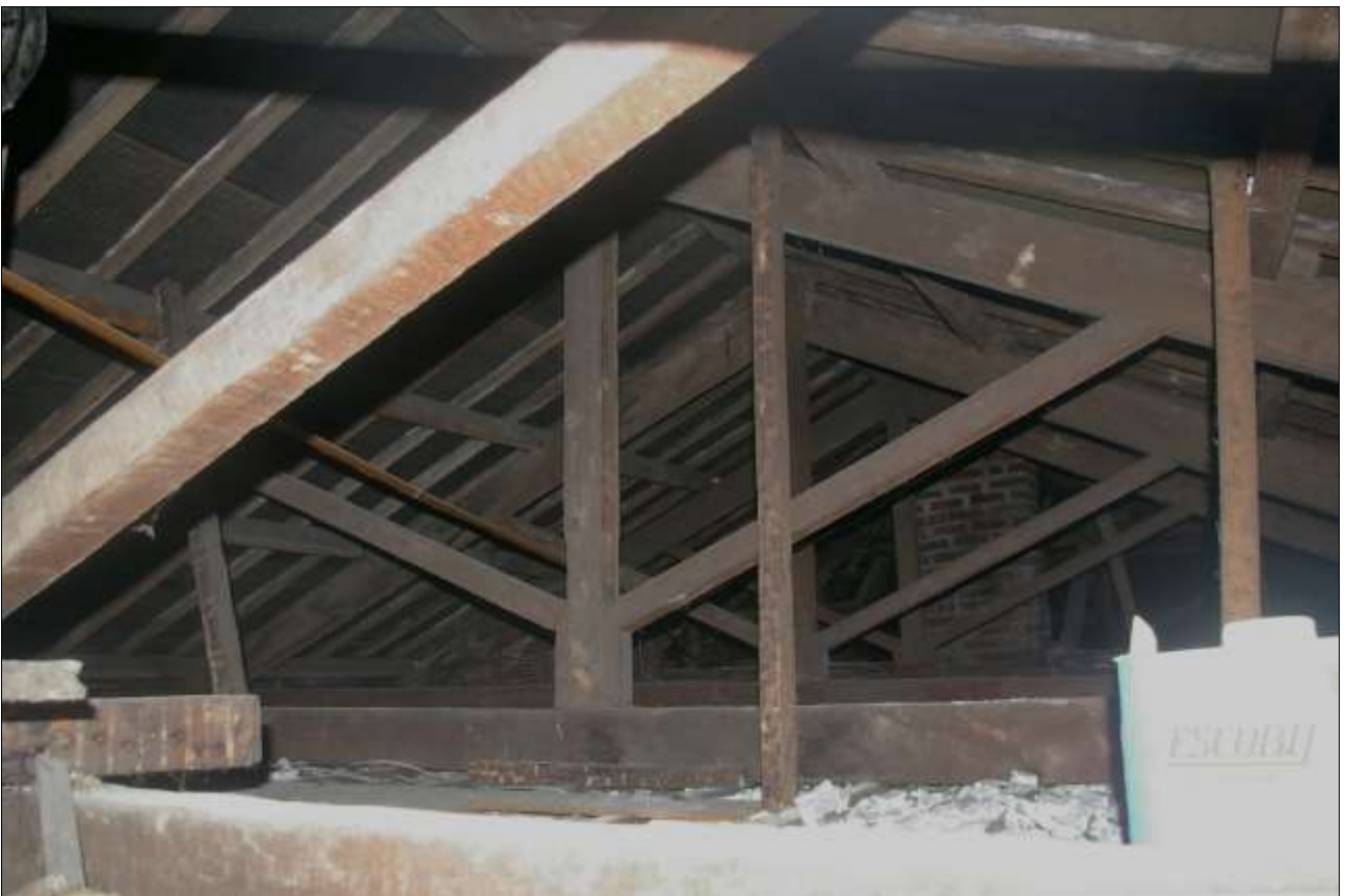
45. THE WIDE SHALLOW ROOF OVER THE WEST BLOCK, A-FRAME KING-POST TRUSSES WITH A STACK TO THE SOUTH END, RAISED IN BRICK WITHIN THE ROOF SPACE; VIEWED FROM THE NORTH-WEST.
