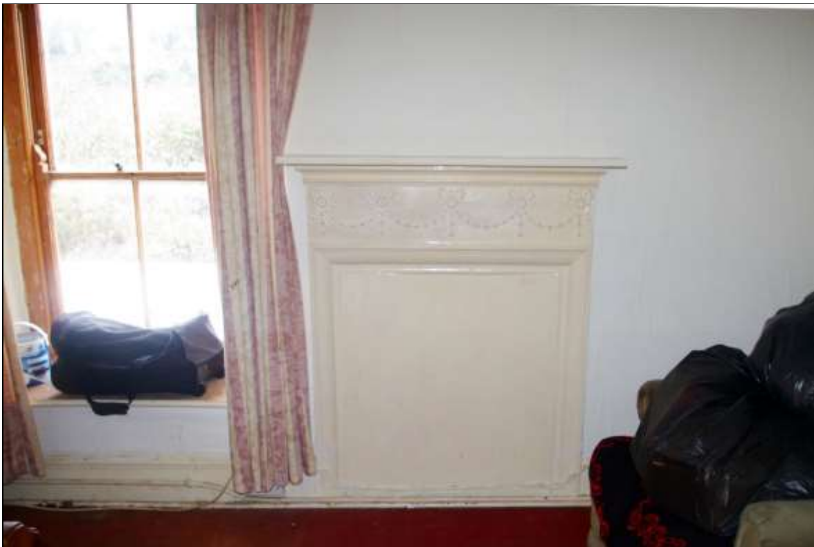
FIGURE 15: BLOCKED FIREPLACE IN ROOM 11 (FP3); VIEWED FROM THE EAST.
