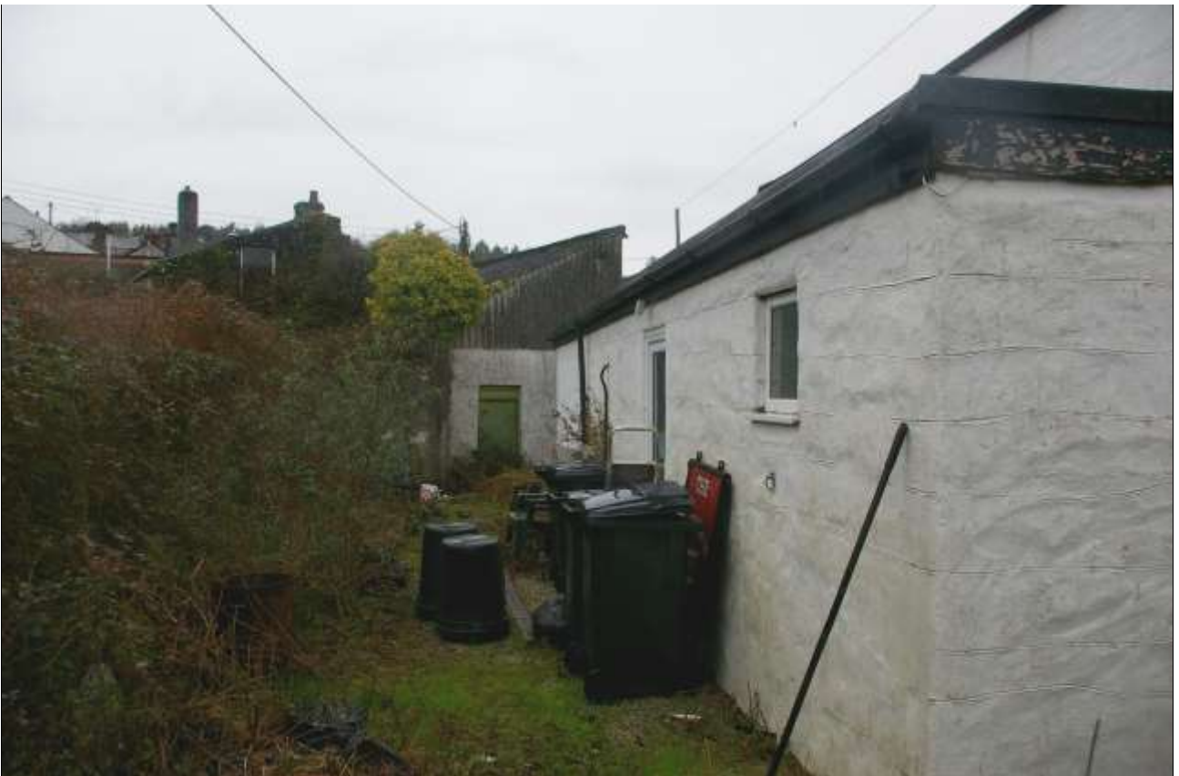
4. VIEW ALONG THE WESTERN ELEVATION OF THE EXTENSION AND THE THICK RETAINING STONE WALLS TO THE NORTH-WEST NOW INCORPORATED INTO THE GARAGE/STORE BUILDING; VIEWED FROM THE SOUTH.
