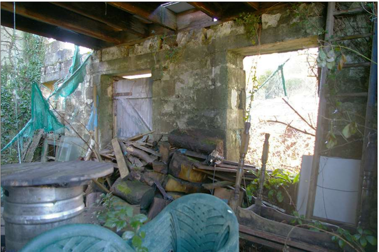
52. DETAIL OF THE INTERNAL WEST ELEVATION OF THE DERELICT OUTBUILDING; VIEWED FROM THE NORTH-EAST.
