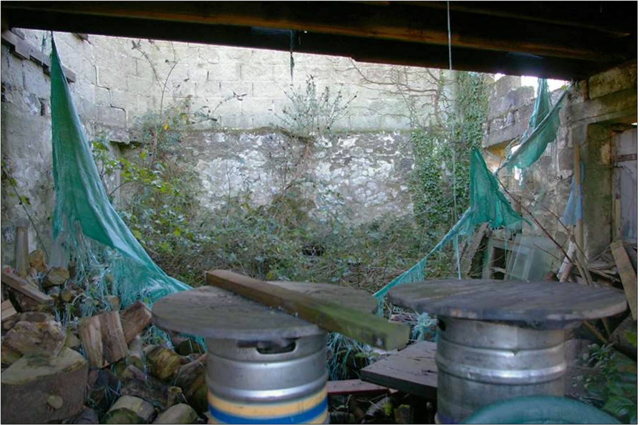
53. DETAIL OF THE INTERNAL SOUTH ELEVATION OF THE DERELICT OUTBUILDING; VIEWED FROM THE NORTH.
