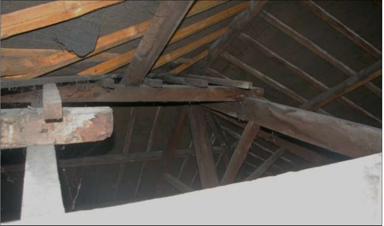
46. THE STEEPER PITCHED ROOF OVER THE SOUTH END OF THE BUILDING, ALSO KING POST A-FRAME, LOOKING AROUND THE END OF THE VALLEY GUTTER; VIEWED FROM THE WEST-NORTH-WEST.
