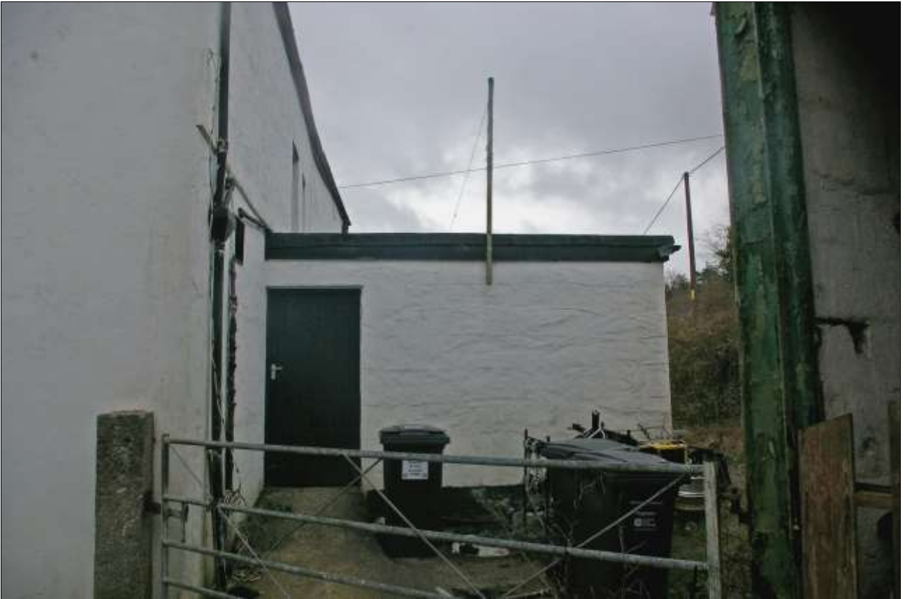
3. THE NORTH ELEVATION OF THE FLAT-ROOFED EXTENSION WITH DOOR TO THE BEER CELLAR; ABOVE, A SLIGHT KINK IN THE WEST ELEVATION OF THE MAIN BUILDING, EVIDENCE OF PHASING; VIEWED FROM THE NORTH.
