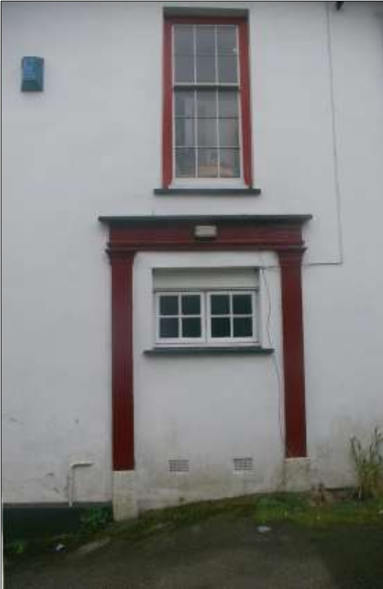
2. THE BLOCKED DOORWAY ON THE NORTH ELEVATION OF THE INN, WITH INSET WINDOW (W4); VIEWED FROM THE NORTH.
