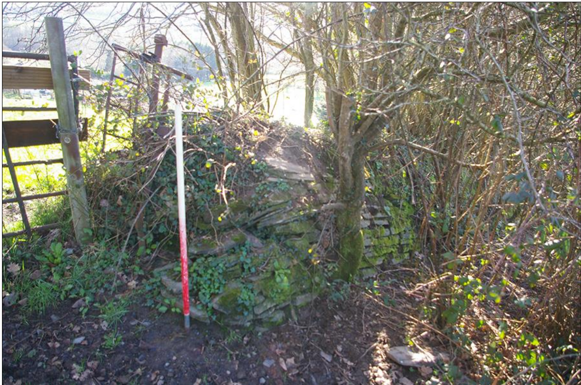
38. DETAIL OF THE STONE FACED HEDGEBANK EASTERN BOUNDARY OF F4; VIEWED FROM THE NORTH (1M SCALE).
