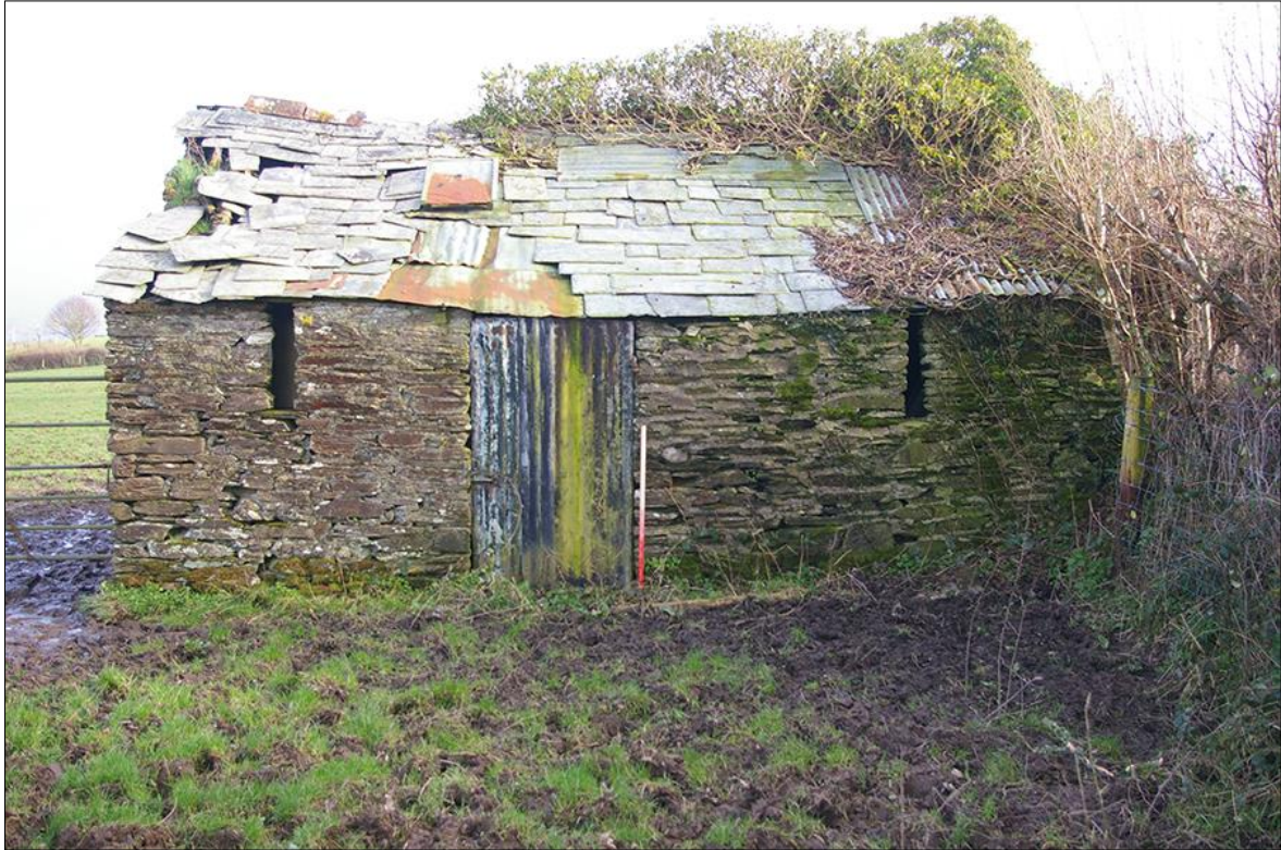
1. WEST-NORTH-WEST ELEVATION OF STRUCTURE IN SOUTH-EAST CORNER OF F1; VIEWED FROM THE WEST-NORTH-WEST (1M SCALE).
