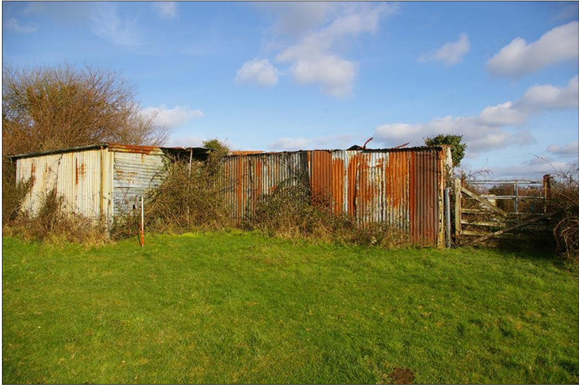
23. DETAIL OF THE CRUDE METAL STRUCTURE IN THE NORTH-EAST CORNER OF F2; VIEWED FROM THE SOUTH (1M SCALE).
