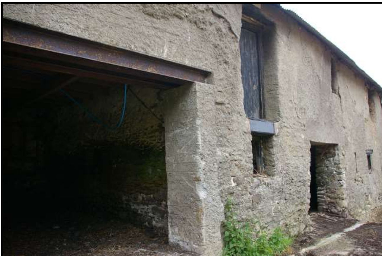
45. THE SOUTH-EAST CORNER OF B2A WITH CONCRETE JAMB OF MODERN OPENING TO B2C (CENTRE LEFT) OBSCURING THE QUOIN STONES; VIEWED FROM THE SOUTH-EAST.
