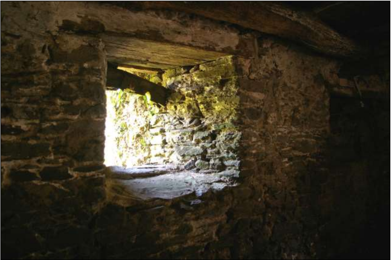
34. THE SMALL WINDOW IN THE NORTH WALL OF B2A REMAINS OF ITS FRAME IN SITU ; VIEWED FROM THE SOUTH-WEST.
