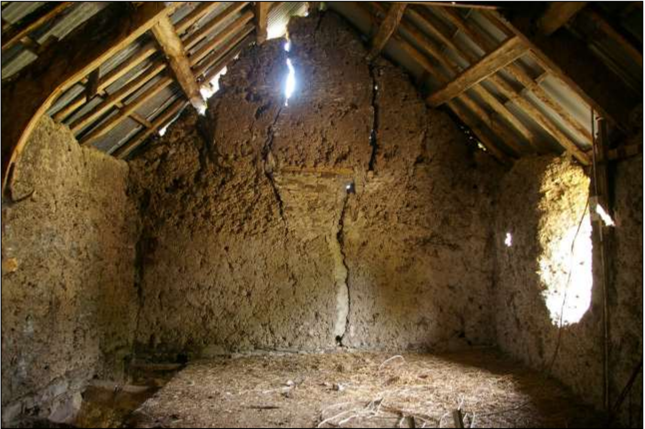
40. THE NORTH END OF LOFT IN B2A. STRUCTURAL CRACKS IN THIS NORTH WALL PROBABLY AROSE DUE TO MOVEMENT OF THE EAST WALL. NOTE THE PRIMARY WINDOW, WHICH MAY HAVE CAUSED THE CRACKS TO START. VIEWED FROM THE SOUTH.
