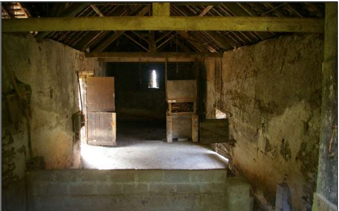
64. THE INTERIOR OF B3A, WITH PLASTERED COB AND STONE RUBBLE WALLS AND REPLACEMENT 19 TH CENTURY TIE BEAM AND KINGPOST ROOF TRUSSES ABOVE. VIEWED FROM THE EAST.
