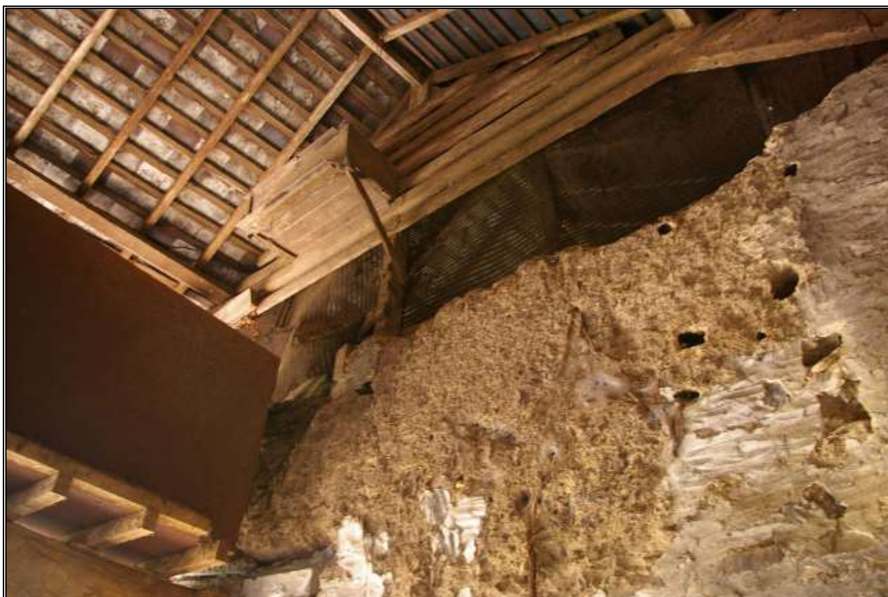
60. THE PART-TIMBERED TRUSS BETWEEN B3B AND B3A, WITH 17 TH CENTURY COB WALL OF B3A AND BAT BOX; VIEWED FROM THE SOUTH-EAST.
