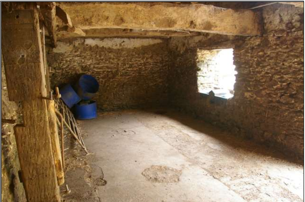
2. THE NORTH END OF B1A; VIEWED FROM THE SOUTH. LARGE PRIMARY CEILING BEAMS AND STALL EVIDENCE.
