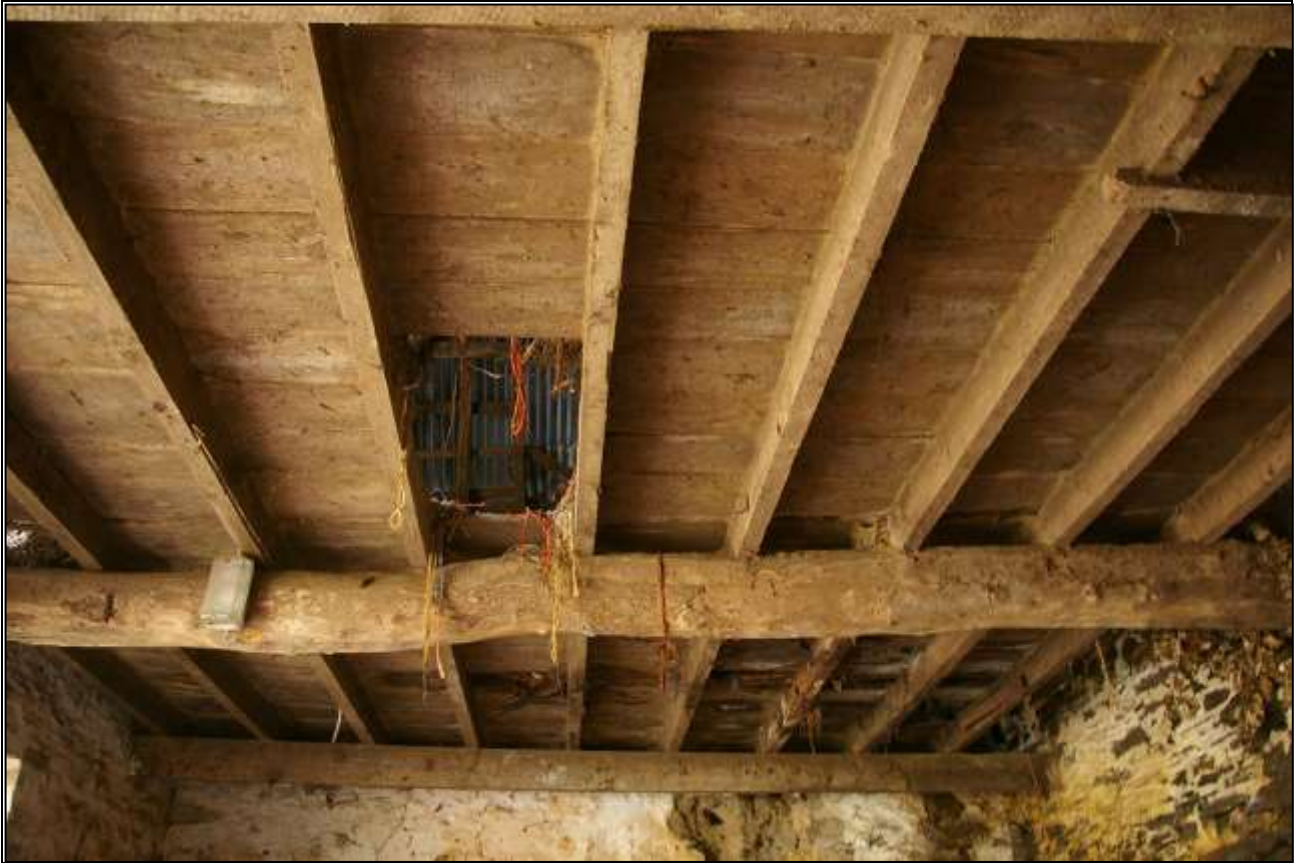
51. THE CEILING STRUCTURE IN B2C, WITH OLD BEAM TO CENTRE AND 20 TH CENTURY LOFT FLOOR ABOVE; VIEWED FROM THE NORTH.
