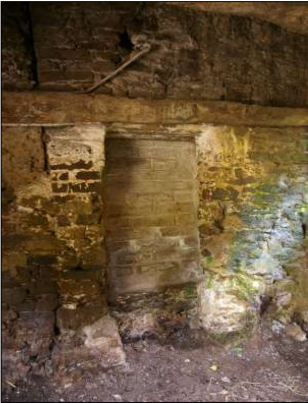
24. FORCED DOOR TO B2A AT THE SOUTH END OF B1C; VIEWED FROM THE NORTH.
