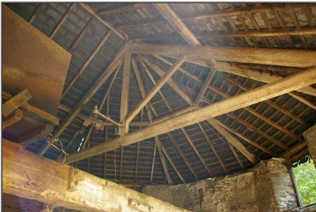
59. LOOKING UP INTO THE ROOF STRUCTURE OF B3B, WITH RADIATING BLADES FROM THE TIE BEAM AND KINGPOST TRUSS SUPPORTING ANGLED ROOF PANELS. LARGE SUPPORT BEAM FOR HORSE ENGINE IS AT LOWER LEFT. VIEWED FROM THE NORTH-WEST.
