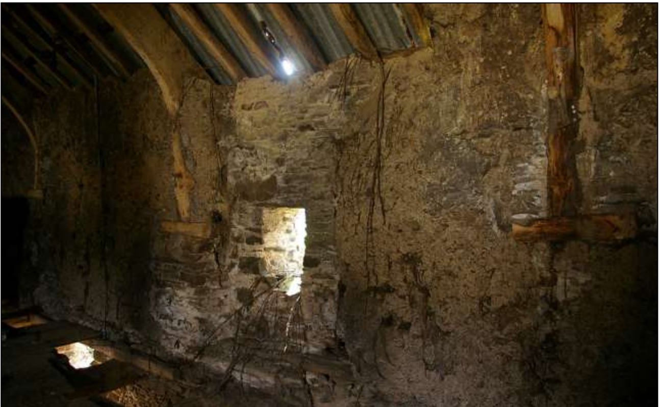
41. THE WEST WALL IN B2A WITH RAISED CRUCK FEET ON TIMBER PADS. NOTE THE BLOCKED LOADING DOOR WITH SMALL WINDOW AND MORTARED RUBBLE UNDERPINNING OF TRUSS FOOT. VIEWED FROM THE NORTH-EAST.
