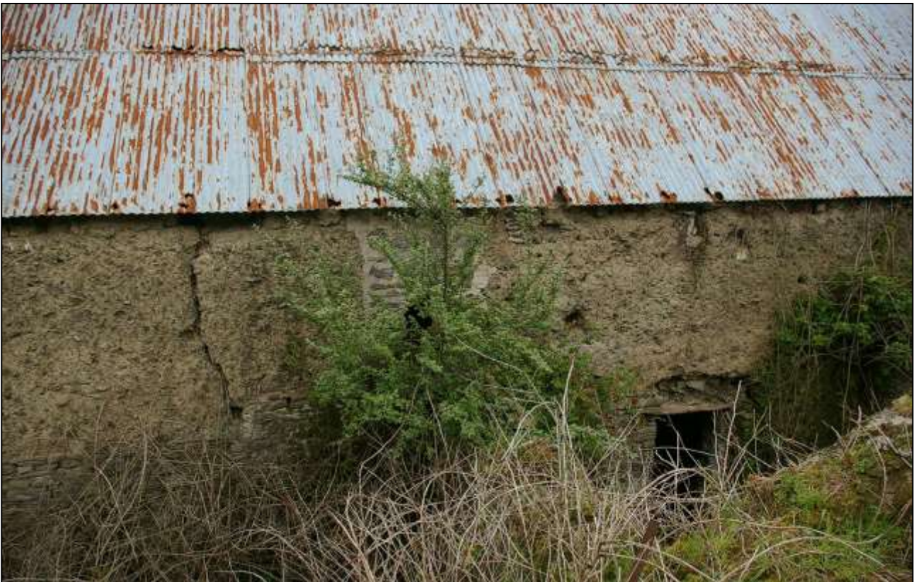
17. WEST WALL OF B1C WITH BLOCKED FIRST-FLOOR LOADING DOOR AND GHOST OF ROOT HOUSE ROOF IN COB WALL FACE; VIEWED FROM THE WEST.
