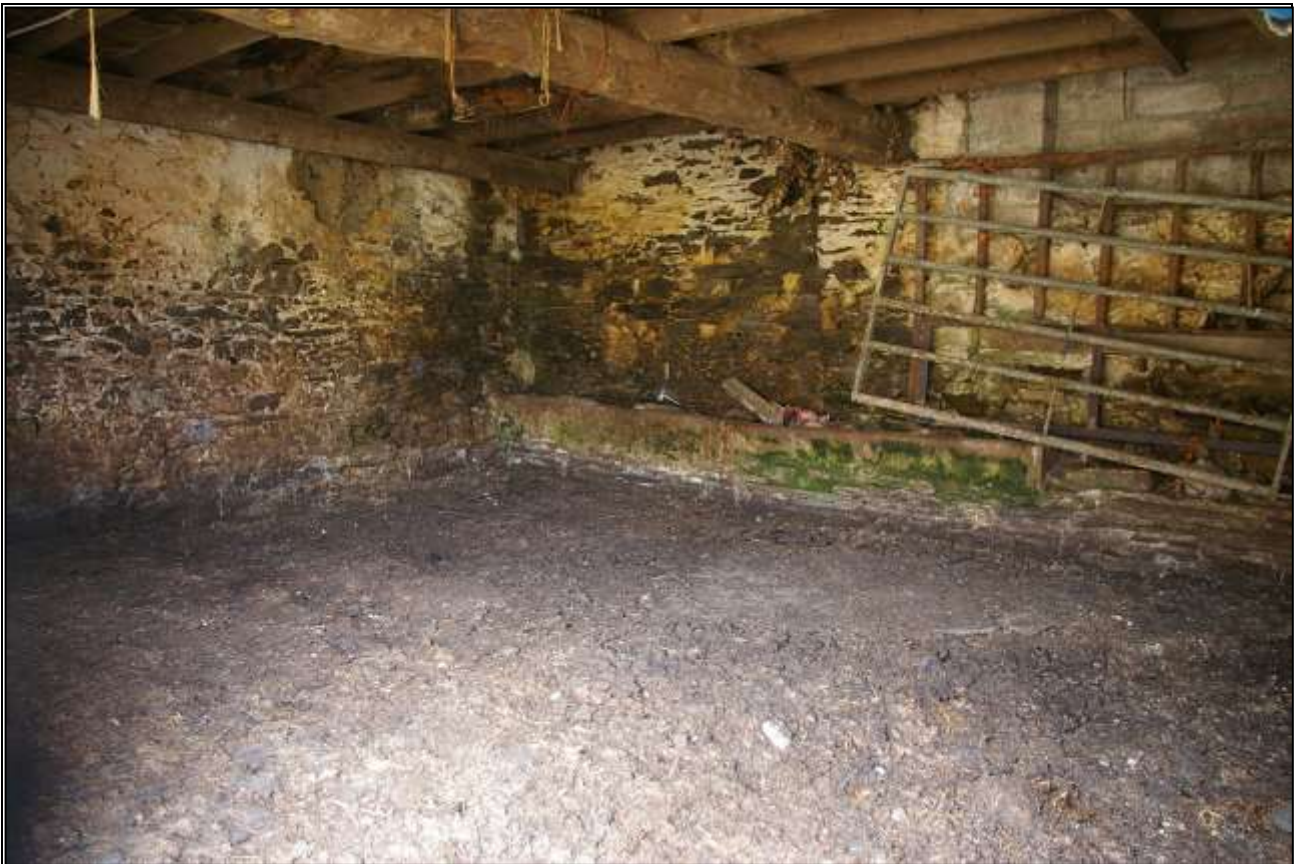
50. THE SOUTH-WEST CORNER OF B2C, WITH CONCRETE BLOCKWORK TO RIGHT REPLACING FAILED COB; VIEWED FROM THE NORTH-EAST.
