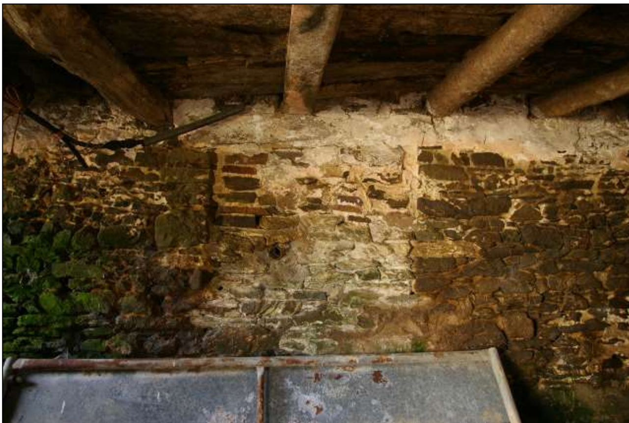
38. BLOCKED PRIMARY WINDOW IN THE SOUTH WALL B2A; VIEWED FROM THE NORTH.
