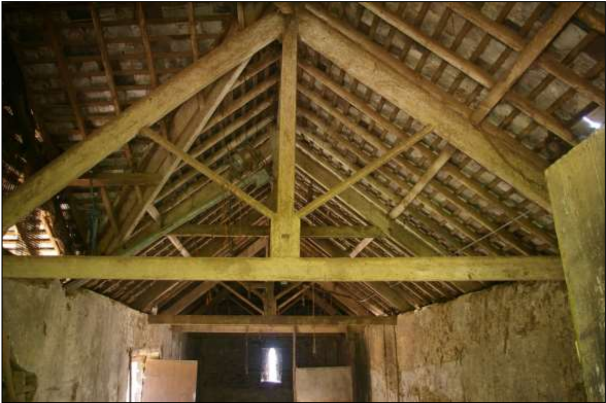
FIGURE 30: THE INTERIOR OF B3A SHOWING THE 19 TH CENTURY TIE BEAM AND KINGPOST ROOF; VIEWED FROM THE EAST.
