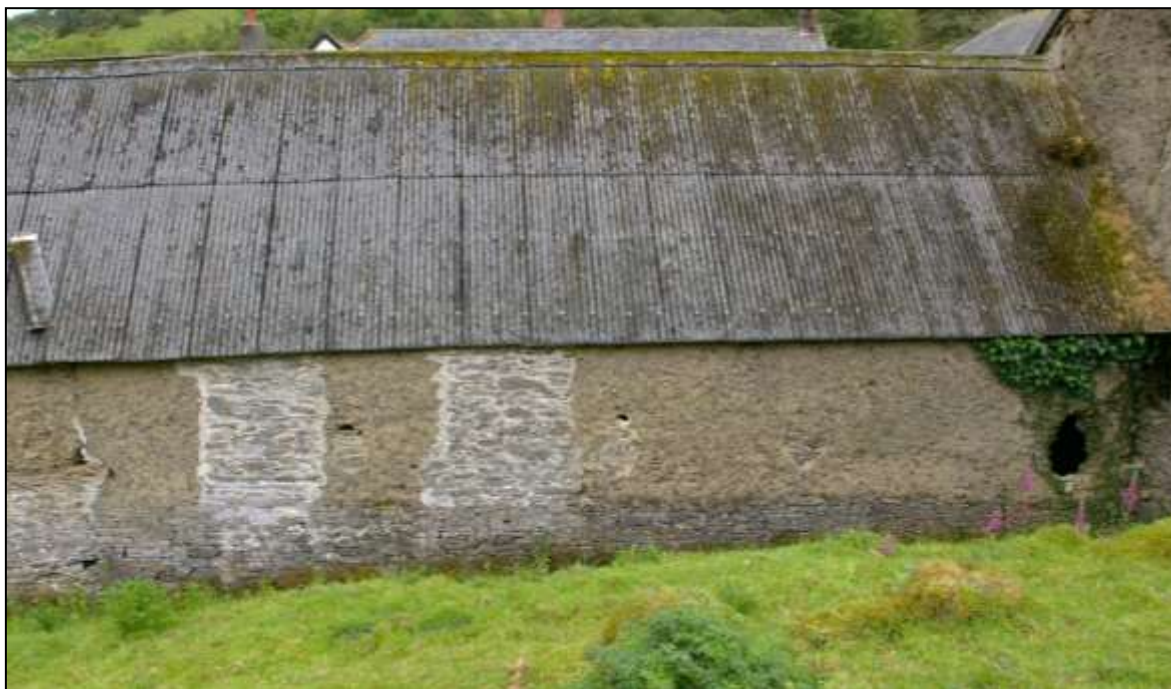
FIGURE 16: WEST (REAR) ELEVATION OF B1c; VIEWED FROM THE WEST. NOTE PATCHED HOLES WHERE FIRST-FLOOR BEAMS WERE INSERTED. THE TWO BLOCKED LOADING DOORS WERE ALSO FORCED INTO THE COB WALL.
