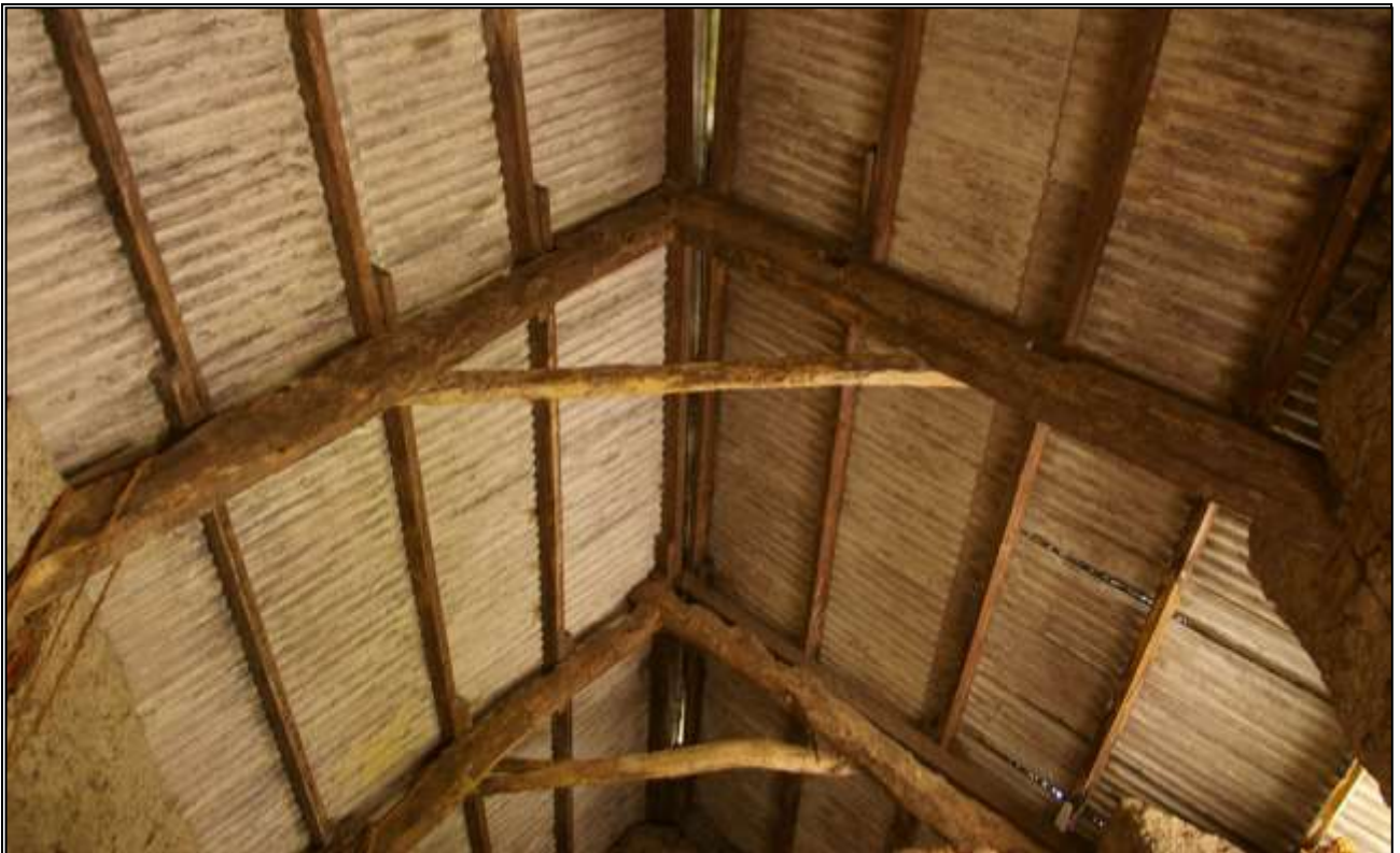
6. OLD ROOF TRUSSES OVER B1A. RIGHT BLADE OF NEAREST TRUSS IS A RE-USED 17 TH CENTURY TIMBER; VIEWED FROM THE NORTH.
