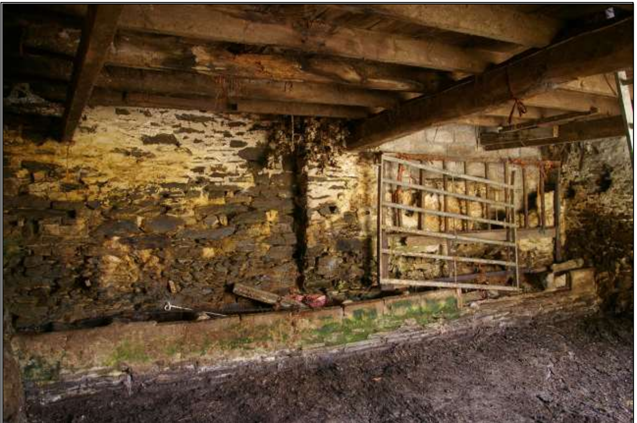
48. WEST WALL OF B2C WITH STUB OF REMOVED CROSS-WALL TO CENTRE AND 19 TH CENTURY FLOOR ABOVE; VIEWED FROM THE EAST.
