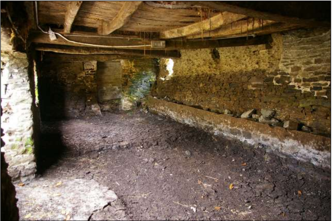
18. SOUTHERN HALF OF B1c, WITH BLOCKED LOADING DOOR IN REAR WALL ON RIGHT, APPARENTLY PREDATING THE BOWED CEILING STRUCTURE; VIEWED FROM THE NORTH-EAST.
