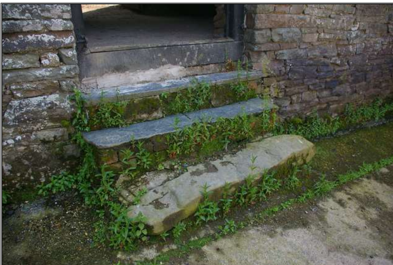
56. DETAIL OF THE 19 TH CENTURY STEPS UP TO THE DRAUGHT DOOR ON THE NORTH SIDE OF THRESHING BARN B3A. BLUE WELSH SLATE ON BRICK RISERS AND POSSIBLE RE-USED GATEPOST AT THE BASE. VIEWED FROM THE NORTH-EAST.
