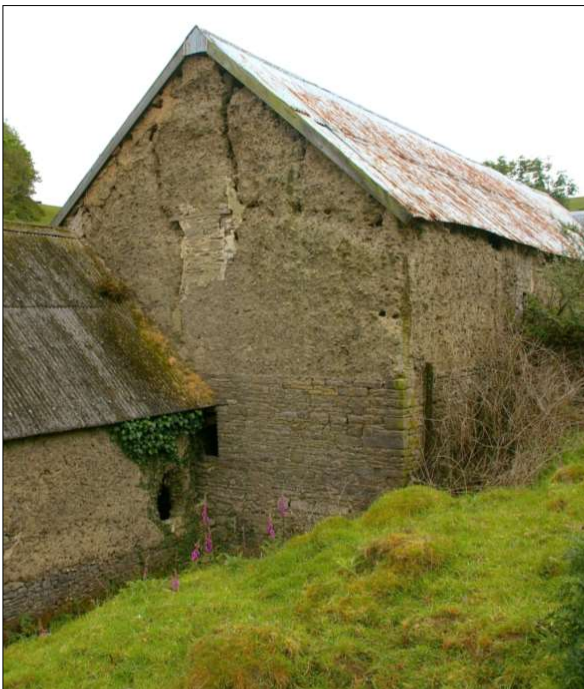
FIGURE 20: THE NORTH GABLE OF B2A; VIEWED FROM THE NORTH-WEST. NOTE THE STRUCTURAL CRACKS.
