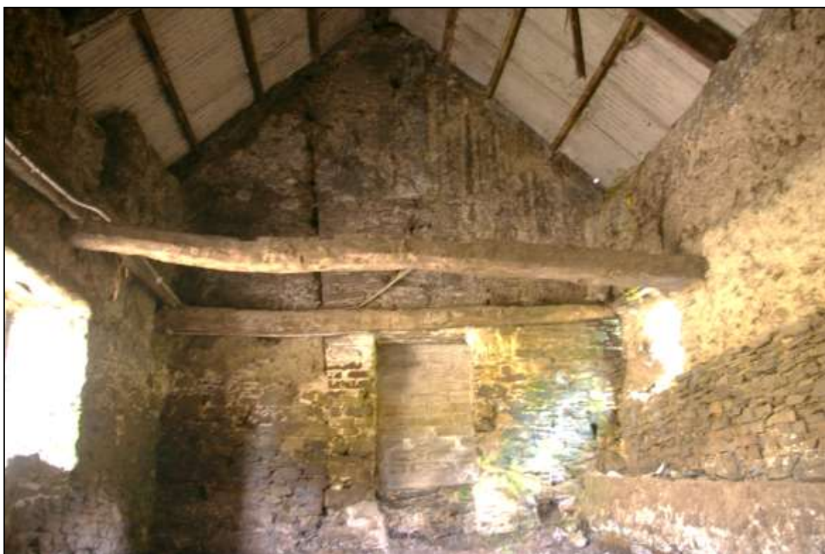
FIGURE 17: THE SOUTH END OF B1c; VIEWED FROM THE NORTH. NOTE THE VERTICAL JOIN WHERE B1c ABUTS B2a TO THE SOUTH, AND HOW THE FRONT WALL OF B2a LEANS OUT TO THE EAST.
