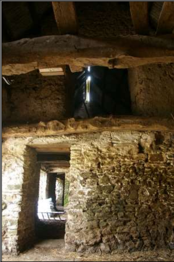
5. SOUTH GABLE OF B1A WITH UPPER LOADING DOOR; VIEWED FROM THE NORTH.
