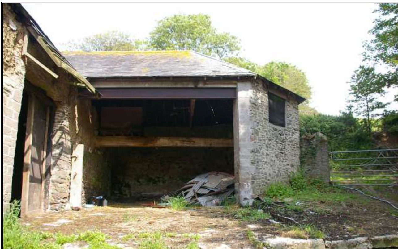
58. WEST ELEVATION OF 19 TH CENTURY HORSE ENGINE HOUSE B3B, WITH LARGE 20 TH CENTURY OPENING IN FORMERLY CLOSED WALL. NOTE MORTARED RUBBLE GATE PIER ABUTTING ON RIGHT, CLOSING THE SOUTH-EAST CORNER OF THE FARMYARD. VIEWED FROM THE WEST.
