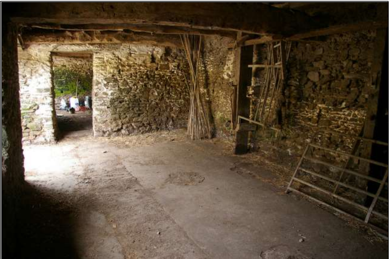
4. SOUTH END OF B1A, GROUND FLOOR, WITH FORCED DOOR TO B1B; VIEWED FROM THE NORTH.
