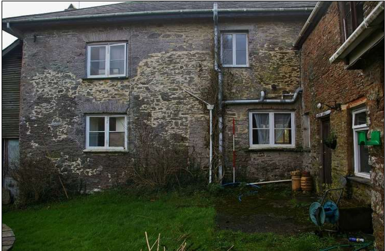
FIGURE 7: THE NORTH ELEVATION OF THE MAIN RANGE, WITH 2M SCALE; FROM THE NORTH.
