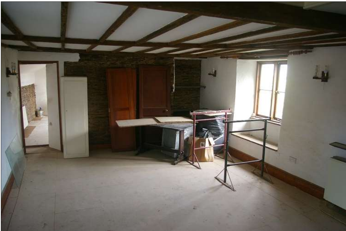
65. R19 OVER THE KITCHEN, THE NORTH ALTERED WALL, WITH FORCED DOOR AND BLOCKED OPENING TO THE EAST AND LANK WINDOW SEAT BELOW REPLACEMENT WINDOW IN THE EAST WALL; FROM THE SOUTH-WEST.
