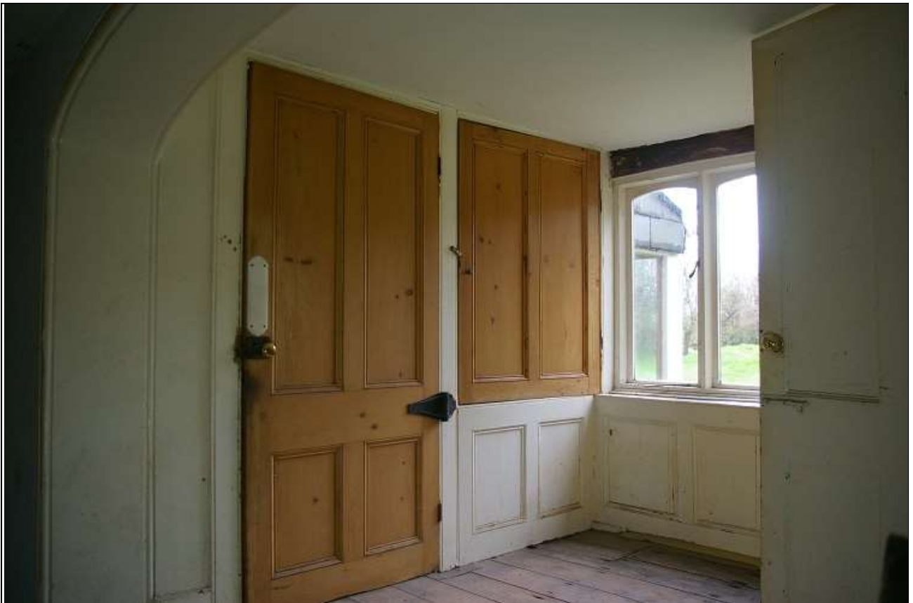
11. THE DOORS AND PANELLING WITHIN THE STAIR PROJECTION R2B, AGGRANDISING THE MAIN SPACE R2A; FROM THE WEST-NORTH-WEST.
