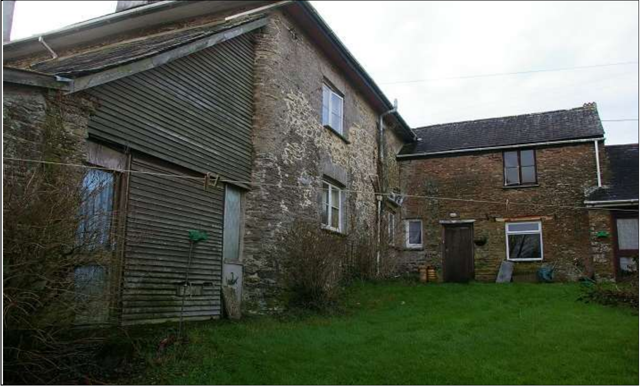
74. VIEW OF THE NORTH ELEVATION OF THE MAIN RANGE AND EAST WALL OF THE REAR SERVICE WING; FROM THE EAST-NORTH-EAST.
