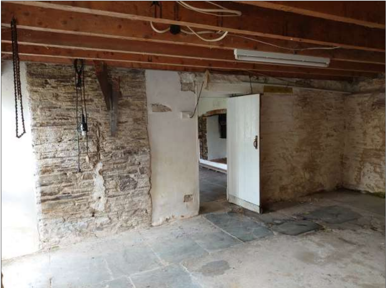
34. THE NORTH WALL OF THE ONE AND A HALF STOREY KITCHEN BLOCK, AS SEEN WITHIN R8; FROM THE NORTH-EAST.
