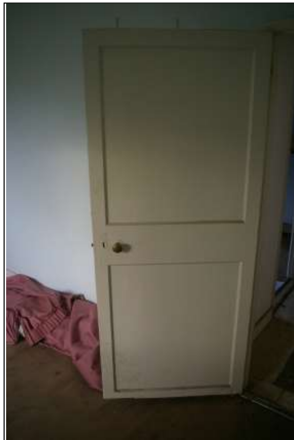
55. THE GOOD LATER 17 TH OR EARLY 1700S TWO PANEL DOOR IN R15, GOOD L-H HINGES, BUT LIKELY RESET WITHIN THE BUILDING, ON A THIN BEADED FRAME; FROM THE SOUTH.
