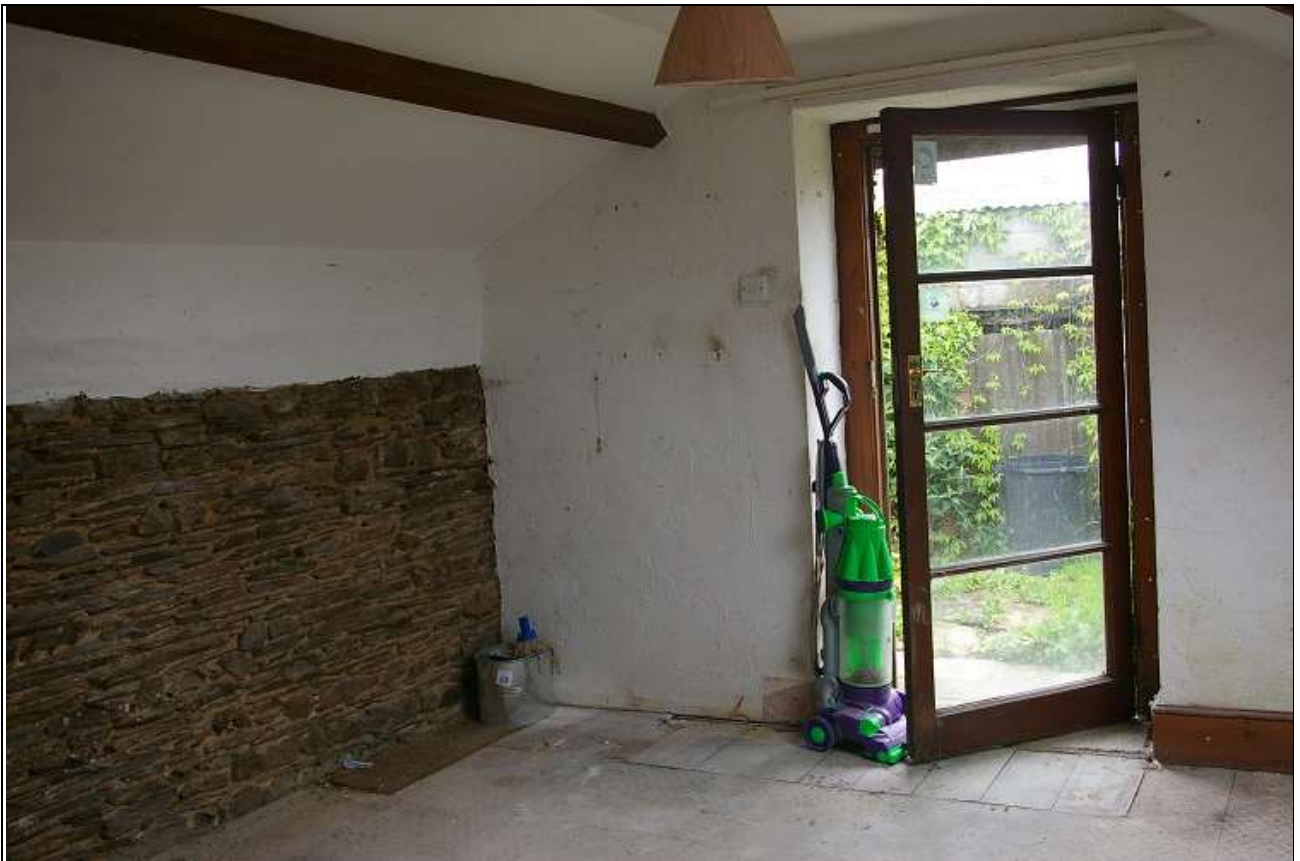
69. R20, THE NORTH WALL, WITH GLAZED DOOR OPENING ONTO THE TERRACED SLOPE OF THE BANK; FORM THE SOUTH-EAST.
