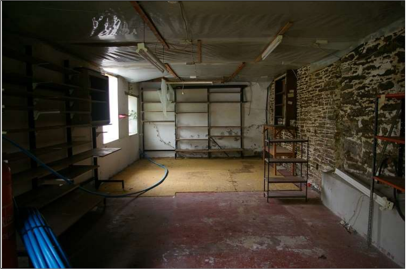
82. OB1, INTERIOR OF THE LARGER LEAN-TO SHED WHICH ABUTS THE EAST WALL OF THE HOUSE; FROM THE NORTH.
