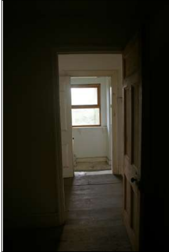
60. VIEW FROM R17, THROUGH R10 AND INTO R9B AT THE WEST END OF THE MAIN RANGE, SHOWING THE LINK BETWEEN MAIN RANGE AND WEST WING; FROM THE NORTH.
