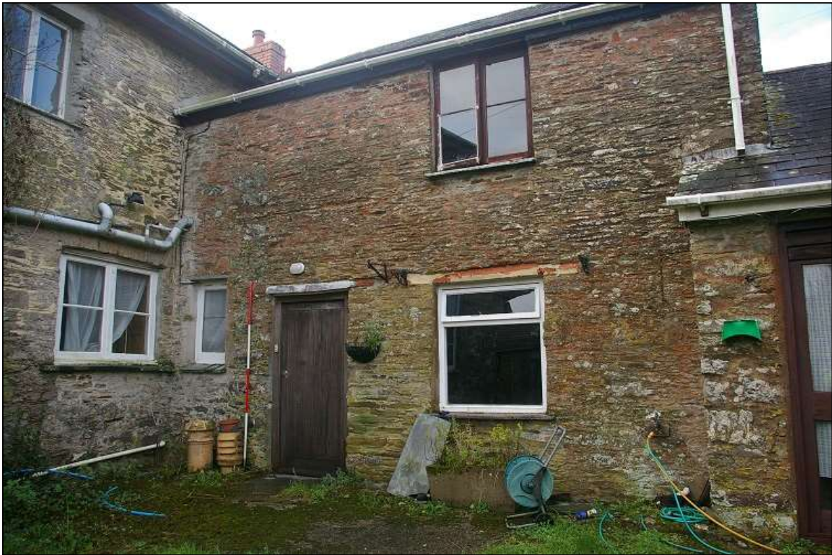
FIGURE 10: THE EAST WALL OF THE REAR SERVICE WING, WITH 2M SCALE; FROM THE EAST-NORTH-EAST.
