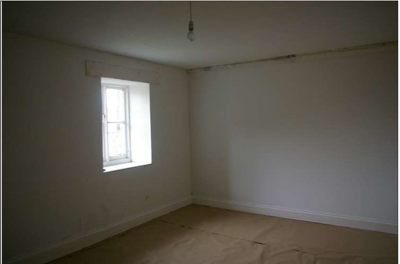
51. R13, CHAMBER OVER HALL, WITH LONG MOULDED BEAM WHICH SEEMS TO BRACE THE END OF THE FORMER HALL AND RUNS THROUGH TO THE EAST EXTENDED WING; FROM THE NORTH-EAST.
