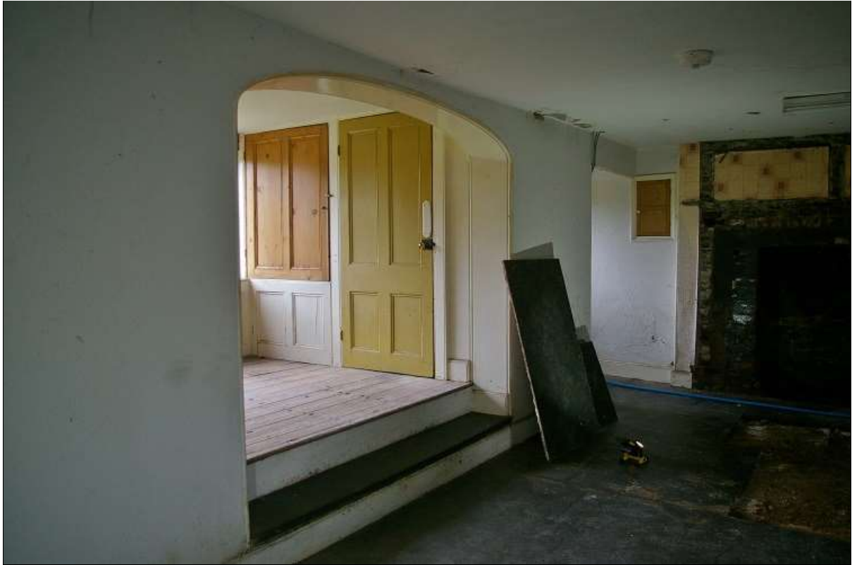
5. THE SOUTH WALL OF R2A, SHOWING THE ADDITION OF THE STAIR PROJECTION; FROM THE EAST-NORTH-EAST.
