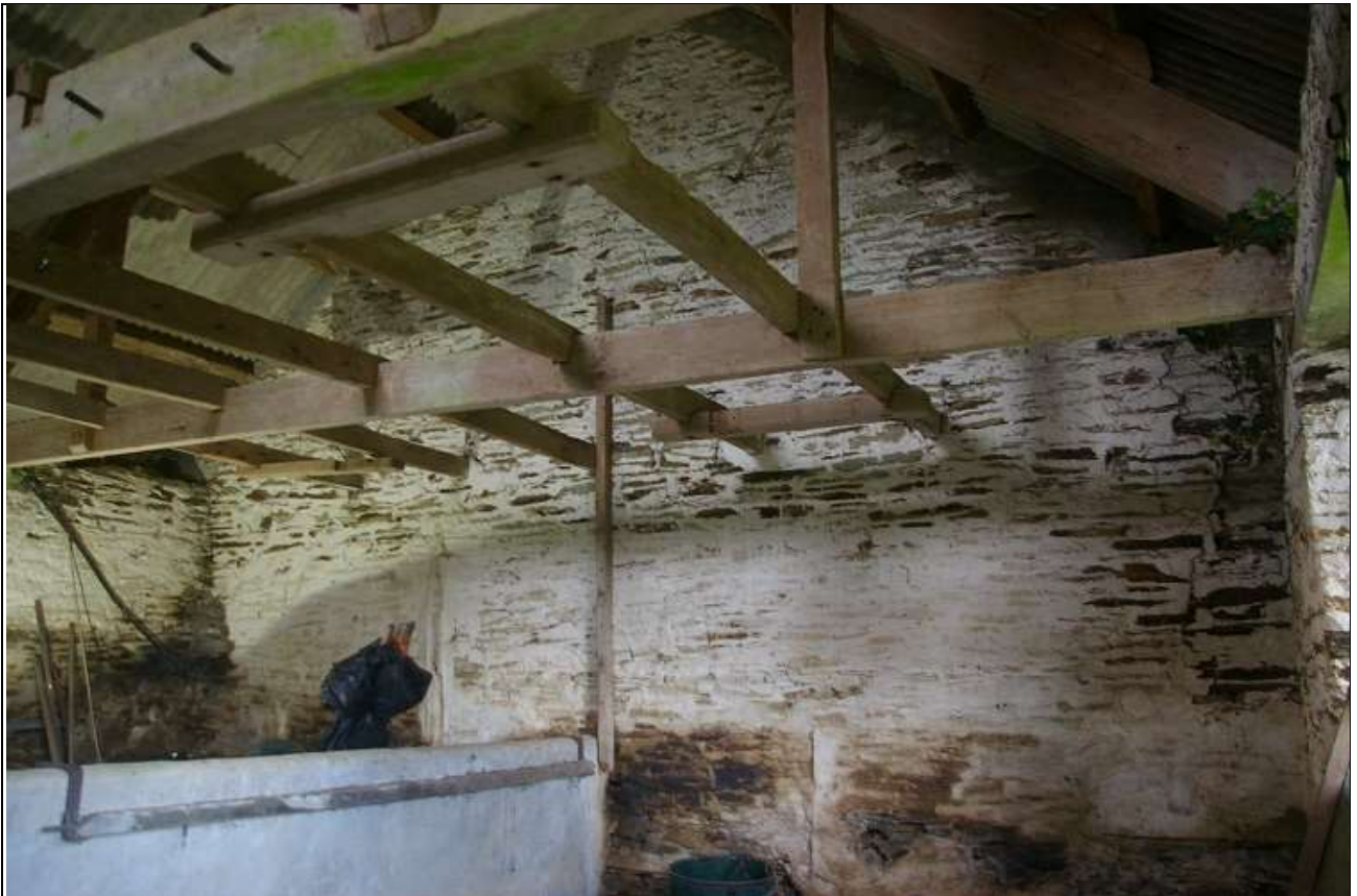
89. THE INTERIOR OF THE WEST WALL OF THE STABLES; FROM THE NORTH-EAST.
