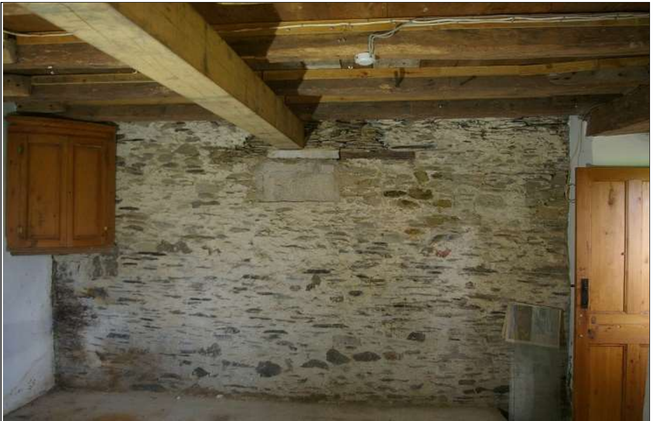
22. THE THICK STONE PARTITION WALL BETWEEN R5 AND R6 IN THE WEST WING; FROM THE SOUTH.
