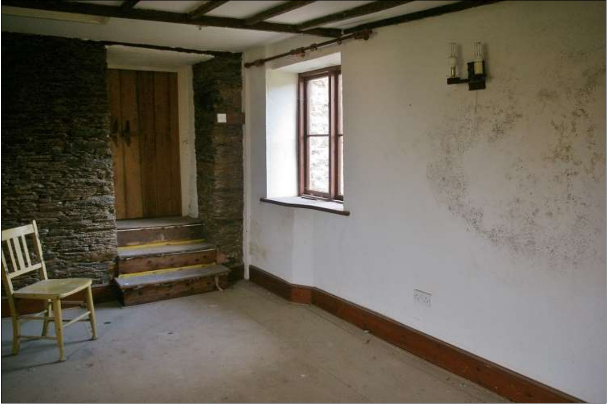
66. VIEW OF WEST WALL OF R19, SHOWING THICK SURVIVING STUD OF EARLIER WALL OF FORMER STAIR TURRET AND OPENING INTO MAIN RANGE, OVER THE FORMER HALL; FROM THE NORTH-EAST.
