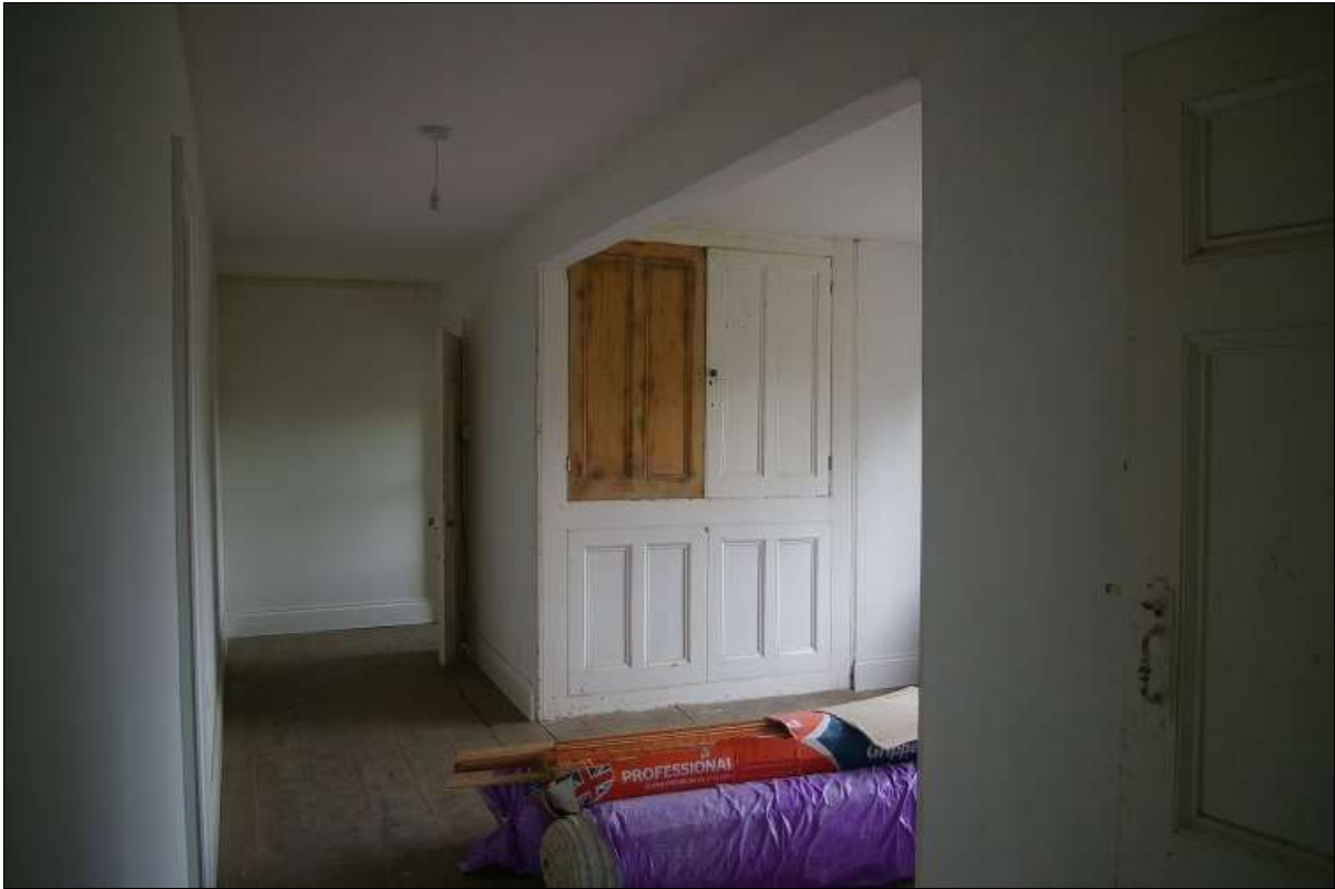
46. R10, THE LANDING WHICH LINKS THE EAST AND WEST WINGS AND REAR WING, CORRIDOR FORMED FROM LATH AND PLASTER PARTITIONS; FROM THE WEST-NORTH-WEST.
