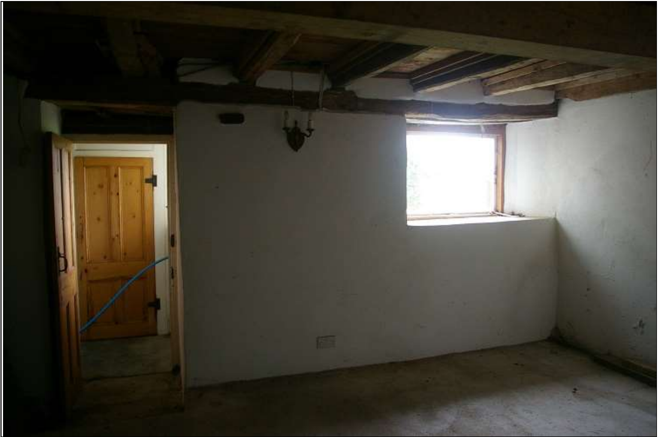
21. R5, THE DOOR TO R2A, WITH LOBBY AND SECOND UNDER STAIR CUPBOARD VISIBLE THROUGH THE DOOR, THE LONG BEAM IN THE EAST WALL OF THE WEST WING; FROM THE WEST-NORTH-WEST.
