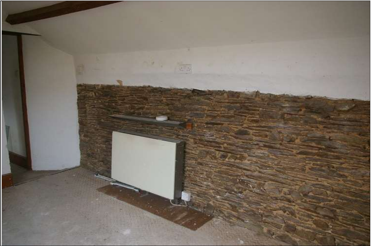
68. EXPOSED STONE OF THE WEST WALL OF R20, SHOWING SMALL SLIT VENT AT SOUTH END; FROM THE NORTH-EAST.
