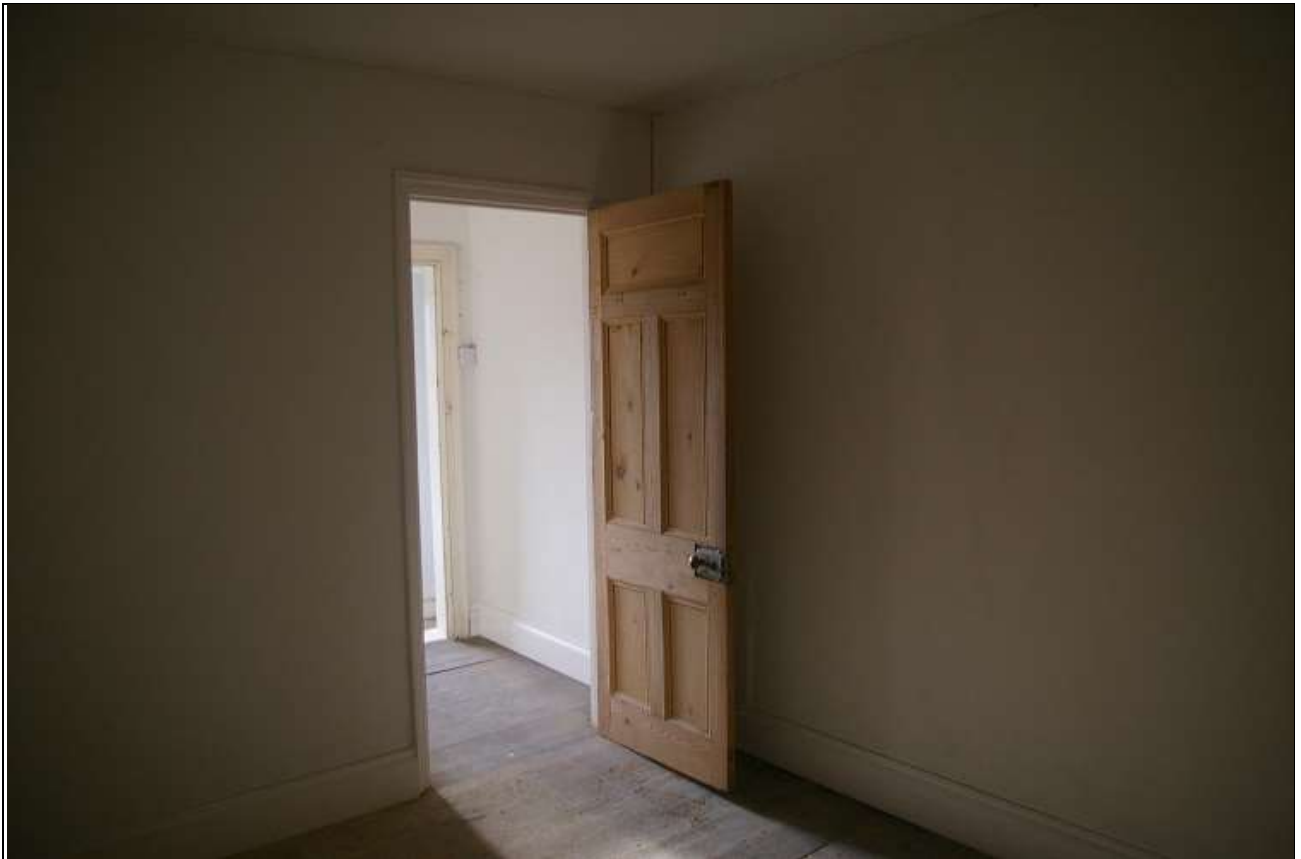
61. R17, A WINDOW LESS ROOM FORMED OVER THE WEST END OF THE HALL; FROM THE NORTH-EAST.
