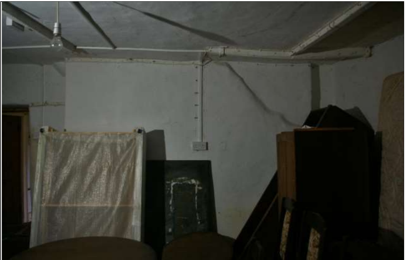
24. THE STACK IN R6, ALSO BEAMS AND TIMBERS WITH HOOKS AND LOOPS AT THE CEILING; FROM THE WEST.
