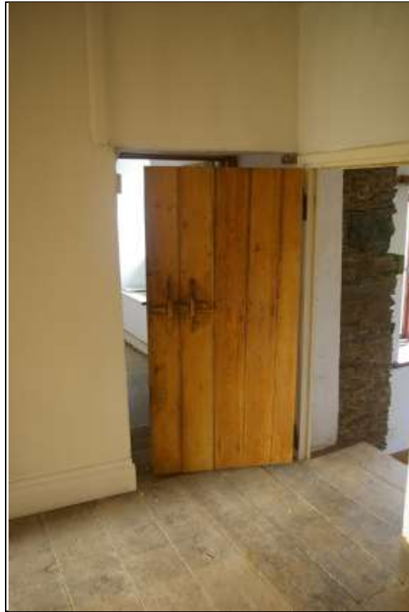
62. R17, FORCED OPENING IN WALL OF WEST WING TO R18 AND GOOD PLANK DOOR IN SMALL OPENING TO REAR SERVICE WING, THE SMALL LOW DOORWAY AND STEPS PART OF AN ORIGINAL STAIR TURRET; FROM THE SOUTH-EAST.
