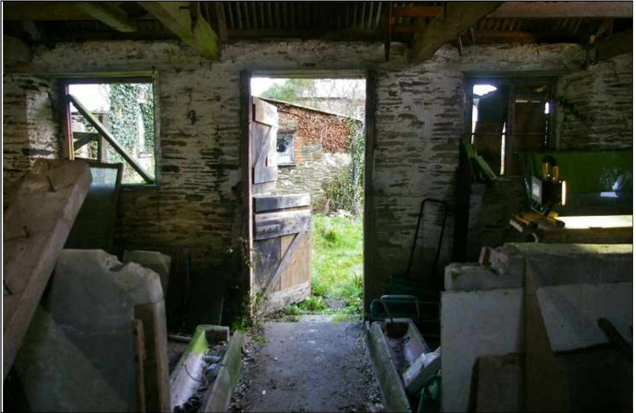
90. THE INTERIOR FACE OF THE NORTH WALL OF THE STABLES; FROM THE SOUTH.
