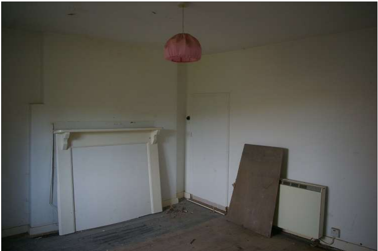
63. R18, WITH STACK WITH FIREPLACE AND BLOCKED DOOR TO THE LOBBY, R14; FROM THE NORTH-WEST.
