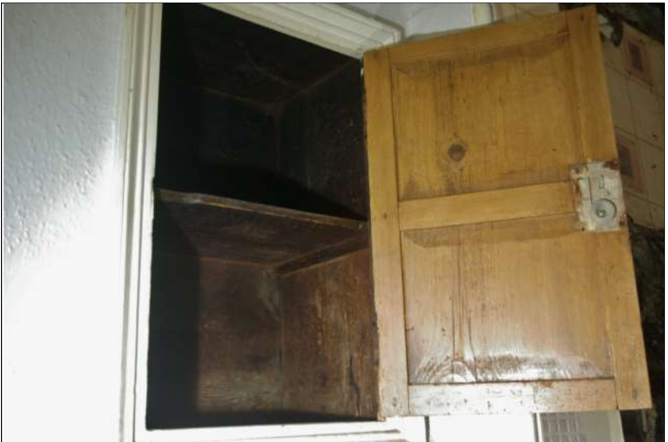
6. THE INTERIOR OF ONE OF THE CUPBOARDS IN THE KITCHEN, LINED IN WOOD, WITH FINE PANELLED DOORS; FROM THE SOUTH-EAST.
