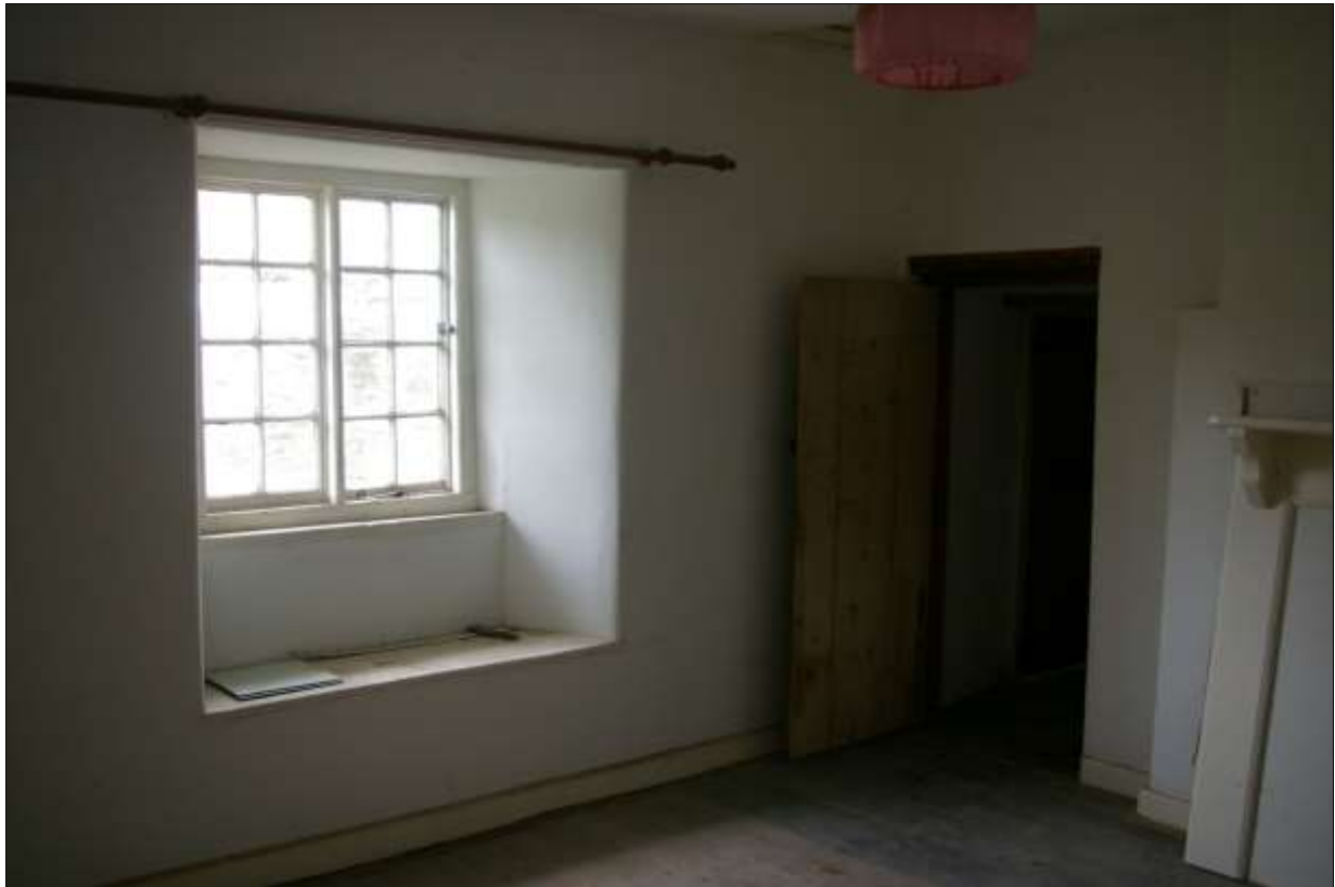
FIGURE 17: ROOM 18, WITH GOOD DOOR AND WINDOW, WITH WINDOW SEAT; FROM THE SOUTH-WEST.
