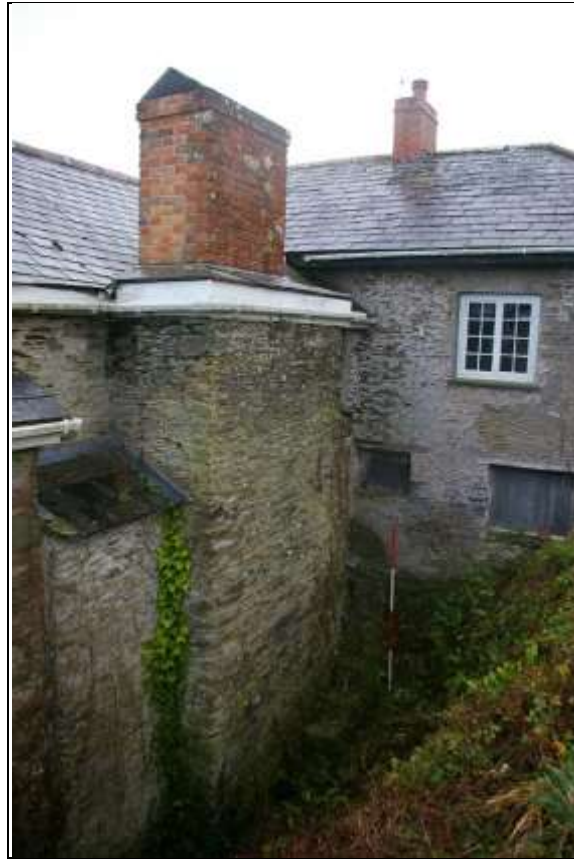
70. DETAIL OF THE STACK TO THE WEST WALL OF THE REAR SERVICE WING, WITH 2M SCALE; FROM THE NORTH-WEST.
