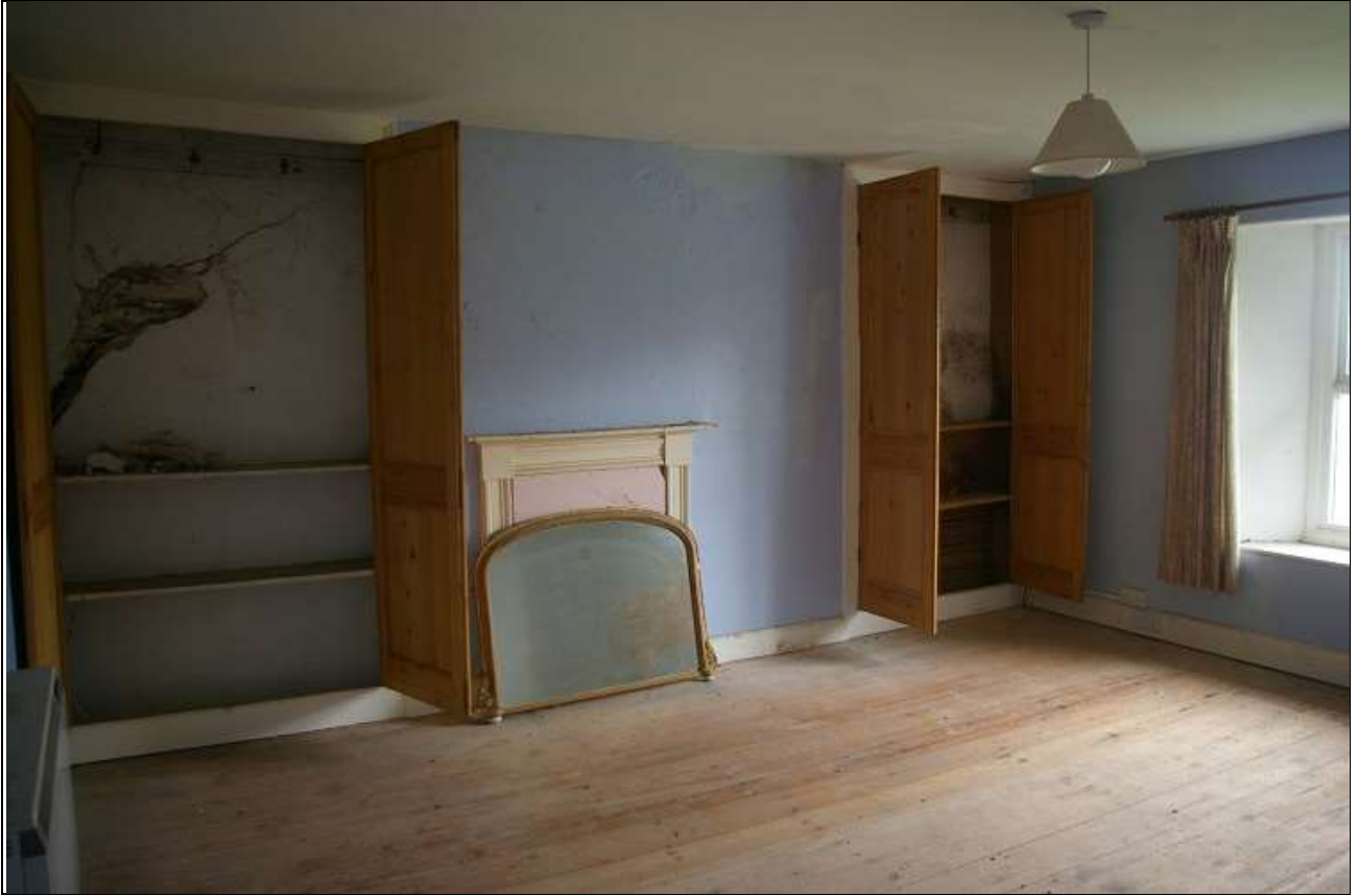
38. THE PAIR OF SHALLOW SHELVED CUPBOARDS IN R11, WITH BLOCKED FIREPLACE WITH MANTLED SURROUND; FROM THE NORTH-WEST.
