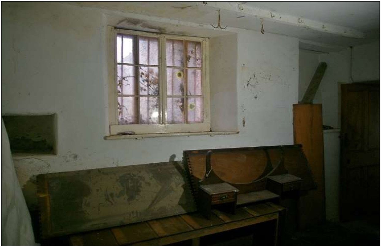
FIGURE 14: THE NORTH WALL OF ROOM 6, WHICH CONTAINS THE MAJORITY OF PRE-1800 FEATURES IN THE STANDING BUILDING; FROM THE SOUTH-WEST.
