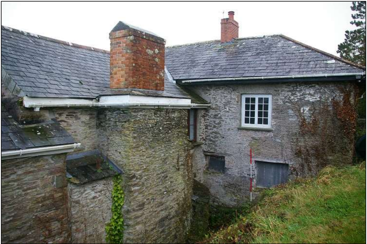
FIGURE 8: THE WEST END OF THE MAIN RANGE, WITH 2M SCALE; FROM THE NORTH-WEST.
