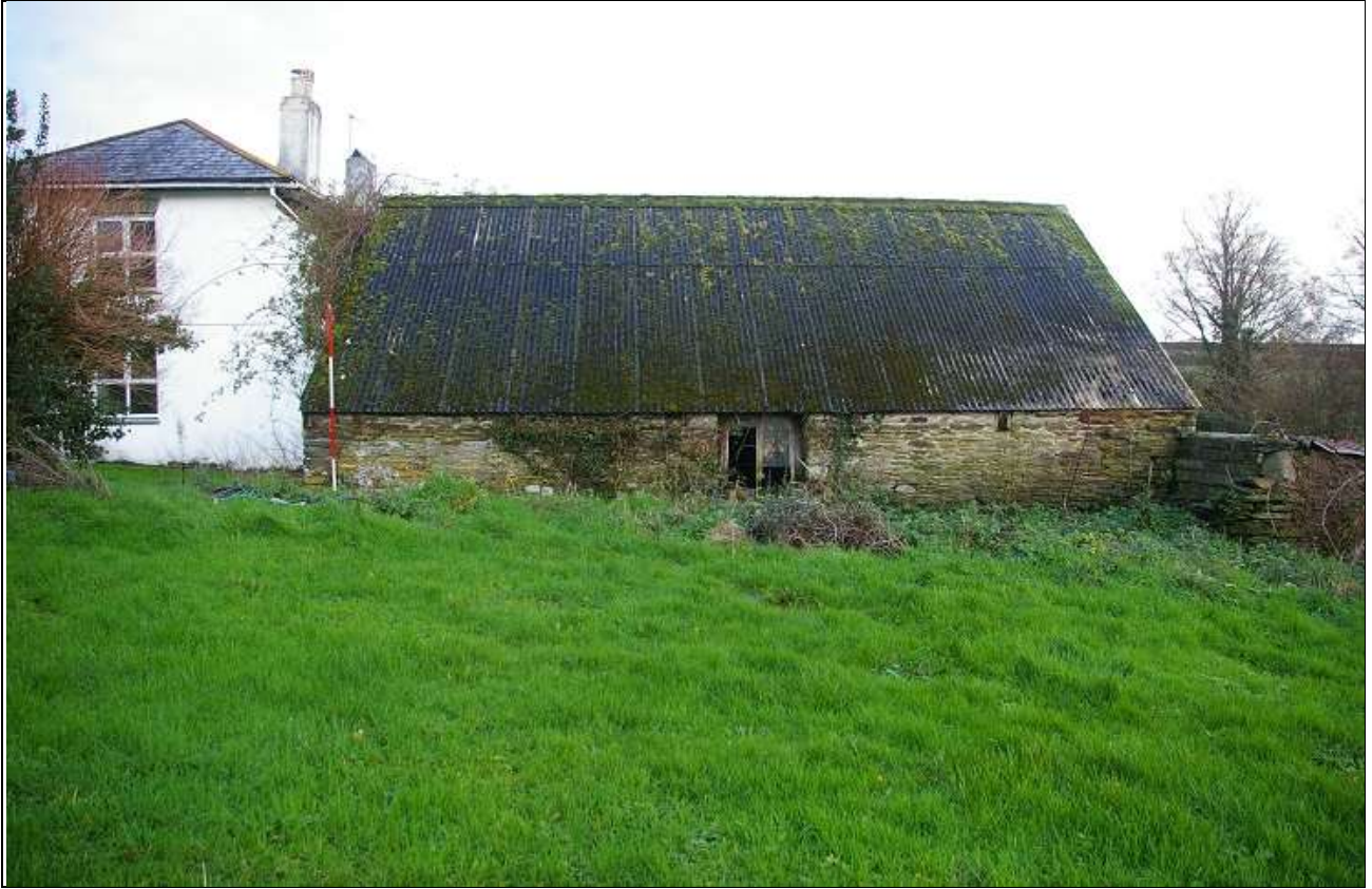
88. THE SOUTH WALL OF THE STABLES BUILT INTO AND ONTO THE SLOPING GROUND, WITH 2M SCALE; FROM THE SOUTH.
