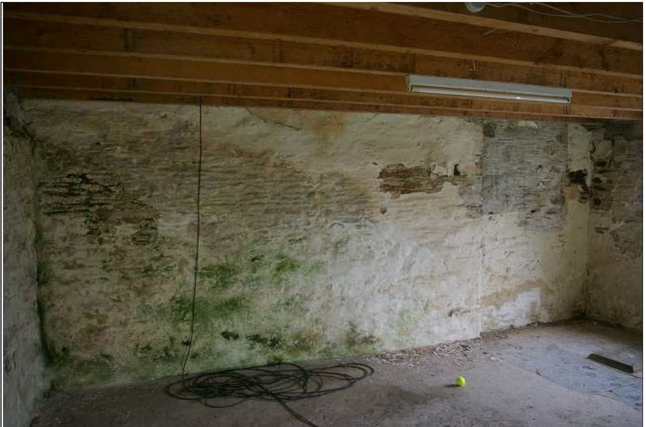
31. R8, AN SEMI AGRICULTURAL SPACE ADDED ONTO THE KITCHEN BLOCK, NORTH WALL, CLEARLY EXTENDED TO THE EAST; FROM THE SOUTH-WEST.
