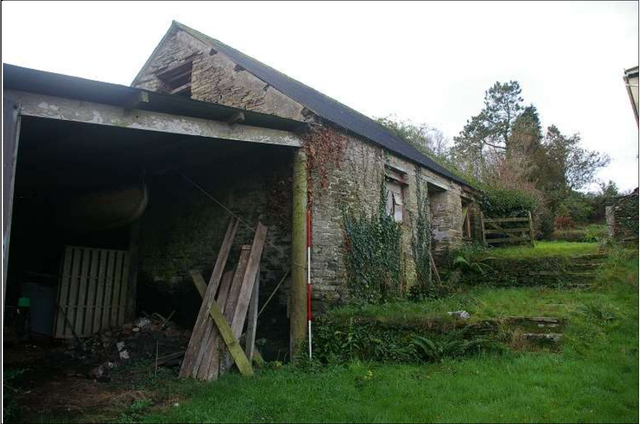
86. THE NORTH AND WEST WALLS OF THE STABLES, AS SEEN ABUTTED BY A TIMBER FRAMED CORRUGATED SHEETING LEAN-TO, WITH 2M SCALE; FROM THE NORTH-EAST.
