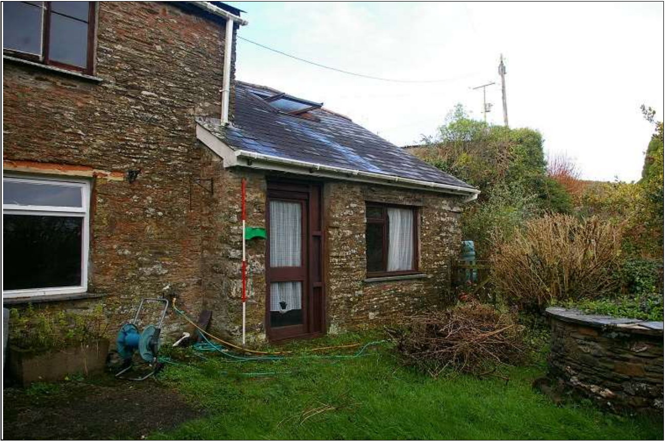
78. THE SINGLE STOREY BLOCK EXTENSION TO THE REAR SERVICE WING, WITH 2M SCALE; FROM THE SOUTH-EAST.
