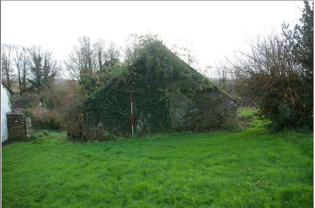
87. THE WEST WALL OF THE STABLES, AS BUILT INTO AND ONTO THE BANK WITH A GABLE, 2M SCALE; FROM THE WEST.
