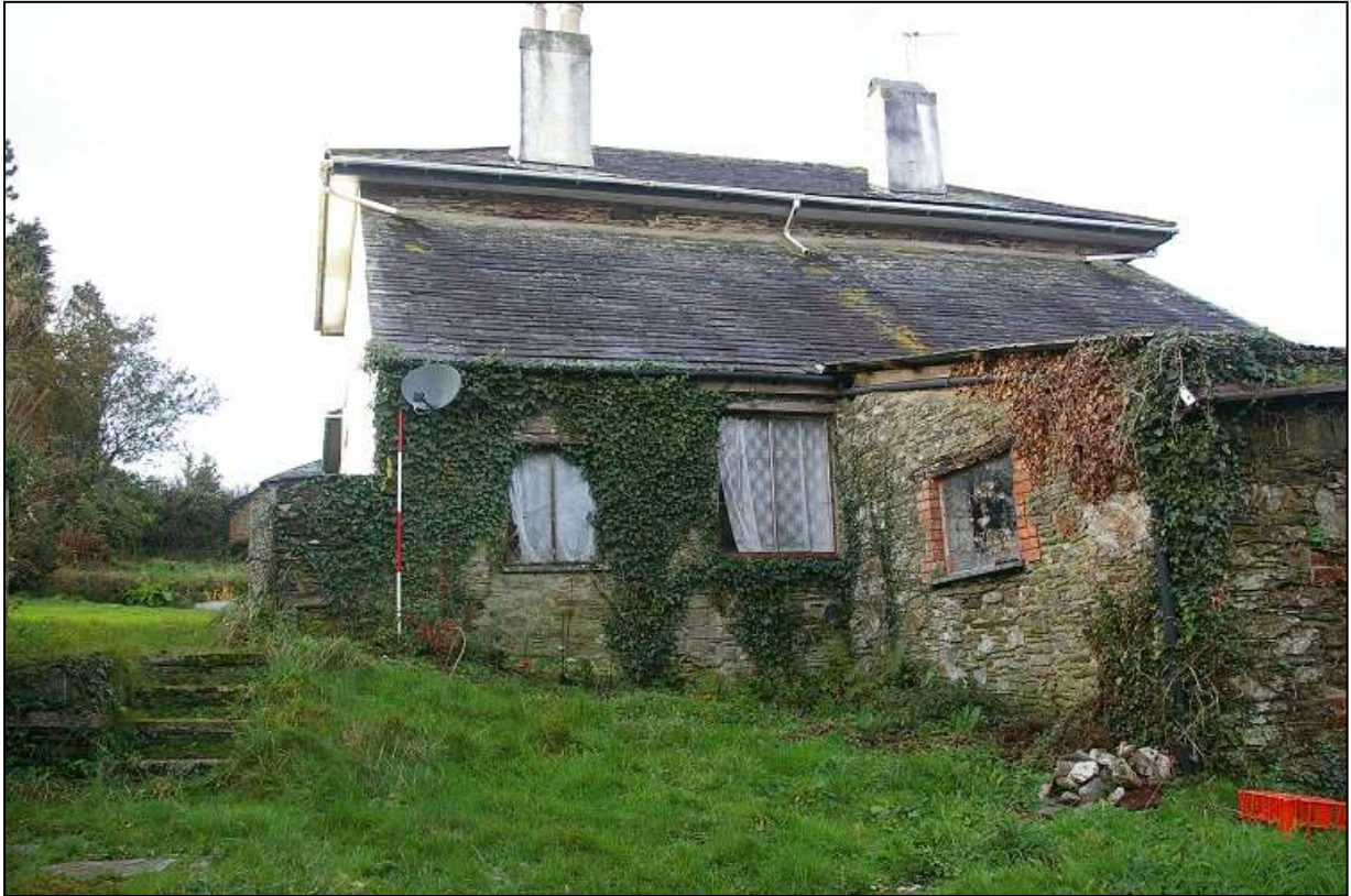
FIGURE 22: THE STONE RUBBLE OUTBUILDINGS ON THE EAST FLANK OF TREVEDDA, WITH 2M SCALE; FROM THE EAST-SOUTH-EAST.
