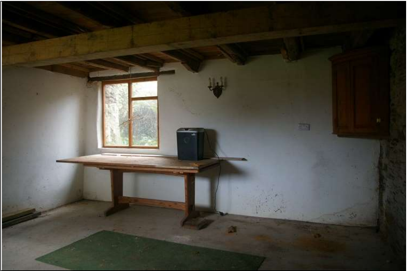
20. R5, A SPACE WITH BOTH A SERVICE AND AGRICULTURAL FUNCTION, WITHIN THE EXTENDED CROSS-WING TO THE WEST; FROM THE EAST-NORTH-EAST.
