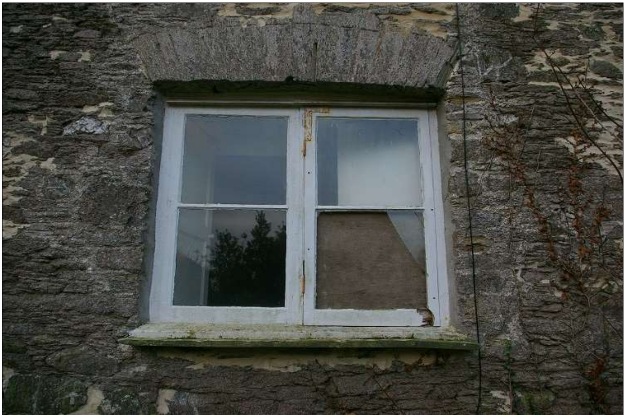
75. W10 ON THE NORTH WALL OF TREVEDDA AN EXAMPLE OF ONE OF THE GOOD SET OF THREE 19 TH CENTURY WINDOWS; FROM THE NORTH.
