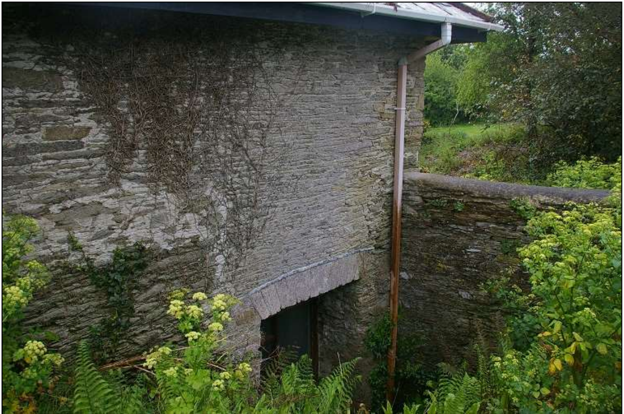
FIGURE 9: THE SOUTH END OF THE WEST ELEVATION, SHOWING THE TERMINUS OF THE OLDER STONEMWORK AND THE DOORWAY FORMED IN THE EXTENDED SOUTH END BLOCKED BY RAISED GROUND LEVELS; FROM THE NORTH-NORTH-WEST.
