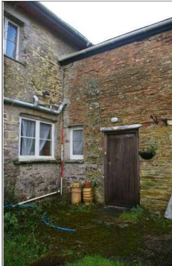
77. THE JOINT BETWEEN THE MAIN RANGE AND SERVICE WING, WITH 2M SCALE; FROM THE NORTH-EAST.
