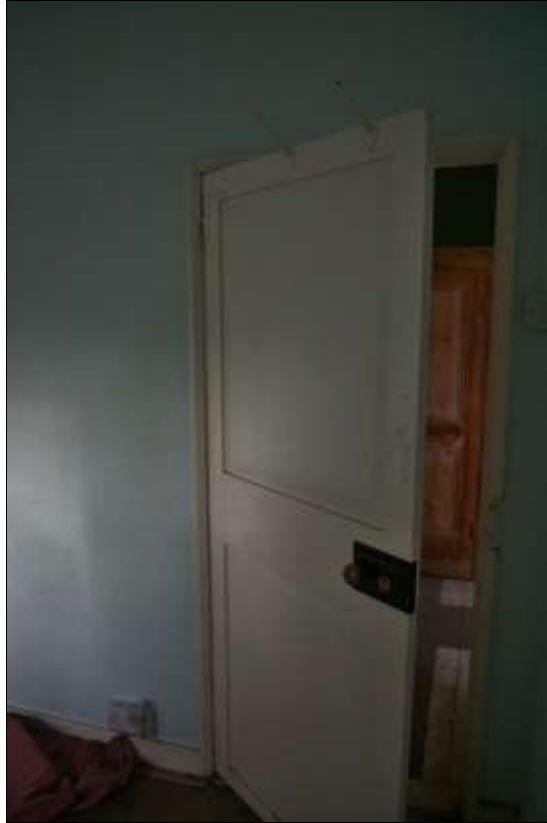
54. THE GOOD LATER 17 TH OR EARLY 1700S TWO PANEL DOOR IN R15, GOOD L-H HINGES, BUT LIKELY RESET WITHIN THE BUILDING, ON A THIN BEADED FRAME; FROM THE SOUTH.
