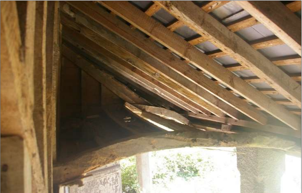
31. THE ARCHED CEILING, MATCHING THAT IN ELEMENTS A, INSERTED INTO THE EARLIER WAREHOUSE STYLE SPACE; FROM THE WEST-NORTH-WEST.
