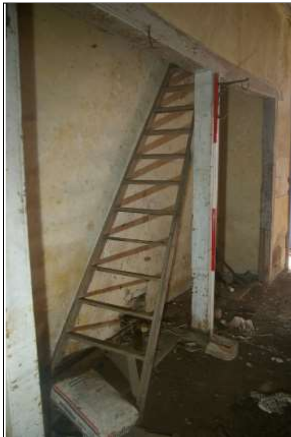
16. THE GOOD TAPERED LADDER, REUSED HERE FROM ELEMENT B; WITH 2M SCALE, SHOWING POSTS AND SADDLE TREES, FROM THE NORTH-NORTH-WEST.
