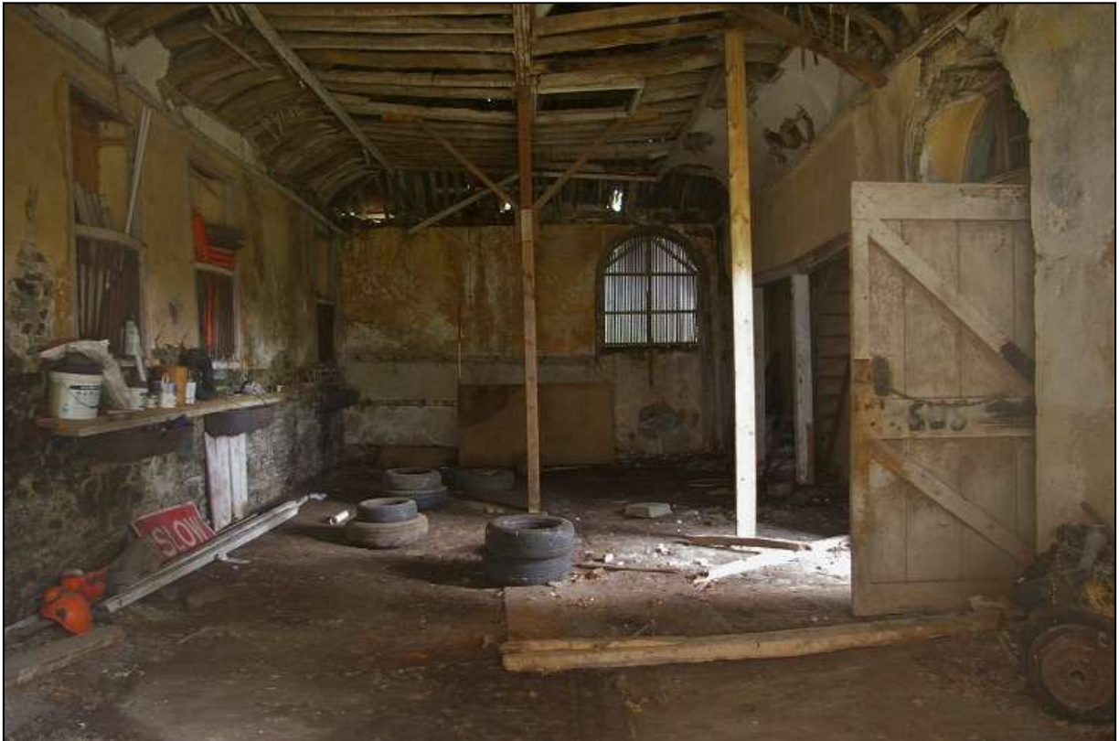
FIGURE 7: THE STABLES RANGE, WITH DRAMATIC VAULTED CEILING; FROM THE SOUTH, WITH 2M SCALE.
