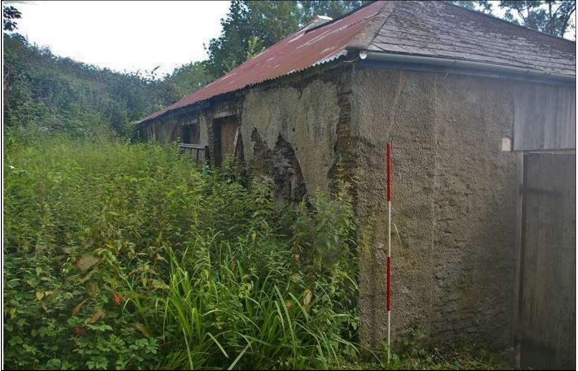
5. THE SOUTH AND WEST ELEVATIONS OF ELEMENT A, WITH 2M SCALE; FROM THE SOUTH-WEST.
