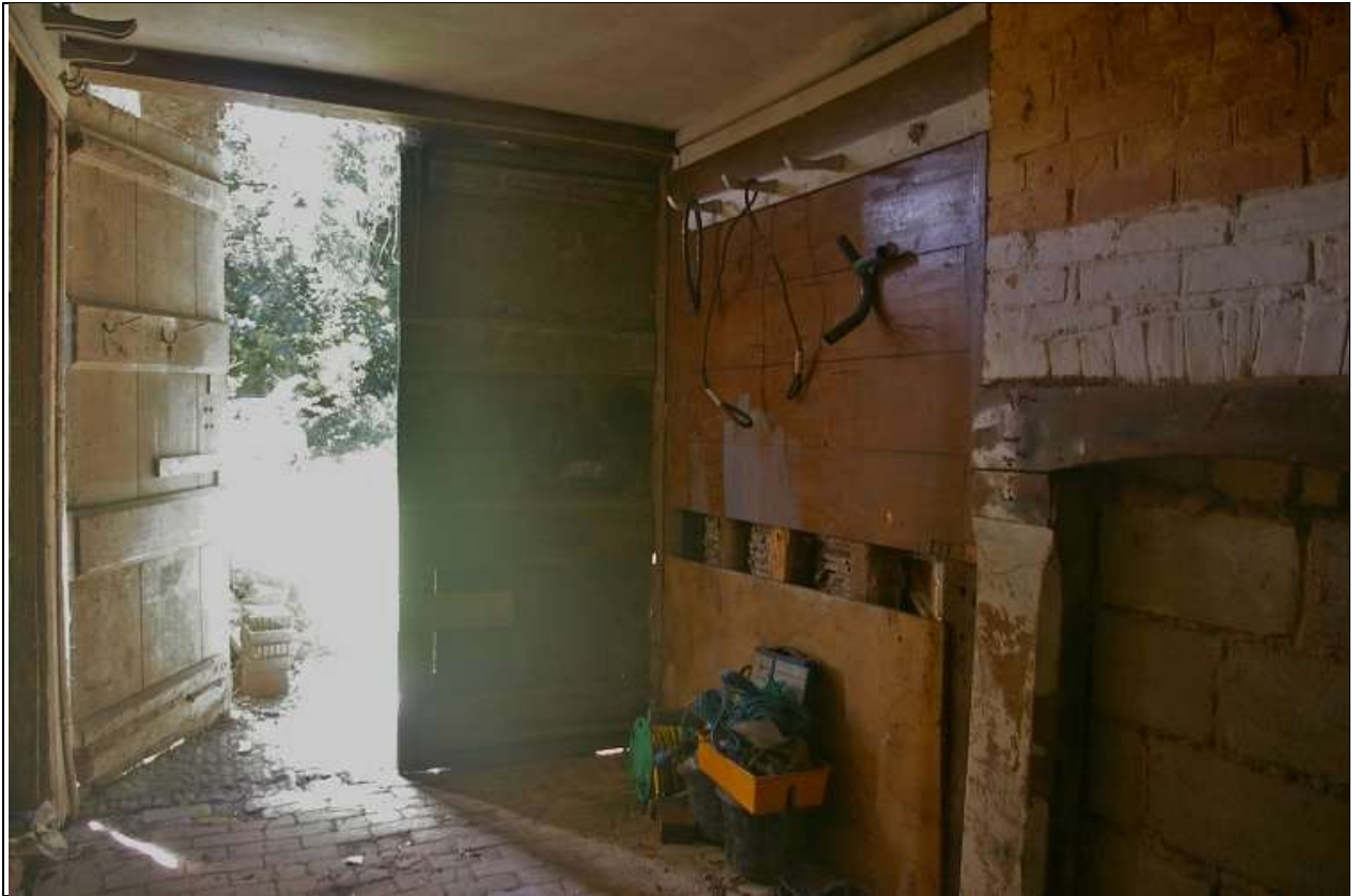
27. THE WEST PARTITION WALL, WITH ROOM 3, SHOWING BOARDING AND FRAMING AND BRICK STACK; FROM THE NORTH-EAST.
