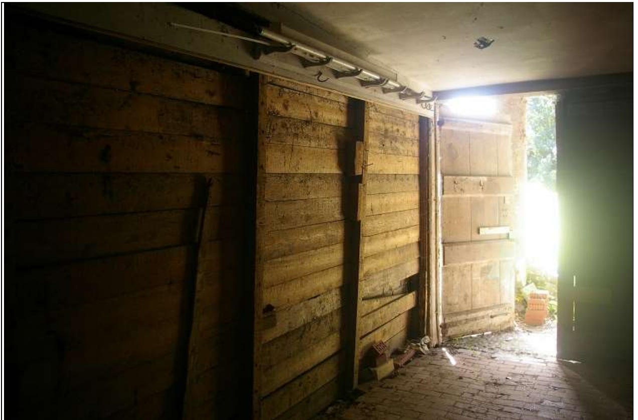
28. THE EAST BOARDED WALL OF THE ELEMENT B, ROOM 3, WHERE THE BUILDING HAS BEEN TRUNCATED; FROM THE NORTH-WEST.
