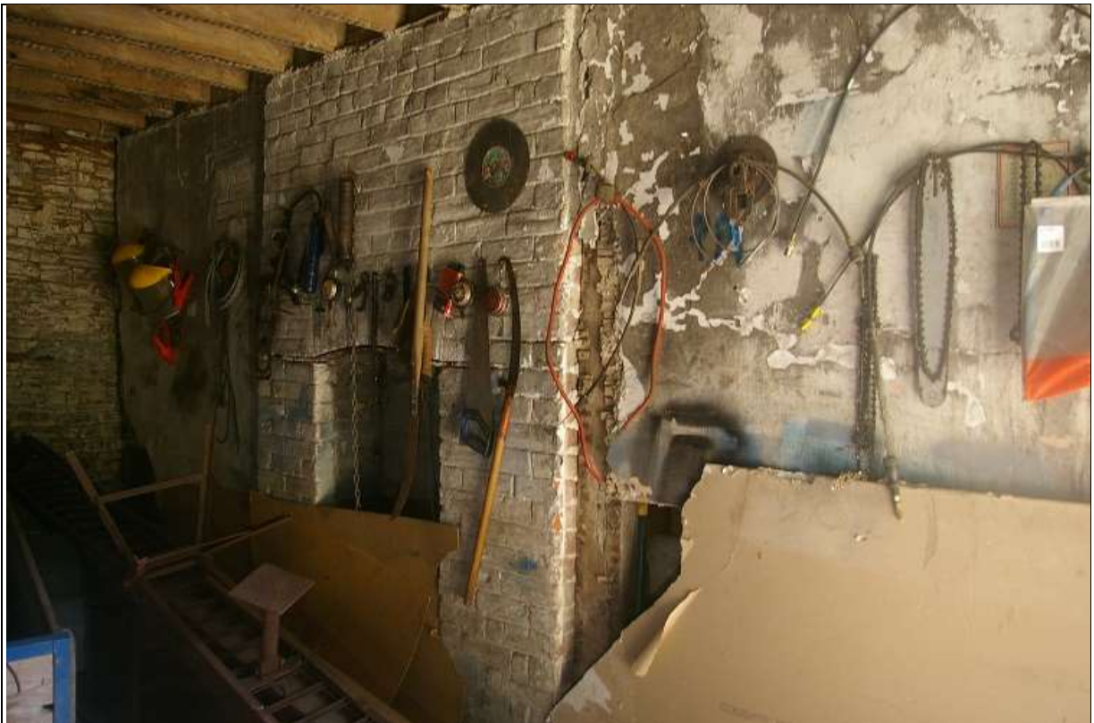
24. THE EAST WALL PARTITION BETWEEN ROOMS 2 AND 3 OF ELEMENT B, WITH INSERTED STACK IN BRICK; FROM THE SOUTH-SOUTH-WEST.
