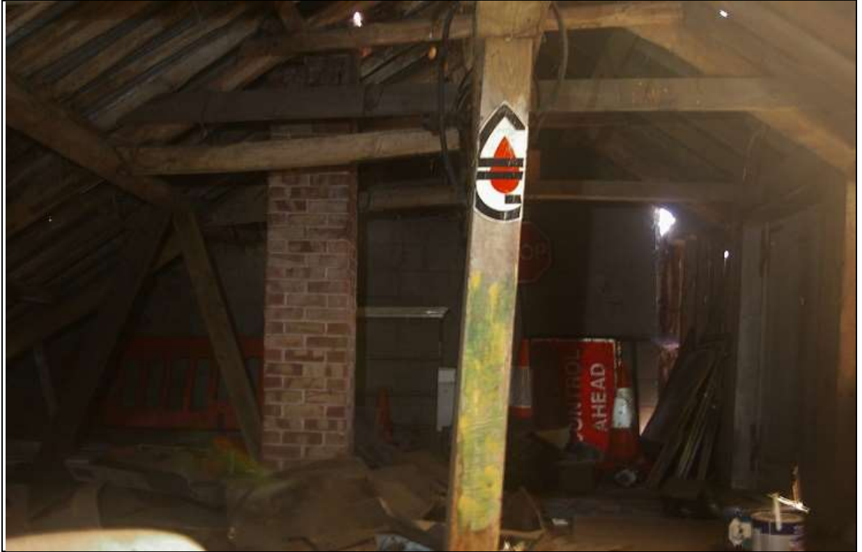
29. THE LOFT ABOVE ELEMENT B, WITH INSERTED BRICK STACK; FROM THE WEST.
