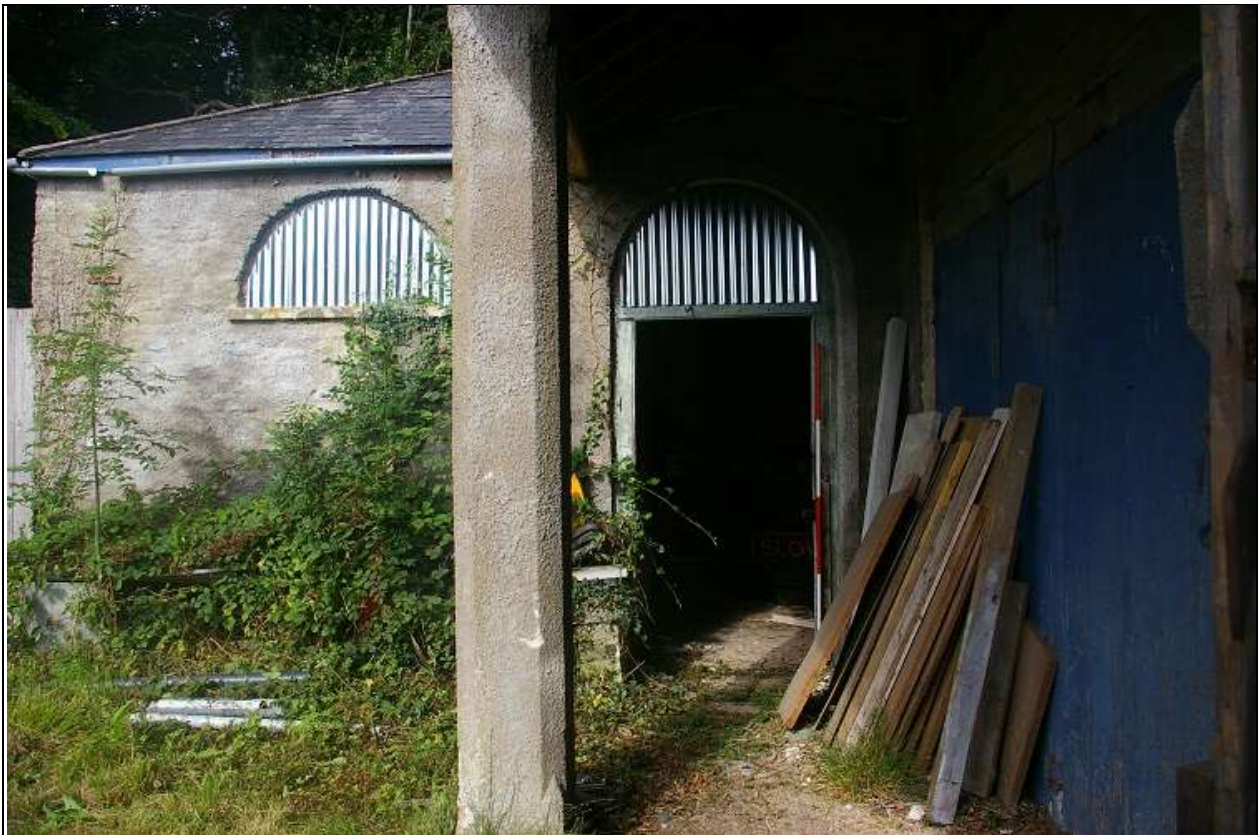
4. THE EAST ELEVATION OF ELEMENT A, FROM WITHIN THE VERANDAH OF ELEMENT B, WITH 2M SCALE; FROM THE EAST.
