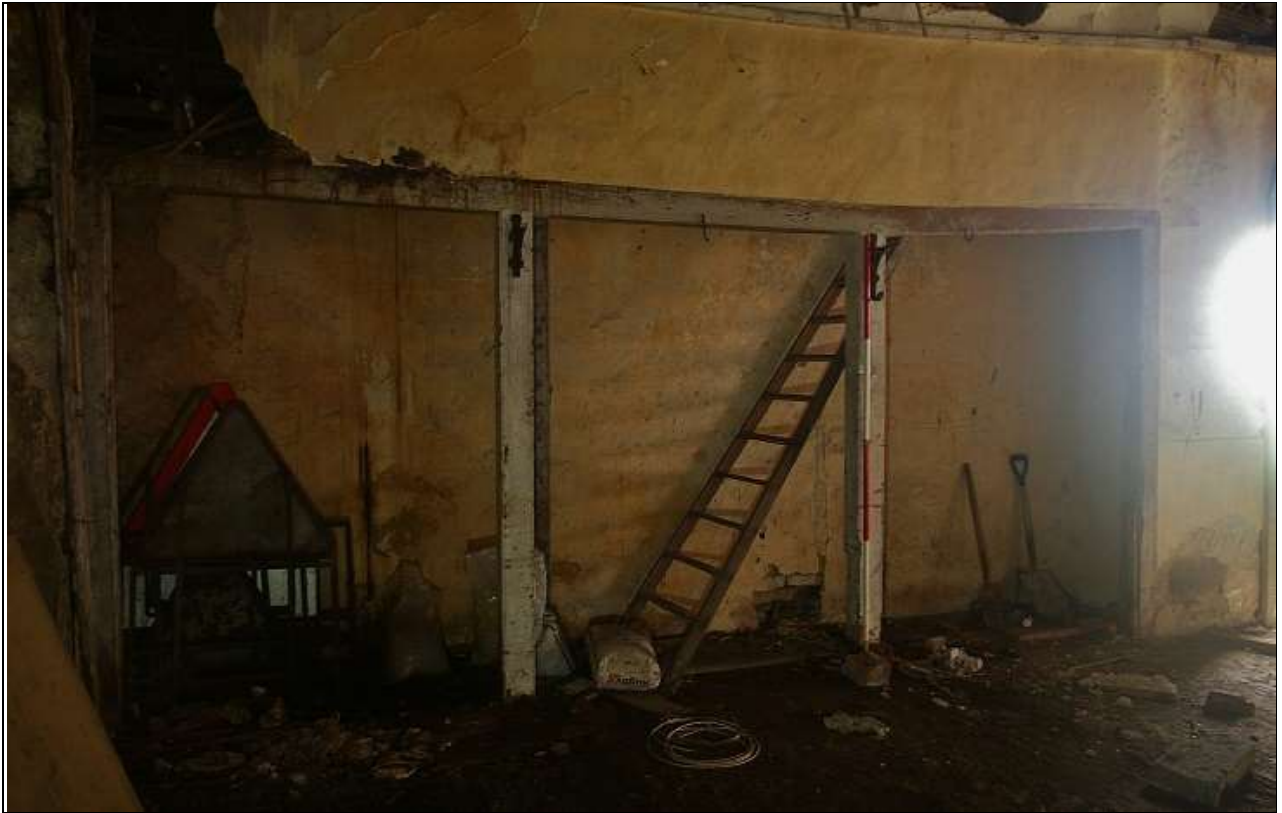
15. THE NORTH END OF THE EAST WALL OF ELEMENT A, THE PARTITION WALL, INSERTED TO DIVIDE THE RANGE, WITH 2M SCALE; FROM THE NORTH-WEST.
