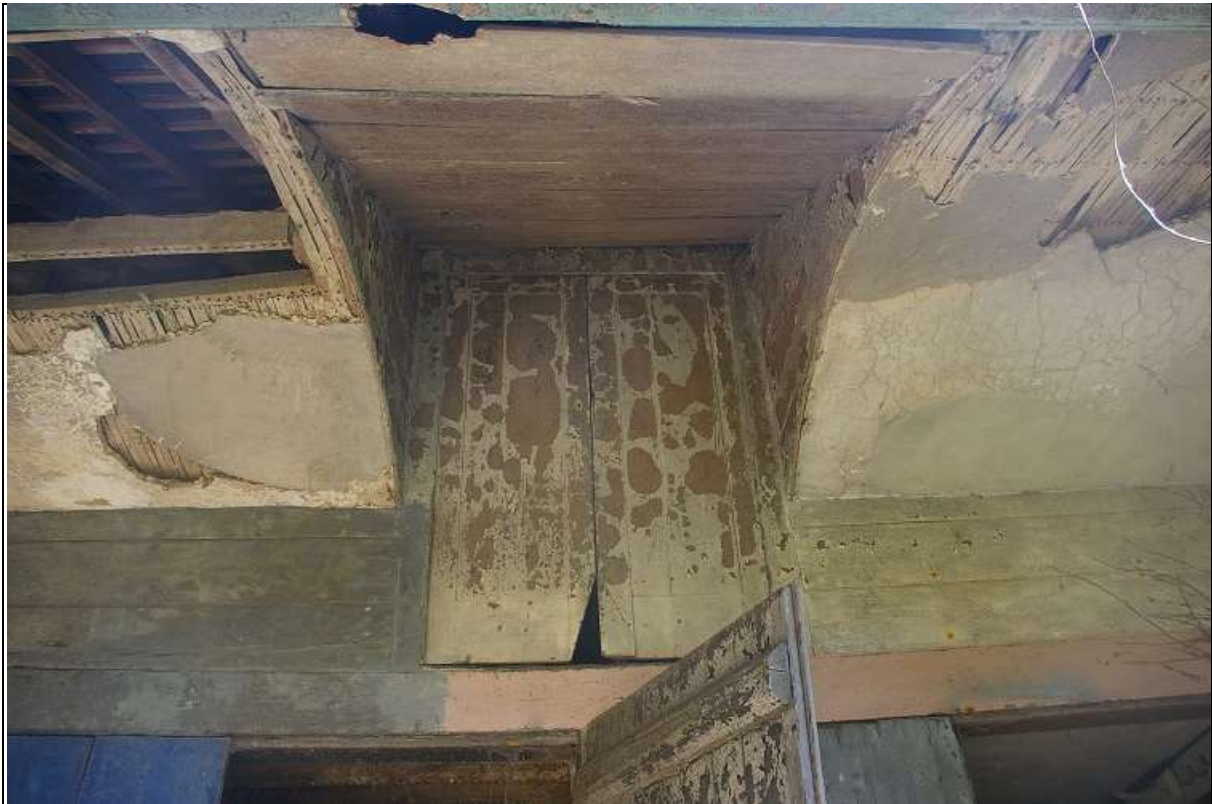
22. THE DOUBLE DOORS SET WITHIN THE LOADING DOOR, ABUTTED BY THE ARCHED INSERTED CEILING; FROM THE SOUTH.
