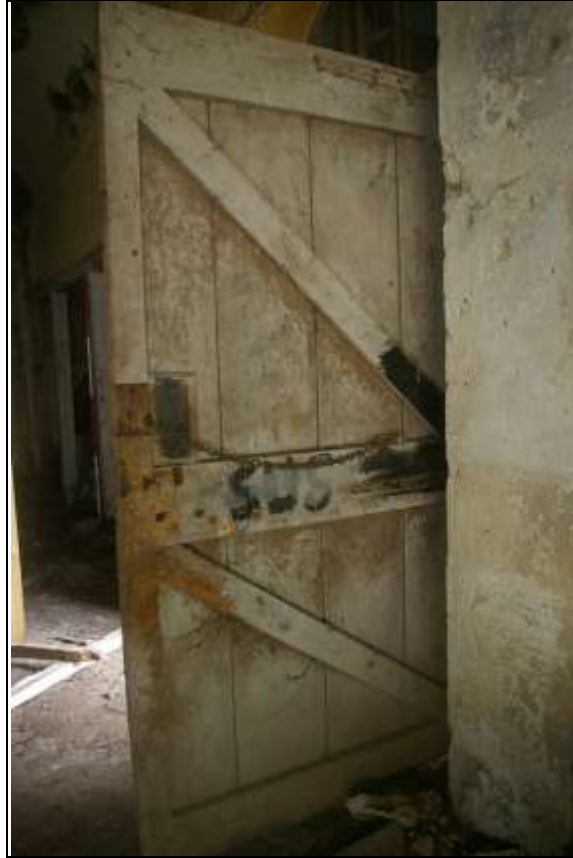
17. THE MASSIVE DOOR TO THE STABLES, IN THE EAST WALL; FROM THE SOUTH-WEST.
