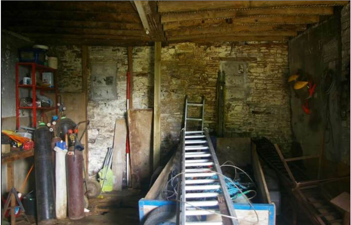
FIGURE 8: THE REAR NORTH WALL OF ROOM 2, IN ELEMENT B, SHOWING THE SERIES OF BLOCKED OPENINGS, WITH 2M SCALE; FROM THE SOUTH.
