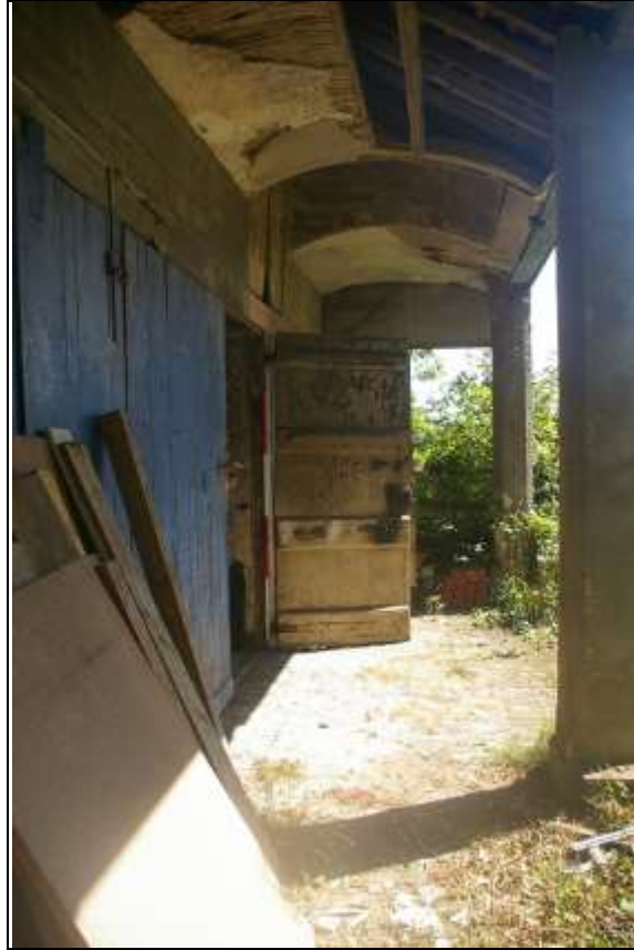
19. ELEMENT B, THE DOORS, THE ARCHED CEILING AND POSTS OF THE VERANDAH, WITH 2M SCALE; FROM THE WEST.
