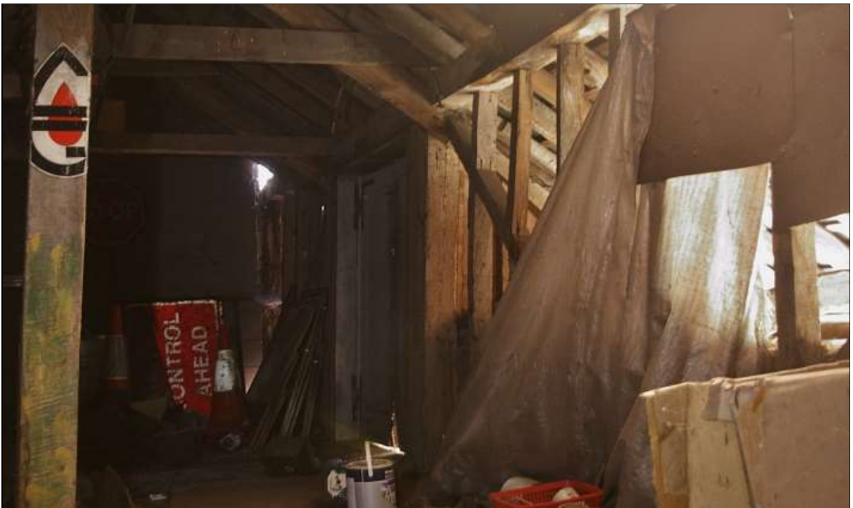
30. THE HEAVY FRAMED TIMBER FRONT WALL OF ELEMENT B, SHOWING LOADING DOOR; FORM THE WEST-NORTH-WEST.
