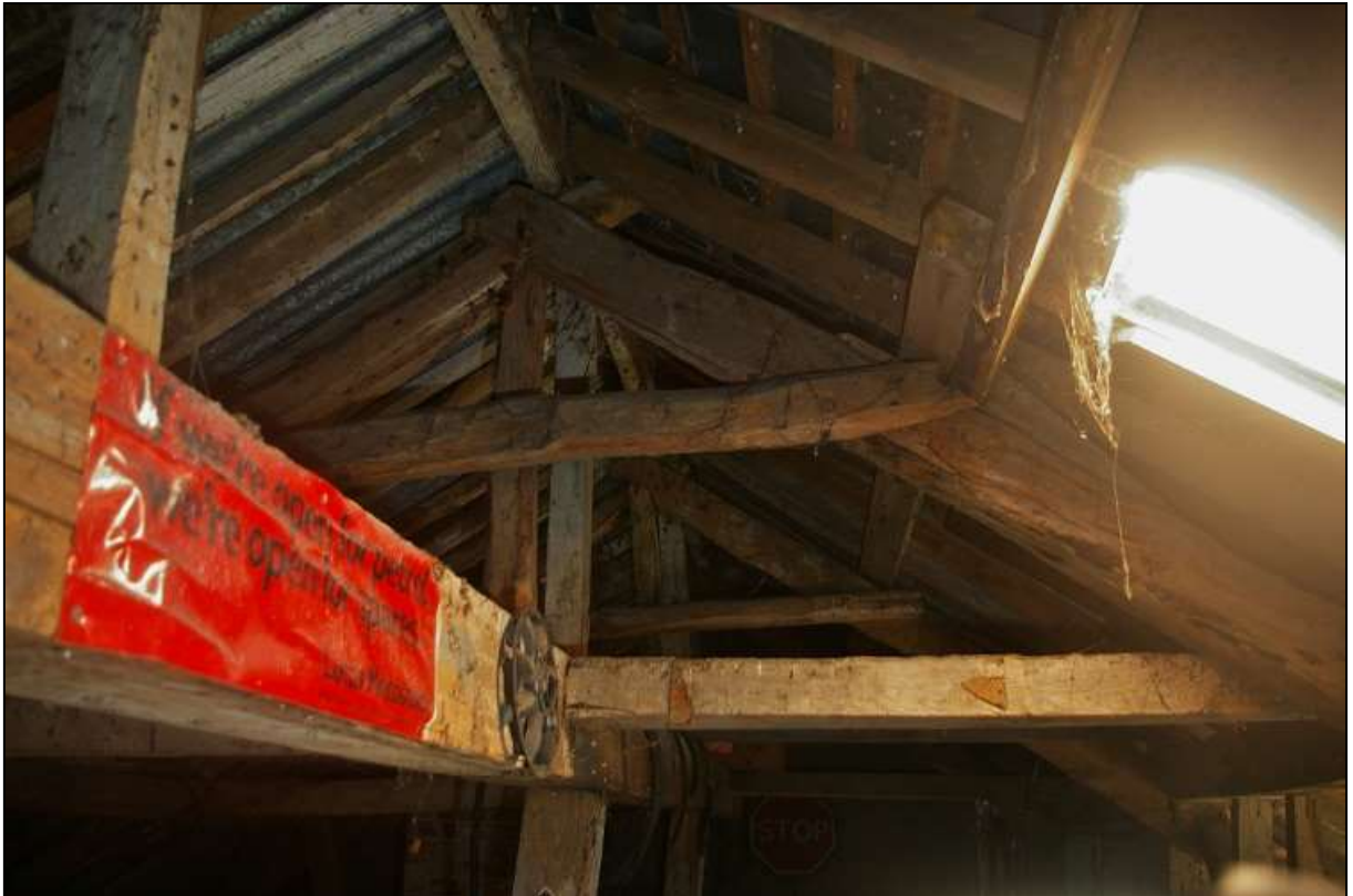
FIGURE 9: THE ROOF ABOVE ELEMENT B, THE LOFT, WITH MASSIVE FRAMEWORK AND RUSTIC POOR QUALITY A-FRAMES ABOVE, TO A CHANGE ROOFLINE; FROM THE WEST.
