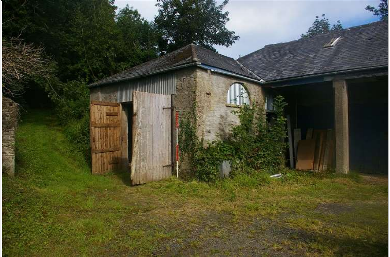
3. ELEMENT A, THE STABLES, SOUTH AND EAST ELEVATIONS, WITH 2M SCALE; FROM THE SOUTH-EAST.
