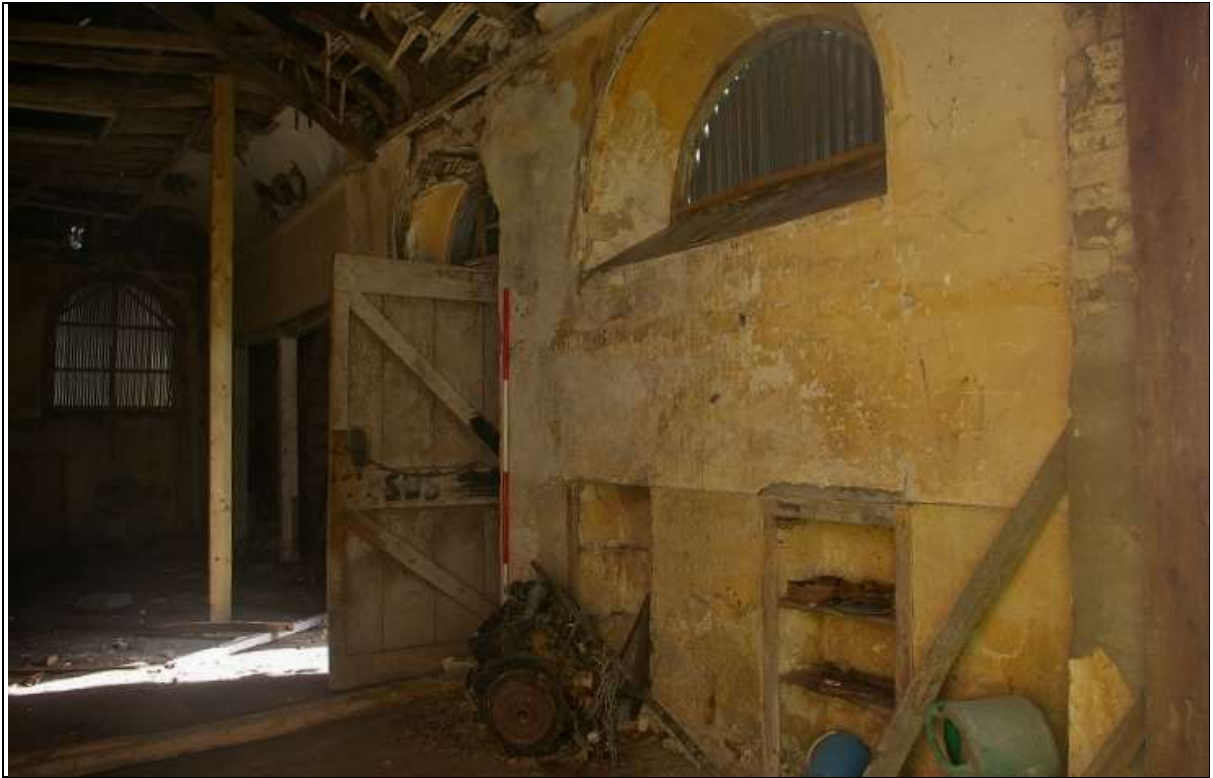
FIGURE 6: THE EAST WALL OF THE STABLES RANGE, ELEMENT A, SHOWING THE DOOR, WINDOW AND FRAMED INTERNAL PARTITION TO THE NORTH END; FROM THE SOUTH-SOUTH-WEST, WITH 2M SCALE.
