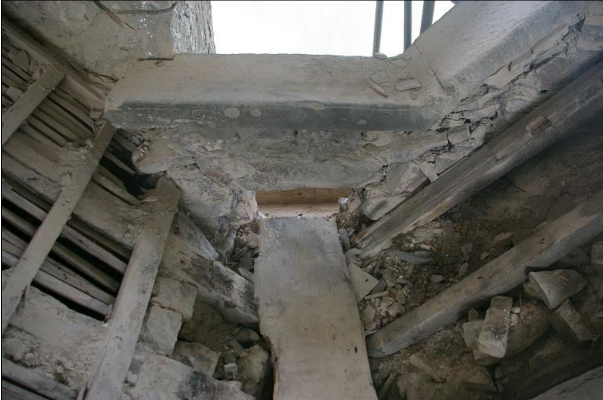
20. THE VALLEY GUTTER AND DRAIN TO THE WEST END; FROM THE EAST.
