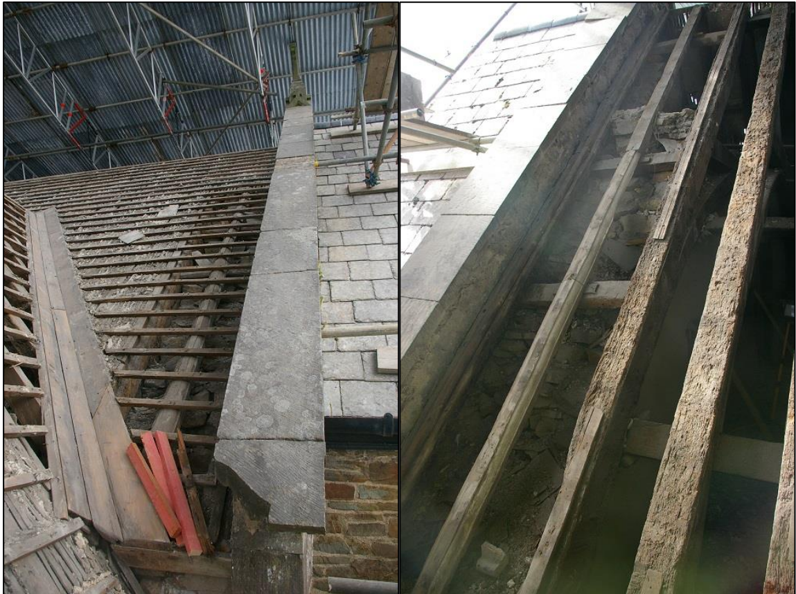
FIGURES 4A & 4B: LEFT; SOUTH SIDE OF THE ROOF, WITH REUSED MOULDED TIMBER. RIGHT, NORTH SIDE OF THE NAVE ROOF, WITH A SIMILAR MOULDED TIMBER, CLEARLY REUSED FROM ELSEWHERE OF TYPICAL 16 TH CENTURY MOULDED FORM.
