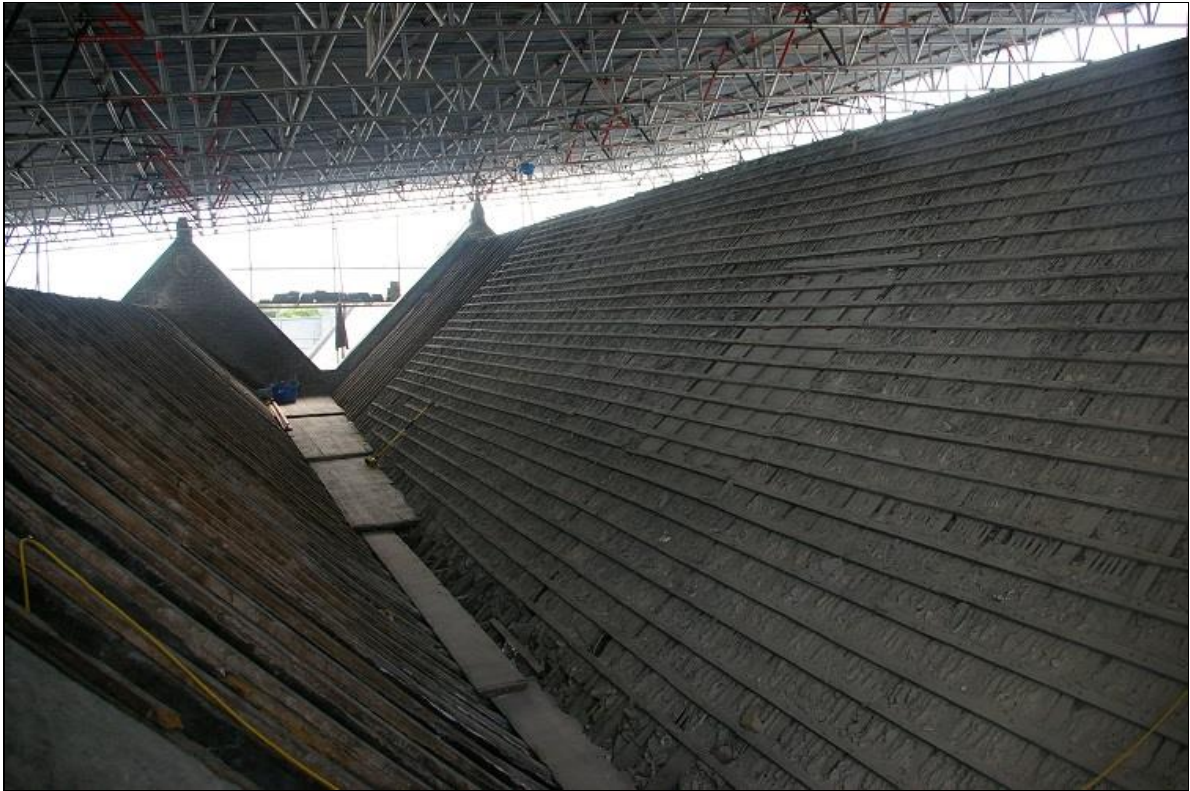
15. THE NORTH AISLE AND NAVE ROOFS STRIPPED OF SLATE; FROM THE WEST-NORTH-WEST.
