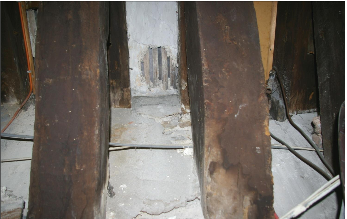
4. THE INTERIOR OF THE NAVE ROOF SHOWING THE LIME PLASTER BETWEEN THE TRUSSES AND VERY THIN LATHS; VIEWED FROM THE SOUTH.
