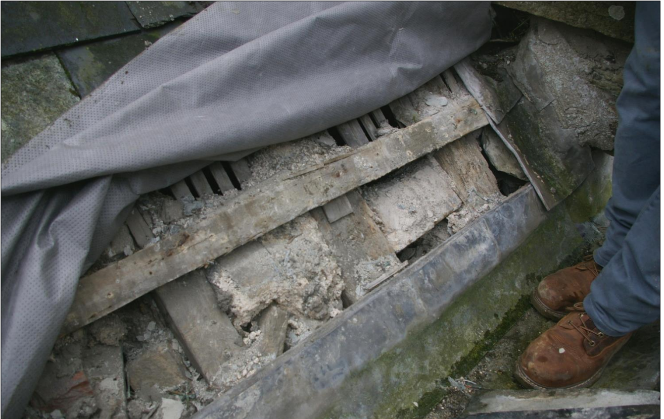
7. EXTERIOR FACE OF THE ROOF WITH SLATES LIFTED AND FELT REMOVED. THERE ARE TWO HEAVY ORIGINAL TRUSS BLADES AND ONE NARROW 19TH CENTURY TRUSS BLADE; VIEWED FROM THE EAST-NORTH-EAST.
