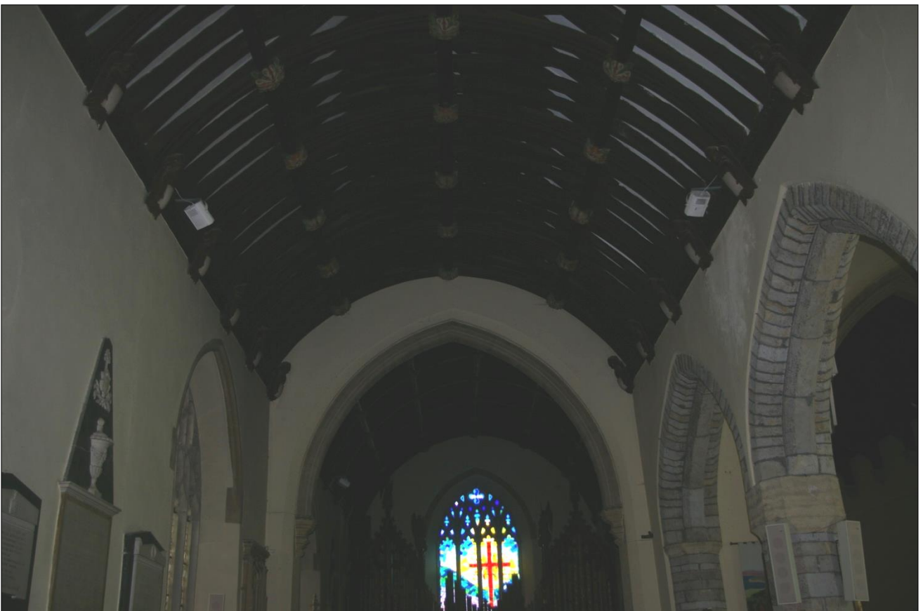
12. VIEW FROM WITHIN THE NORTH AISLE SHOWING THE OFFSET ROOF; VIEWED FROM THE WEST.
