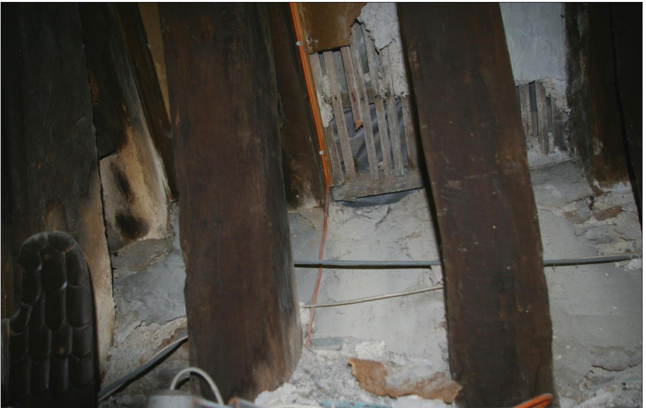
6. THE CEMENT RENDER TREATMENT OF THE WALL TOPS, THE RUBBLE BUILD IN LIME MORTAR BEHIND IT, AND AN ATTEMPT TO COVER THE FAILING LIME PLASTER WITH FIBRE PANELS; VIEWED FROM THE SOUTH-EAST.
