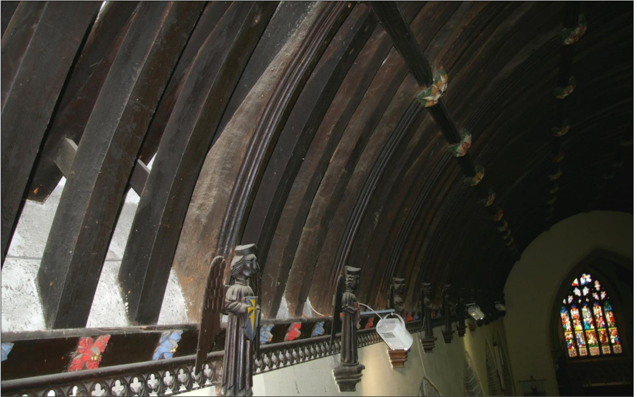
5. THE NORTH SIDE OF THE NAIVE ROOF, CLEARLY SHOWING THE DIFFERENCES IN TEXTURE AND SLIGHT VARIATIONS IN COLOUR, WHERE MEDIEVAL TIMBERS HAVE BEEN INCORPORATED INTO A 19 TH CENTURY ROOF REPAIR; VIEWED FROM THE WEST-SOUTH-WEST.
