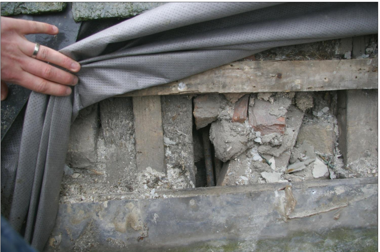
8. MEDIEVAL HEAVY TRUSS BLADE, JUST BEYOND THE LIGHTER 19 TH CENTURY ONE; THIS MEDIEVAL TRUSS HAS HAD A LIGHT PINE BATTEN FOR THE SLATES ATTACHED TO ITS REAR WITH IRON NAILS; VIEWED FROM THE NORTH-NORTH-EAST.
