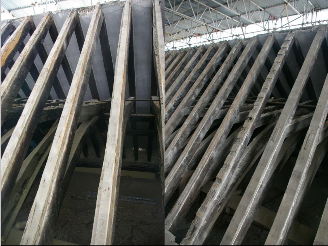
17. LEFT: SAW MARKS ON TRUSSES OF NORTH AISLE, INDICATING 19 TH CENTURY DATE.
