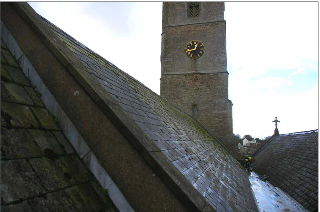
10. VIEW BACK ALONG THE VALLEY GUTTER AND TO THE TOWER, SHOWING HOW IT NARROWS AND HOW THE ROOFS ARE OFFSET; VIEWED FROM THE EAST-NORTH-EAST.
