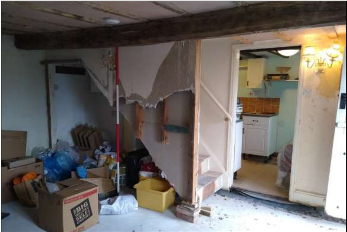
FIGURE 11: HONEY COTTAGE: GROUND FLOOR R1 & R2, LOOKING THROUGH DOORWAY TO R3; VIEW FROM SOUTH-WEST. ALL PARTITIONS ARE MODERN, IN POSITIONS OF LATER C19 ONES, BUT BEAM ABOVE IS C17. RECENT LIMECRETE FLOOR.
