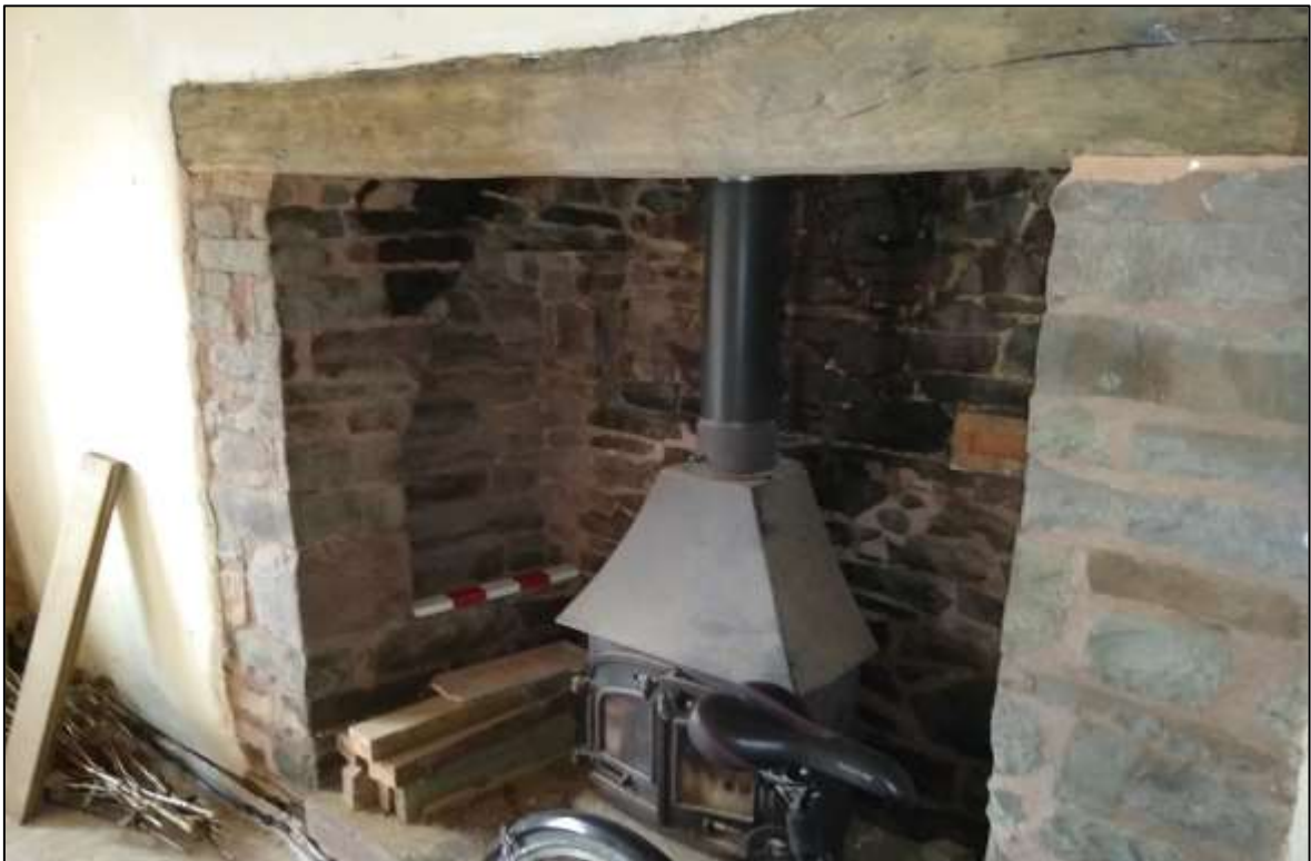
FIGURE 12: HONEY COTTAGE: C17 FIREPLACE IN GROUND FLOOR R2, FROM NORTH-EAST. 50CM SCALE BAR IS IN CORBELLED RECESS FOR C17 OVEN IN SOUTH JAMB; RECYCLED C17 CEILING BEAM REPLACED ORIGINAL LINTEL IN C19/C20.
