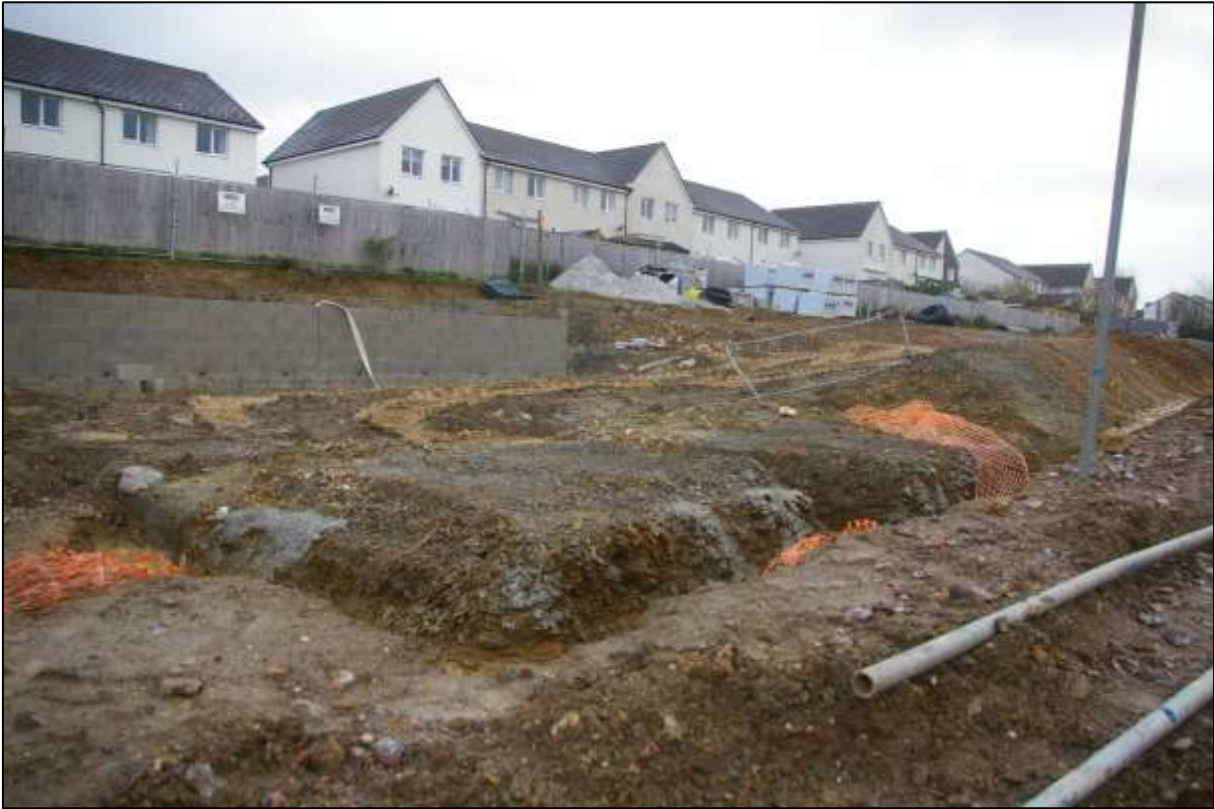
1. VIEWS ACROSS AREAS OF ALREADY EXCAVATED HOUSE PLOTS TOWARDS THE NORTH-WEST CORNER OF THE SITE; VIEWED FROM THE SOUTH-WEST.
