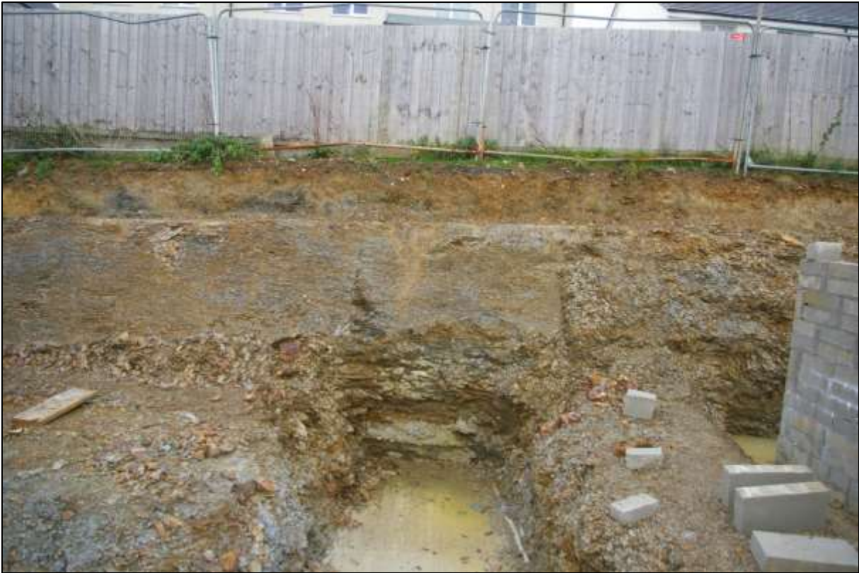
3. DETAIL OF EXCAVATED FOUNDATION TRENCHES DEMONSTRATING THIN LAYERS OF TOPSOIL AND SUBSOIL OVERLYING NATURAL BEDROCK; VIEWED FROM THE SOUTH.
