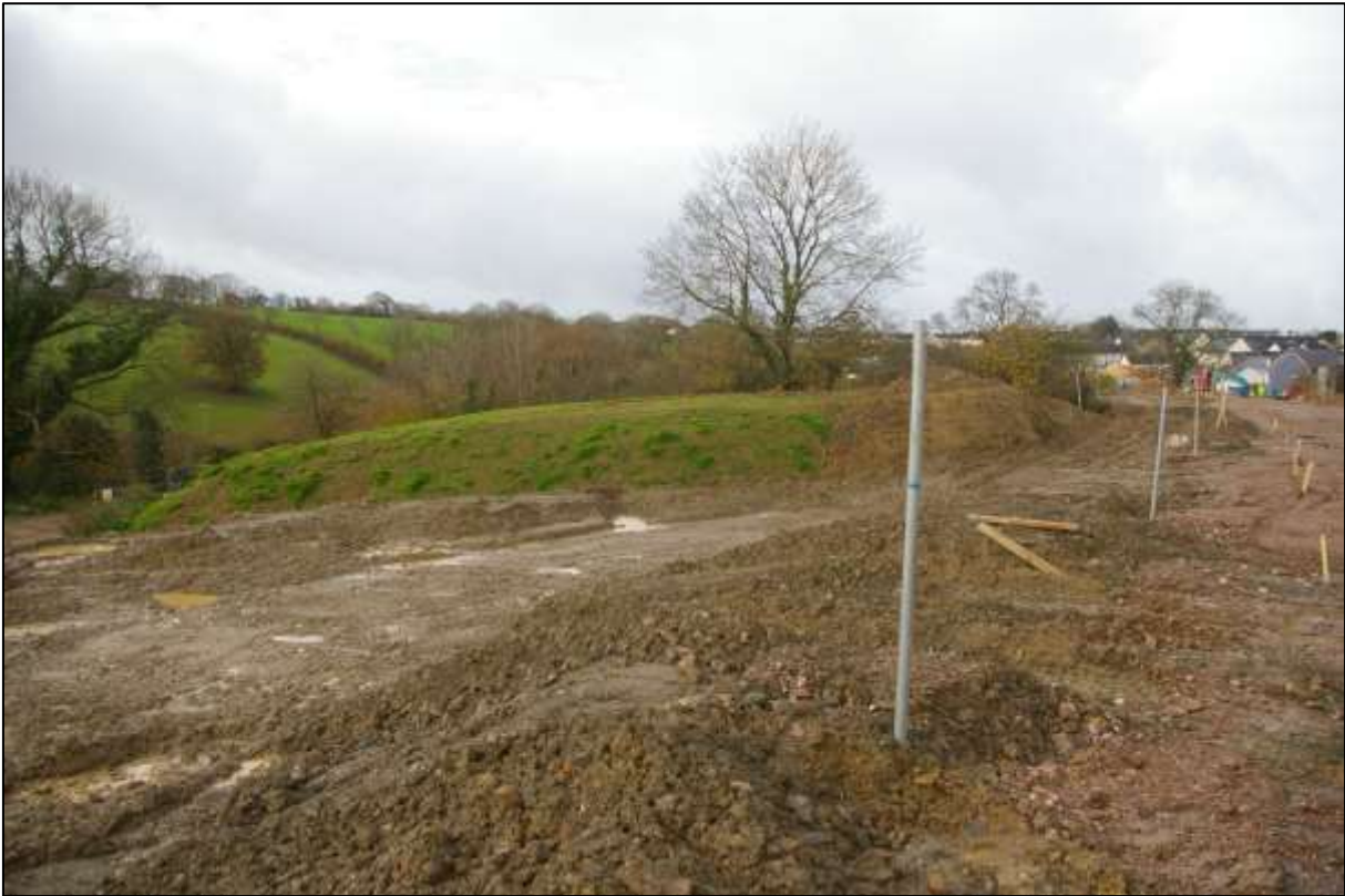
7. DETAIL OF ONE OF THE SPOIL STORAGE AREAS TO THE SOUTH OF THE ROAD STRIP; VIEWED FROM THE NORTH-EAST.
