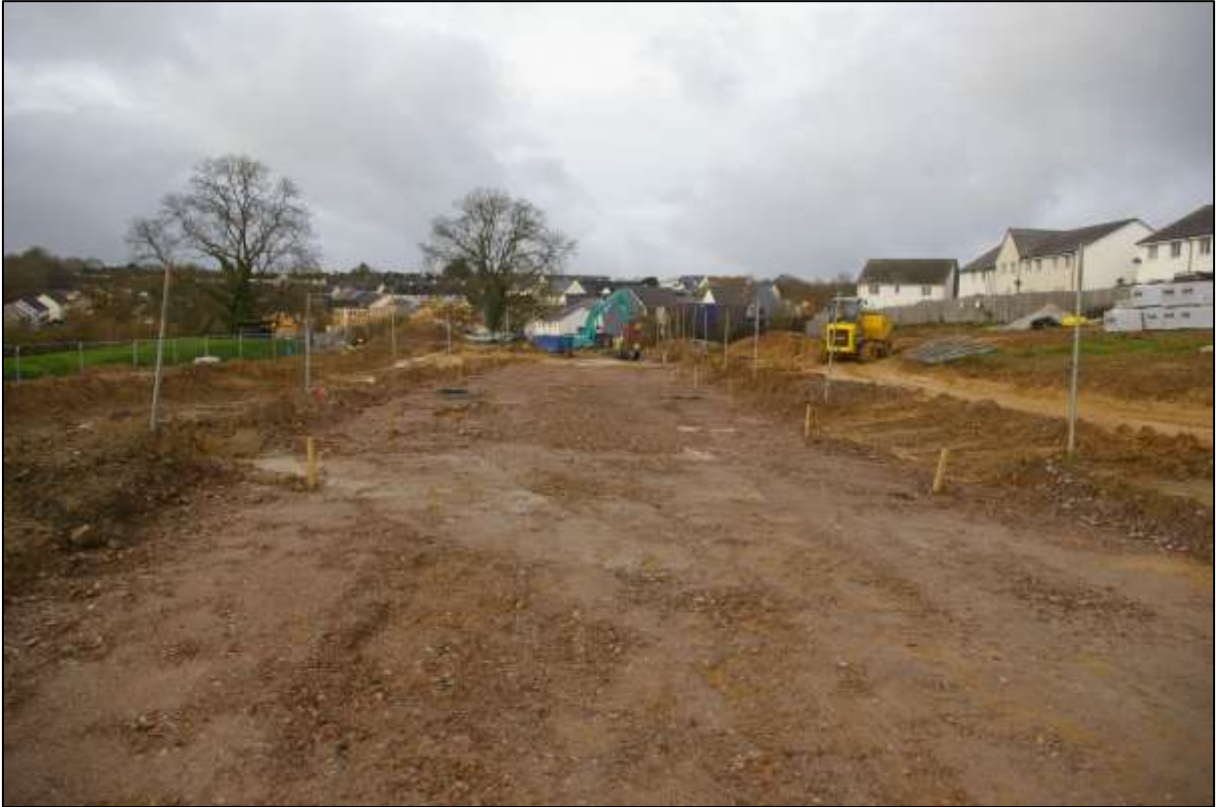
5. VIEW ALONG THE STRIPPED AND STONED ROAD TO THE SOUTH OF THE NORTHERN ROW OF HOUSING; VIEWED FROM THE EAST.
