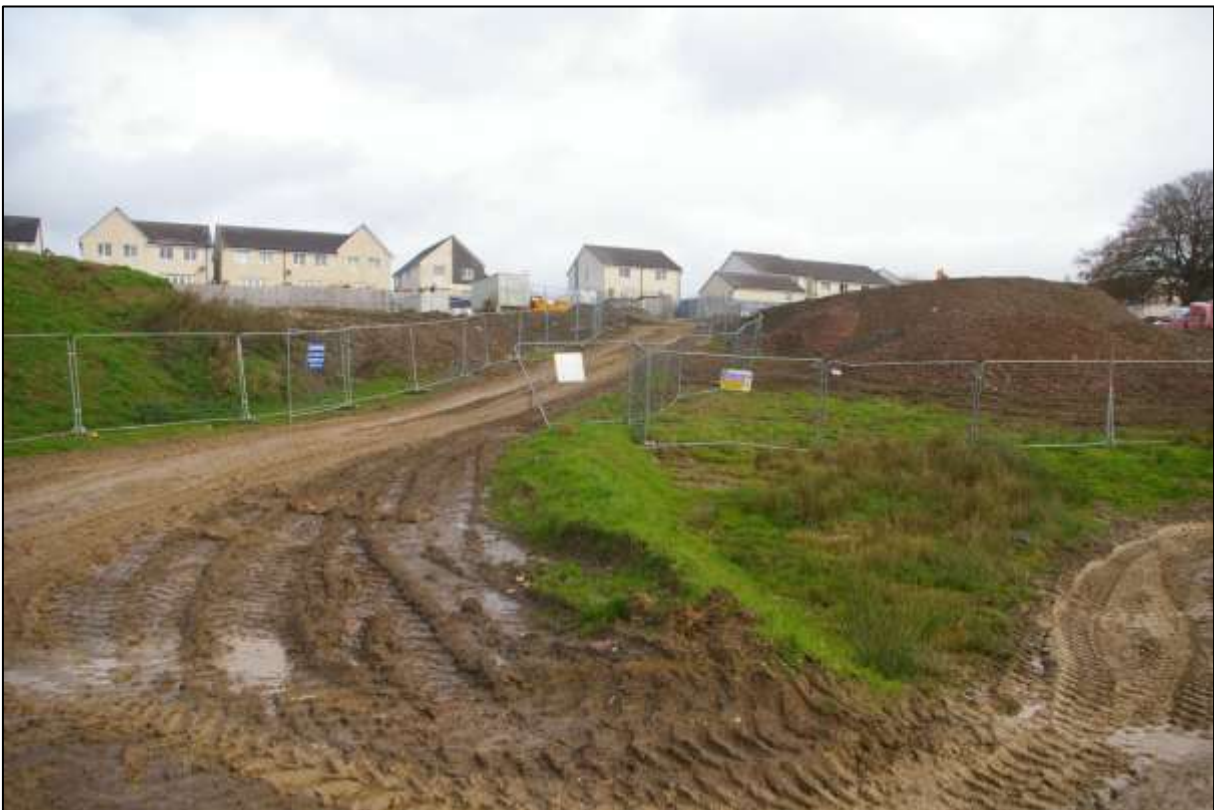
8. VIEW OF THE EASTERN END OF THE SITE WITH SPOIL STORAGE, FROM SOUTH OF THE SITE; VIEWED FROM THE WEST-SOUTH-WEST.
