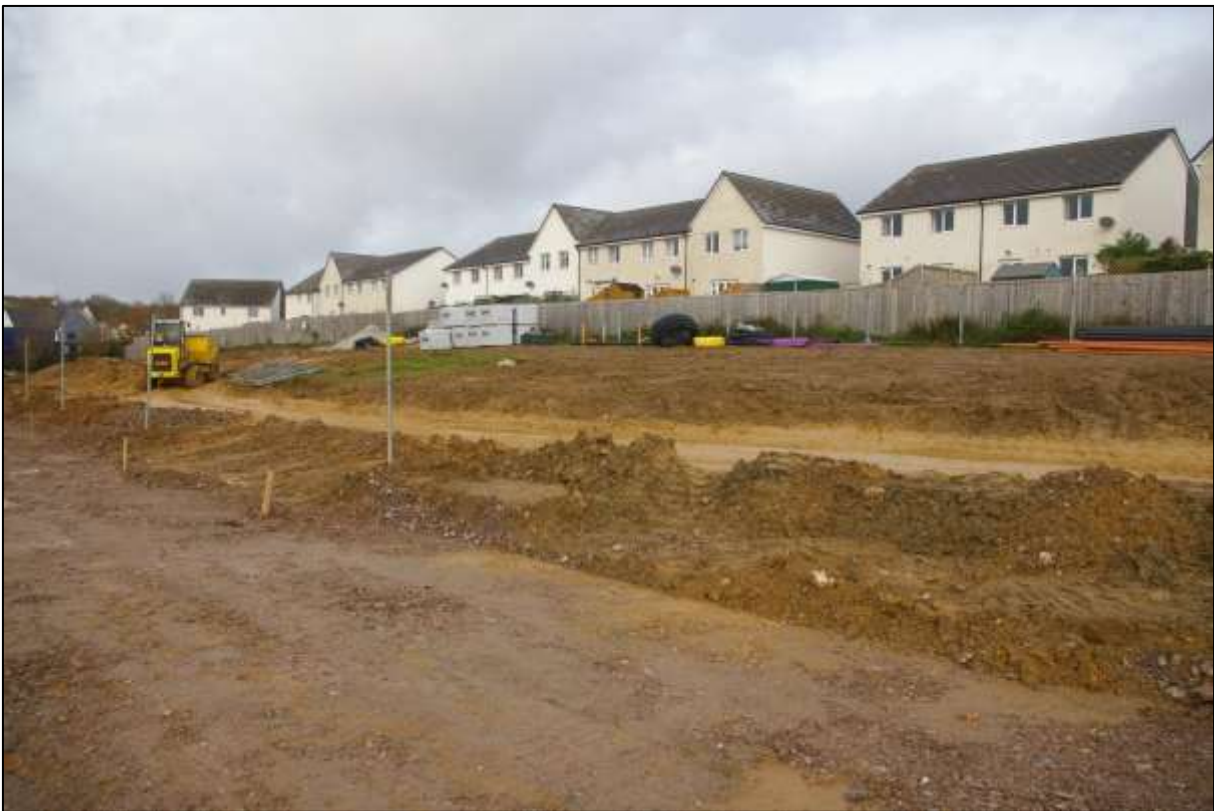
4. VIEW OF THE UN-STRIPPED AREA ALONG THE NORTHERN BOUNDARY OF THE SITE; VIEWED FROM THE SOUTH-EAST.
