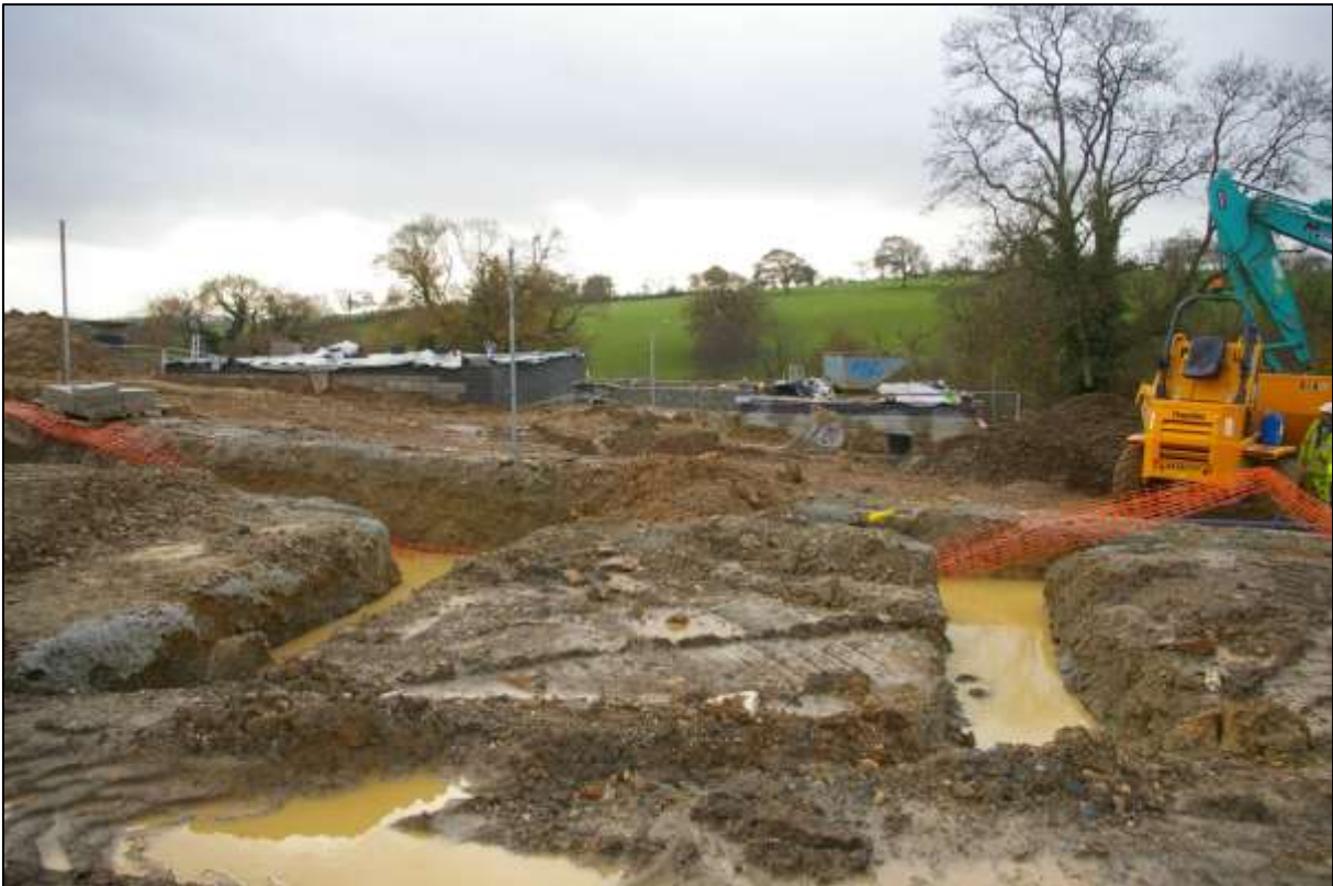
2. VIEW ACROSS AREAS OF ALREADY EXCAVATED HOUSE PLOTS AT THE WESTERN END OF THE SITE; VIEWED FROM THE NORTH.
