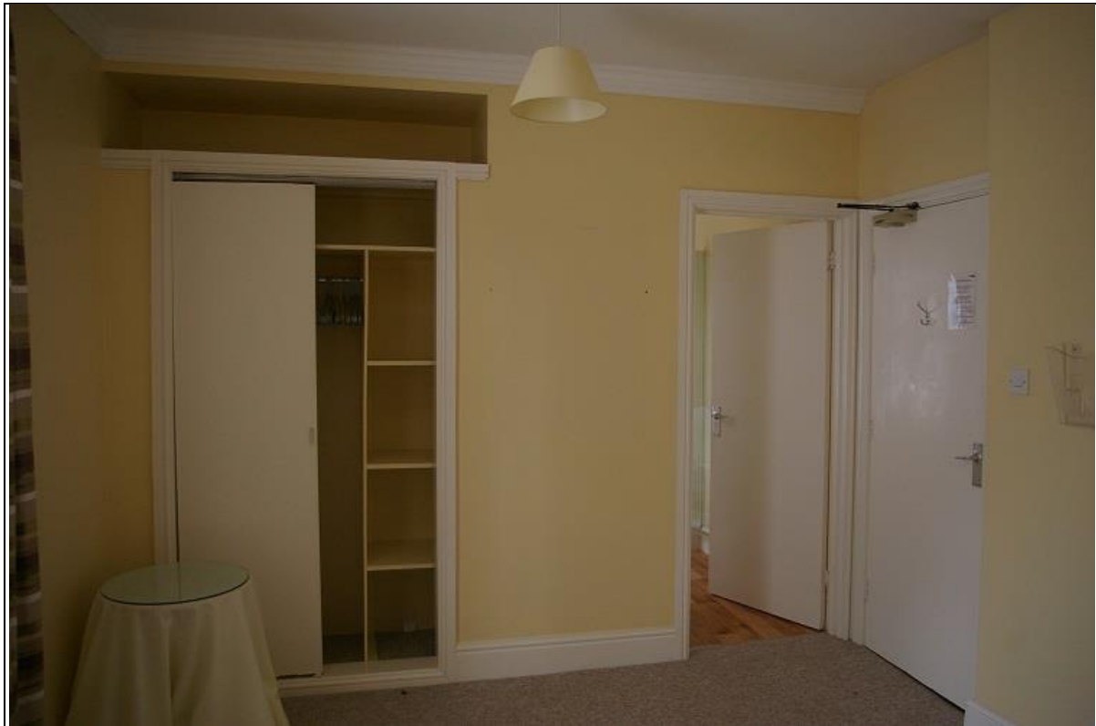
FIGURE 13: BEDROOM 32A, WITH SOME SURVIVING SKIRTING BOARDS AND PLASTER CORNICE, AS WELL AS REMAINS OF TRUNCATED WEST GABLE END STACK; FROM THE SOUTH-EAST.
