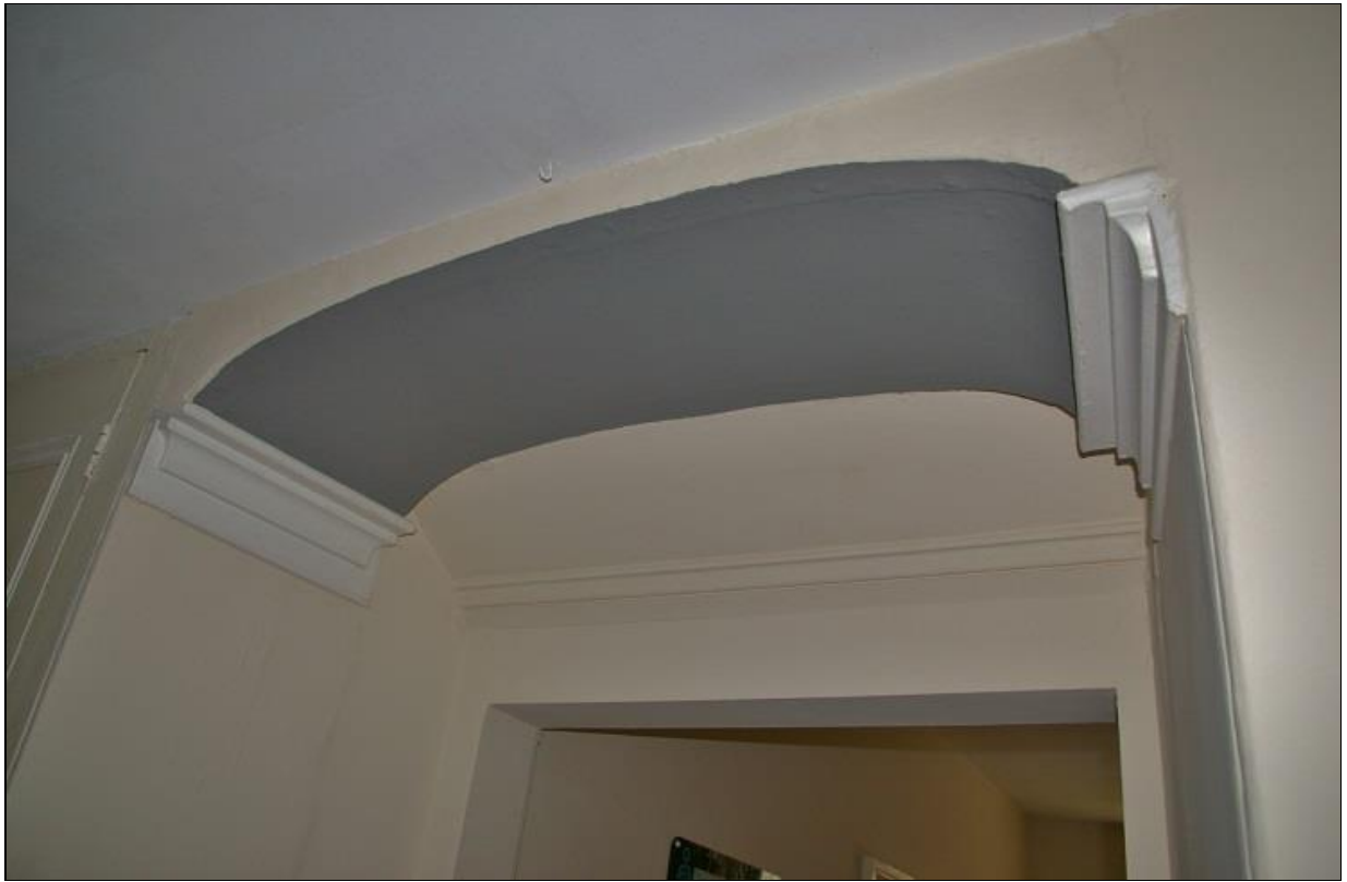
FIGURE 18: THE BASKET-ARCH SHAPED ARCHWAY BETWEEN THE ENTRANCE HALLWAY AND REAR CORRIDOR WITHIN THE PARALLEL RANGE; FROM THE WEST-NORTH-WEST.
