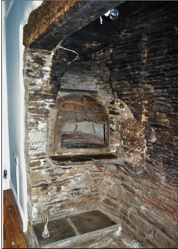
FIGURE 15: THE VICTORIAN CLOAM OVEN THAT HAS BEEN FORCED INTO THE SIDE OF THE 17 TH CENTURY STACK, REPLACING AN EARLIER OVEN; FROM THE NORTH-NORTH-EAST.
