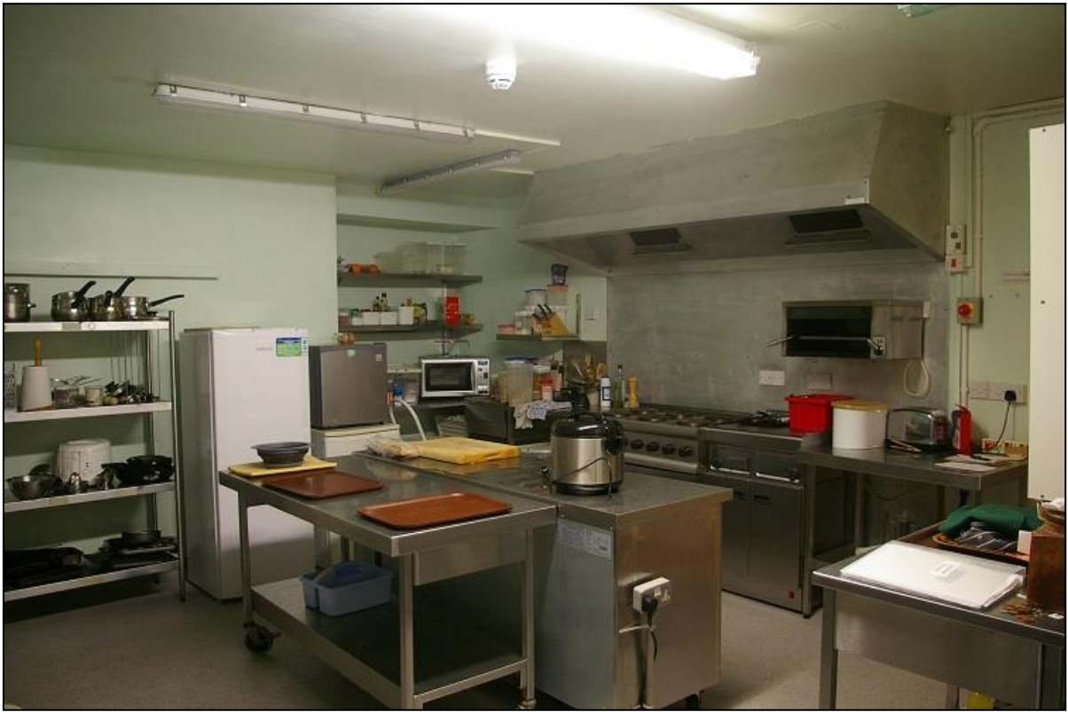
FIGURE 10: THE COMMERCIAL KITCHEN, R5, WITH VISIBLE BLOCKED WINDOW TO THE NORTH-WEST CORNER; FROM THE SOUTH-EAST.
