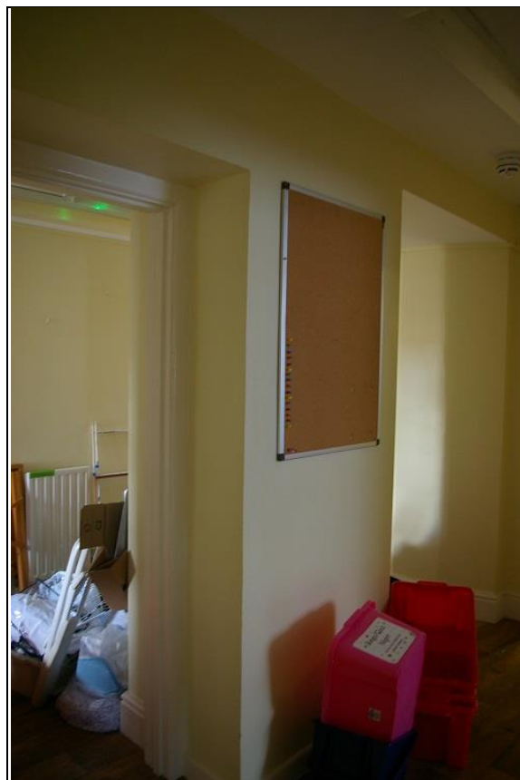
15. THE TWO DOORS OR DOOR AND WINDOW IN THE THICK FORMER WALL OF THE SERVICE WING, R14; FROM THE NORTH-WEST.
