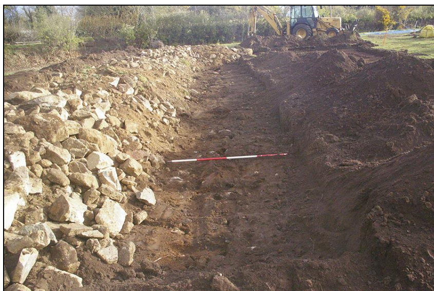
FIGURE 4: WEST SIDE OF THE EXCAVATED AREA FOR THE SWALE; VIEWED FROM THE SOUTH (2M SCALE).
