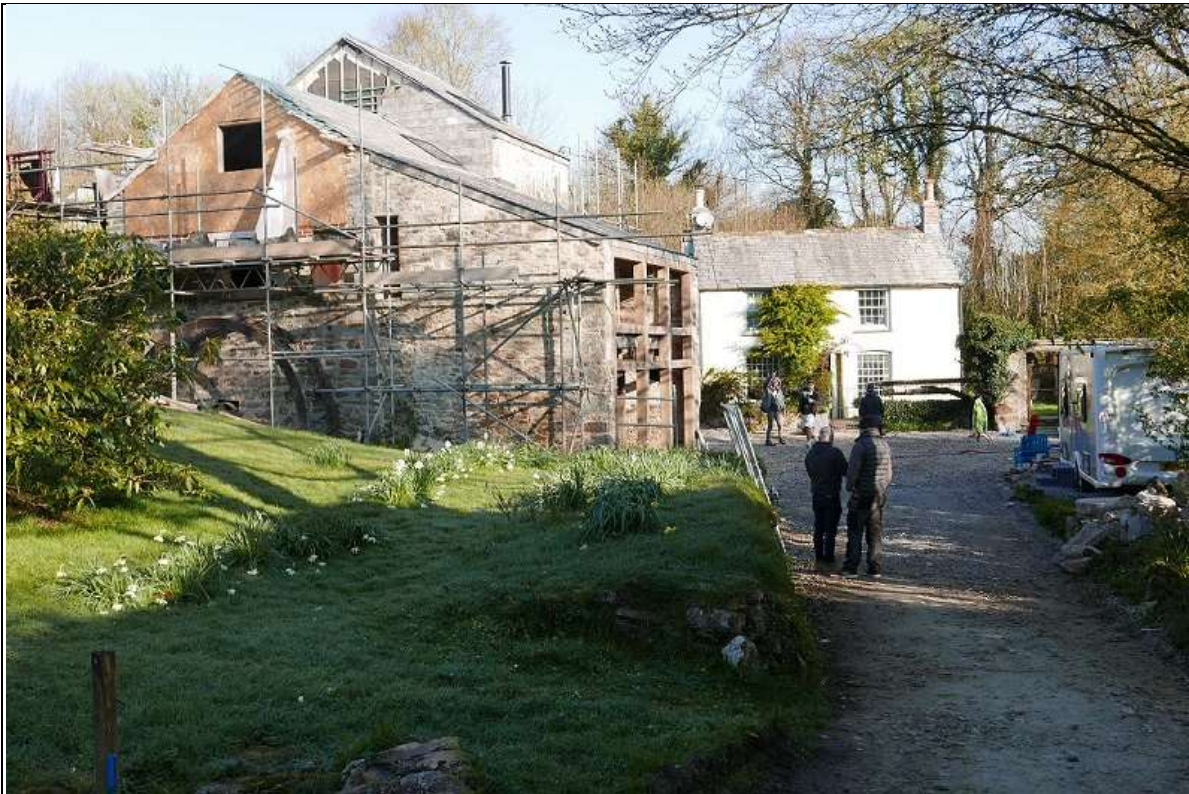
13. 2021 PHOTO OF THE WATERMILL BUILDING UNDER RENOVATION, WITH THE HOUSE BEHIND; FROM THE
