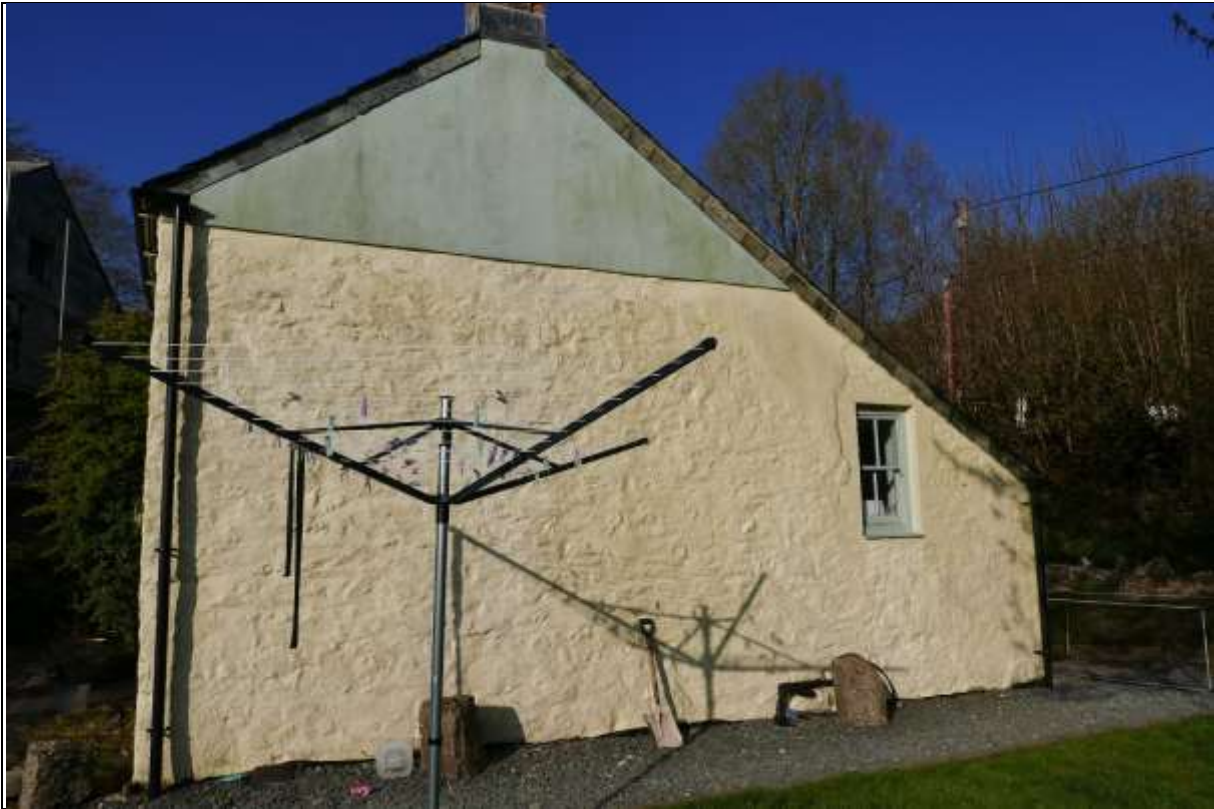
15. THE ..... ELEVATION, WHICH WILL BE ABUTTED BY THE EXTENSION, WITH A DOOR FORCED THORUGH TO CONNECT; FROM THE
