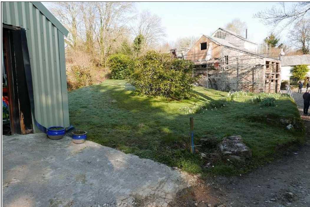
20. THE MILL BUILDING UNDER RENOVATION AND THE CURRENT AGRICULTURAL SHED; FROM THE SOUTH-EAST.
