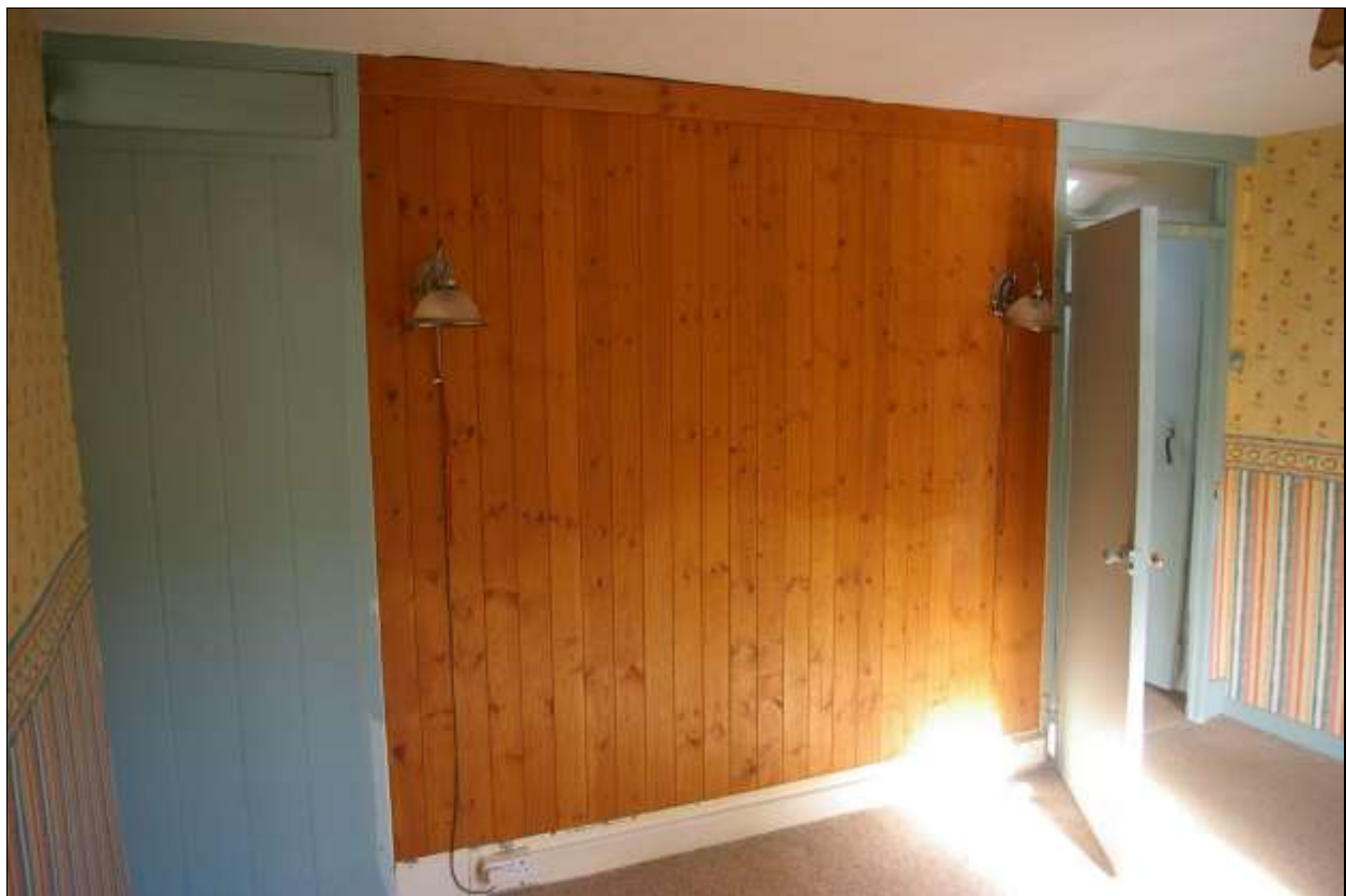
9. THE EASTERN BEDROOM, SHOWING REMOVAL OF A DIVIDING PARTITION WALL; FROM THE SOUTH-WEST.
