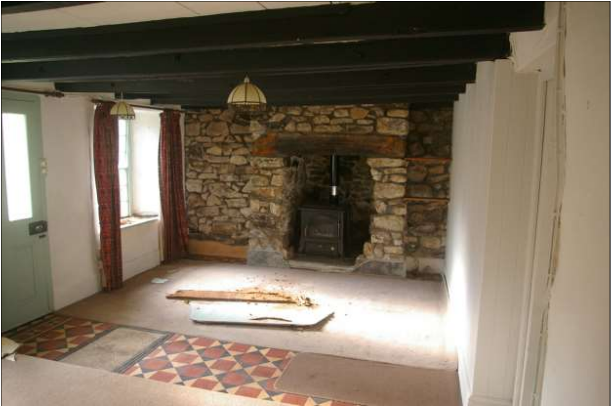
3. THE MAIN GROUND FLOOR SPACE IN THE MILL HOUSE, OPENED UP FROM TWO SEPARATE ROOMS; FROM THE EAST-NORTH-EAST.
